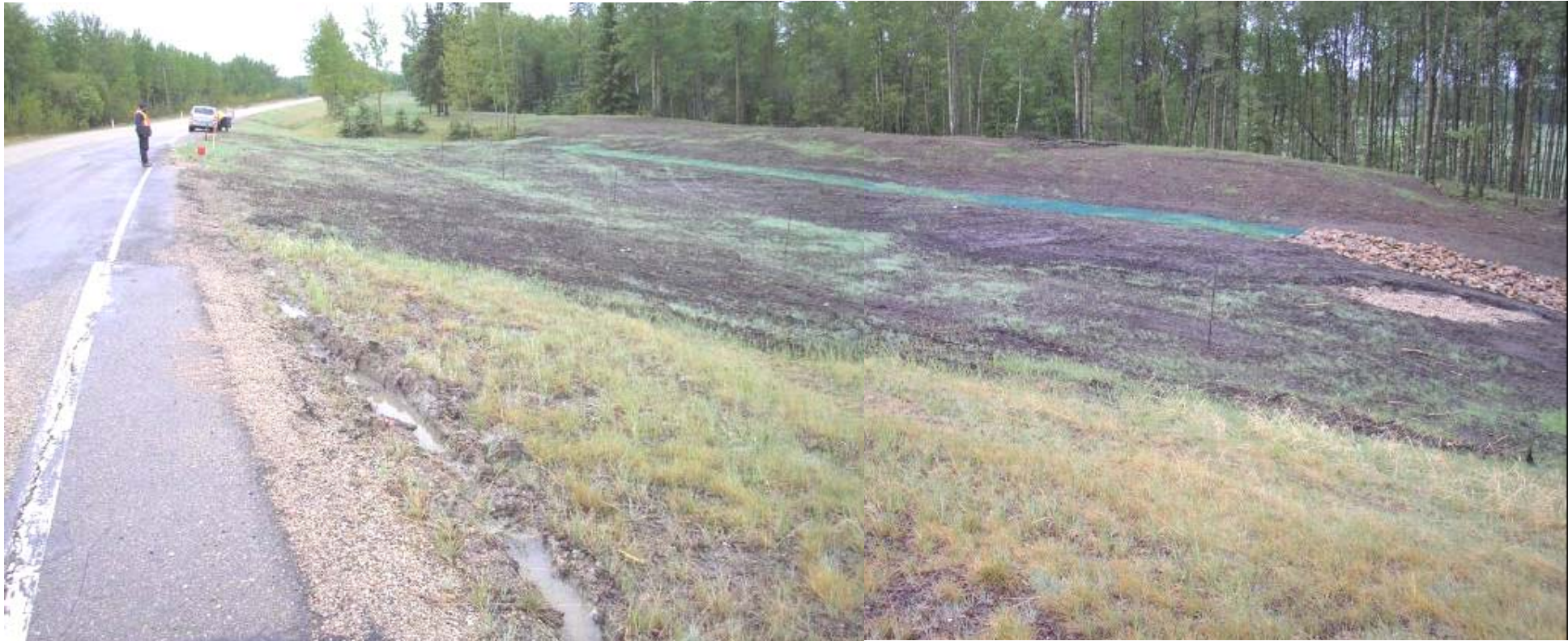
Photo 1 - Panoramic view of the Banana Belt Slide Area, May 24, 2006.
