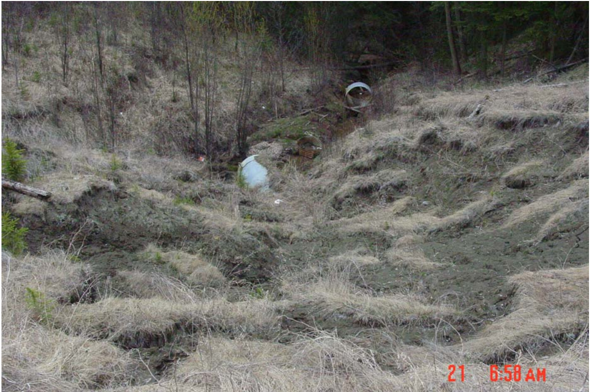
Photo 5: View of slope failure at culvert outlet location looking north.
