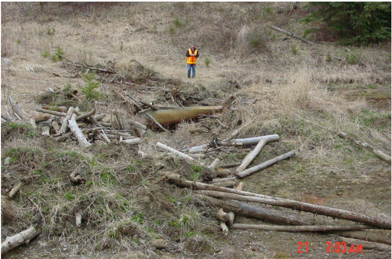
Photo 2: Damaged culvert inlet tilted upwards, looking east.
