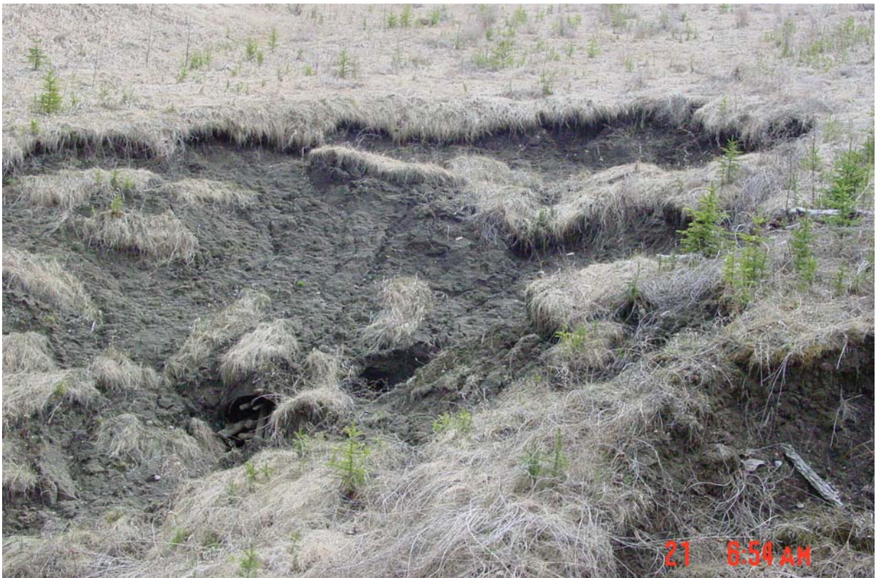
Photo 8: View of backscarp and clogged pipe above the culvert outlet location, looking northwest.
