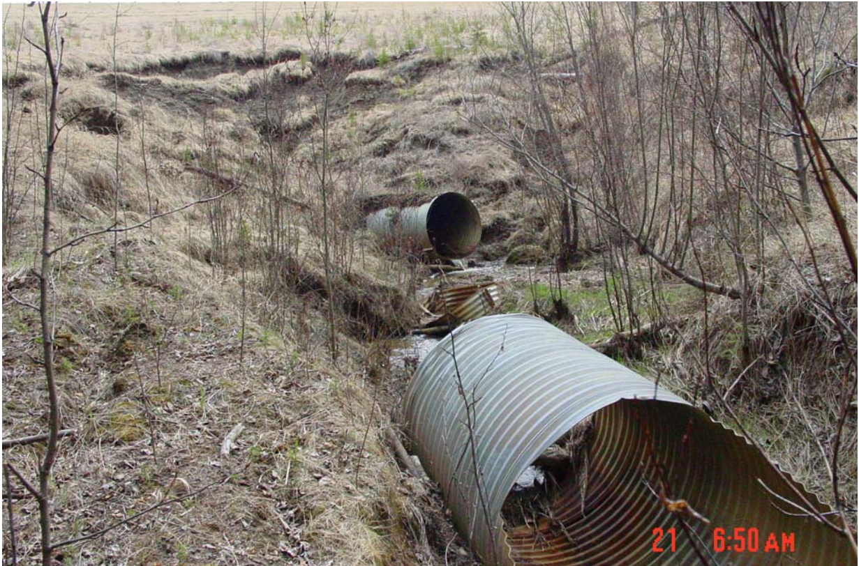
Photo 7: Pipe destroyed at culvert outlet location, looking south.
