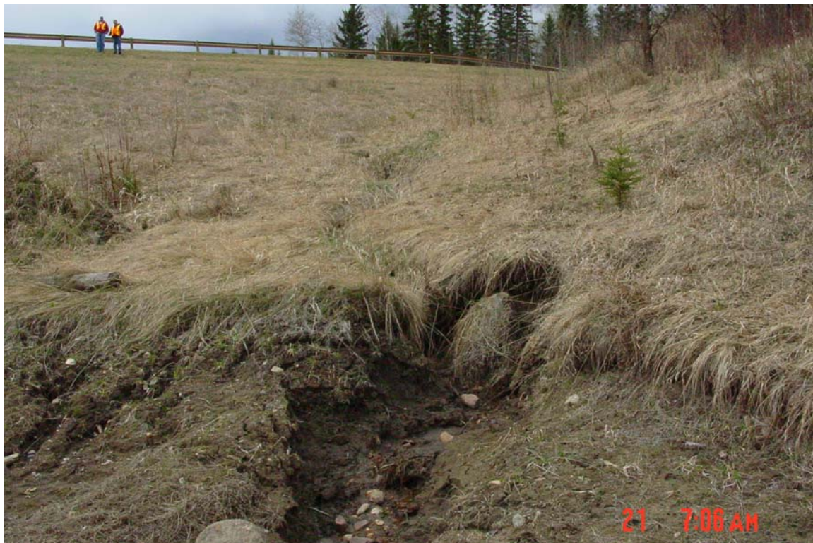
Photo 4: Erosion rill extending from highway, east of culvert inlet, looking northeast.
