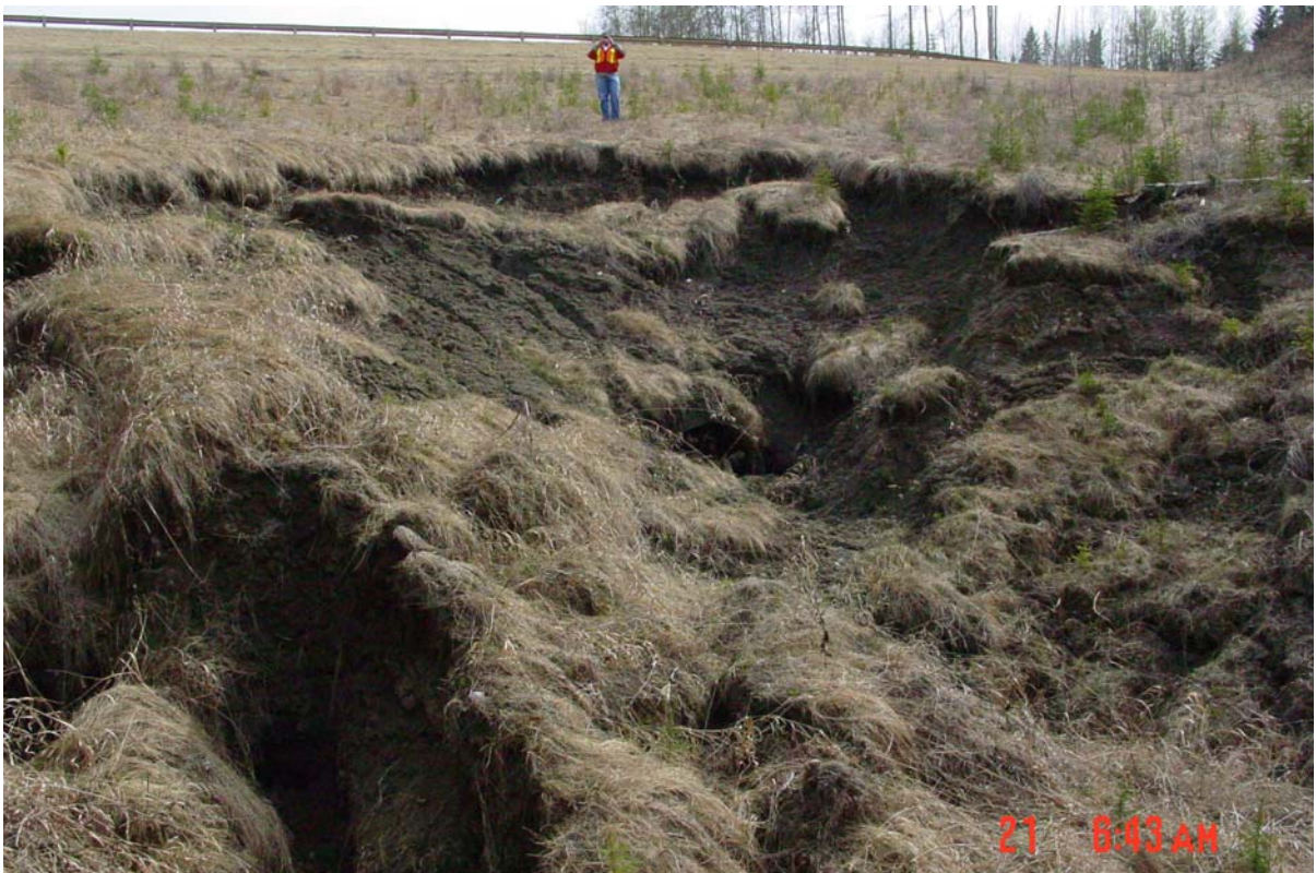
Photo 6: View of pipe severed by slope failure a few meters above the culvert outlet location, looking south.
