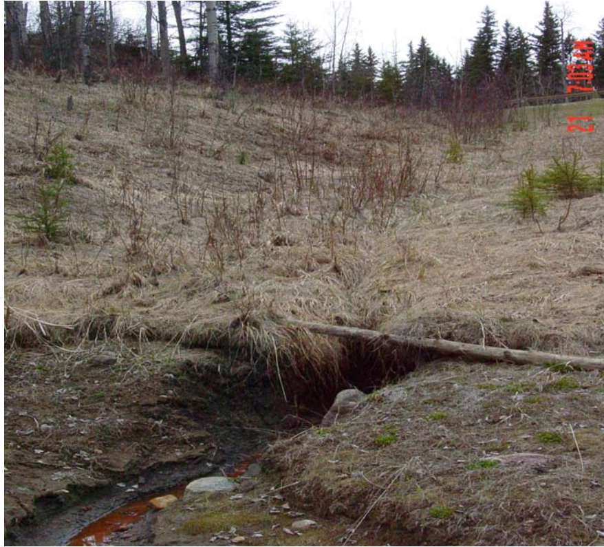
Photo 3: Erosion rill extending from highway, west of culvert inlet, looking northwest.
