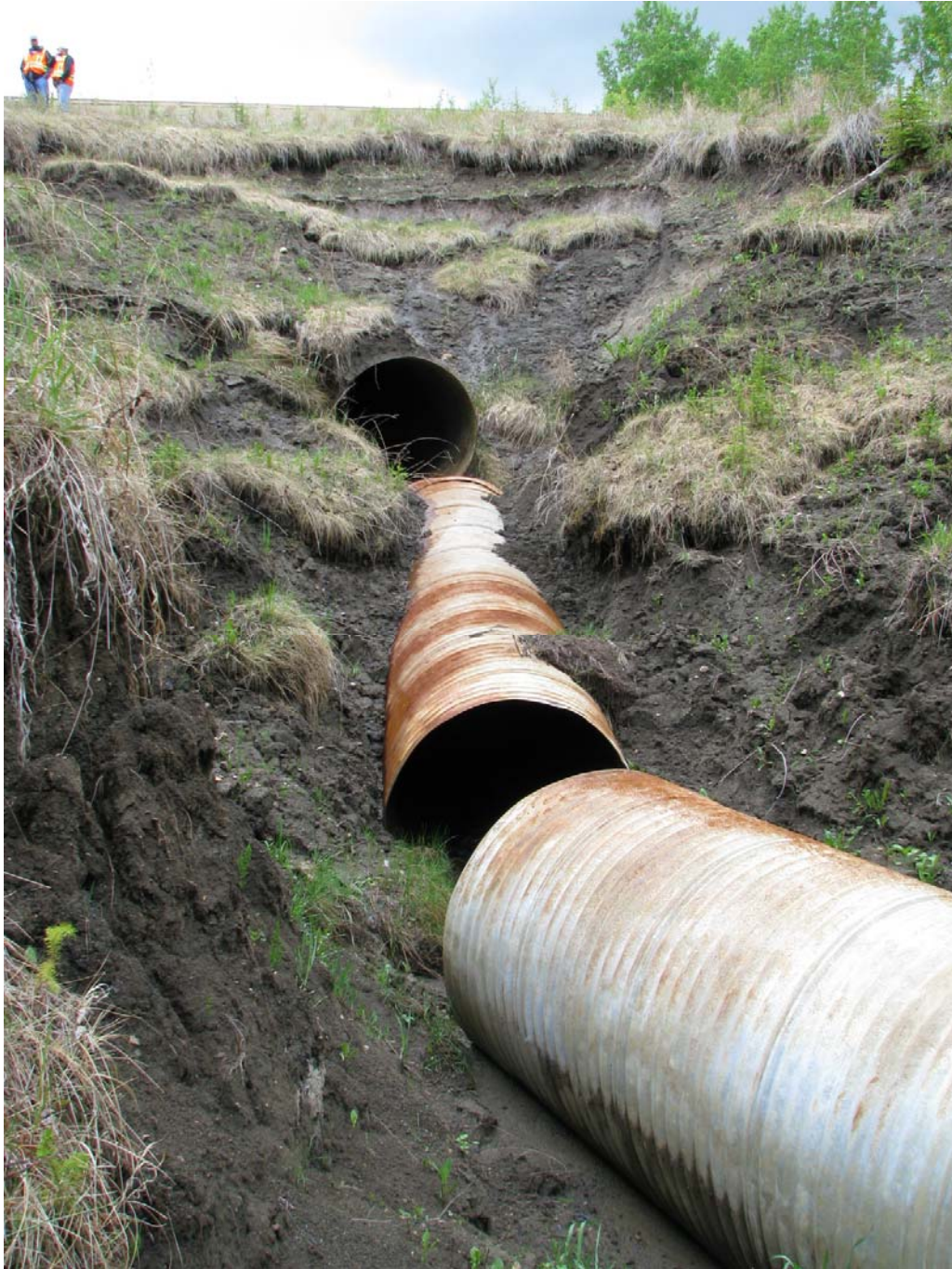
Photo 7: Pipe destroyed at culvert outlet location, looking upslope.
