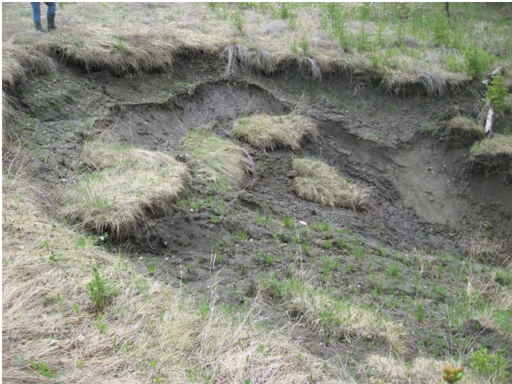
Photo 6: Increased backscarp retrogression at culvert outlet, looking west.
