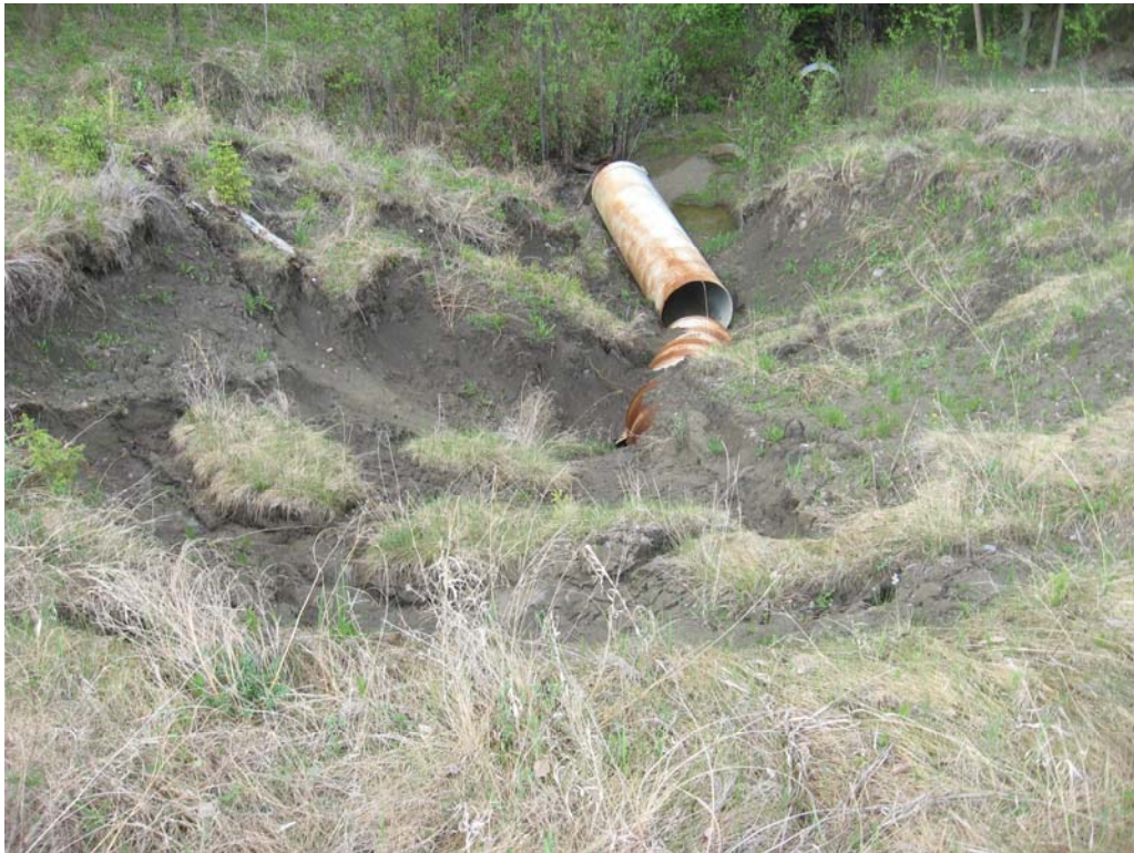
Photo 4: Broken culvert and increased slope movement at the outlet, looking north.
