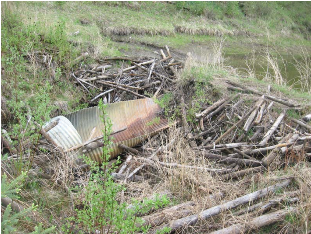
Photo 2: View of beaver dam and culvert inlet, broken and tilted upwards, looking east.
