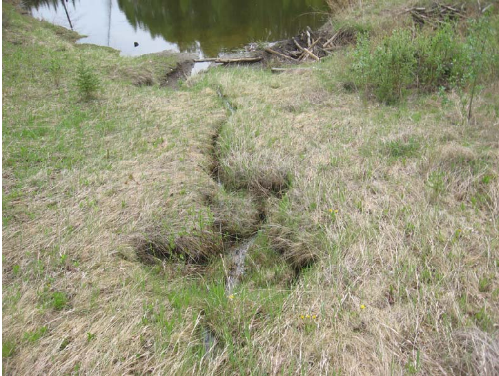
Photo 3: Increased erosion in rill located east of culvert inlet.
