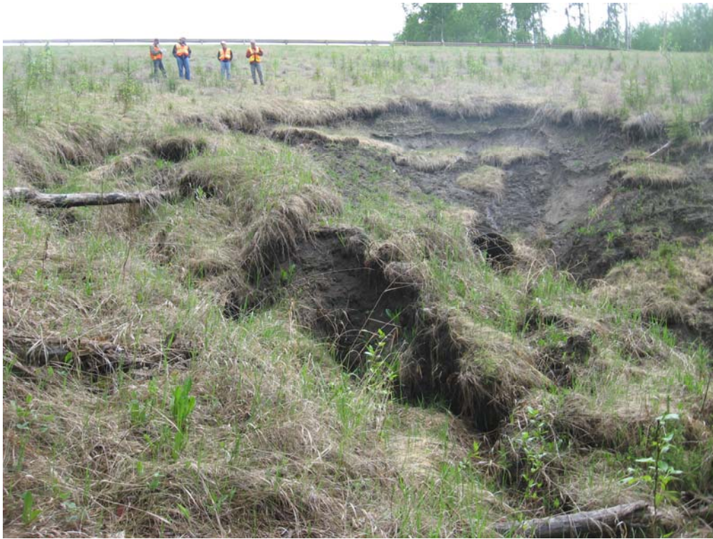
Photo 5: View of slope failure and broken culvert outlet, looking upslope.
