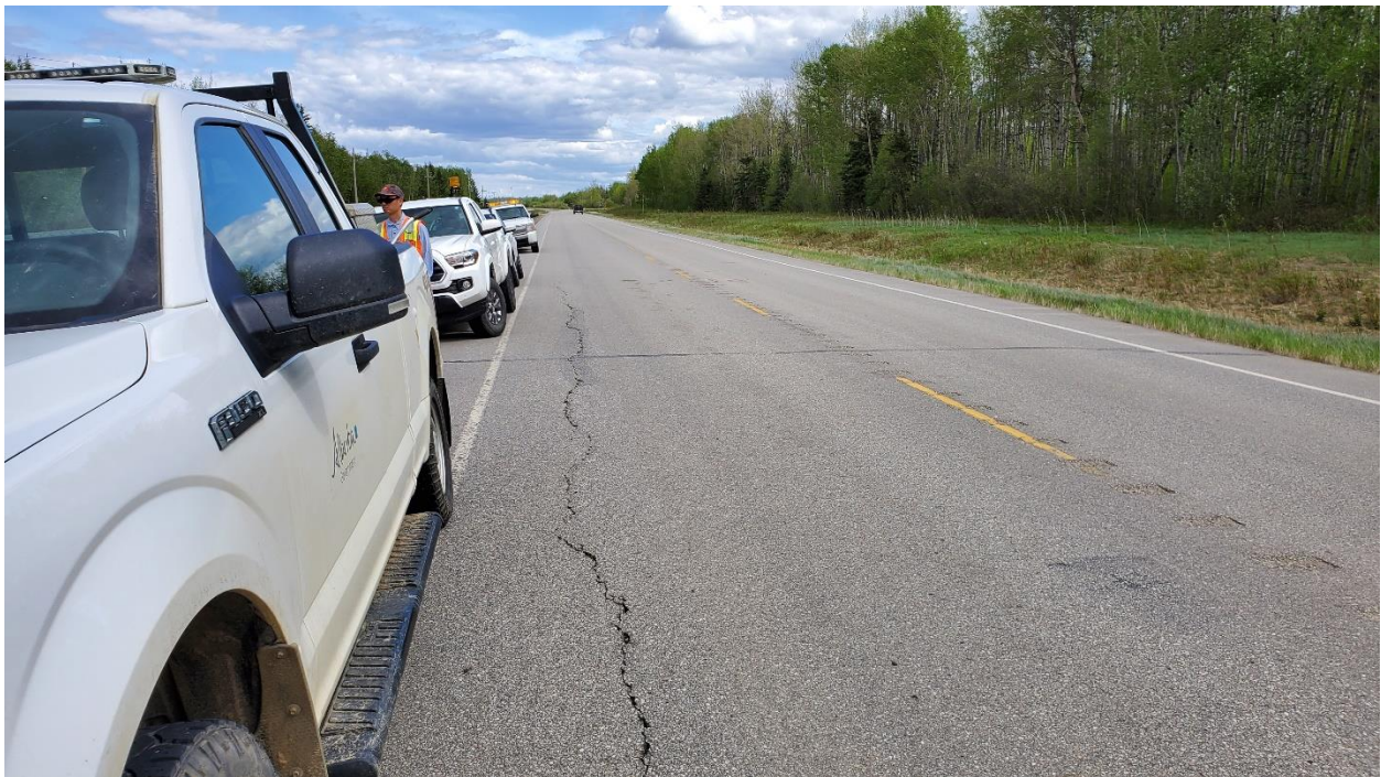
Photo 4 – Looking west at developing extension of the crack.
