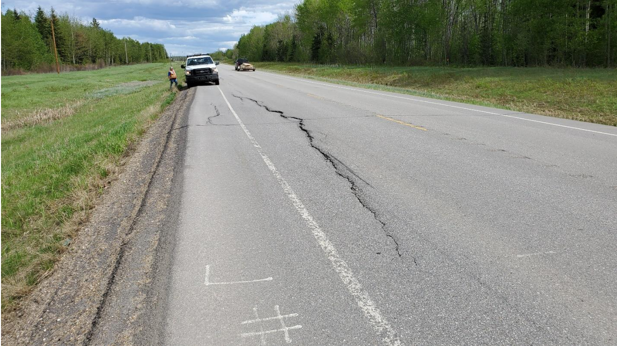
Photo 1 – Looking west along the EBL at the main crack and dip (at the fog line).
