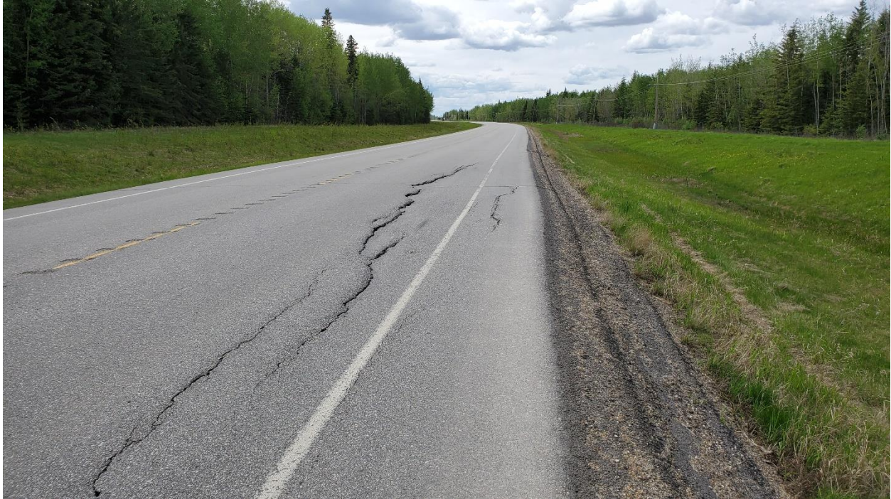
Photo 3 – Looking east at the main area of distress.
