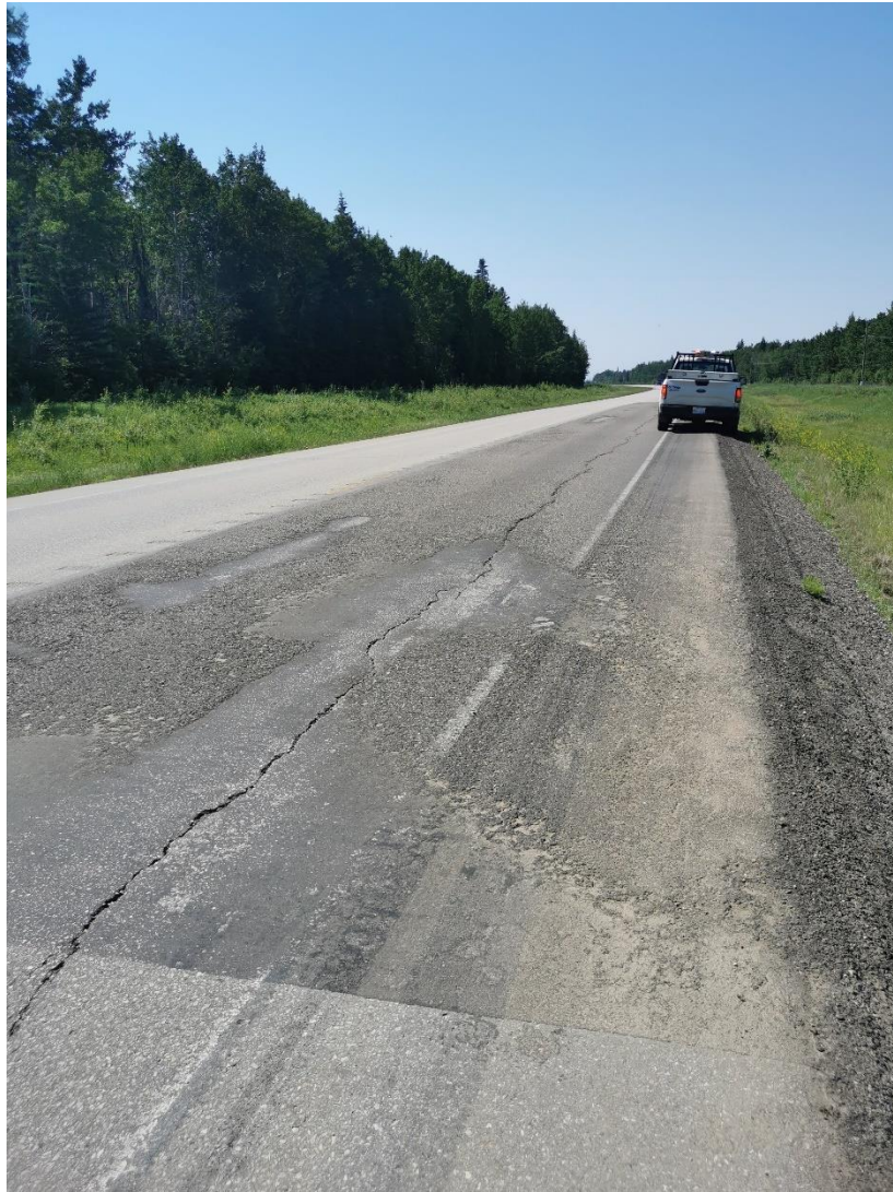
Photo 3 – Looking west at the main area of distress. Note the crack at bottom of photo extending past the patched area
