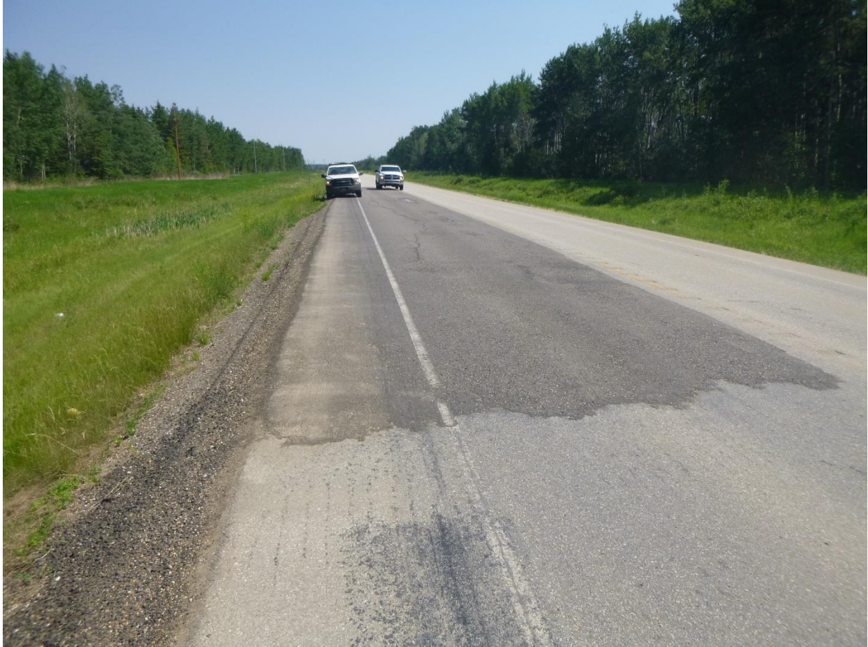
Photo 2 – Looking east at the sideslope below the main crack where there may be a toe roll in the ditch.
