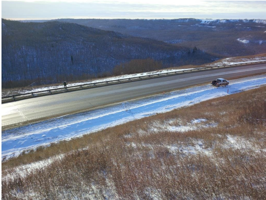
Photo 1 – Looking southwest at section of highway that is affected by landslide (Jan. 28, 2015)
