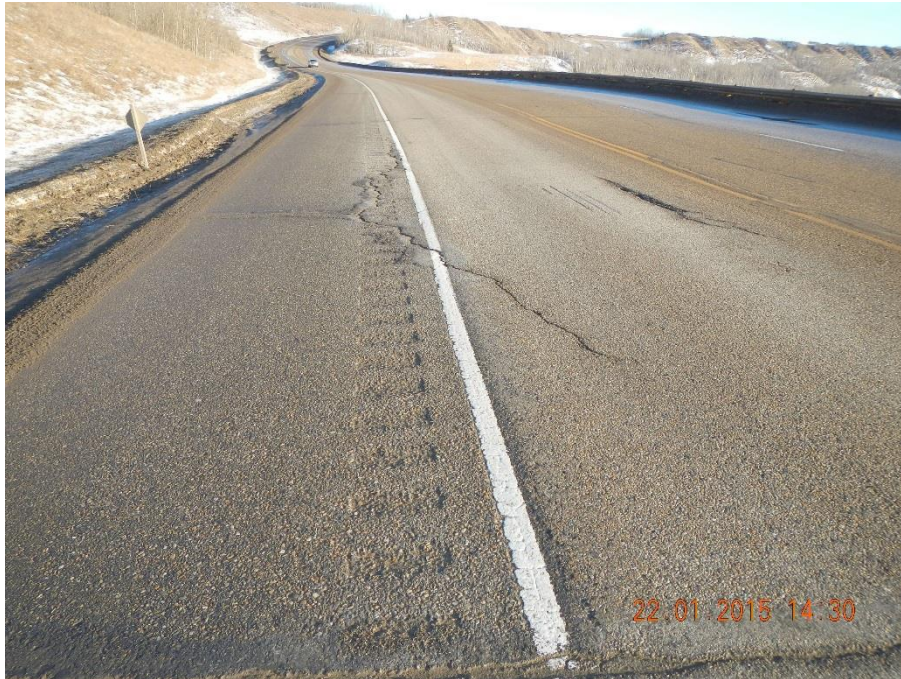
Photo 3 – Looking east at dip and tension cracks near headscarp of landslide (Jan. 22, 2015)
