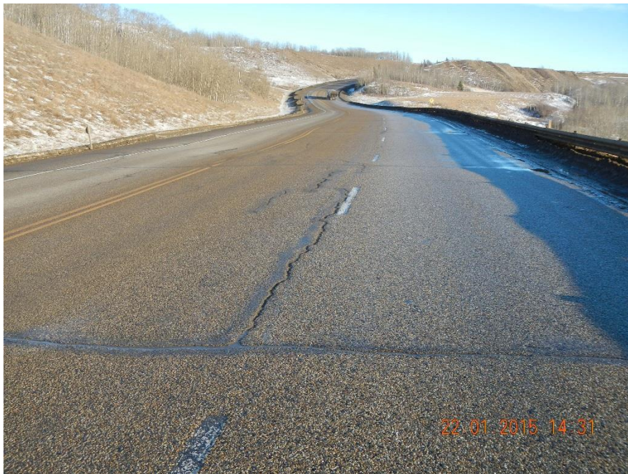
Photo 4 – Looking east at cracks propagating in EB lanes, from original landslide area. Water is ponding in dipped areas. (January 22, 2015)
