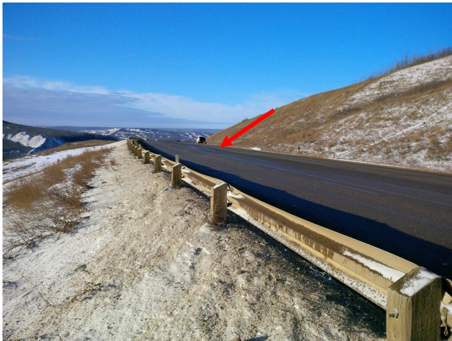
Photo 2 – Looking west at sideslope area between highway and valley slope and the main dip the roadway (January 28, 2015)
