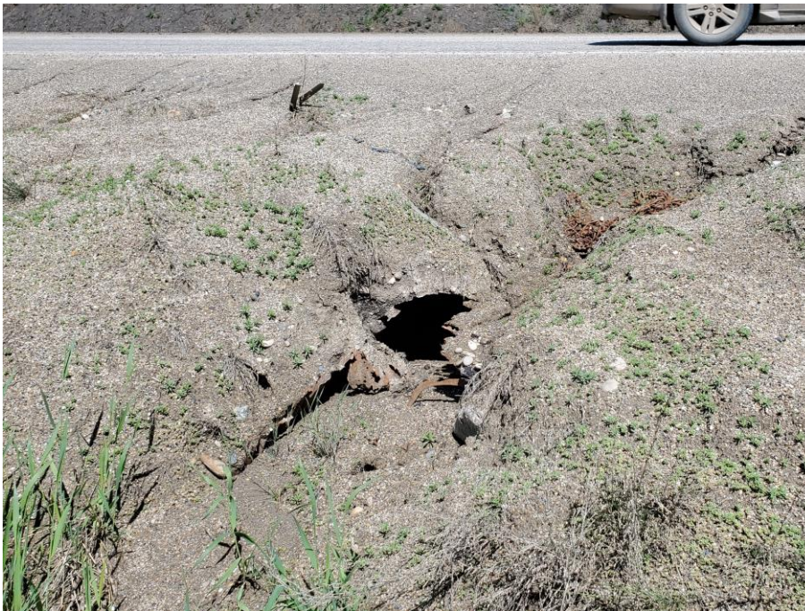
Photo 59-04. Looking at damaged culvert outlet (35+100).
