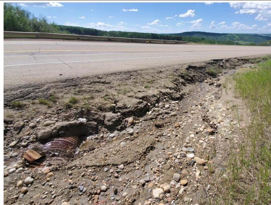
Photo 59-06. Buried and blocked culvert inlet near 35+475. Significant north ditch erosion upslope and downslope of inlet (up to 1.5 m deep).
