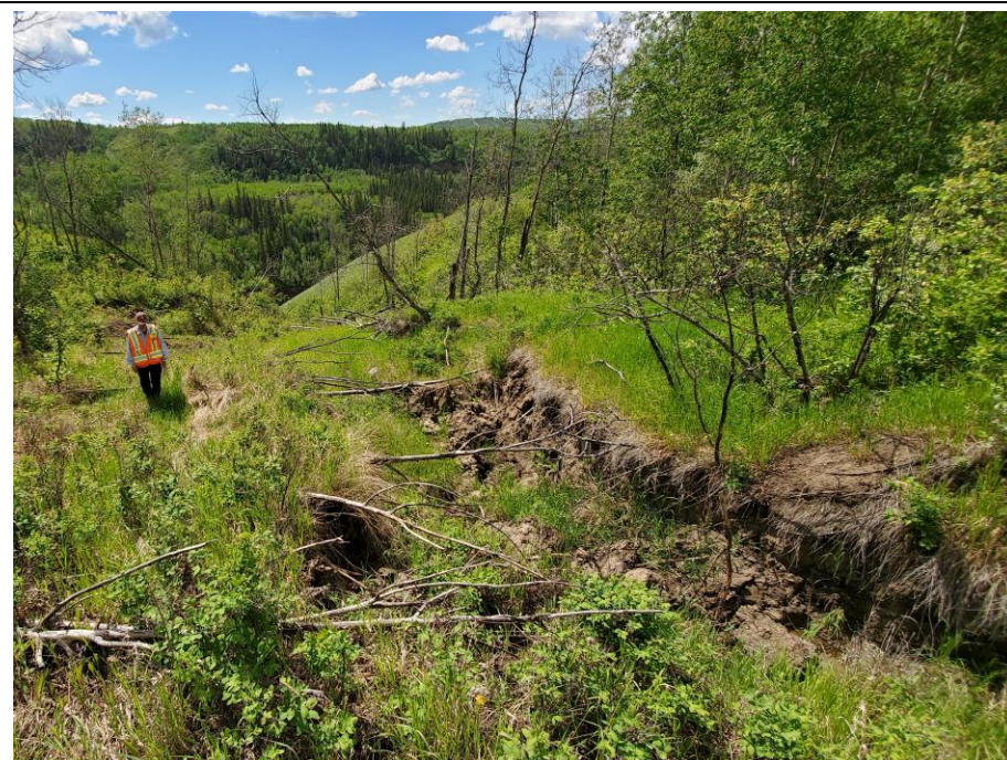
Photo 59-08. Overgrown erosion gully downstream of gabion culvert outlet near (35+500). Minor ongoing erosion/expansion at the flanks but no major retrogression since previous inspection.
