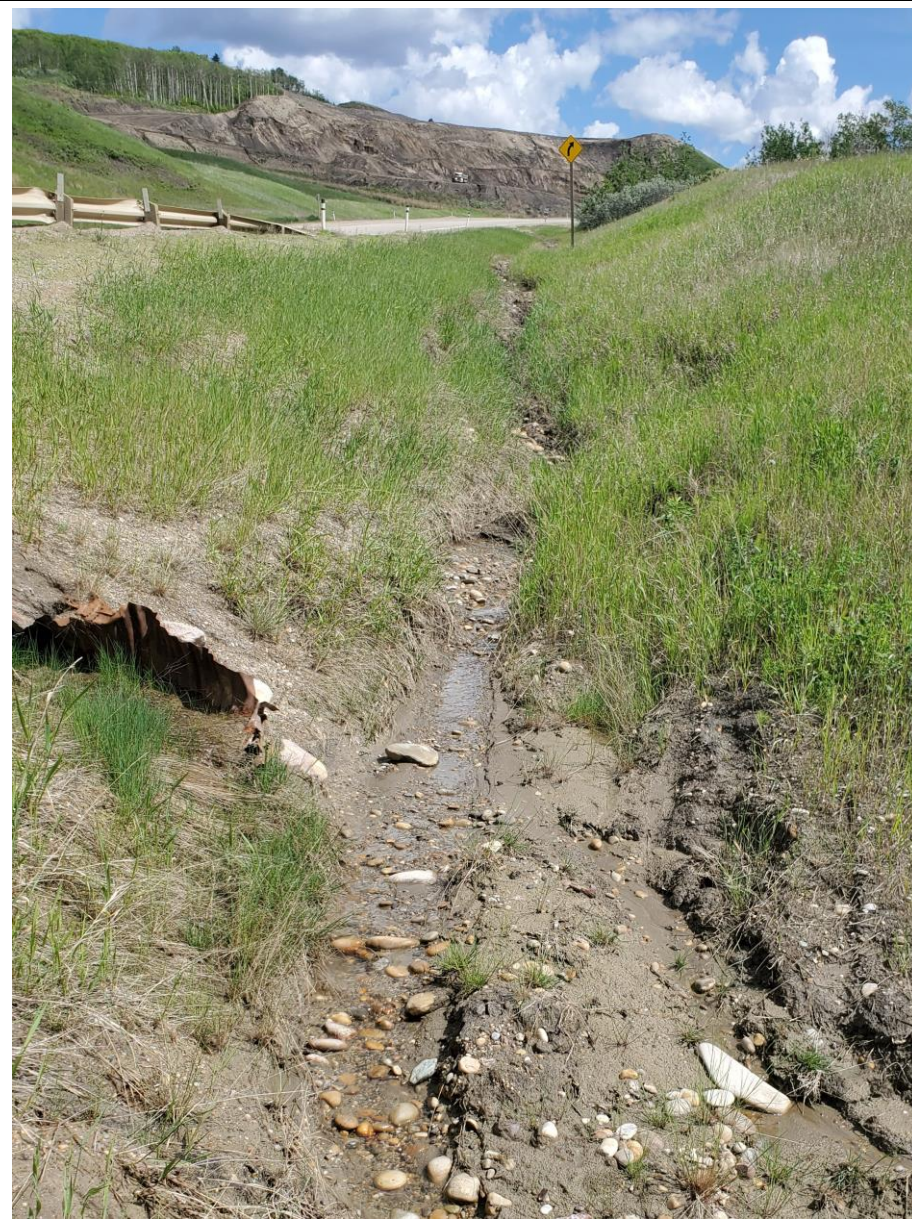
Photo 59-09. Looking east towards the south ditch erosion upslope from the culvert outlet that drains towards the river (35+500). No significant change from 2019.
