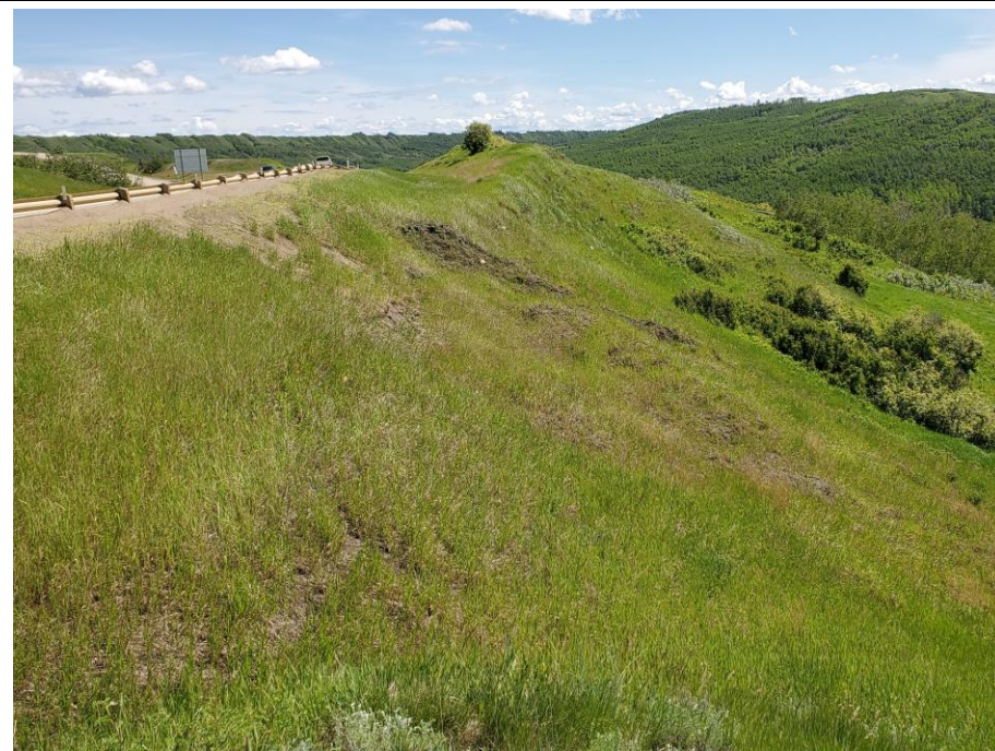
Photo 59-01. Looking east at headscarp area of shallow landslide on downslope side of roadway. Small downslope movement within displaced slide mass but no major expansion at the main scarp since 2009 (34+850).
