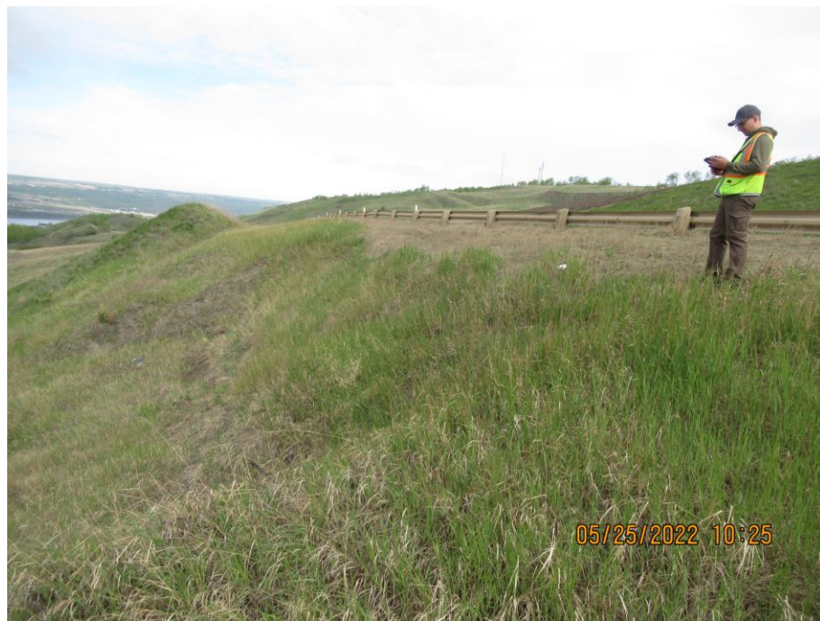
Photo 59-01. Looking east at headscarp area of shallow landslide on downslope side of roadway. Some downslope movement within displaced slide mass but no major expansion at the main scarp since 2009 (34+850).
