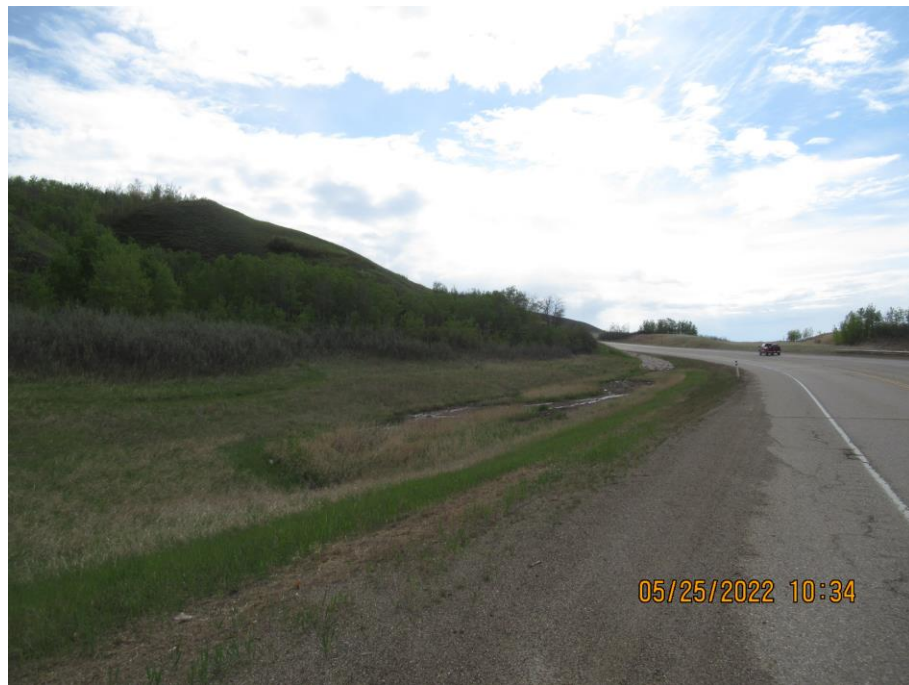
Photo 59-02. Look east at ditch erosion near the west end of the new ditch armoring before the culvert inlet (35+650).
