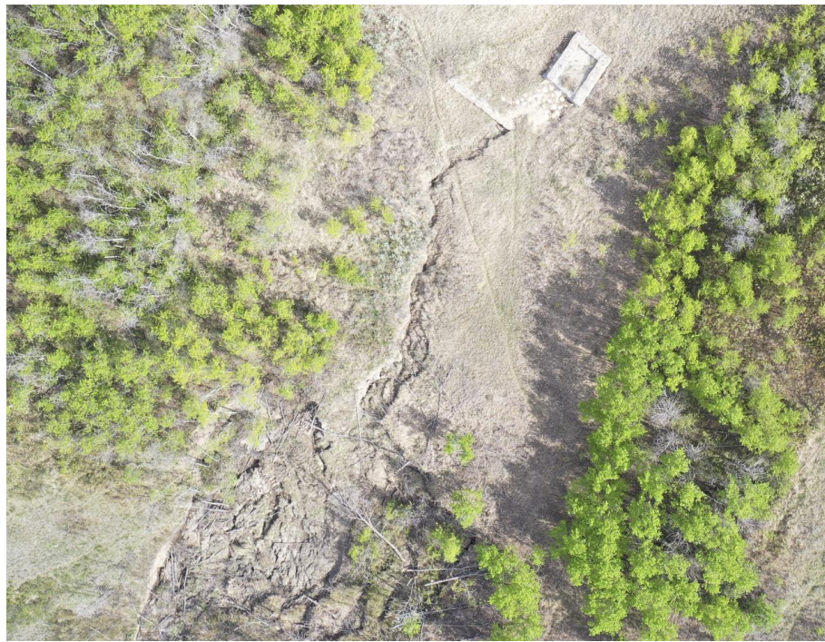
Photo 59-03. Overhead drone image of erosion and slide damage downslope from the gabion culvert outlet structure (35+500).
