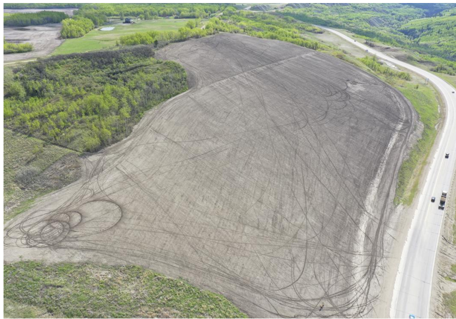
Photo 59-04. Oblique drone view towards the east of the graded borrow area above the highway (35+200). Minor rill erosion was noted.
