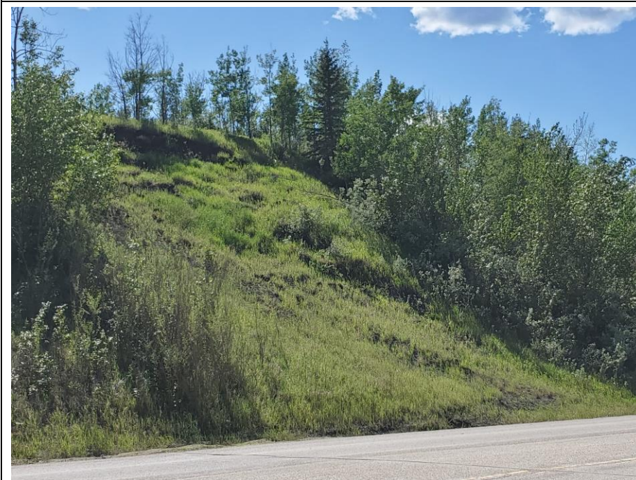
Photo 60-05. Shallow slide/flow within through-cut area on the south cut slope (35+830). First observed in 2016, no further expansion or blocking of ditch.
