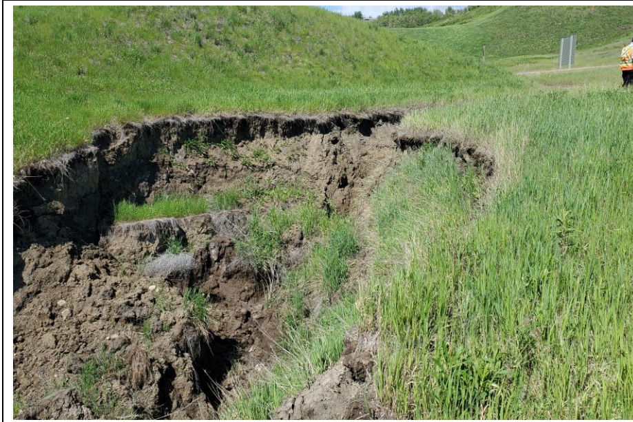
Photo 60-06. Headcutting and erosional gully occurring below roadway (36+050).
