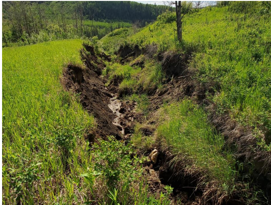
Photo 60-02. Looking downslope at erosional gulying below culvert shown in Photo 60-01 (35+700). Active slumping on gully walls.
