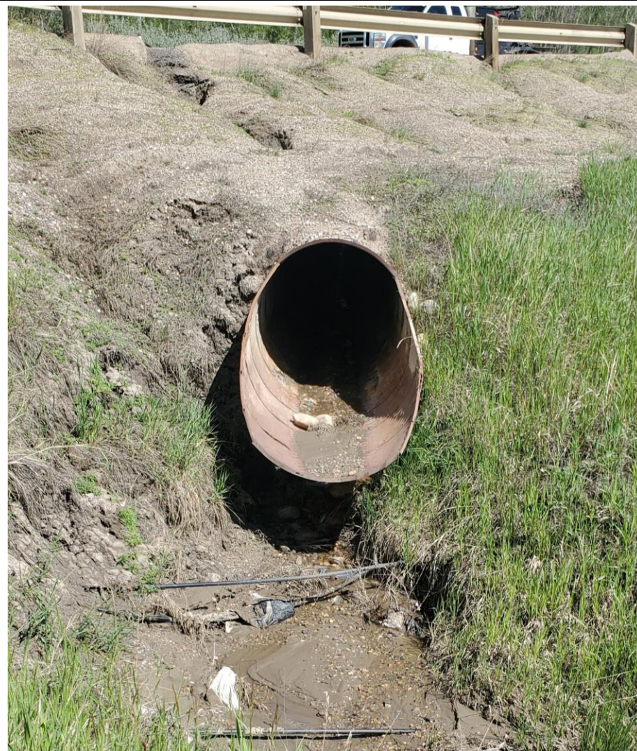
Photo 60-01. Close-up of hanging culvert outlet (35+700). Ongoing erosion below culvert and rilling above. No major change from the 2019 condition.
