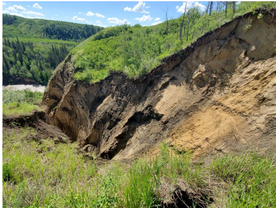
Photo 60-03. Gully and slide area below the culvert outlet at 35+700, offset approximately 125 m from the highway. Mass movement occurred in 2016, ongoing minor retrogression but no new major retrogressions or movements were noted in 2020. Gully sidewalls are intermittently stable.
