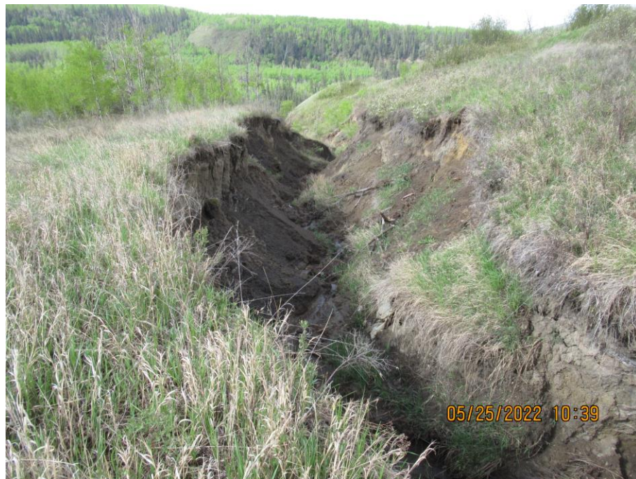
Photo 60-02. Looking downslope at erosional gully below culvert shown in Photo 60-01 (35+700). Active slumping on gully walls. Worse from the 2020 condition.
