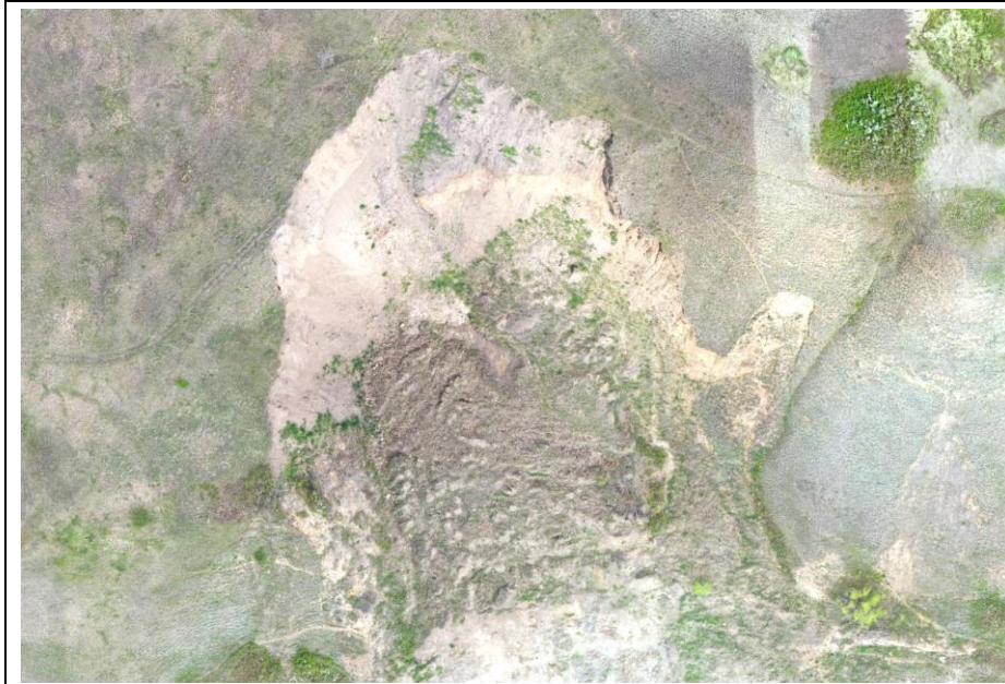
Photo 60-04. Overhead drone image of a major slide/earth flow that occurred in 2016. Ongoing erosion of exposed scarp but overall minor retrogression since that time. Slide area is offset approximately 180 m from the highway (35+950).
