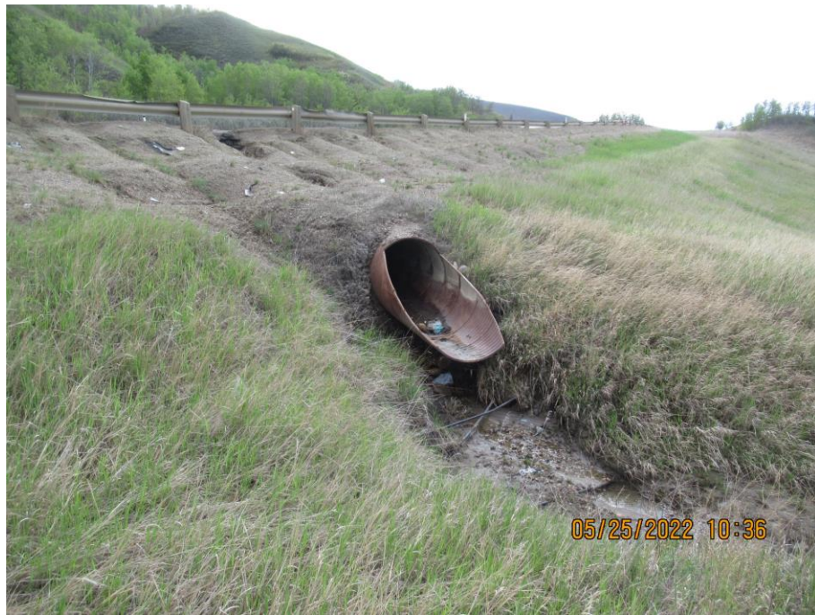
Photo 60-01. Close-up of hanging culvert outlet (35+700). Ongoing erosion below culvert and rilling above. Rill erosion slightly deeper but no major change from the 2020 condition. Scour depth below culvert inlet was 0.7 m.
