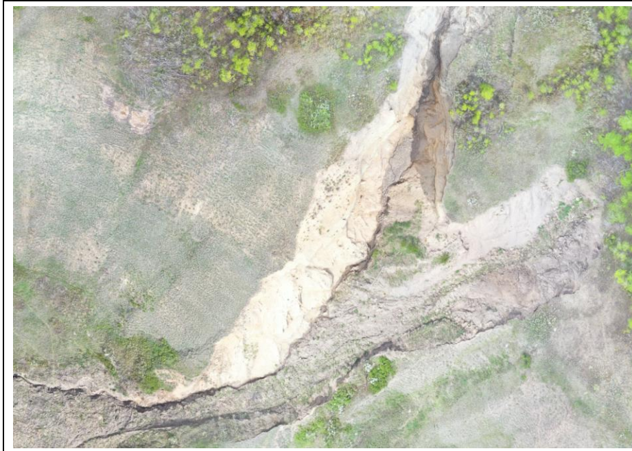
Photo 60-03. Overhead drone image of gully and slide area below the culvert outlet at 35+700, offset approximately 125 m from the highway. Mass movement occurred in 2016, increased gully incision, ongoing erosion of the flanks and further retrogression of slide on the right (east) side. Gully sidewalls are intermittently stable.
