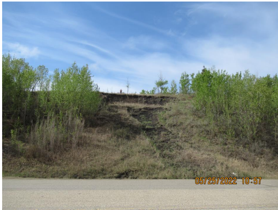
Photo 60-05. Shallow slide/flow within through-cut area on the south cut slope (35+830). First observed in 2016, further displacement of the slide mass since 2020. Backscarp is now 3 m high and the slide toe is partially blocking the ditch.
