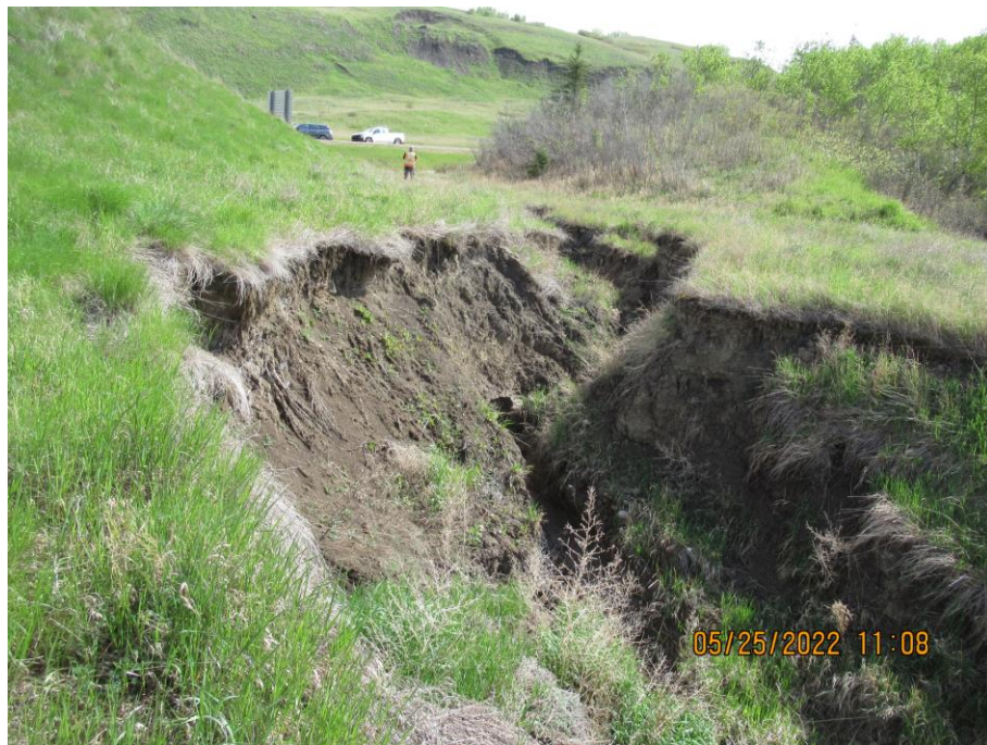
Photo 60-06. Headcutting and erosional gullying occurring below roadway (36+050).
