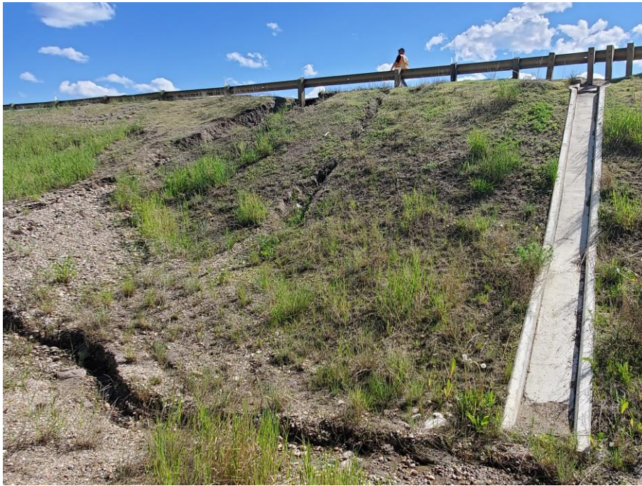
Photo 61-04. Erosion within southeast side of Grouard Bridge abutment slope (37+050). Concrete swale and slope repairs were constructed in 2017/2018. Road runoff is draining over the pavement edge before reaching the swale due to sand and gravel buildup. Gravel and geocell slope repair was effective in select areas but has washed out in others.
