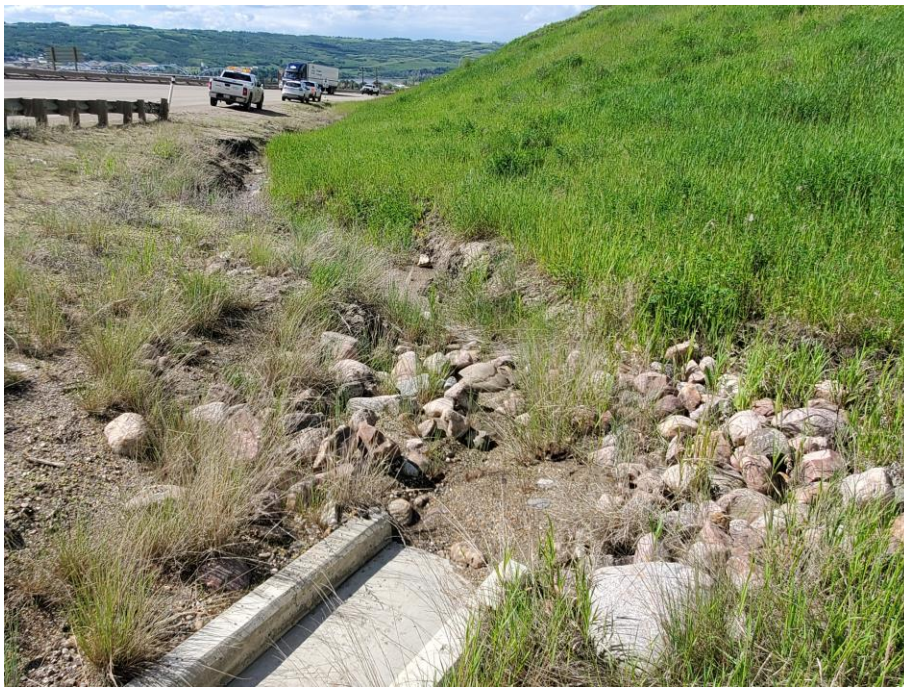
Photo 61-05. Swale and cobble armor outlet at the northeast side of the Grouard Bridge (37+125). Ditch erosion is active further downstream from outlet.
