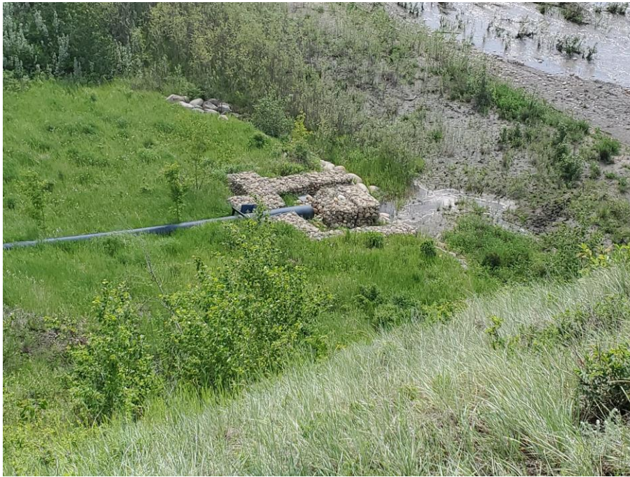
Photo 61-03. Looking towards trunk drain outlet structure which was functioning as intended.
