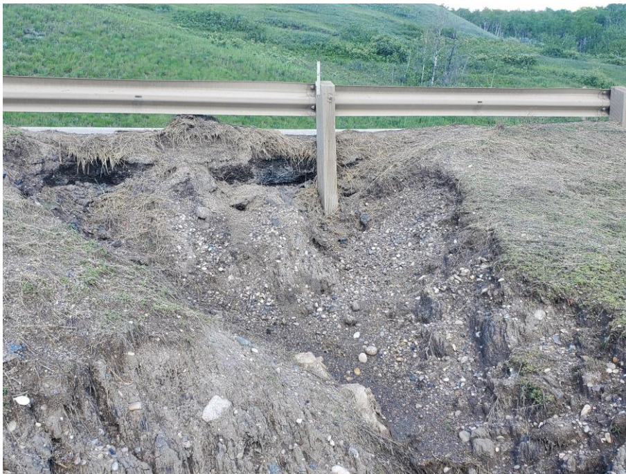
Photo 61-02. Local erosion around guardrail post and gully of embankment slope below (36+470). Erosion ongoing with minor lateral expansion since the previous inspection.
