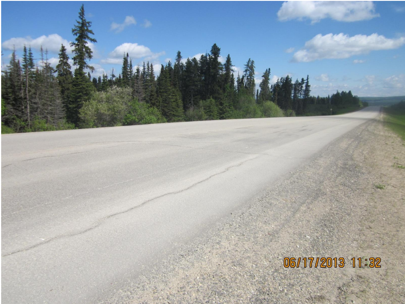
Photo 1: Looking north. Note pavement cracking and distortion.
