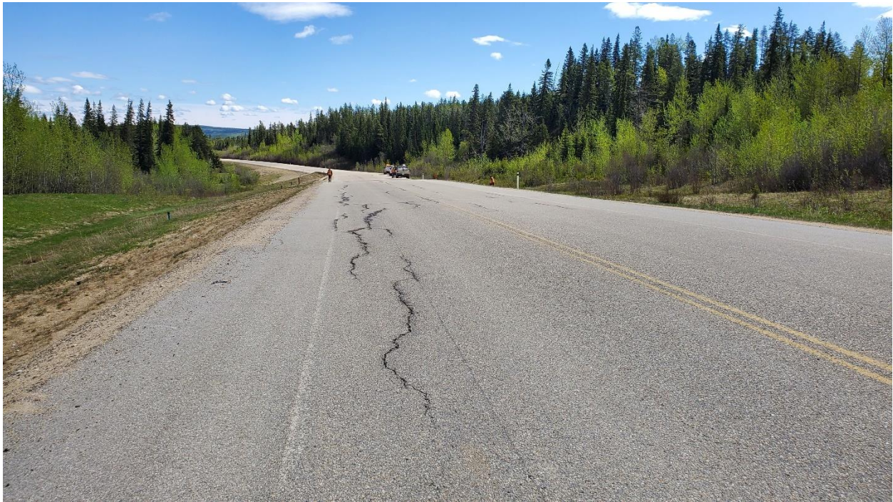
Photo 2 – Looking north at cracking in highway surface immediately south of the pile wall.
