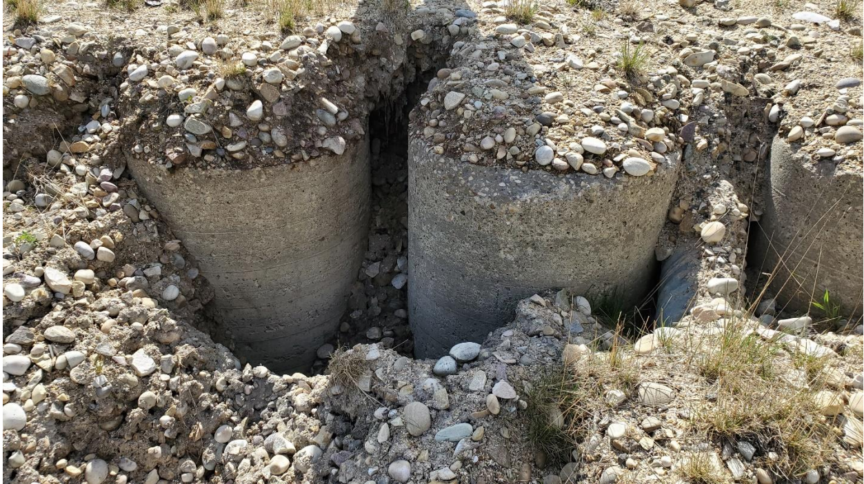
Photo 9: Erosion and/or movement away from the piles around the southwest down drain.
