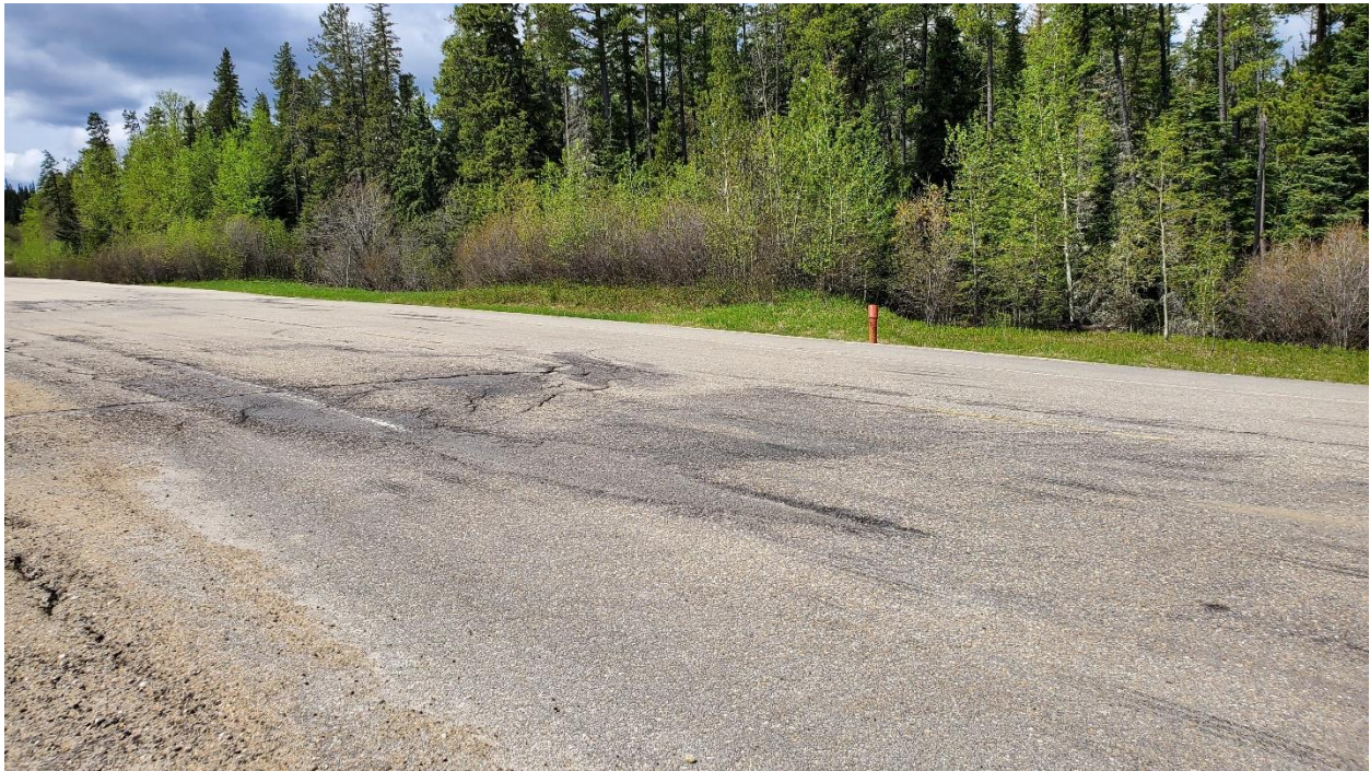
Photo 12 – Crack pattern at SH001A site.
