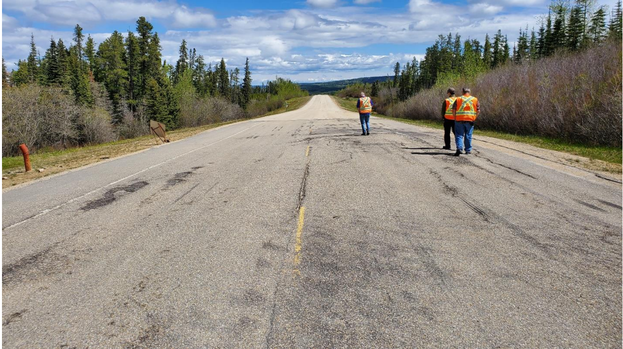
Photo 13 - Looking northeast at second crack with slight pavement dip just beyond at SH001A site.
