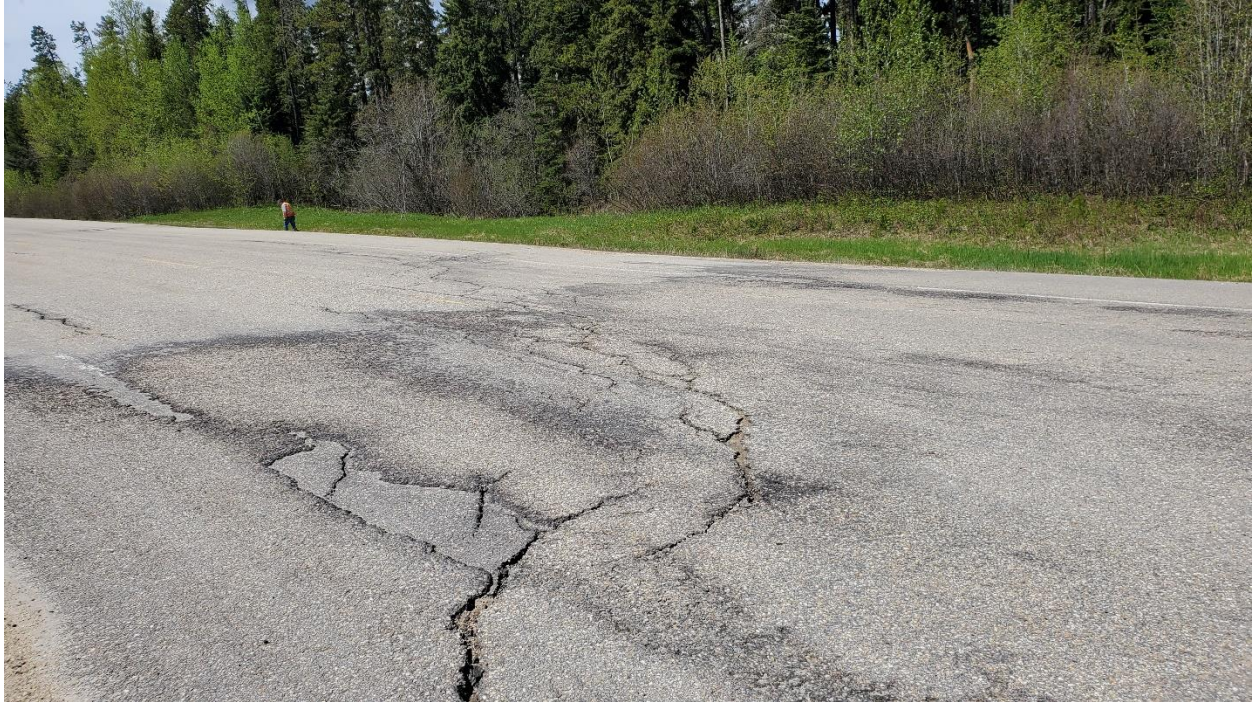
Photo 15 - Looking west at cracks at south end of patch at SH001A site.
