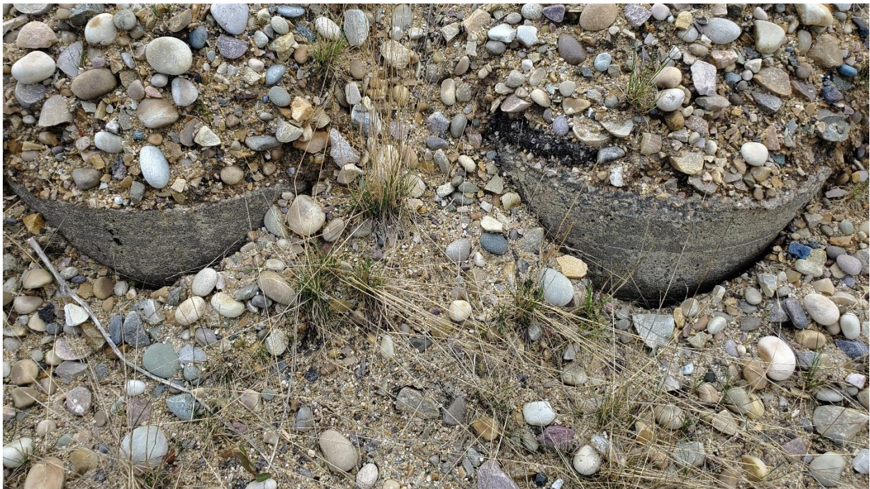
Photo 10: Soil pulling away from the downslope side of piles near the northwest down drain.
