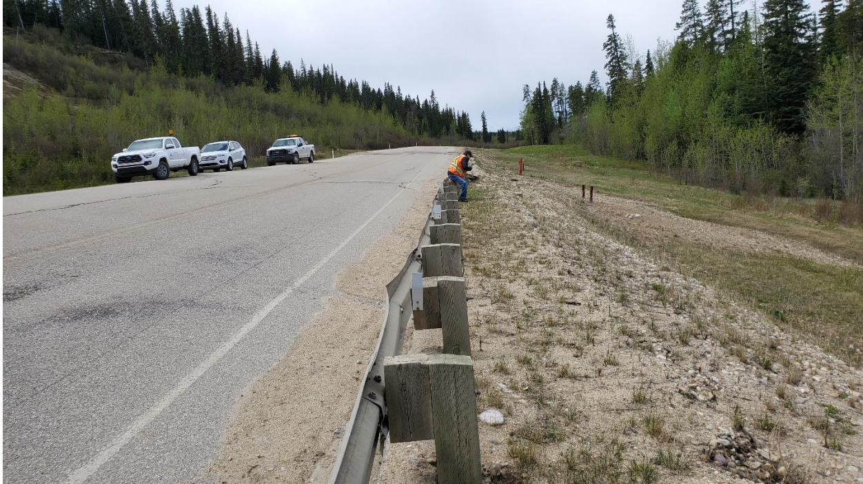
Photo 7 – Looking southwest at cracked curb at south end of guardrail.
