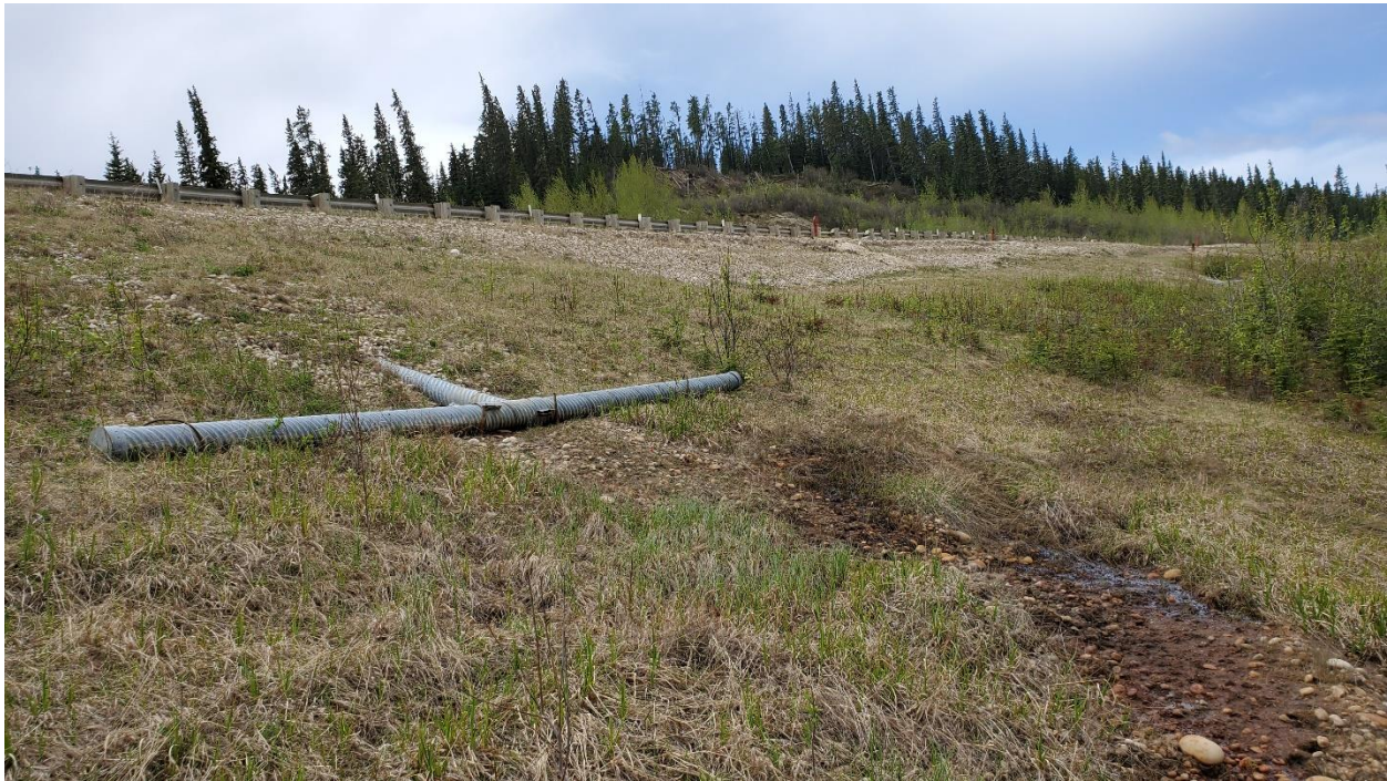
Photo 8 – Seepage out of slope below north-most T-drain.
