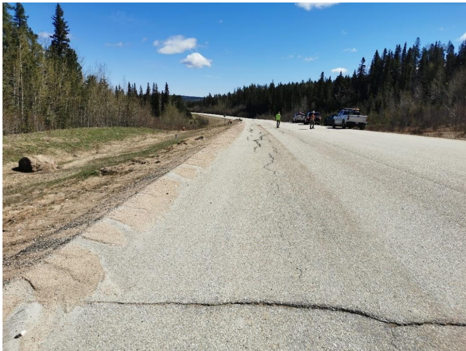
Photo 2, SH001-1 – Looking north at cracking in highway surface immediately south of the pile wall.
