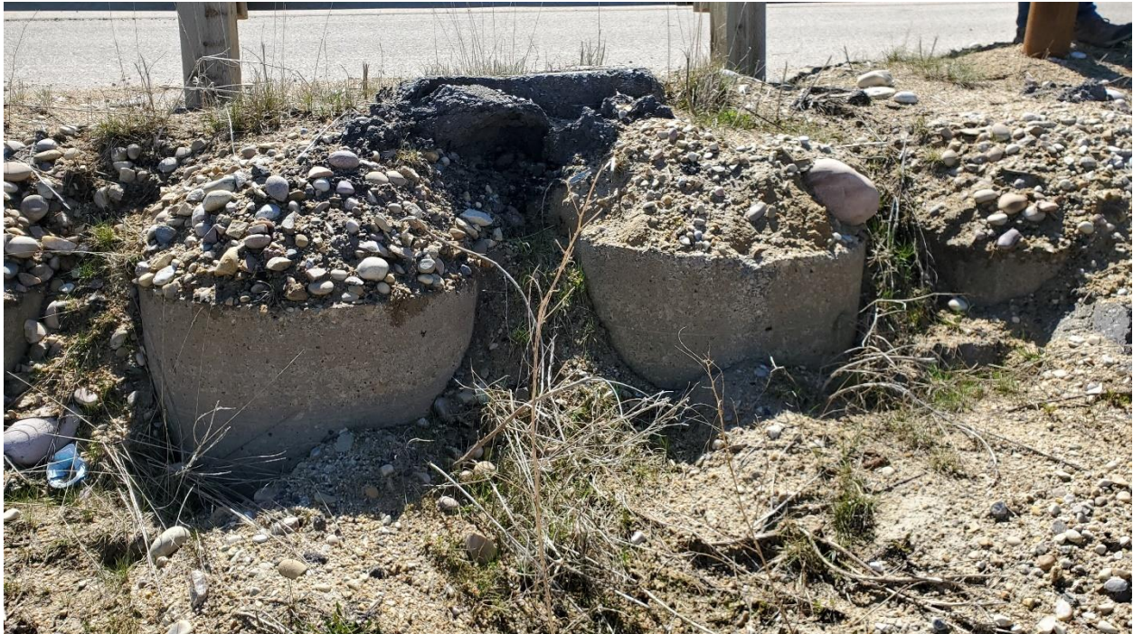
Photo 10, SH001-1 – Soil pulling away from the downslope side of piles near the northwest down drain.
