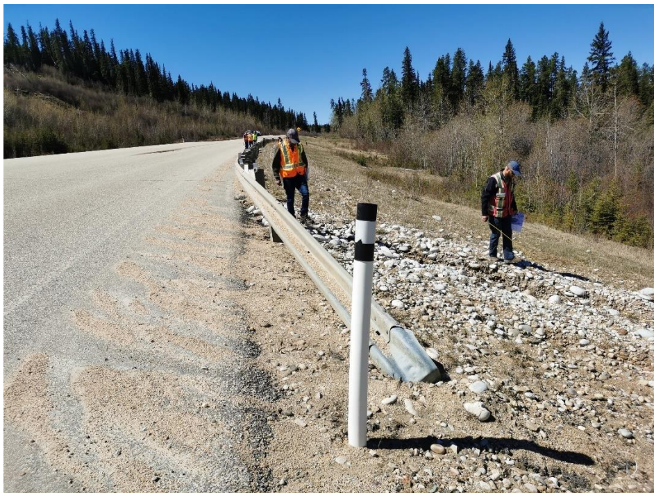
Photo 6, SH001-1 – Looking south at cobbles placed in gully at north end of guardrail.
