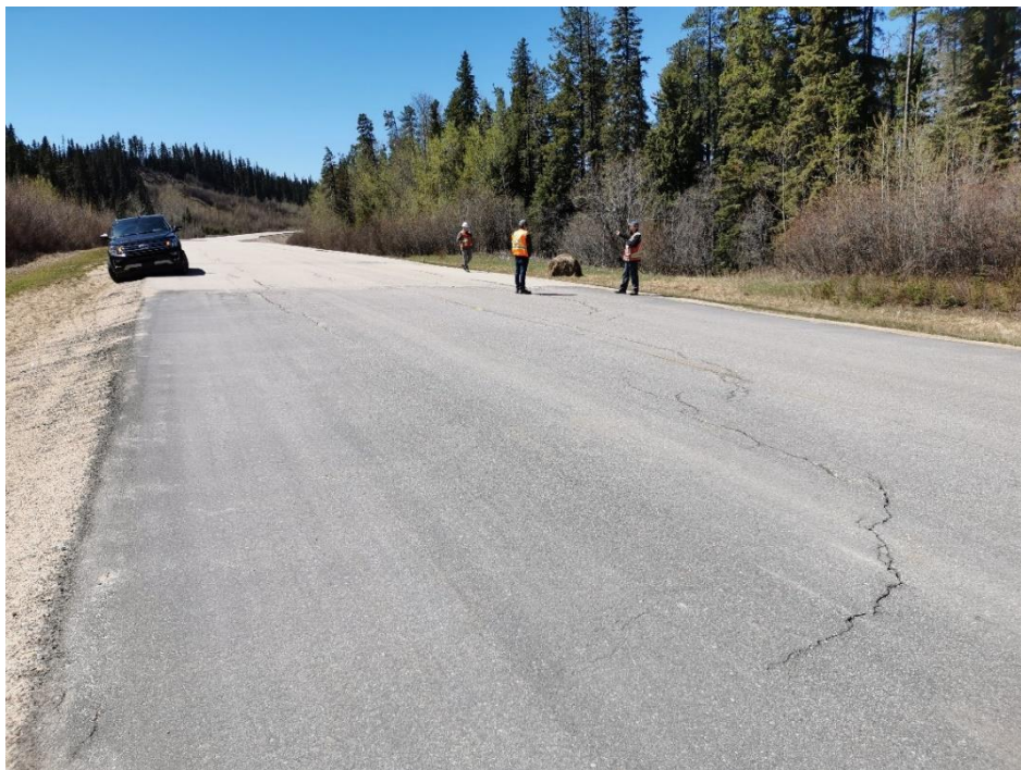
Photo 16, SH001A-1 - Looking west at cracks at south end of patch.
