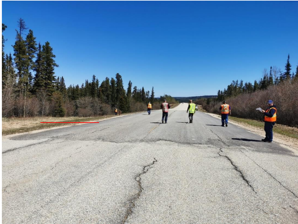
Photo 15, SH001A-1 – Looking northeast at roadway crack and scarp (red line) at tree line.
