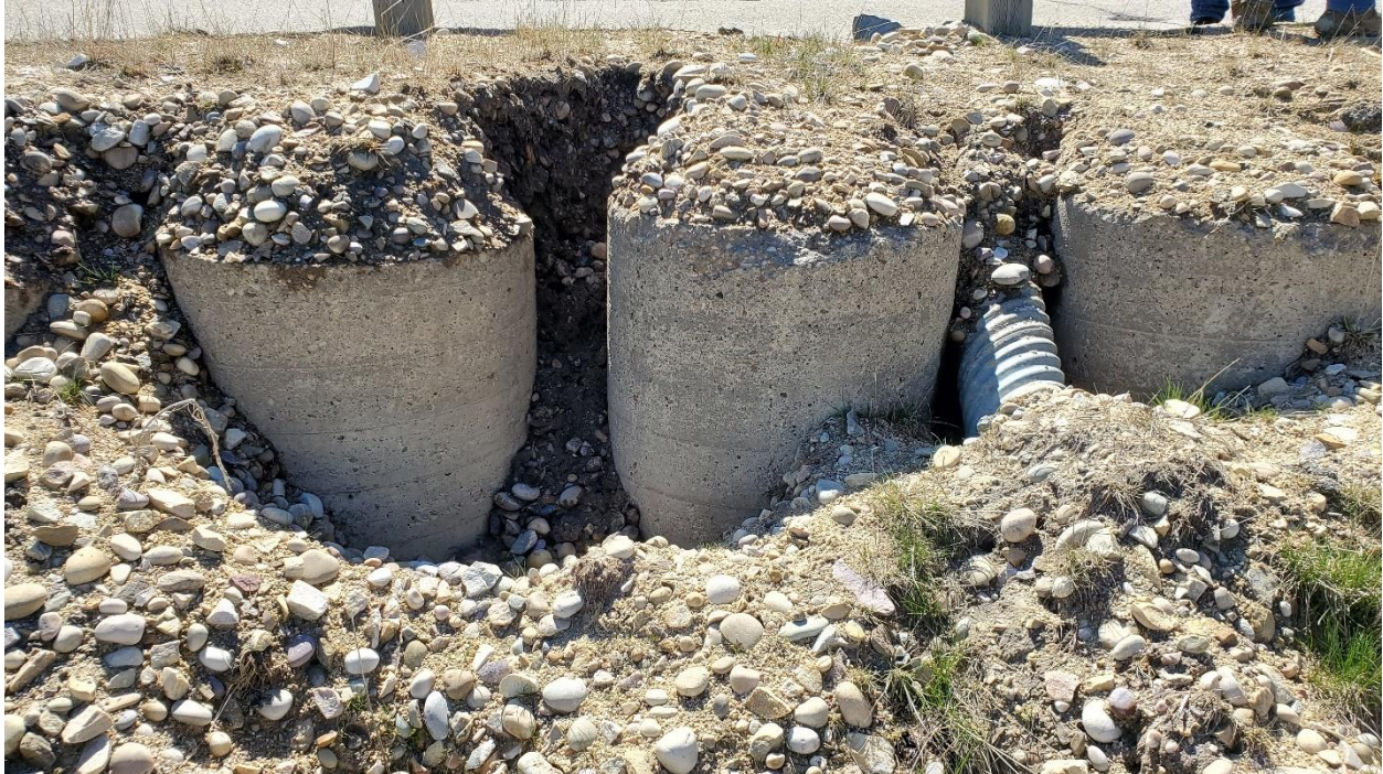
Photo 9, SH001-1 – Erosion and/or movement away from the piles around the southwest down drain.
