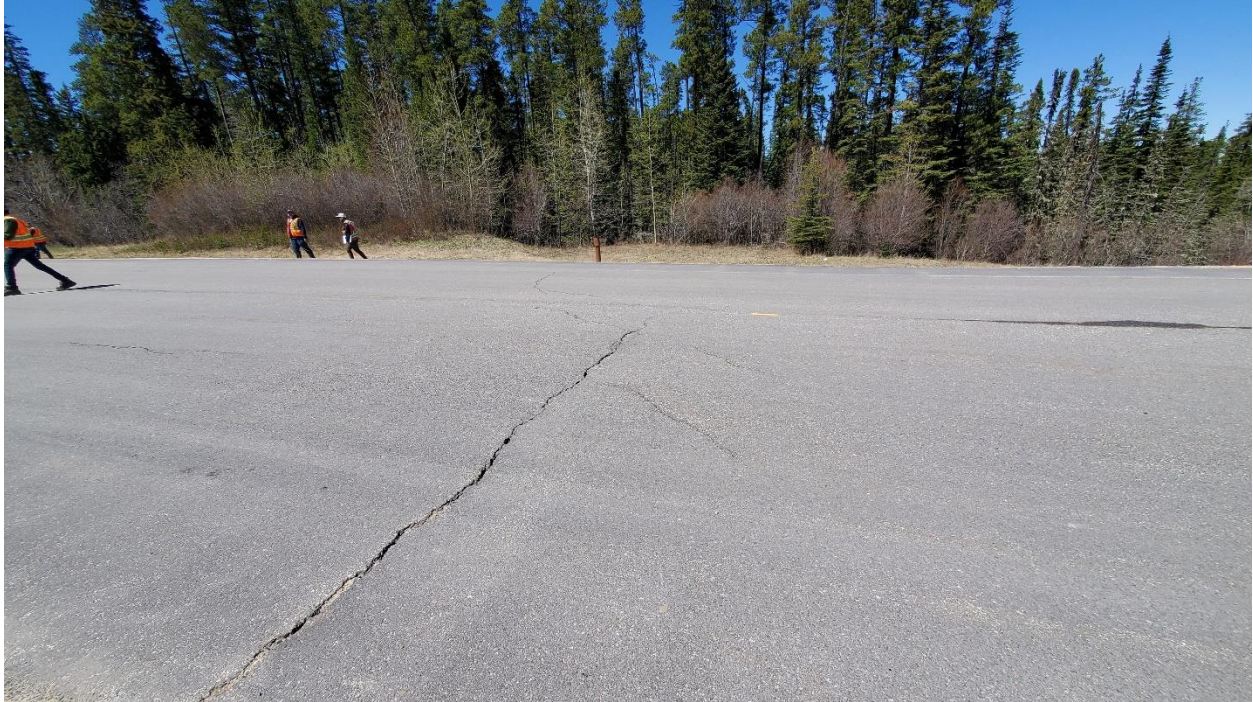
Photo 13, SH001A-1 – Crack pattern at the north end of the Site.
