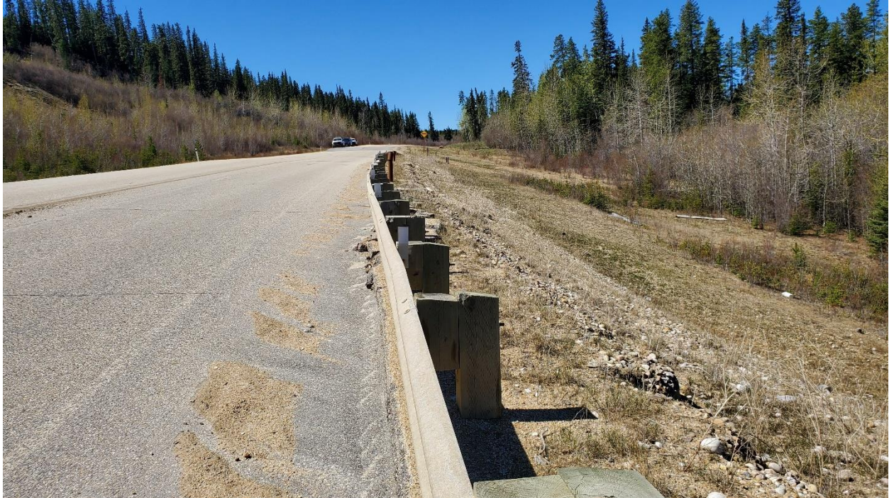
Photo 7, SH001-1 – Looking southwest at cracked curb at south end of guardrail.
