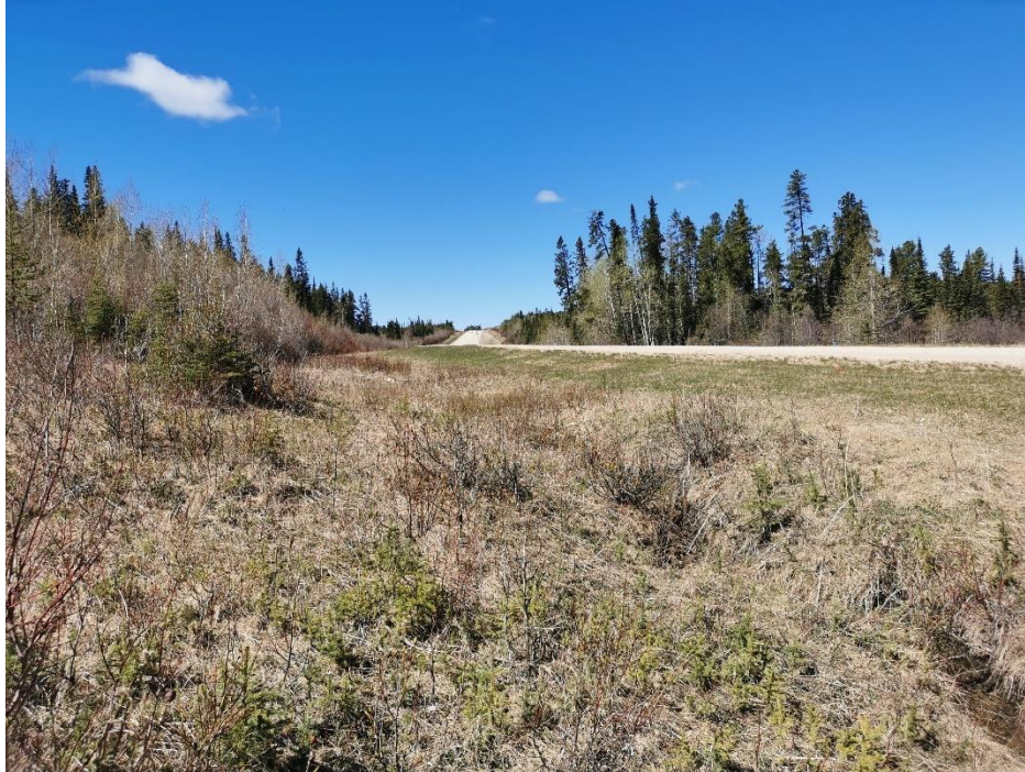
Photo 5, SH001-1 – Looking south at erosion in east ditch.
