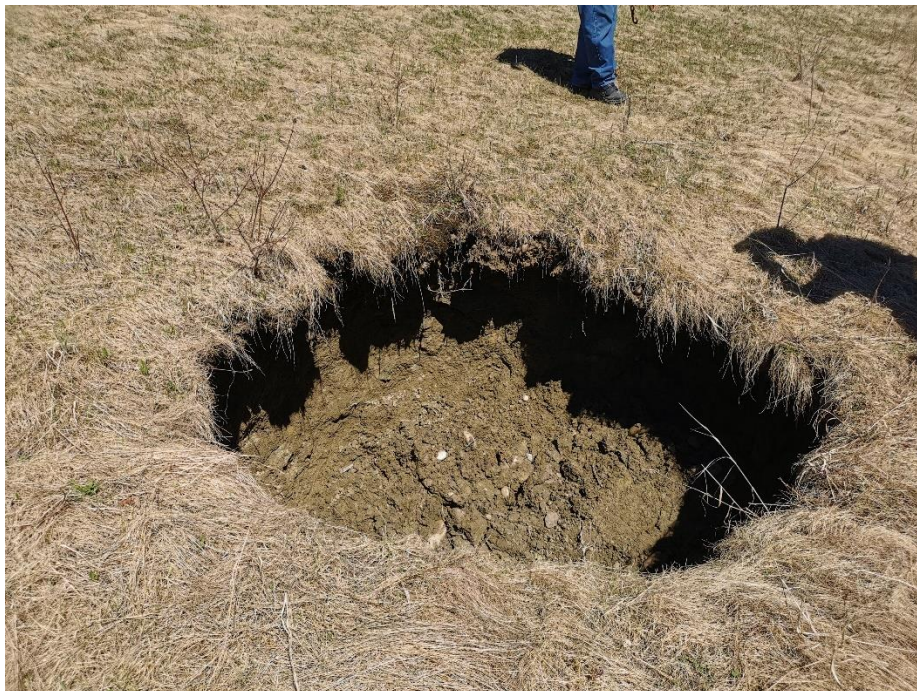
Photo 12, SH001-1 – Two sinkholes at culvert inlet have combined to form a larger sinkhole.
