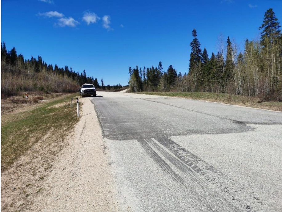
Photo 1, SH001-1 – Looking southwest at patch over cracks forming at the southwest end of the wall .
