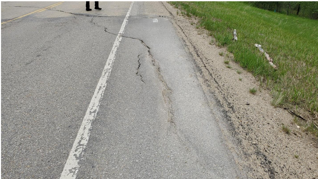
Photo 4: Looking south at crack at south end of patch at north end of the site.
