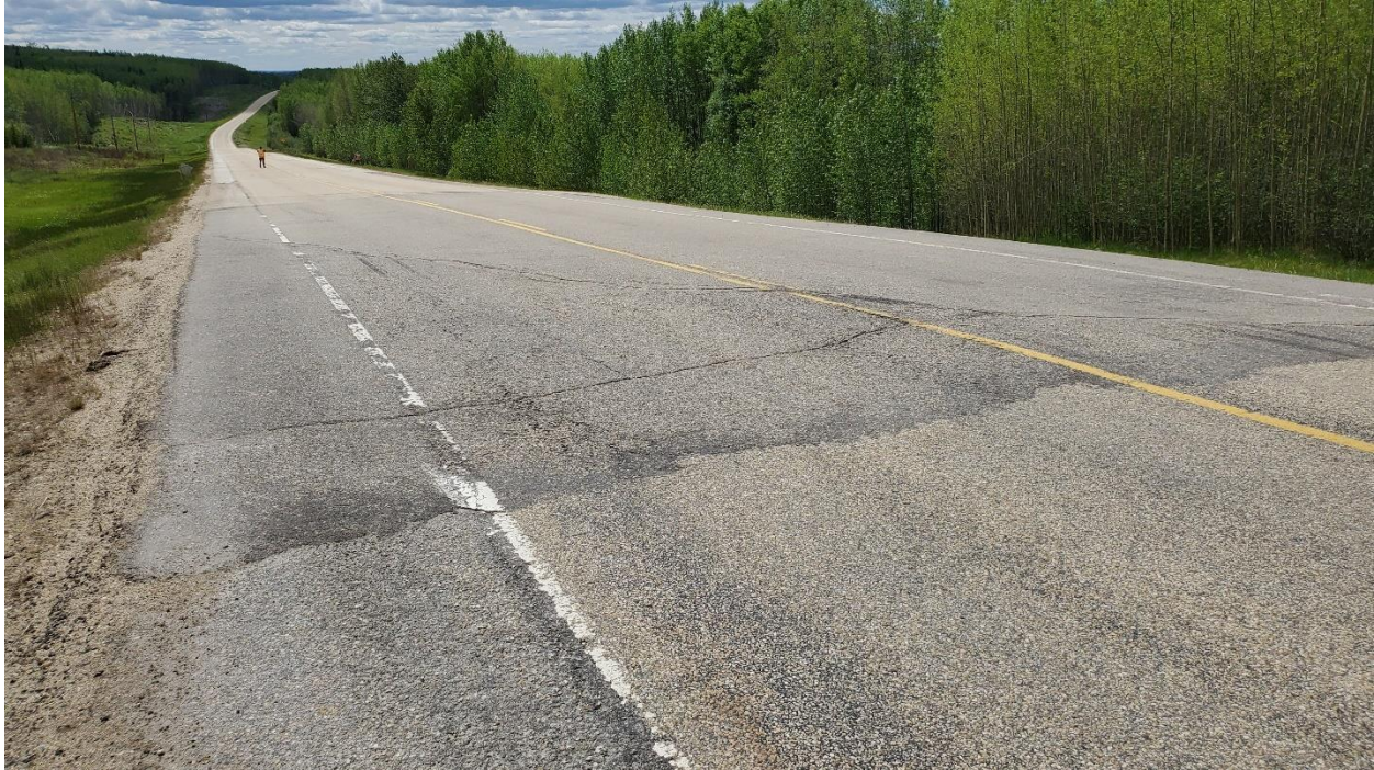
Photo 1 – Looking south from east shoulder at main scarp crack and patch at north end of site.
