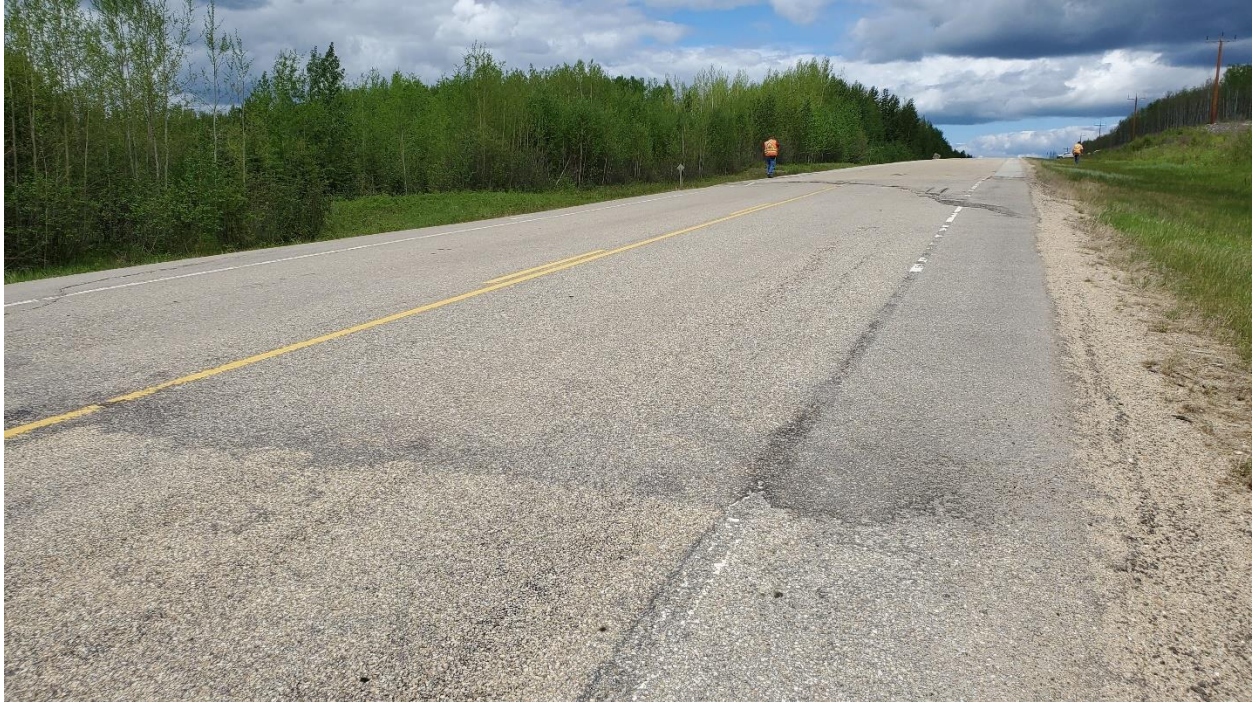
Photo 3: Looking north at hump over main scrap crack at north end of the site.
