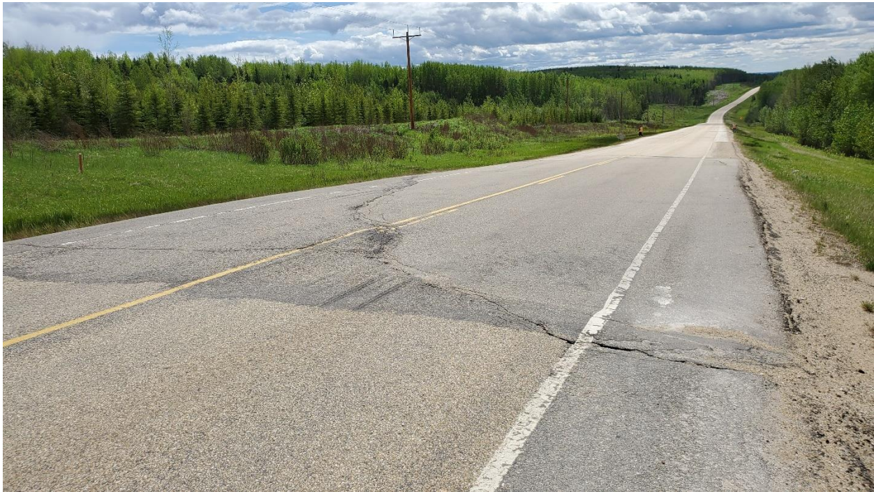
Photo 2 – Looking south from west shoulder at main scarp crack and patch at north end of site. Note powerline installed on east side of highway since 2017 visit.
