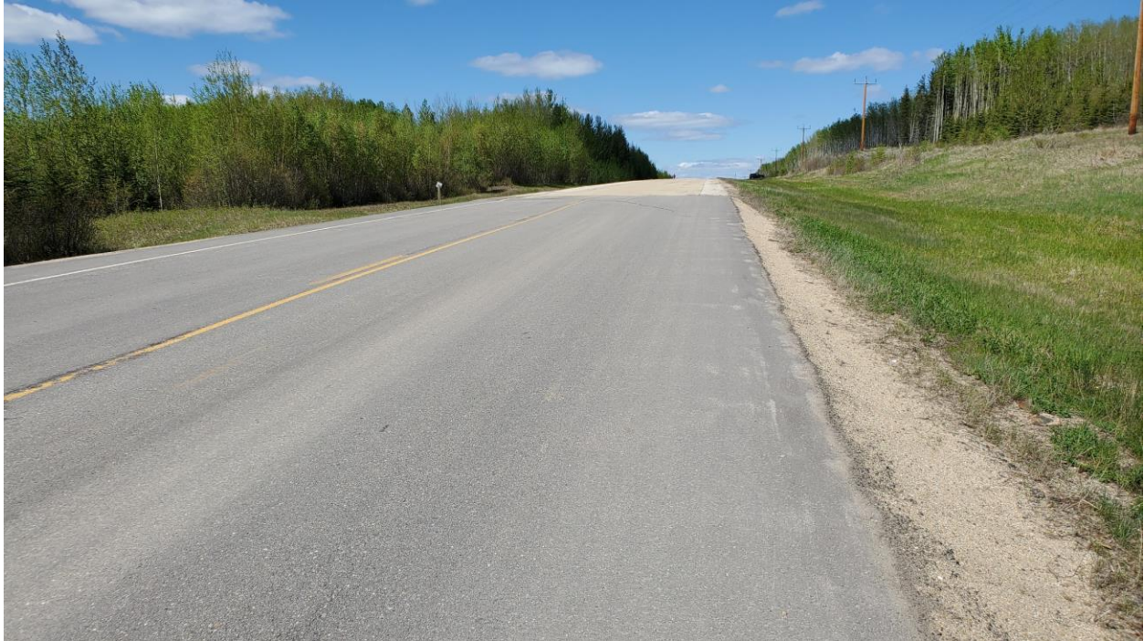
Photo 3: Looking north at hump over main scrap crack at north end of the site.
