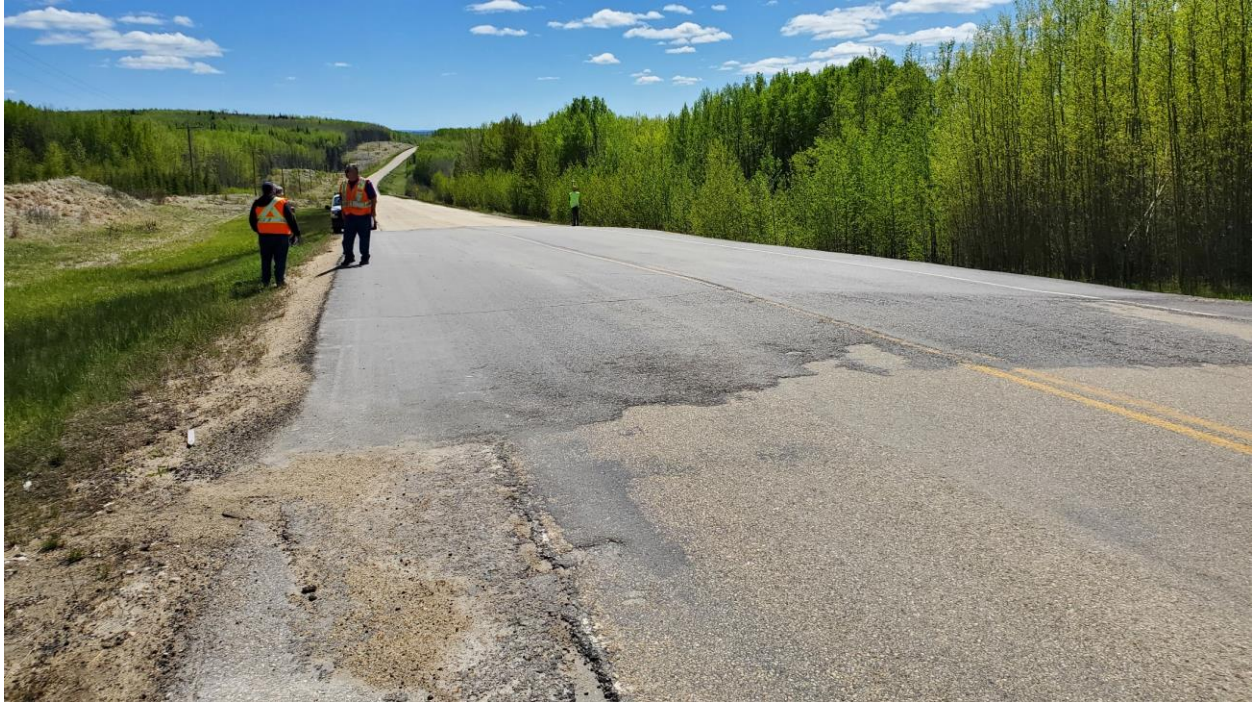
Photo 1 – Looking south from east shoulder at main scarp crack and patch at north end of site.
