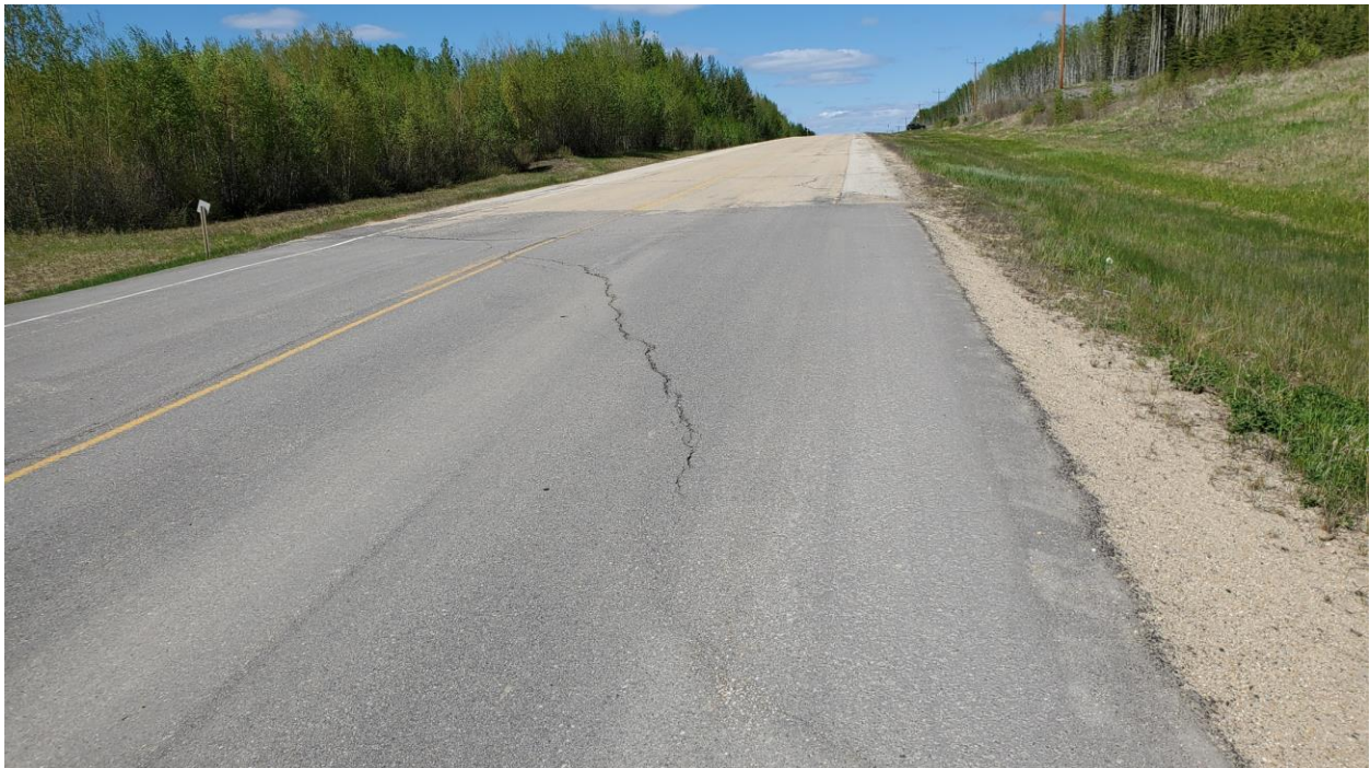
Photo 4: Looking south at crack at south end of patch at north end of the site.
