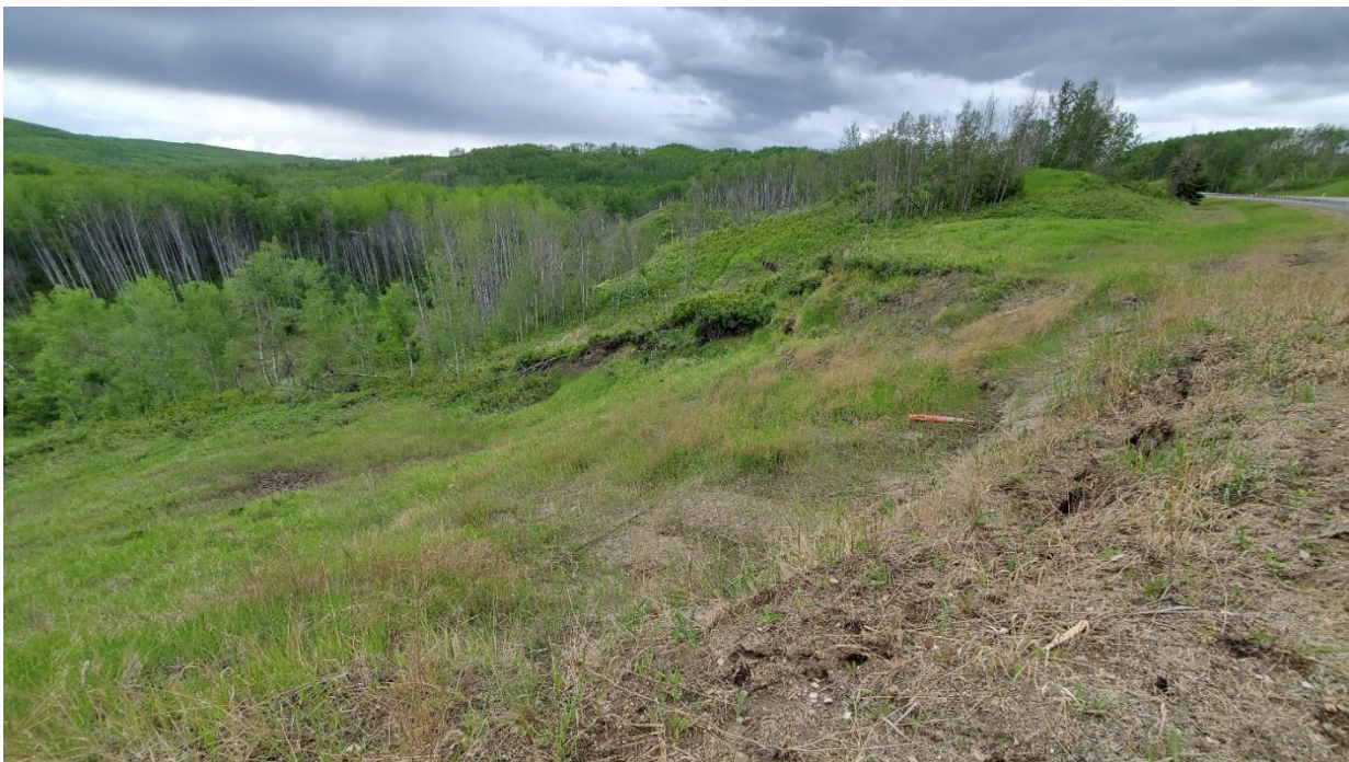
Photo 4 – Slide B: View of backscarp looking north.
