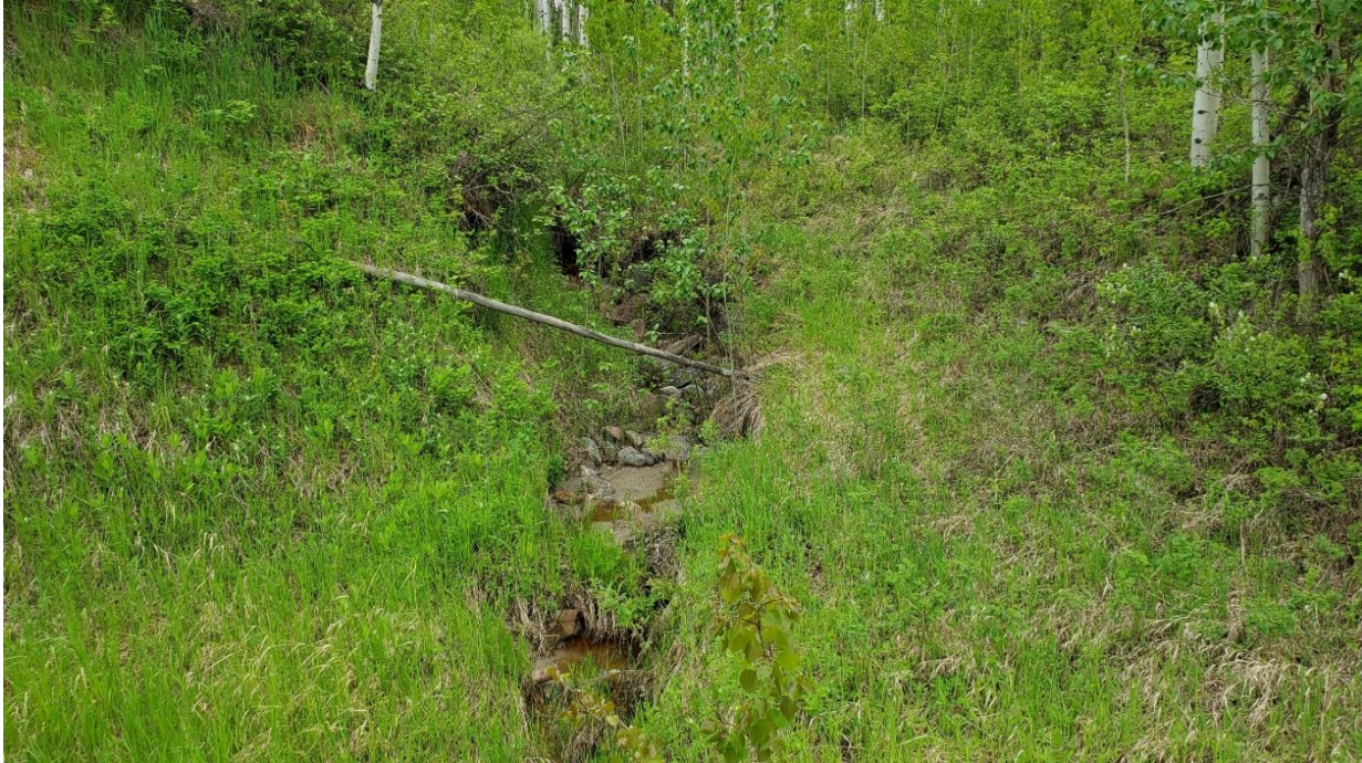
Photo 9 – Slide A: Erosion gully outside culvert inlet, looking northeast.
