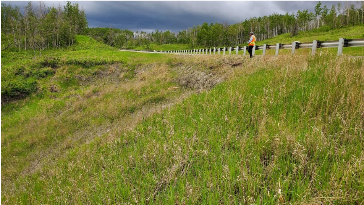
Photo 1 – Slide B: Backscarp and highway, looking north.
