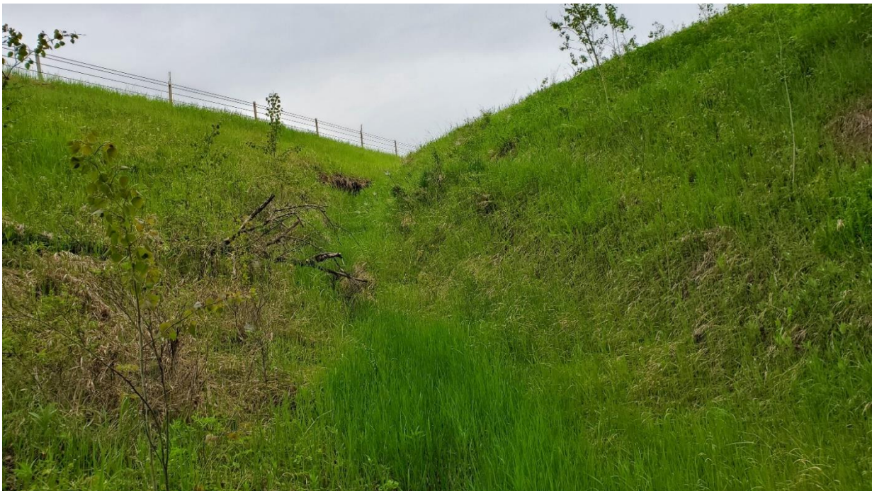
Photo 10 – Slide A: Erosion gully in sideslope draining towards culvert inlet, looking north.
