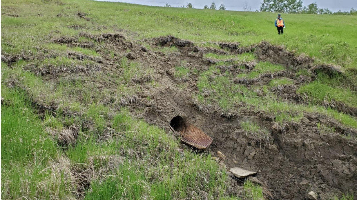
Photo 7 – Slide A: Slope movement near the toe of the slope, looking east. Culvert outlet became buried in 2017 and exposed again in 2019 (deteriorated significantly since 2015).
