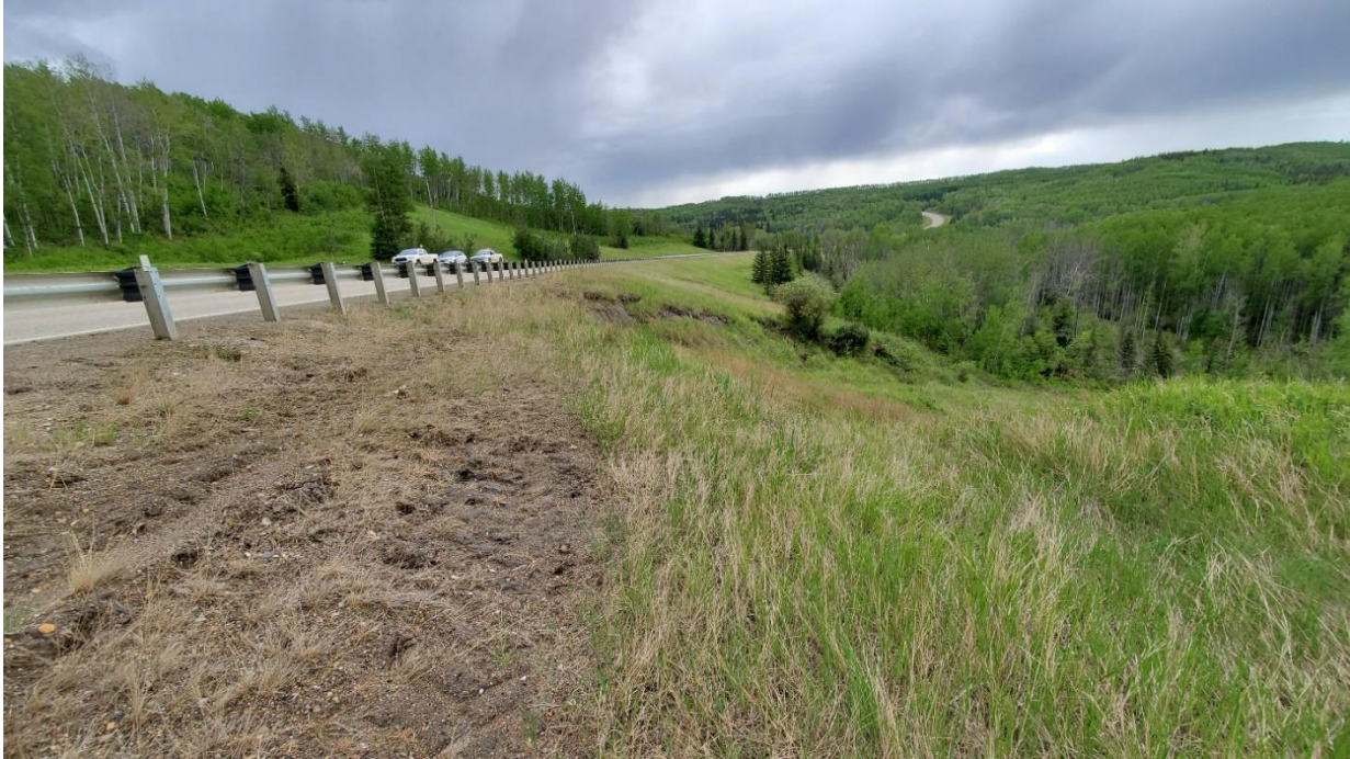
Photo 3 – Slide B: Backscarp and highway, looking south.
