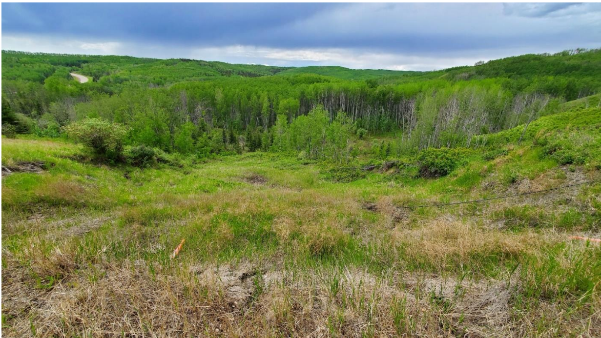
Photo 2 – Slide B: View of slope failure and slide block, looking southwest.
