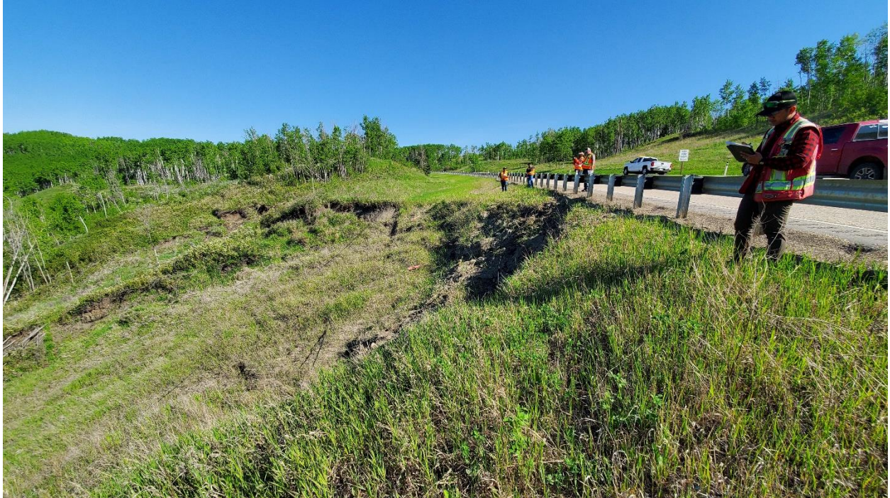
Photo 1 – Slide B: Backscarp and highway, looking north.
