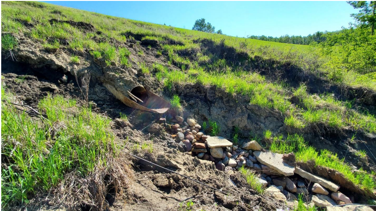
Photo 8 – Slide A: Slope movement near the toe of the slope, looking east. Recent movement has occurred below and to the left of the culvert outlet.
