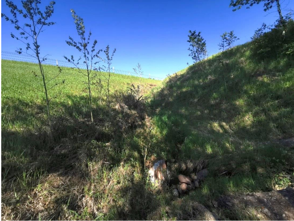
Photo 11 – Slide A: Erosion gully in sideslope draining towards culvert inlet, looking north.
