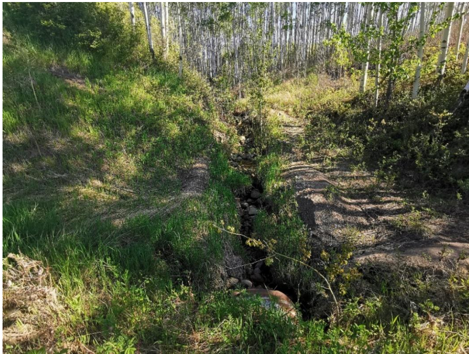
Photo 10 – Slide A: Erosion gully outside culvert inlet, looking northeast. Note fresh silt deposit on the right-hand side.
