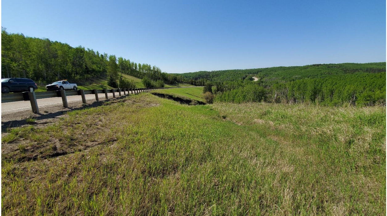
Photo 3 – Slide B: Backscarp and highway, looking south.
