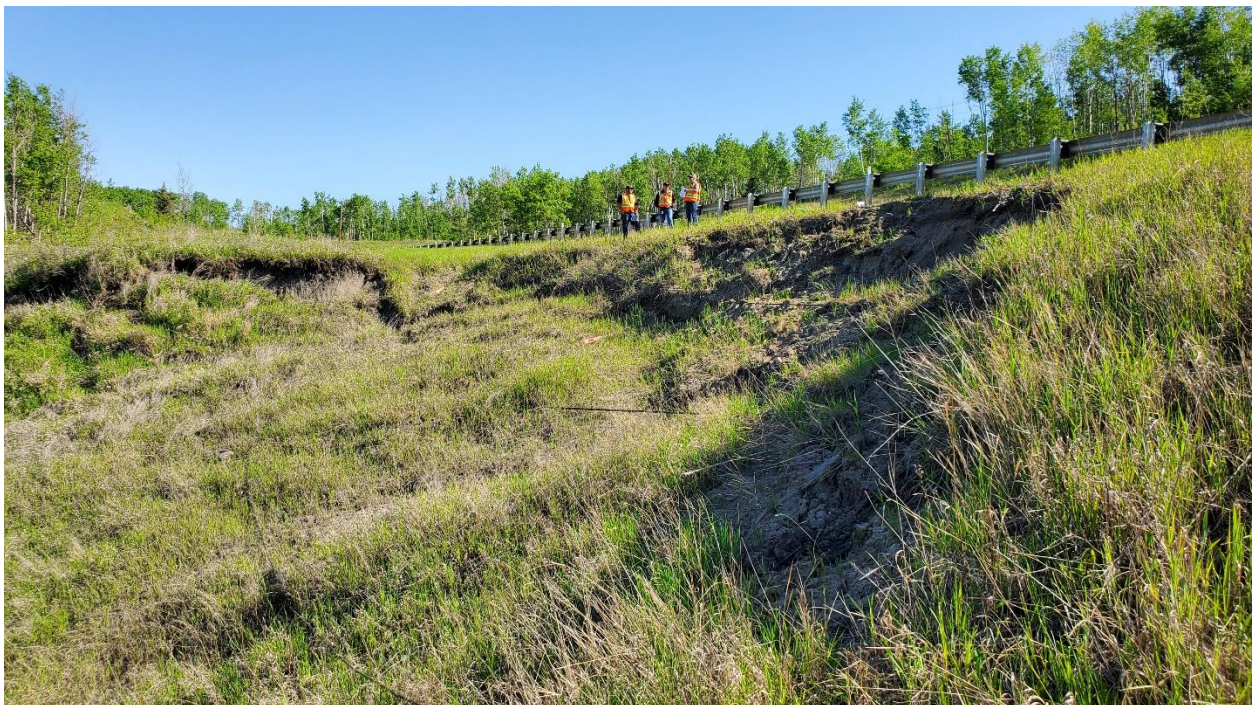
Photo 4 – Slide B: View of backscarp looking north.
