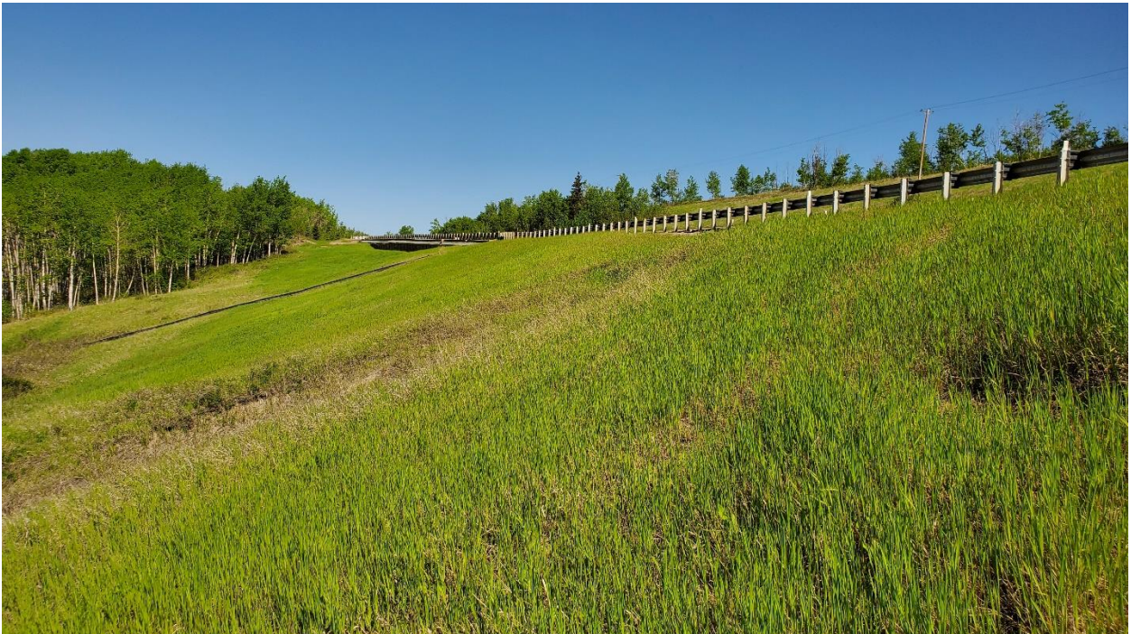
Photo 6 – Slide A: Embankment sideslope, looking north.
