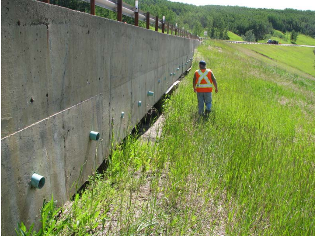
Photo 3 – Voids Underneath Cap Beam, Looking Southeast
