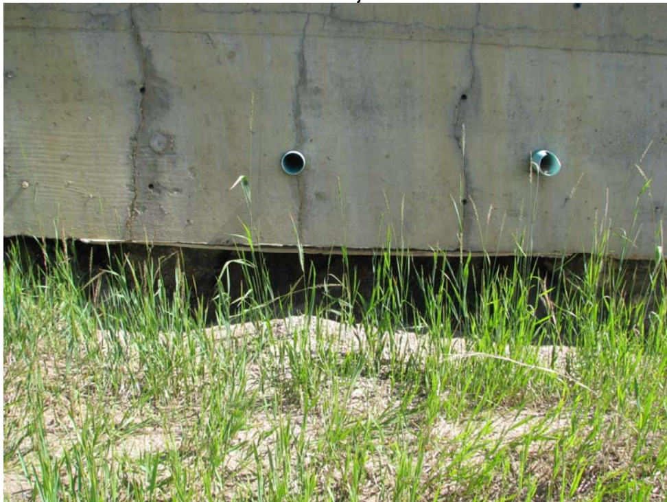
Photo 6 – Void underneath the pile cap showing sand washed out from the front of the pile cap.
