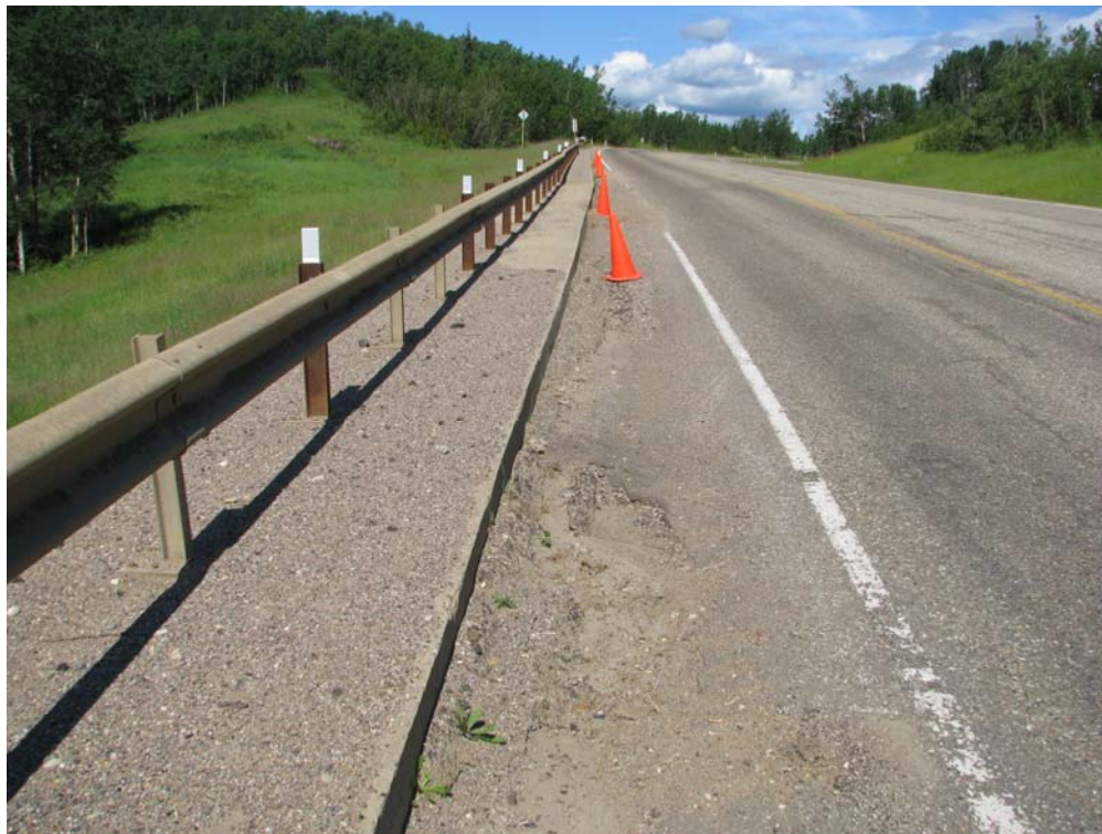
Photo 4 – Developed Piping holes in front of pile wall, looking northwest.
