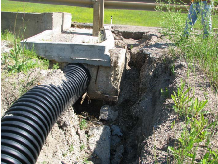
Photo 1 – View of pile wall looking northwest, showing the drainage inlet (Plugged with Sand).
