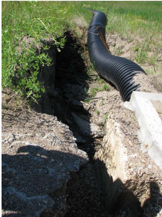
Photo 2 – Downslope view of drainage pipe, showing erosion around it.
