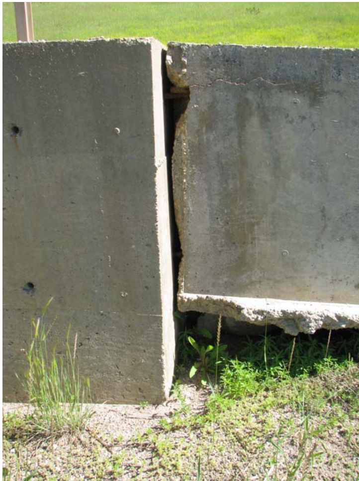
Photo 5 – Concrete joint Worsened.
