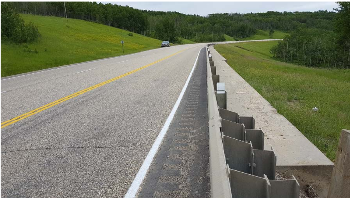
Photo 6 – Looking southeast at repaired and overlaid asphalt surface. Note new bridge rail installed along the top of the cap beam.
