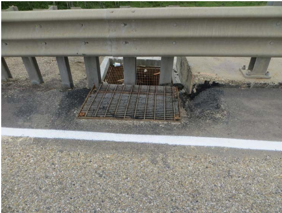
Photo 2 – Catch basin inlet at south end of wall leading to the elephant trunk downpipe.
