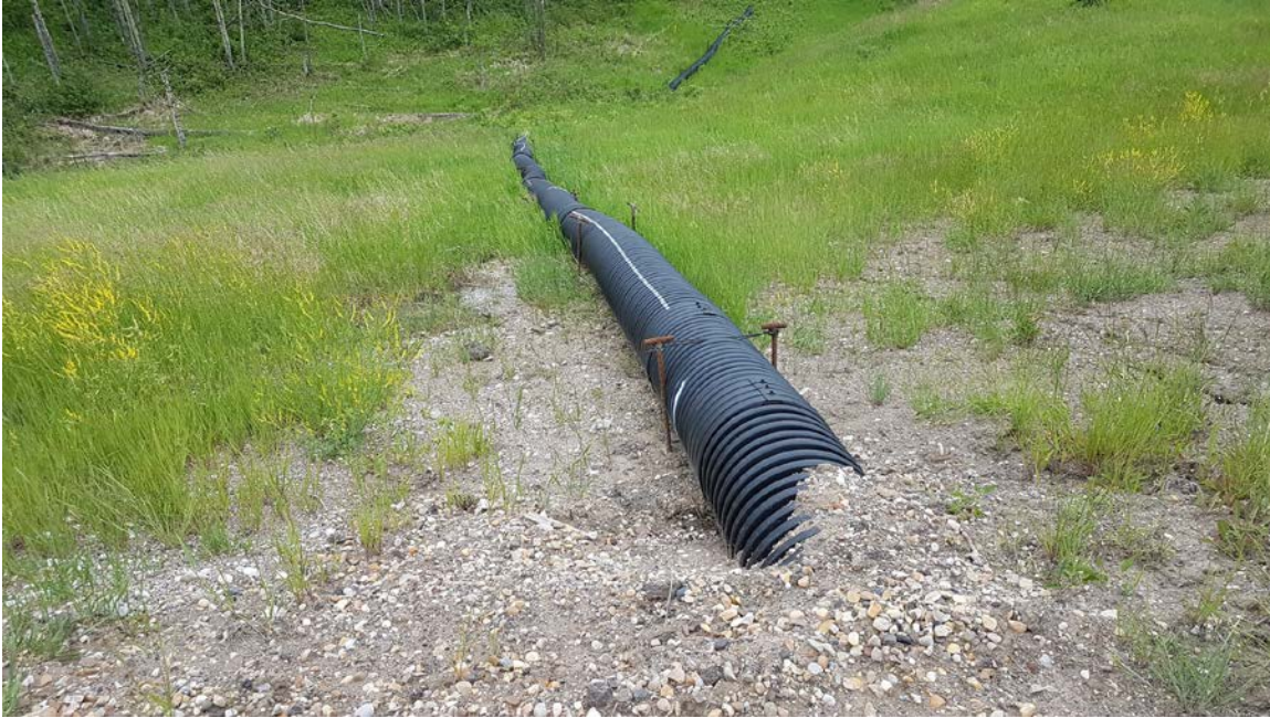
Photo 3 – Looking downslope at “elephant trunk” drain pipe.
