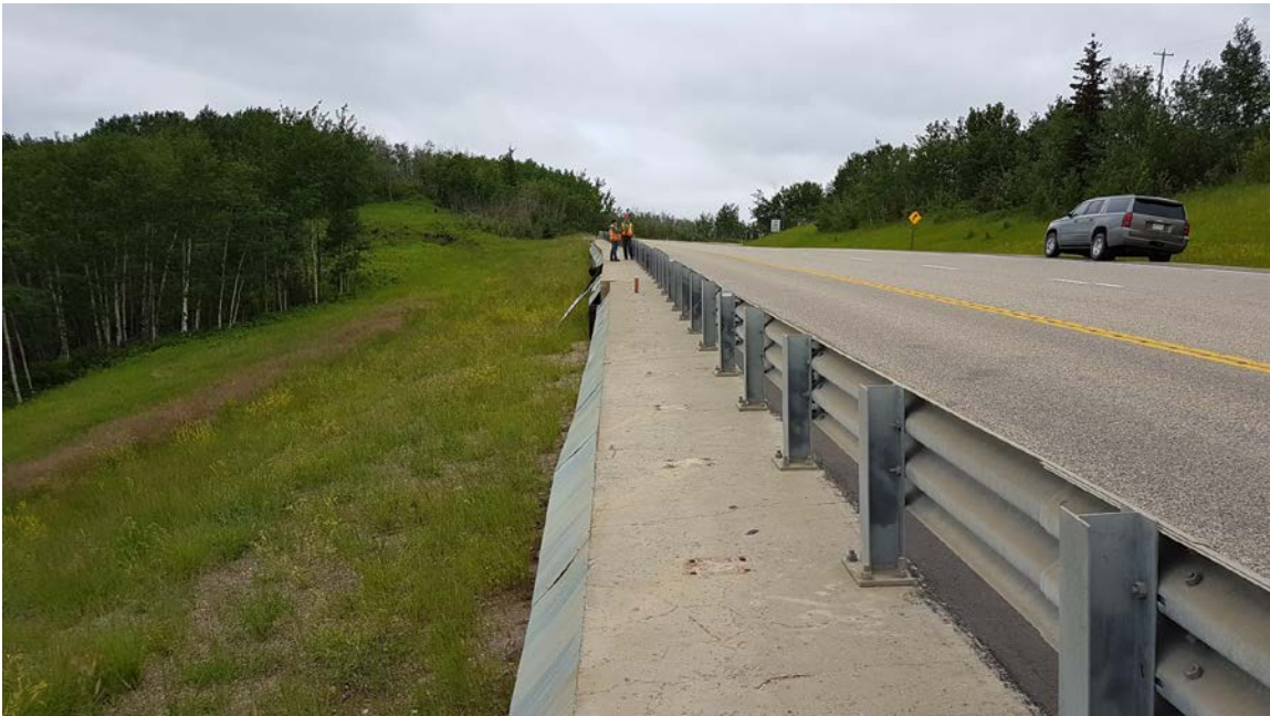
Photo 4 – Looking northwest at repaired and overlaid asphalt surface. Note new bridge rail installed along the top of the cap beam and damaged flashing at about the center of the wall.
