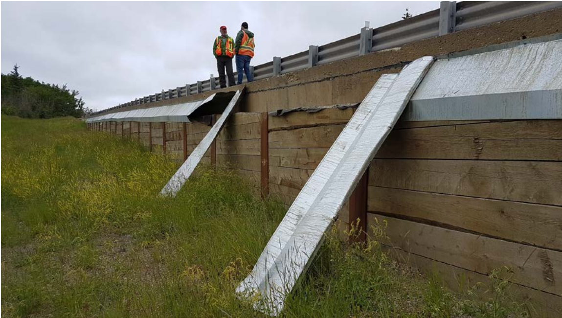
Photo 5 – Looking northwest at main section of damaged flashing.
