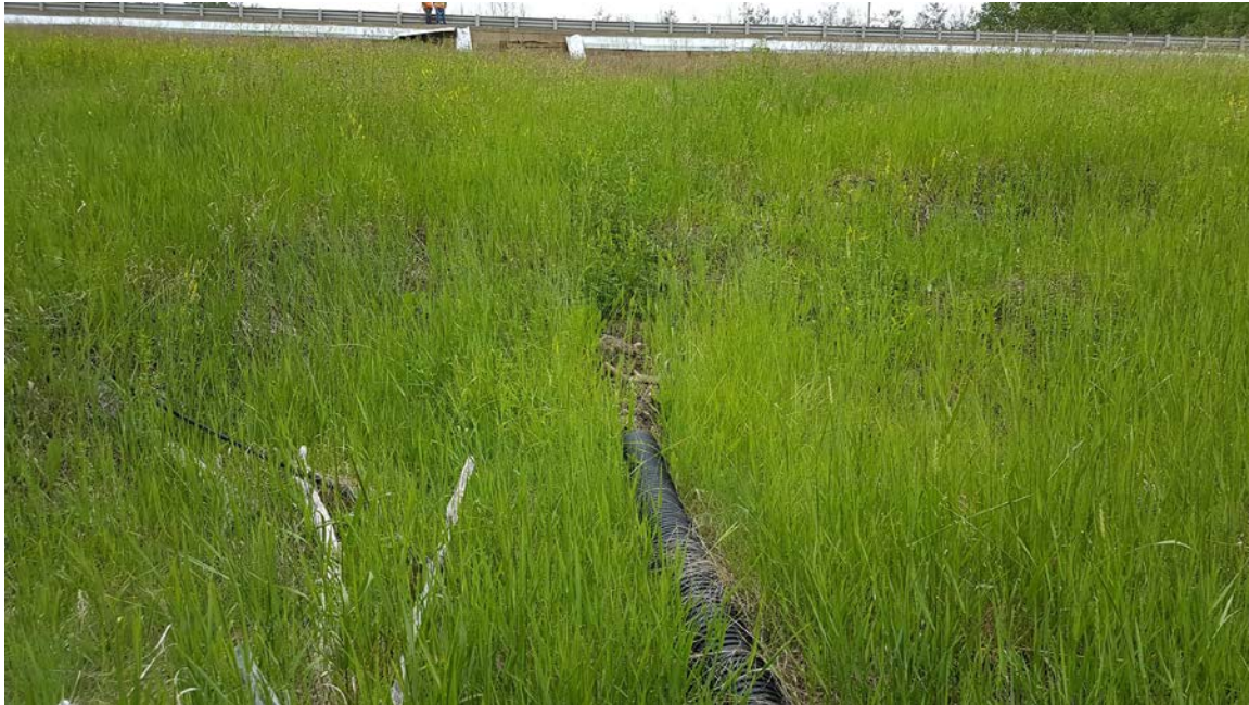
Photo 7 – Looking northeast at subdrain in the lower part of the slope that was located and extended during 2016 construction.
