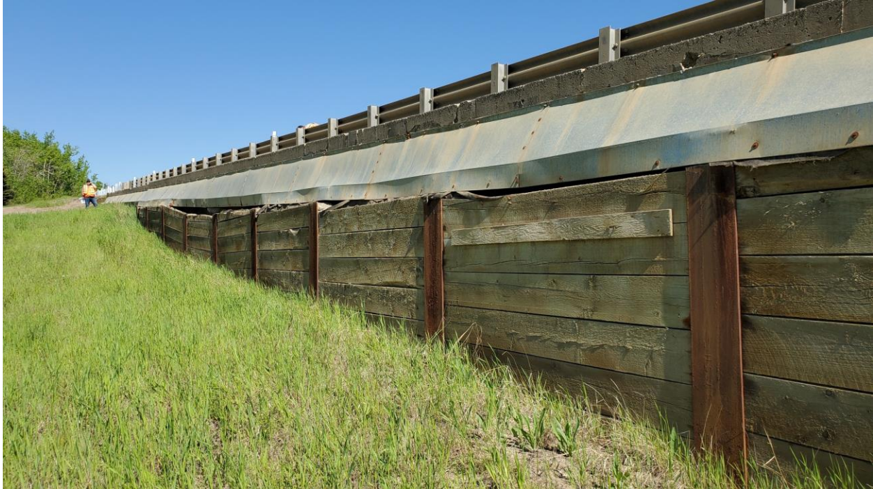
Photo 5 – Looking north at the displaced H-pile and timber lagging wall near the scarp at the north end of the wall.
