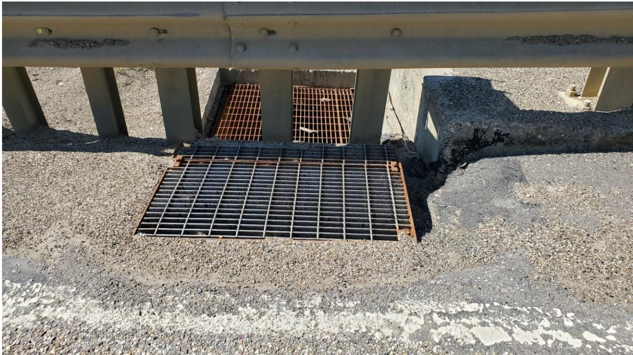
Photo 2 – Catch basin inlet at the south end of the wall leading to the elephant trunk downpipe.
