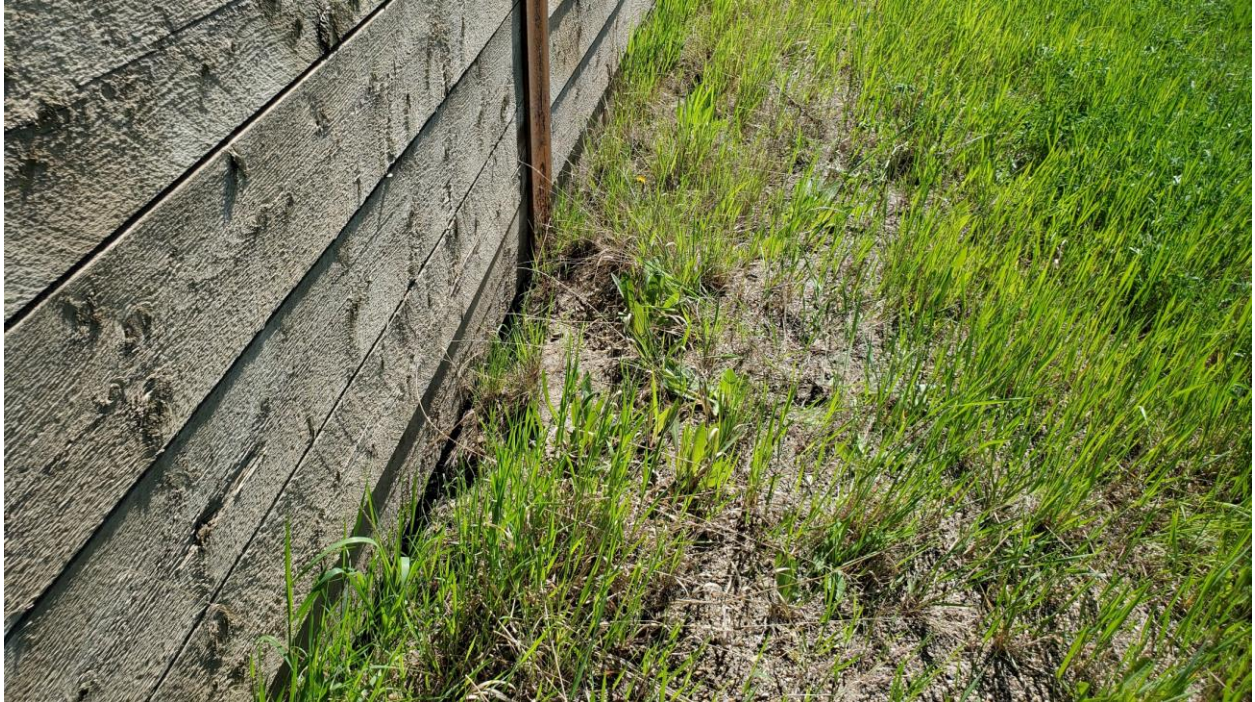
Photo 9 – The crack forming below the lagging wall at the south end where the soil is starting to pull away.
