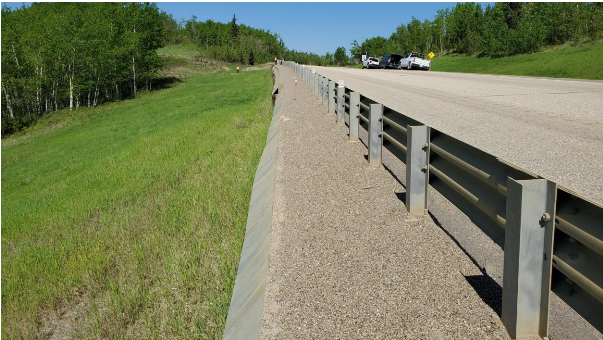
Photo 4 – Looking northwest at repaired and overlaid asphalt surface. A new bridge rail was installed during construction and damaged flashing at about the center of the wall noted previously has been repaired.
