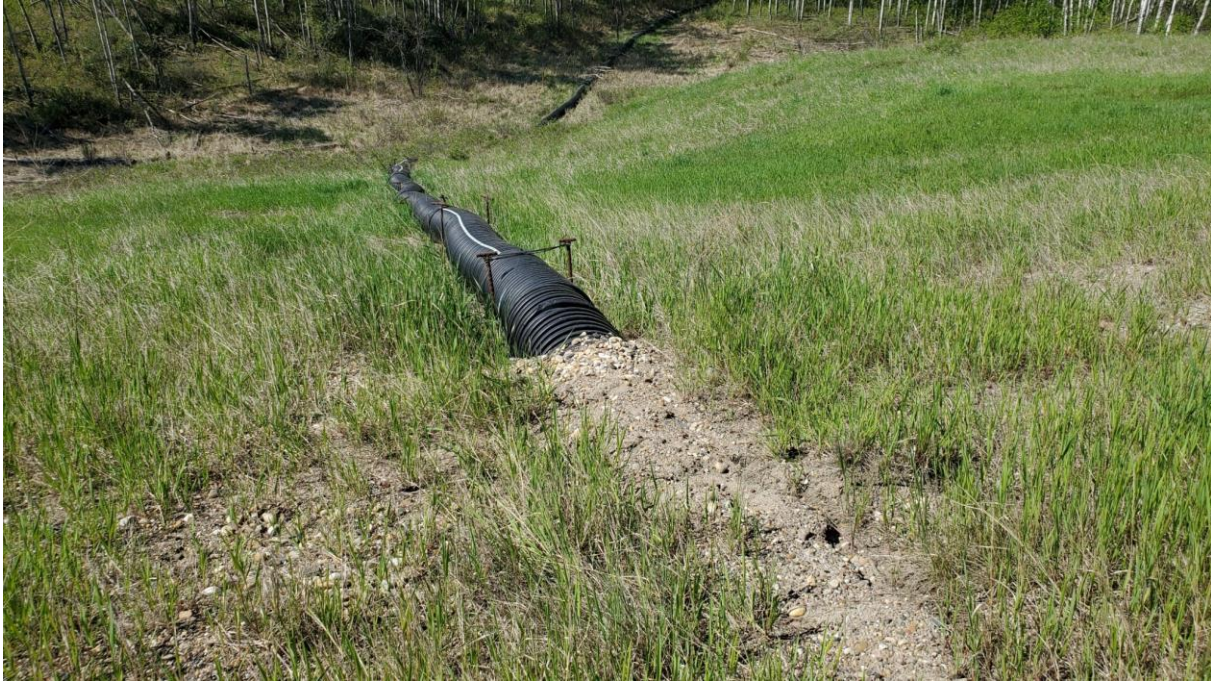
Photo 3 – Looking downslope at “elephant trunk” drain pipe. There is some erosion forming in mower ruts on the left (south) side of the drain pipe.
