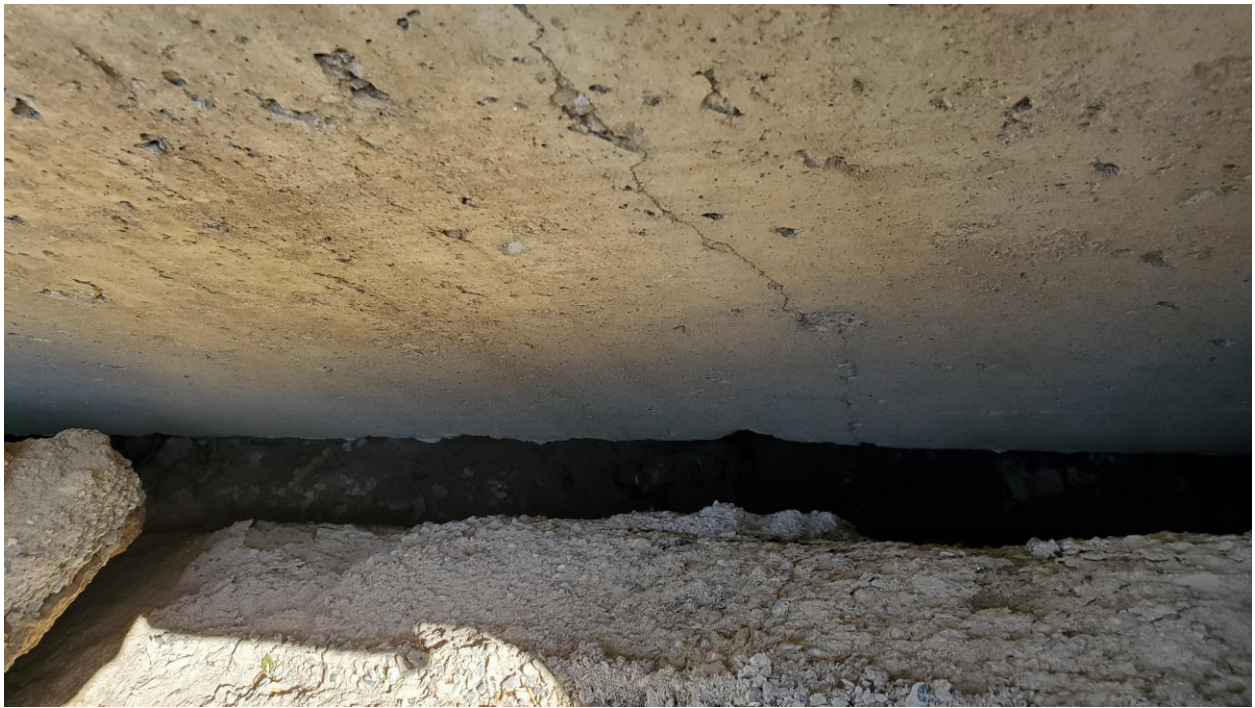
Photo 10 – The void forming in front of and behind the cap beam as the lagging wall and grout backfill is displaced by slope movement.
