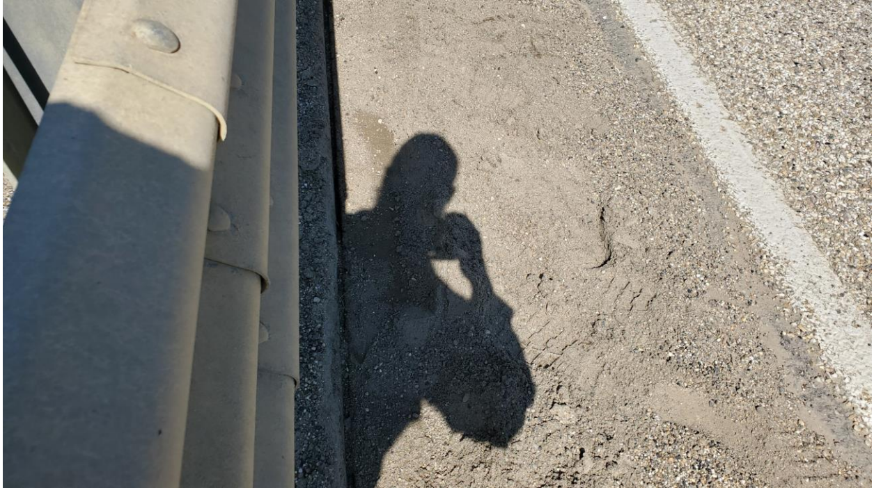
Photo 7 – Looking at the crack that is opening up again between the cap beam and asphalt.
