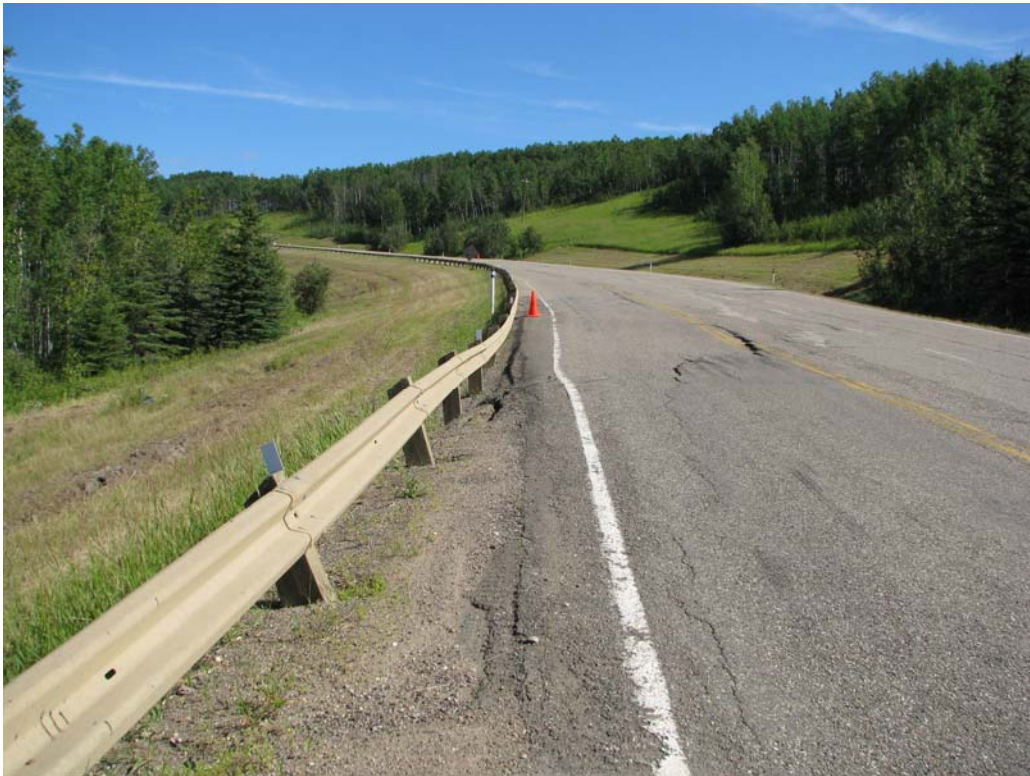
Photo 1 - View of asphalt patch and cracks on Highway 35:08, looking northeast.
