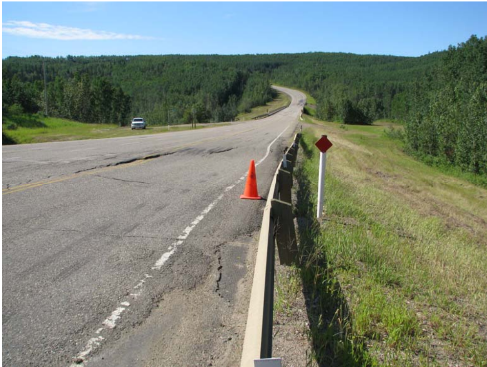
Photo 3 – Fresh Cracks beyond and along the ACP patch, looking southwest
