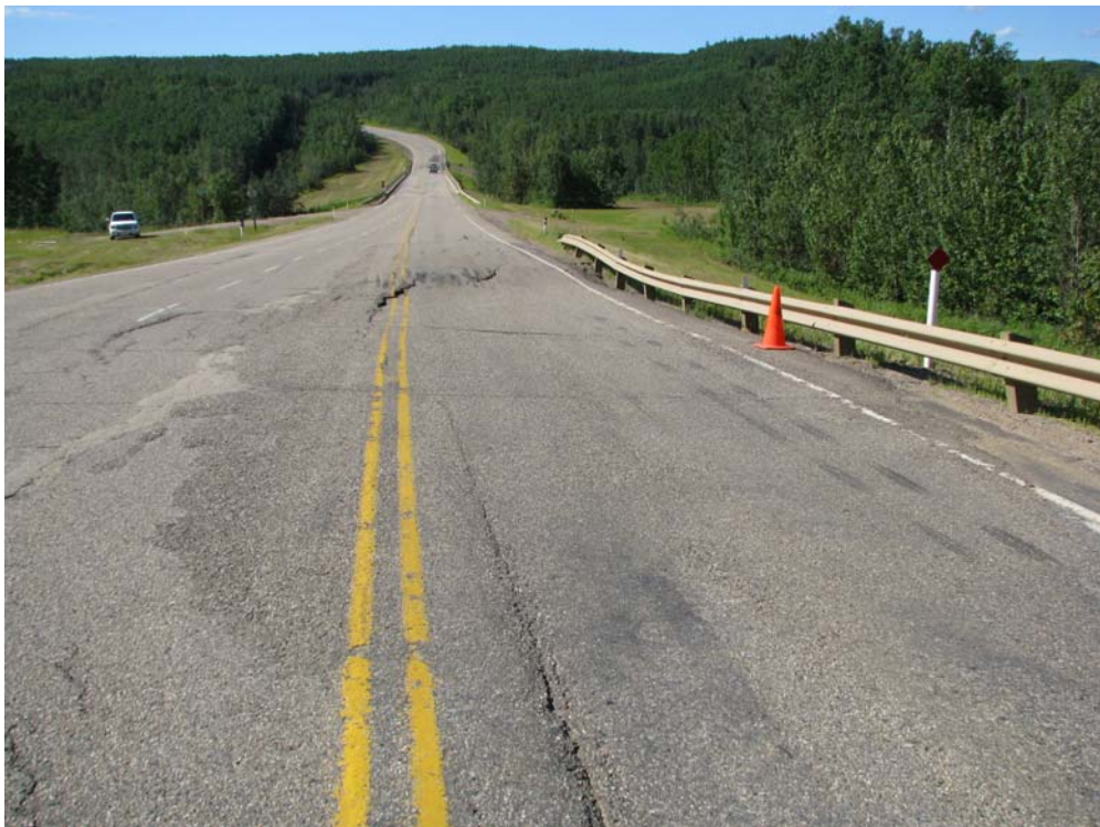
Photo 4 – Additional cracking along the ACP patch, looking southwest.
