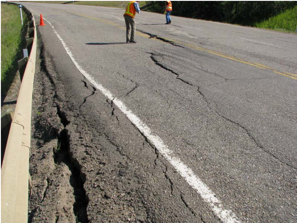
Photo 2 – Fresh Pavement cracks through ACP patch and near guard rail looking northeast.
