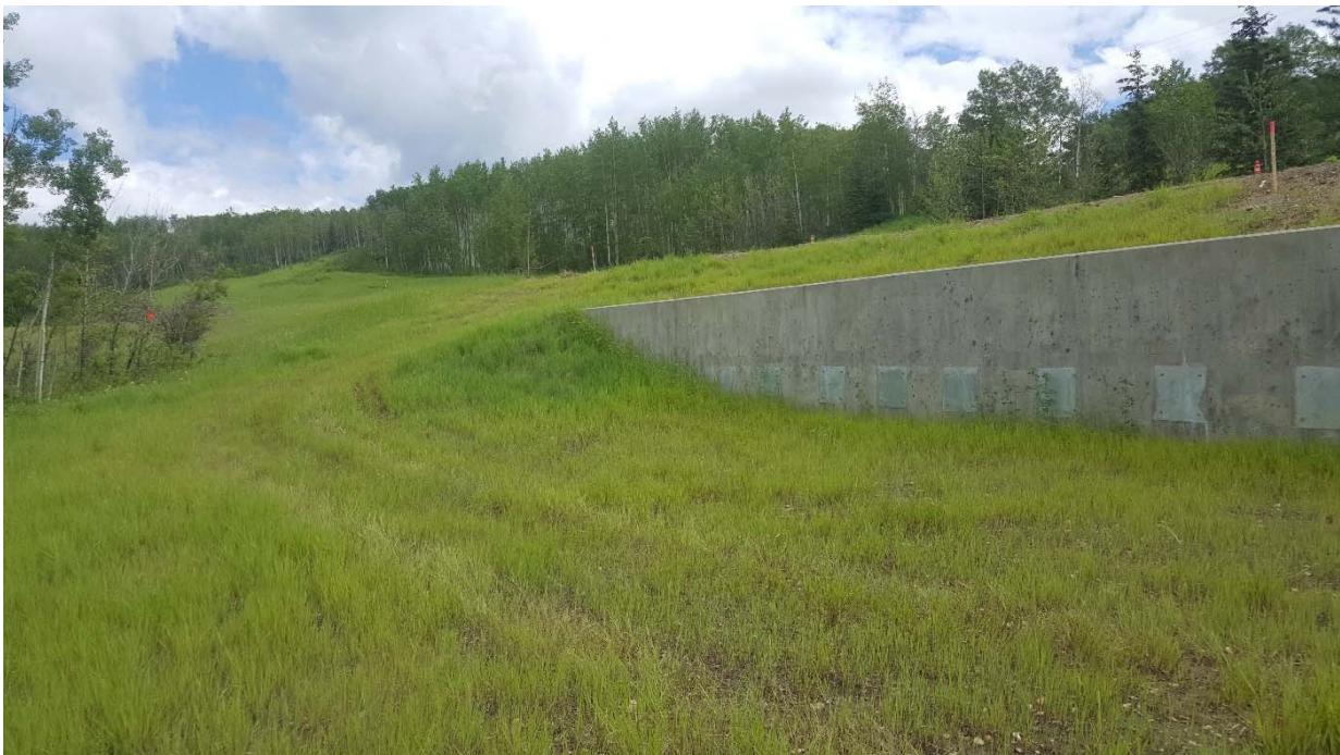
Photo 2 – Looking northeast at north end of the pile wall. Note the plates along the bottom of the water covering the sleeves for future tie-back installation, if required.
