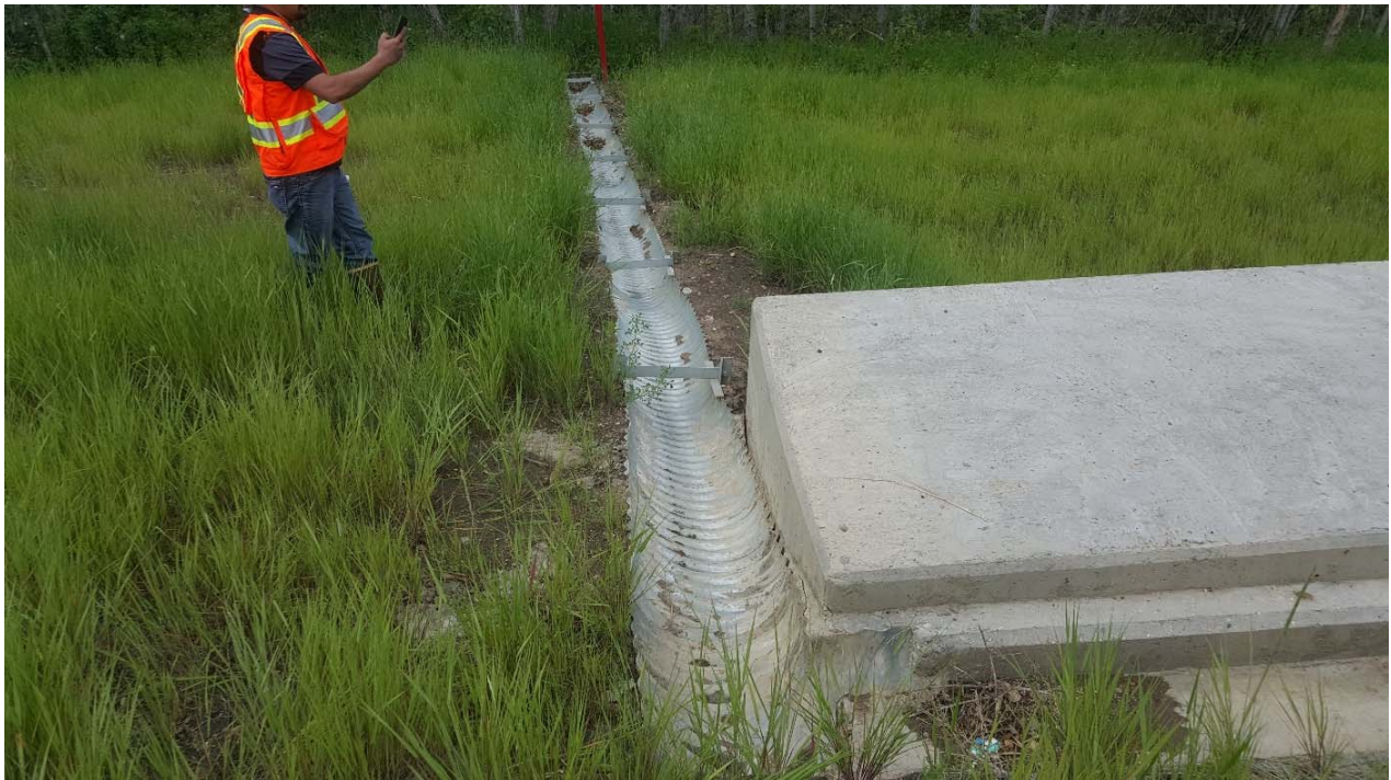
Photo 4 – Looking west along half-culvert down drain at the south end of the water.
