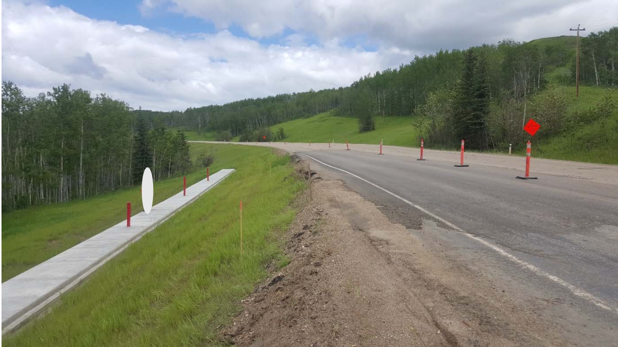
Photo 1 – Looking north along rebuilt slope with pile wall. Guardrail was removed as part of the milling and overlay contract underway on Highway 35.
