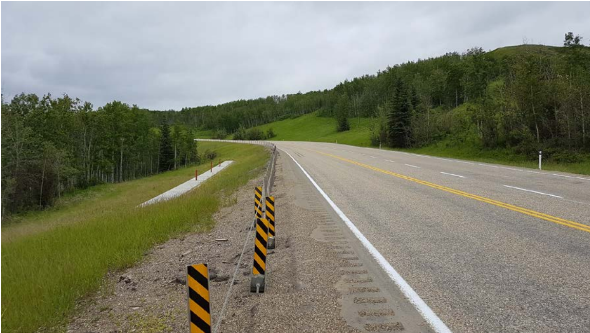
Photo 1 – Looking north along rebuilt slope with pile wall. Guardrail was removed as part of the milling and overlay on Highway 35 and replaced with a high-tension cable barrier.
