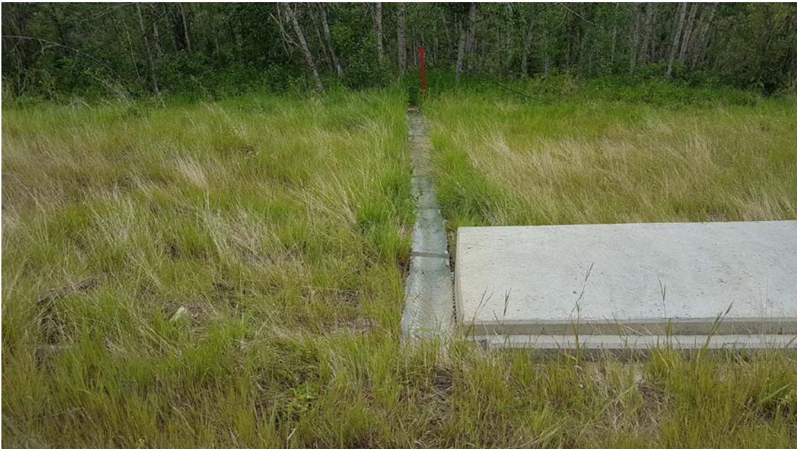
Photo 4 – Looking west along half-culvert down drain at the south end of the wall.
