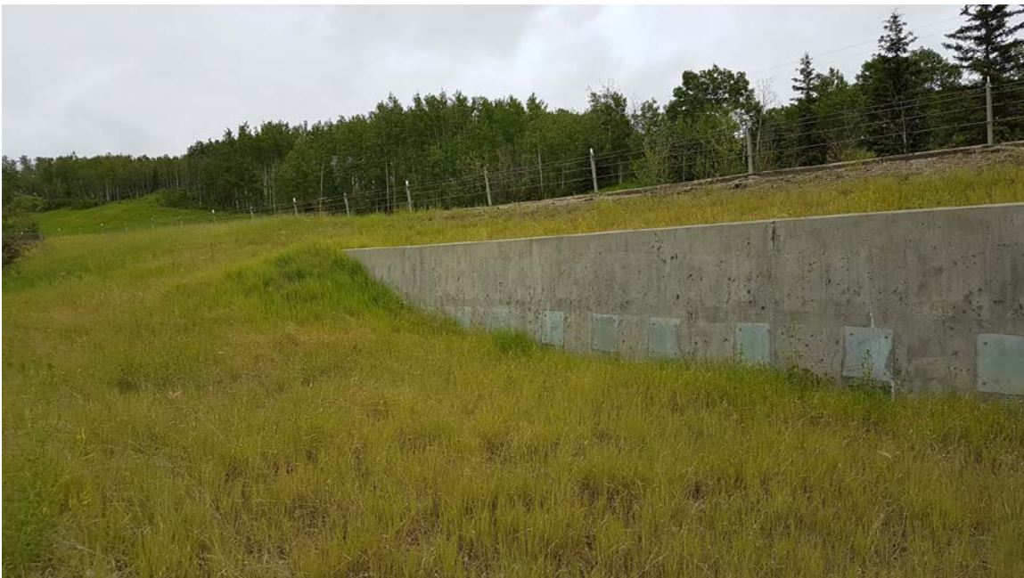
Photo 2 – Looking northeast at north end of the pile wall. Note the plates along the bottom of the wall covering the sleeves for future tie-back installation, if required.
