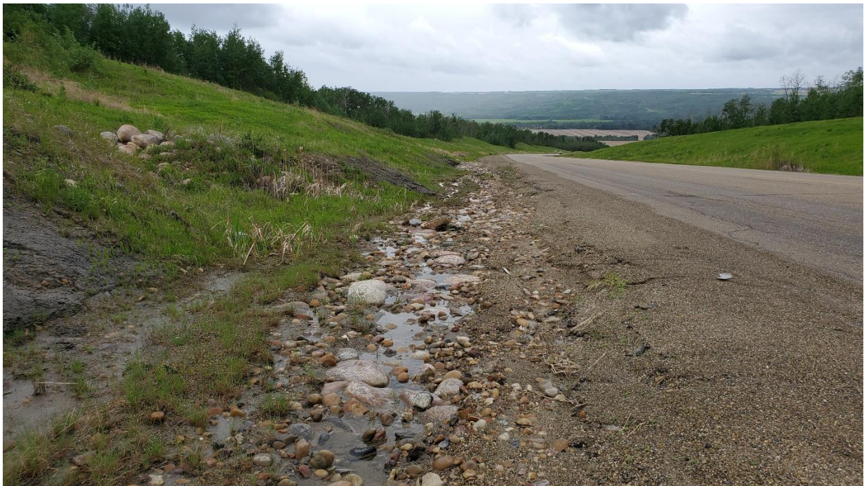
Photo 4 – Looking west at the toe of Slump B.
