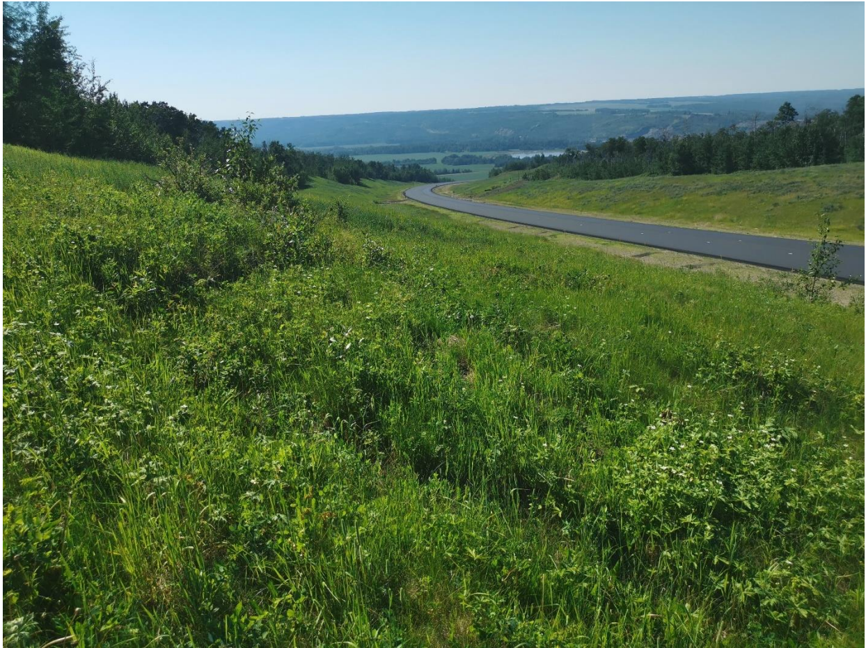
Photo 3 – Looking west at crest of Slump D
