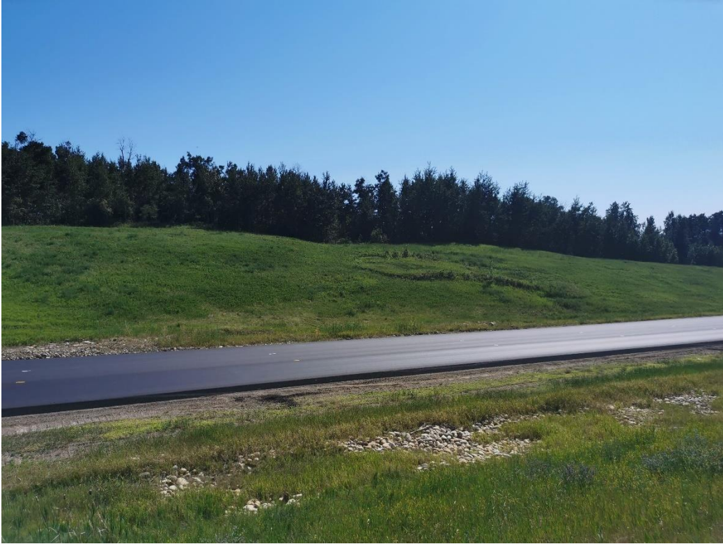
Photo 6: Looking southwest at Slump D.
