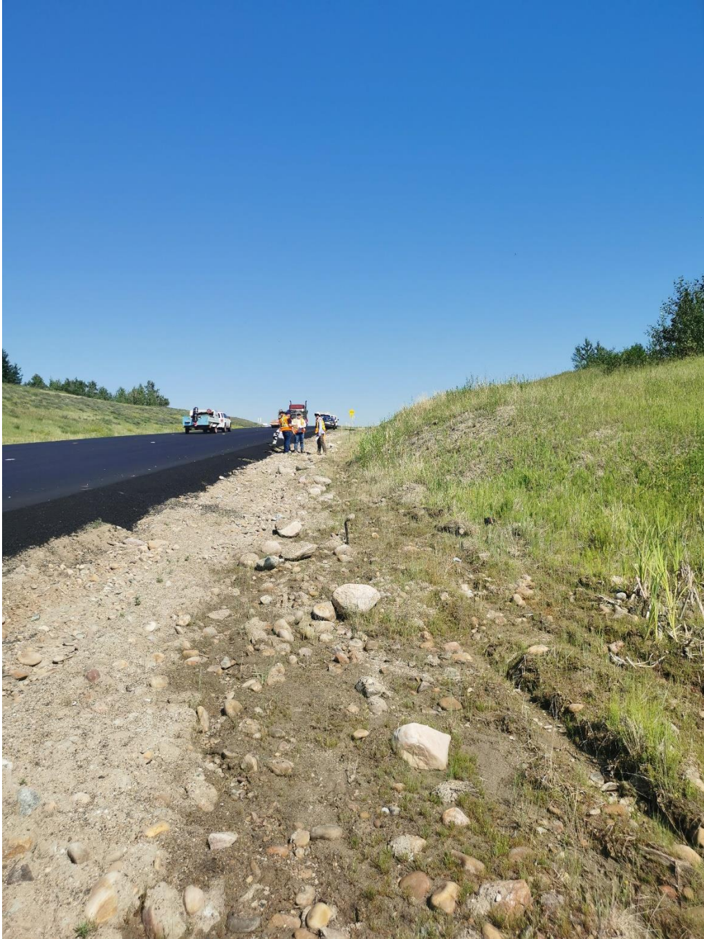
Photo 1 – Looking east at toes of Slumps B and A which were excavated in 2019 to improve ditch flow with the material placed back onto the slide masses.
