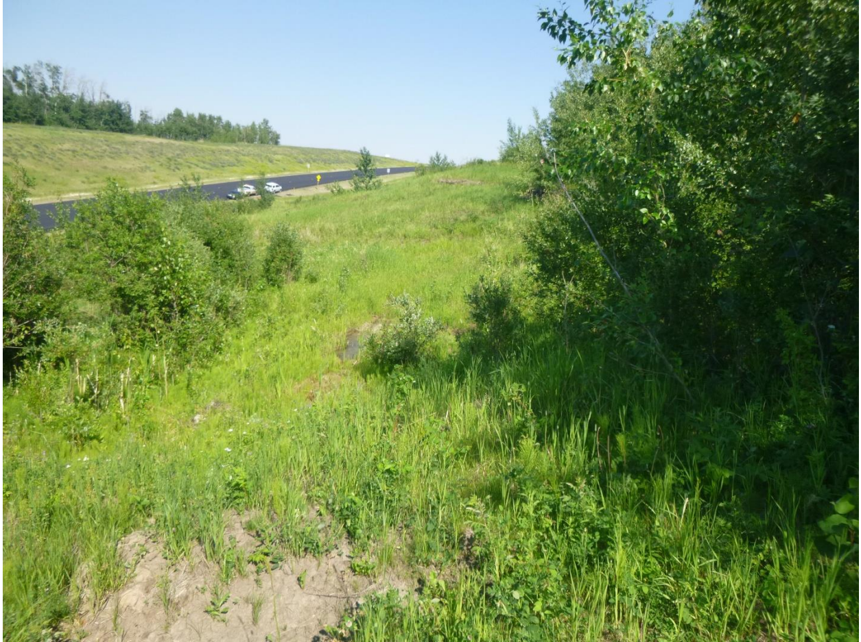
Photo 2 – Looking southeast at the top of Slump B. Disturbances from 2019 regrading becoming vegetated.
