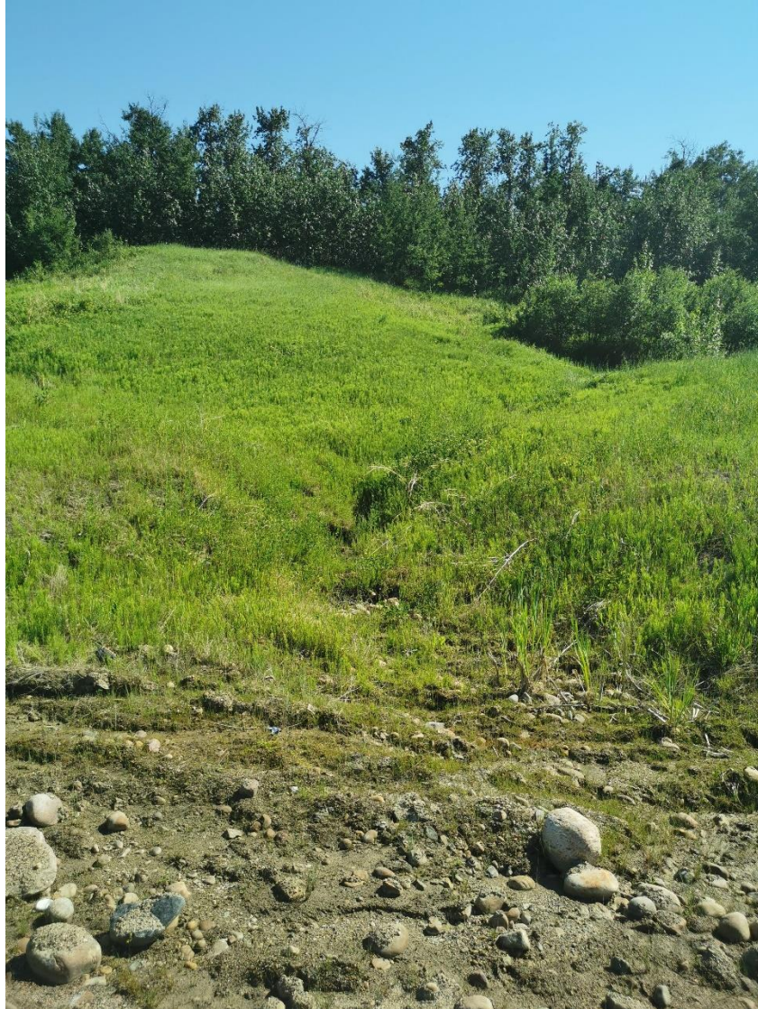
Photo 5: Recent grading (2019) of lower portion of the slope at toe of Slump B becoming vegetated.
