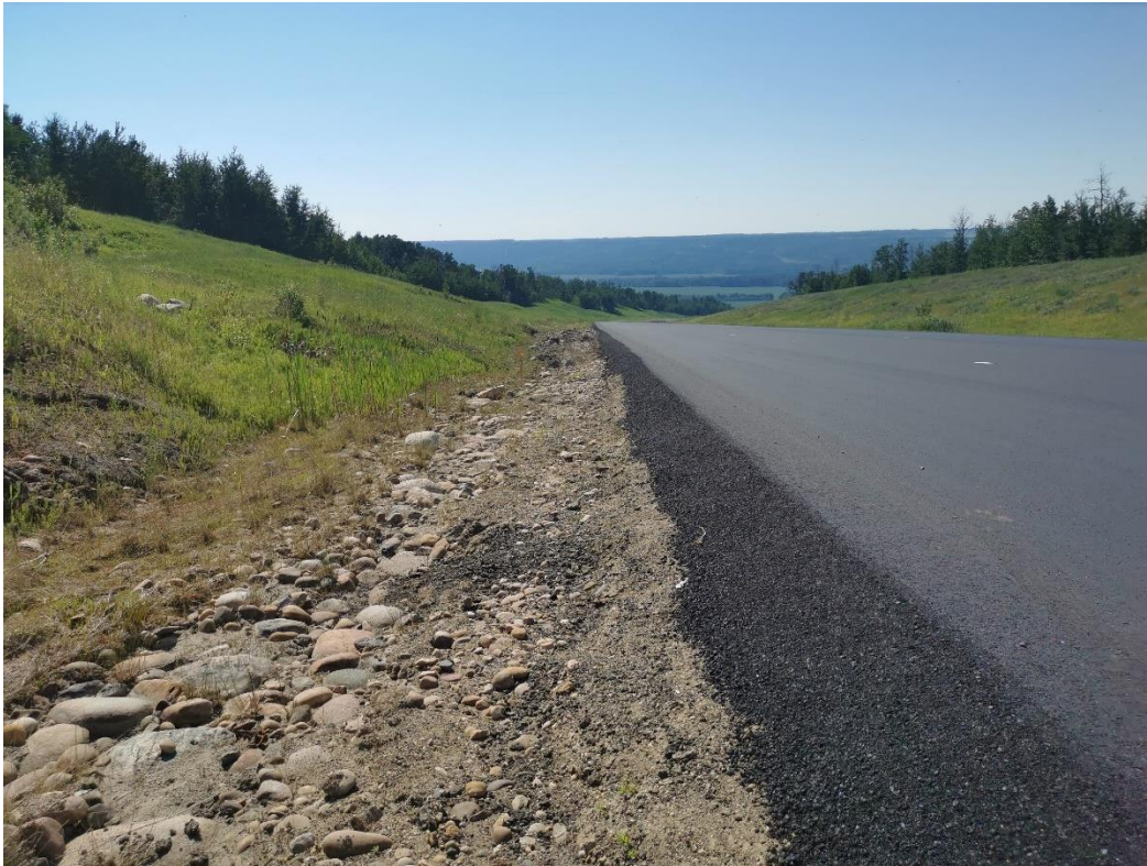
Photo 4 – Looking west at the toe of Slump B.
