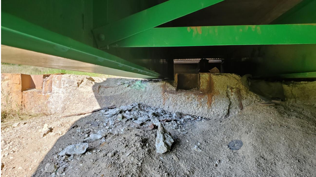
Photo 3 – Looking towards the West Abutment where portions of the old foundation concrete was removed to allow movement of the girders between the West Abutment and Abutment 1.
