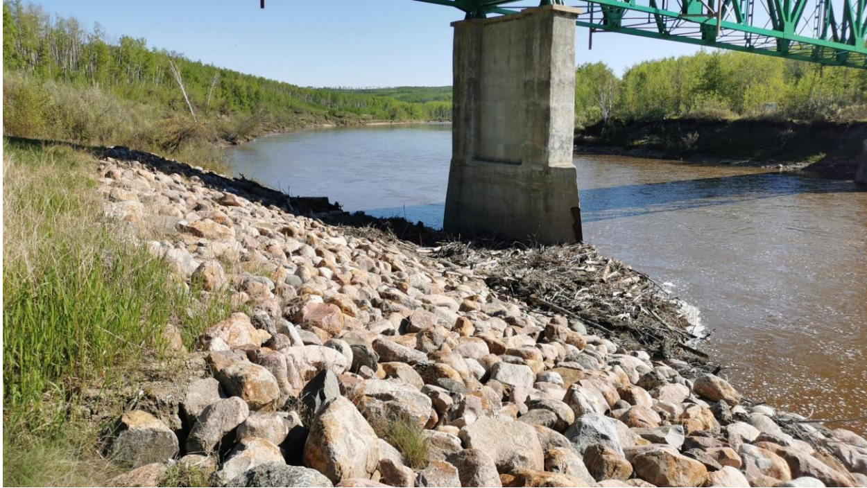
Photo 11 – Looking north at accumulated tree debris against Pier 2.
