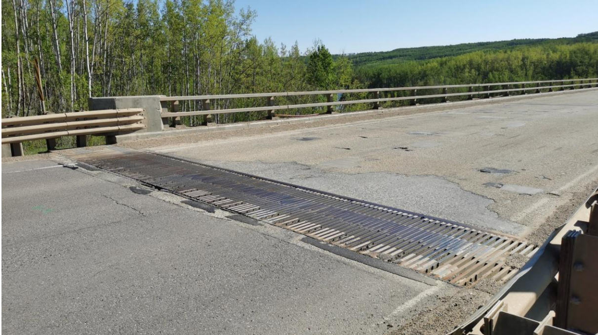
Photo 1 – Looking southeast at crack pattern forming at the west abutment expansion joint. This was overlaid or patched since 2020.
