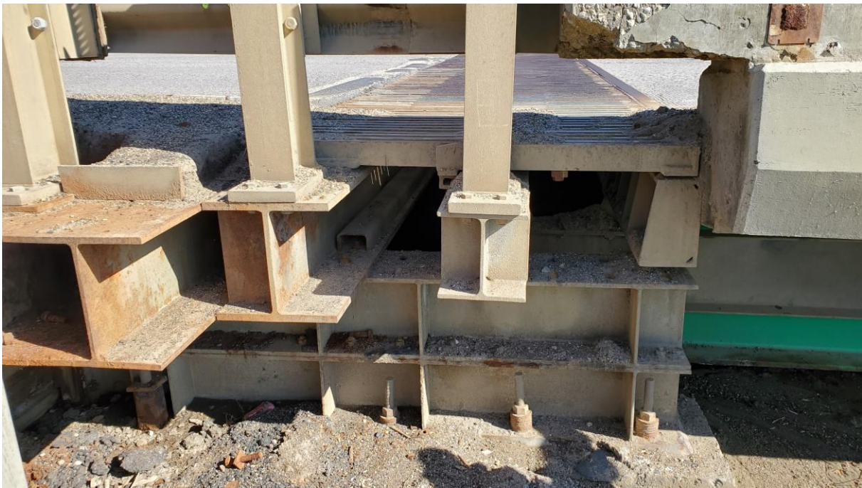
Photo 2 – Looking north at west bridge abutment. Distance between angle iron and concrete of bridge deck was 2.42 m (2.60 m in 2020, 2.69 m in 2019, 2.72 m in 2018, 2.82 m in 2017). The two I-beams at the edge of the wingwall are the remainder of the 5 installed in 2000.
