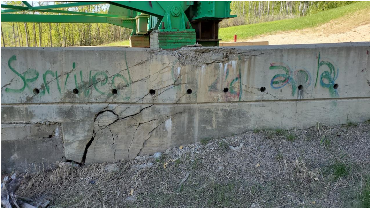
Photo 8 – Looking south at Pier 1 wingwall at arc-shaped compression crack pattern in foundation. Left-hand portion of foundation is pile supported; right-hand is on-grade. Crack at the base is 40 mm in width.
