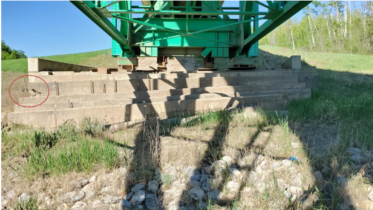
Photo 9 – Looking west at Pier 1 foundation which is tilted downward to the south. The angle from horizontal was 4° at the top and 7° at the bottom stage. Concrete is starting to crack and spall in circled area.
