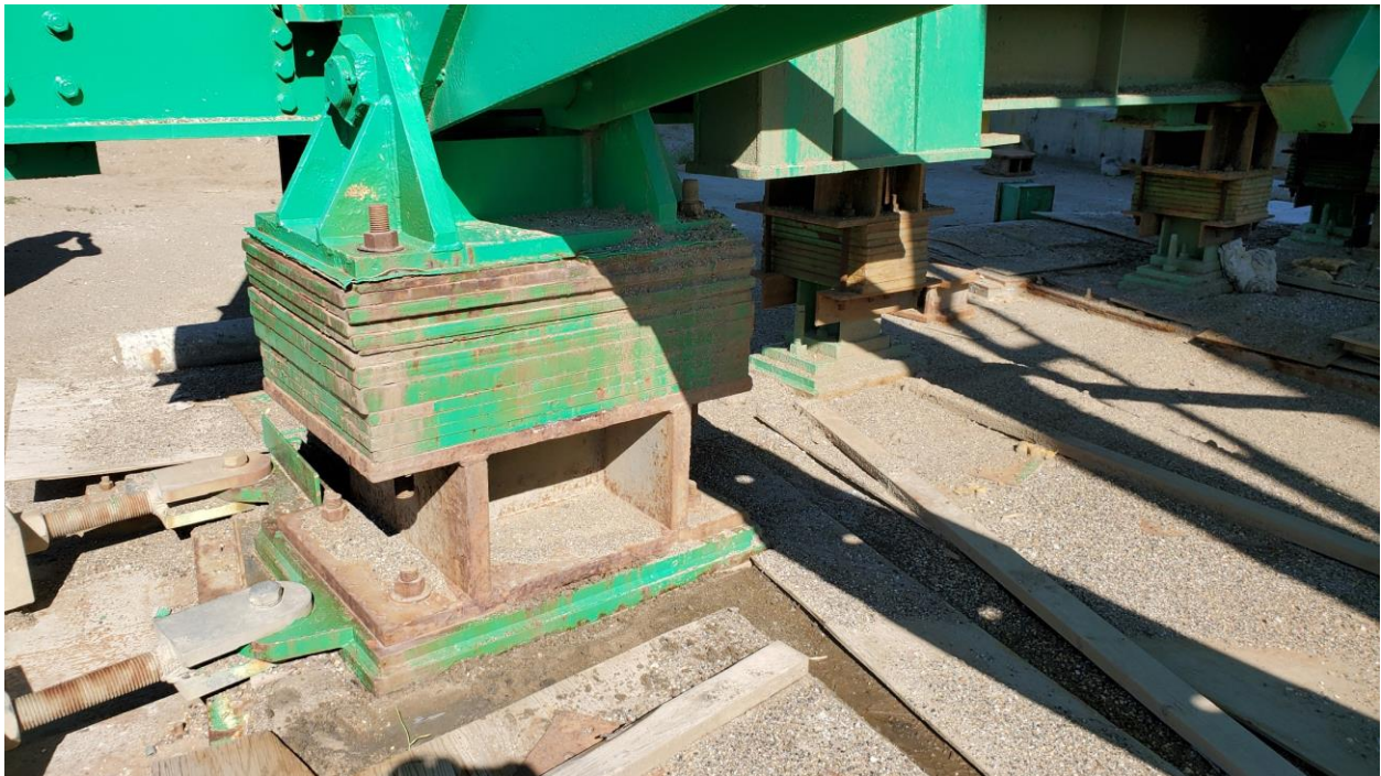
Photo 6 – Shims (increased to 0.84 m from 0.755 m) under rocker bearings at Pier 1: remained 0.84 m at the south bearing plate (left-most) and 0.76 m at the north bearing plate (right-most).
