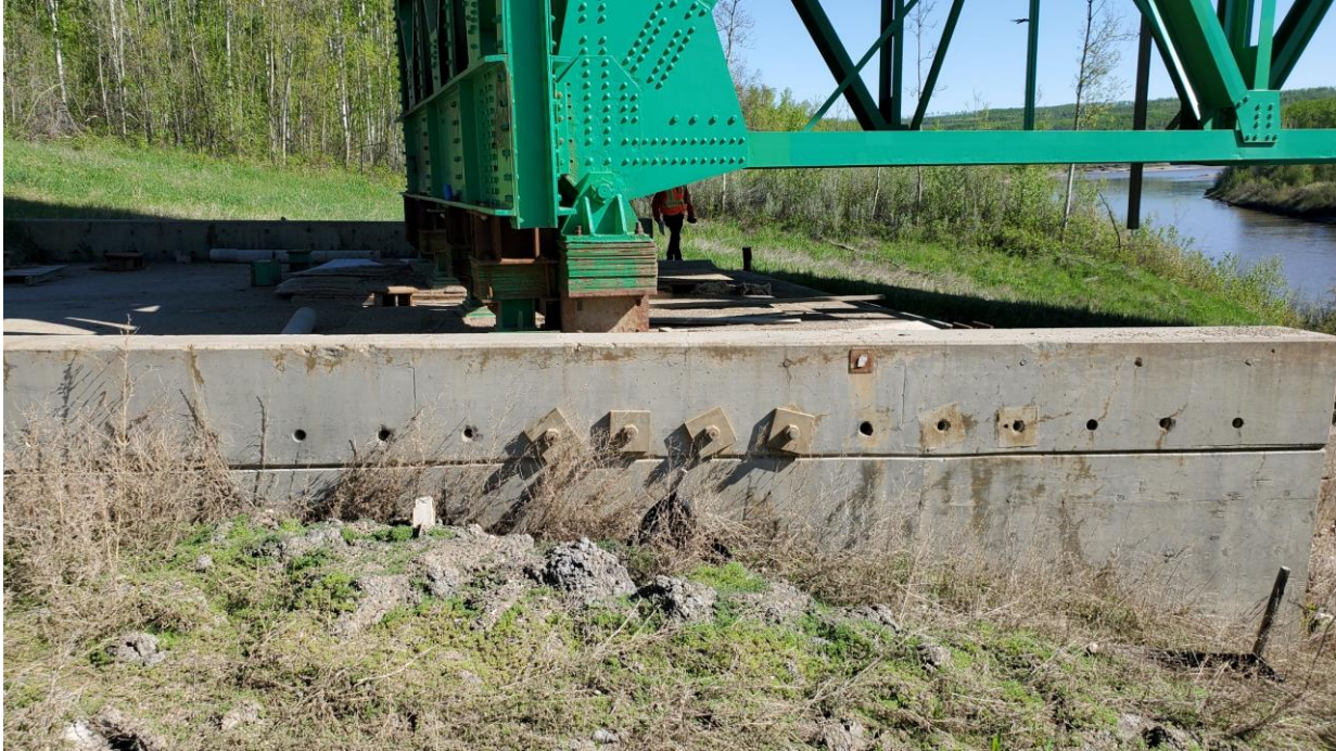
Photo 7 – Looking north at Pier 1 wingwall where bolts have been moved over 1.18 m since construction in 2000.
