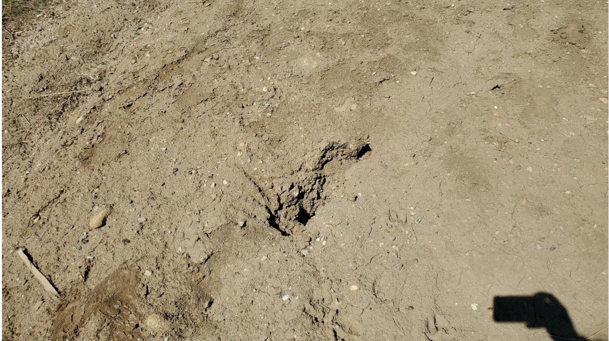
Photo 5: Shallow voids on headslope below Abutment 1. The voids, now combined, showed up in 2021 and the cause is unknown.
