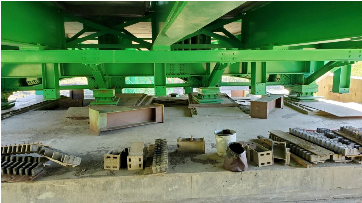
Photo 4: Sliding configuration at Abutment 1. Movement at right-most (south) bearing plate in June 2020 was 35 mm since May 14, 2020, and 121 mm since June 10, 2019.
