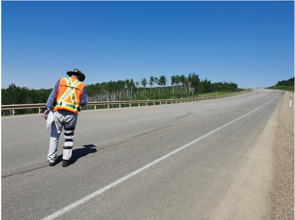
Photo 4 – Looking northeast at fresh cracks which are part of the main graben block movement between Sta. 0+600 and 0+800.
