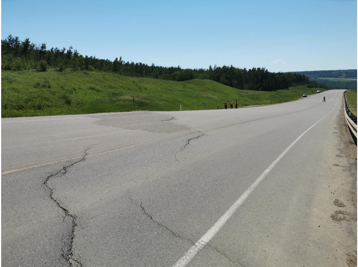
Photo 5 – Looking south at cracks at northeast end of main graben block at Sta. 0+600.
