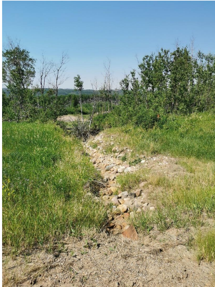
Photo 1 – Erosion gully at outlet of culvert at about Sta. 0+450.
