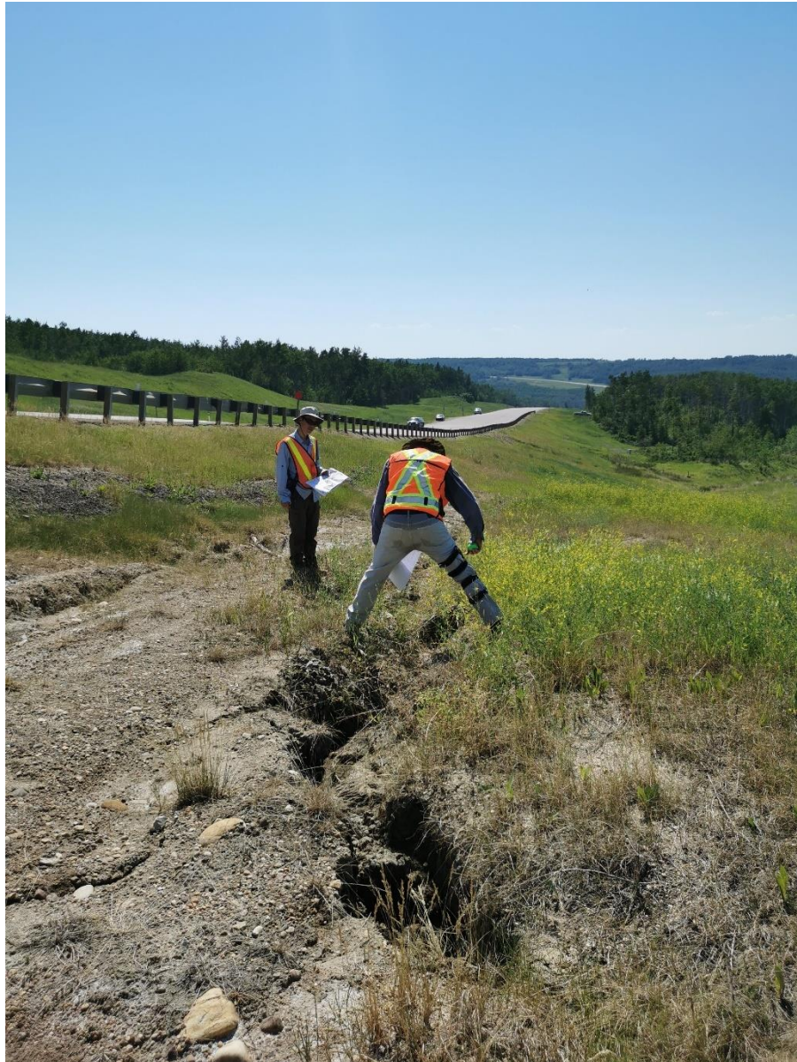
Photo 2 – Looking southeast along erosion gully near Sta. 0+550. Note windrow of milled materials on sideslope of highway.
