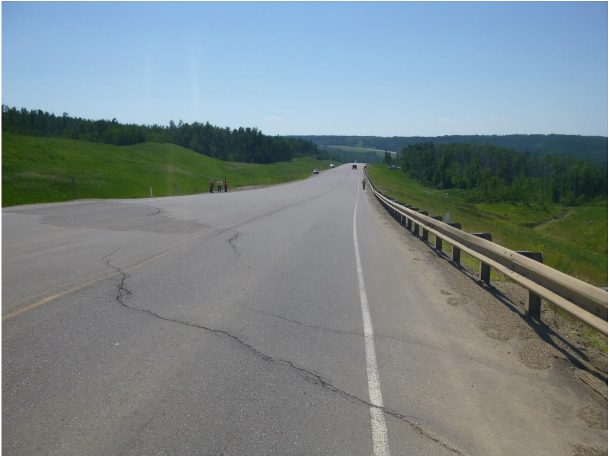
Photo 3 – Looking southwest over the main sag (graben) area extending from Sta. 0+600 to 0+800.
