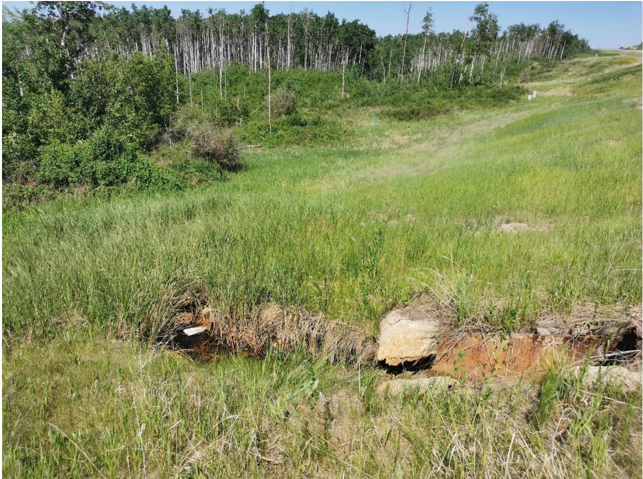
Photo 7 – Developing erosion bowl at outlet of culvert at about Sta. 0+800.
