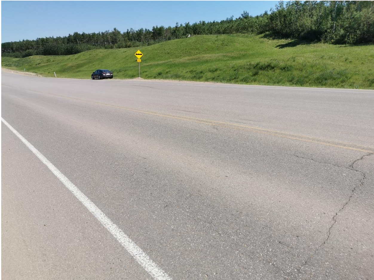
Photo 6 – Looking east where previous cracks were paved over on the southwest end around Sta. 0+800.
