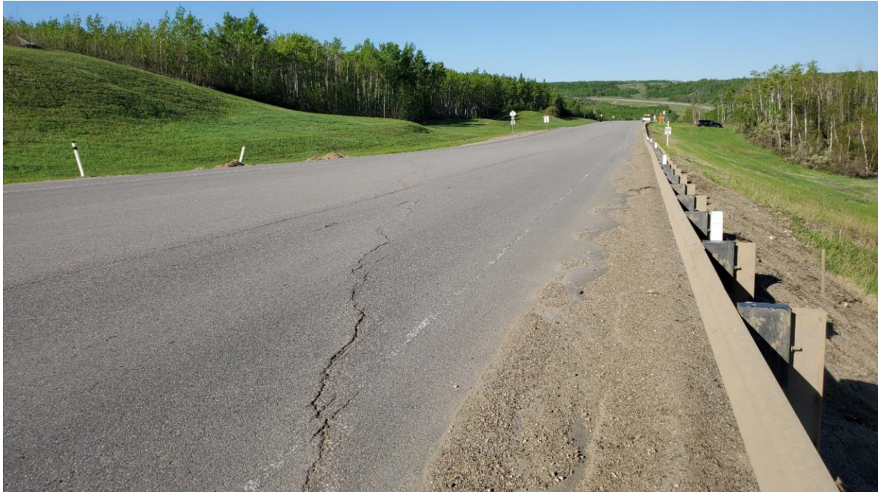
Photo 6 – Looking south at cracks at northeast end of main graben block at Sta. 0+600.
