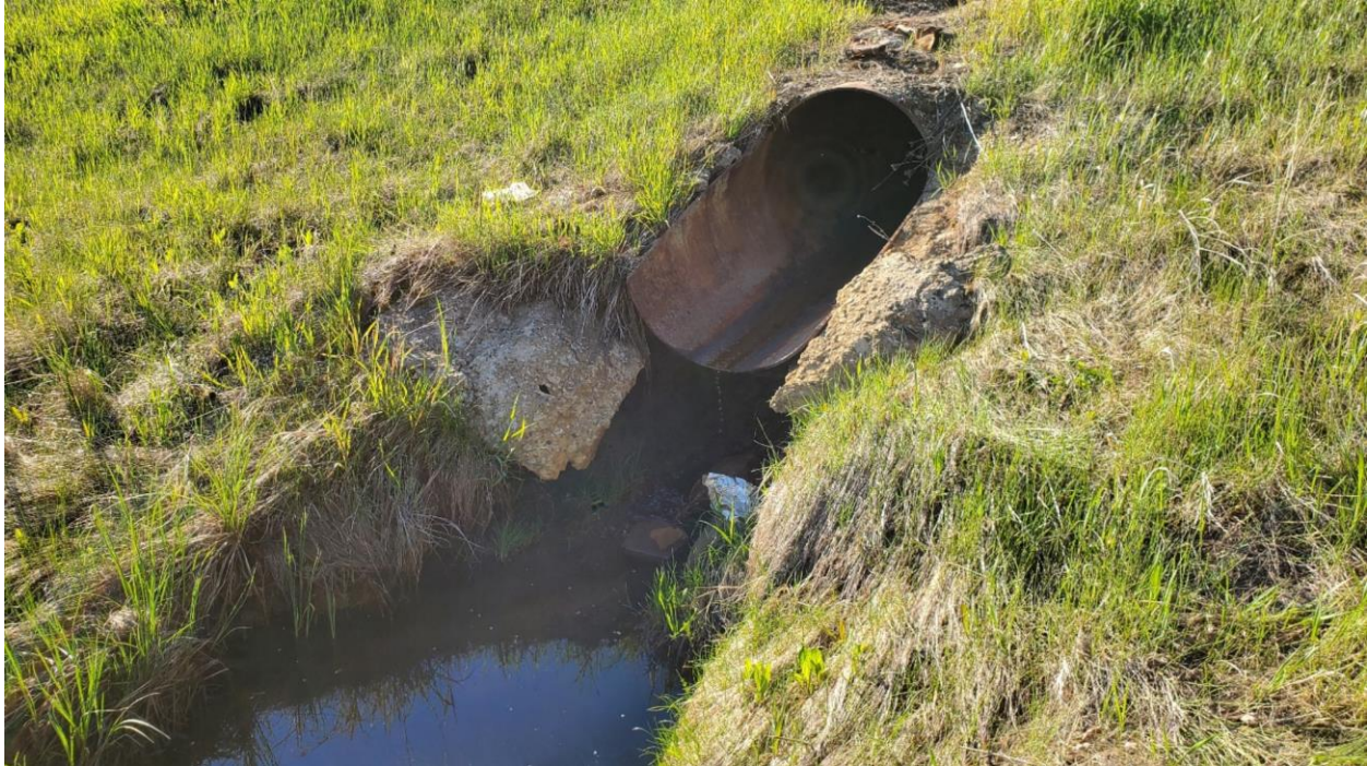
Photo 8 – Developing erosion bowl at outlet of culvert at about Sta. 0+800.
