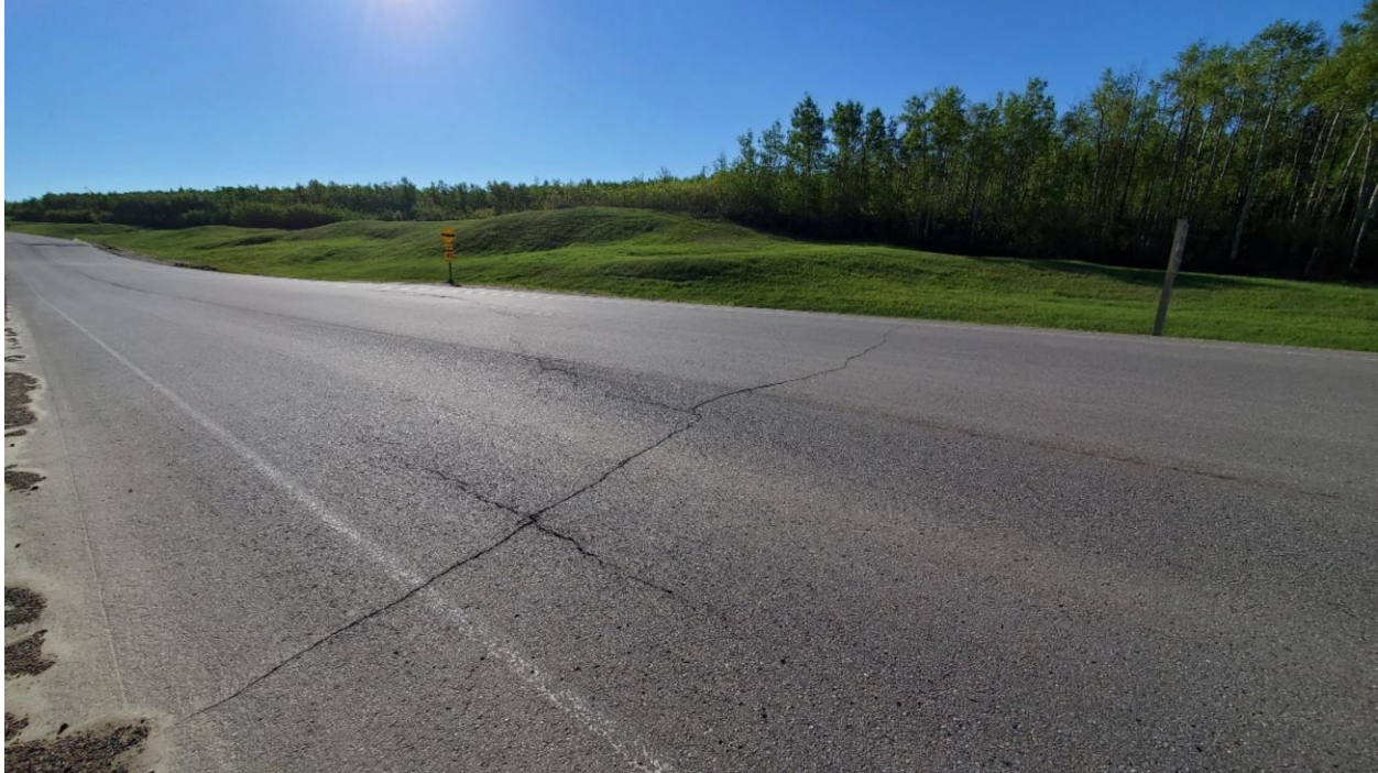
Photo 7 – Looking east at the cracks on the southwest end of the main graben.
