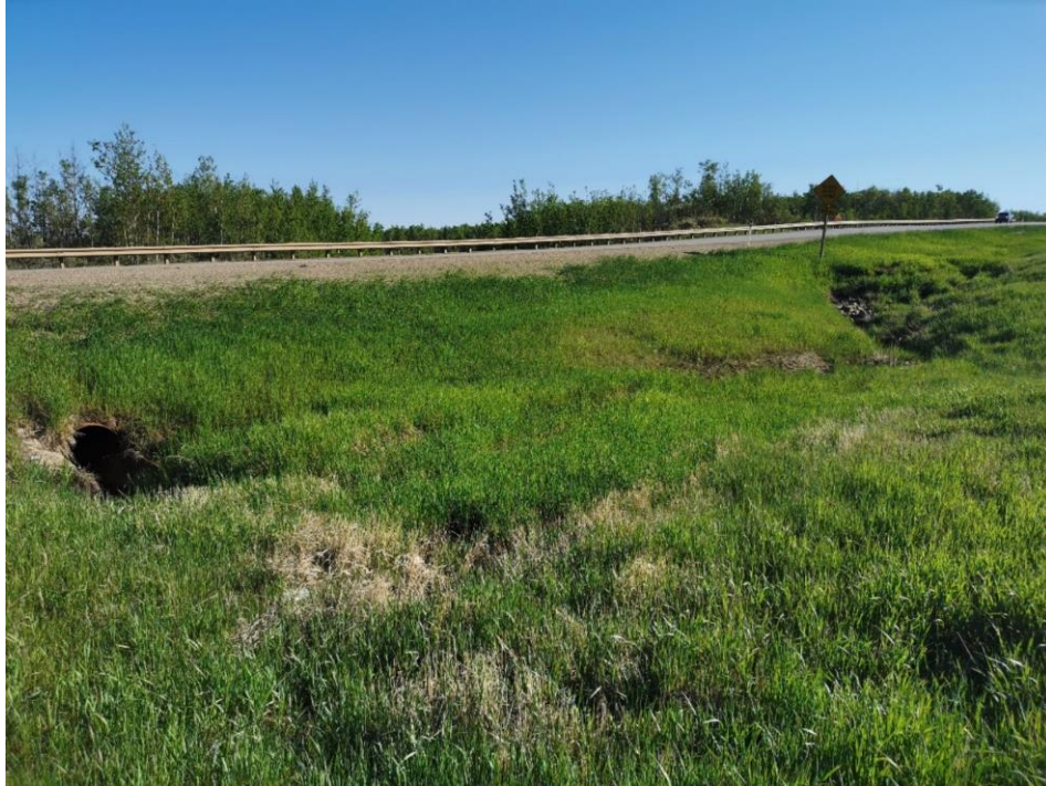
Photo 9: Erosion at the culvert inlet (left side) and scour bowl (right side) at Sta. 0+430 is starting to encroach towards the highway.
