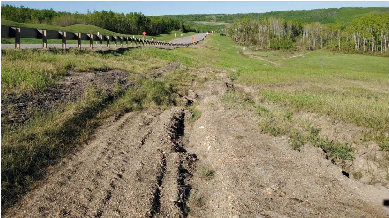
Photo 2 – Looking southeast along erosion gully near Sta. 0+550.
