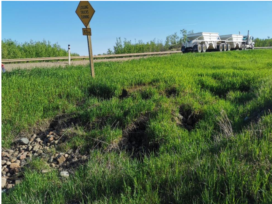
Photo 10: Scour bowl forming close to the edge of the highway at Sta 0+430.
