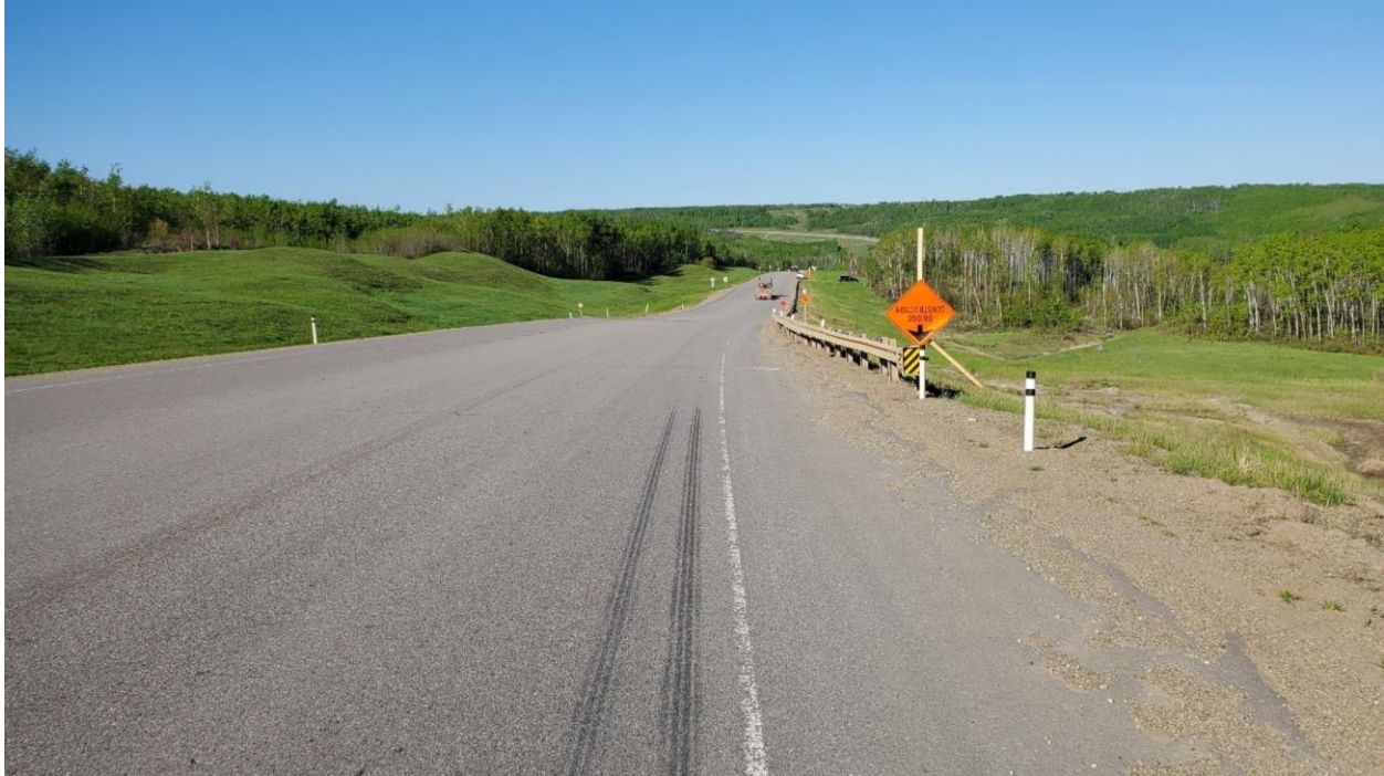
Photo 3 – Looking southwest over the main sag (graben) area extending from Sta. 0+600 to 0+800.
