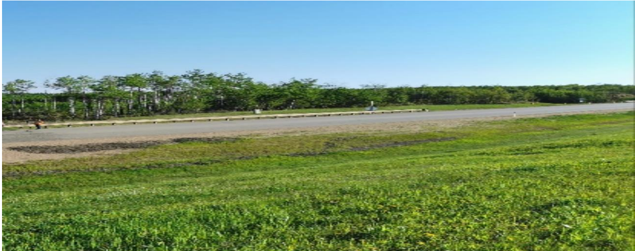
Photo 4 – Looking north at the main graben at about Sta. 0+600 where dips in the highway surface are starting to become re-established.
