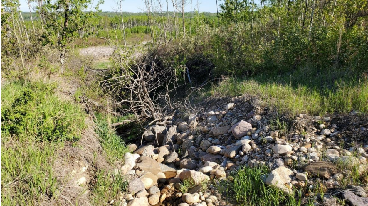
Photo 1 – Erosion gully at outlet of culvert at about Sta. 0+450.
