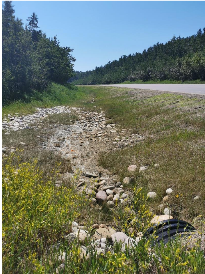
Photo 5 – Looking south along downslope ditch at sedimentation at inlet of 760 mm plastic culvert.
