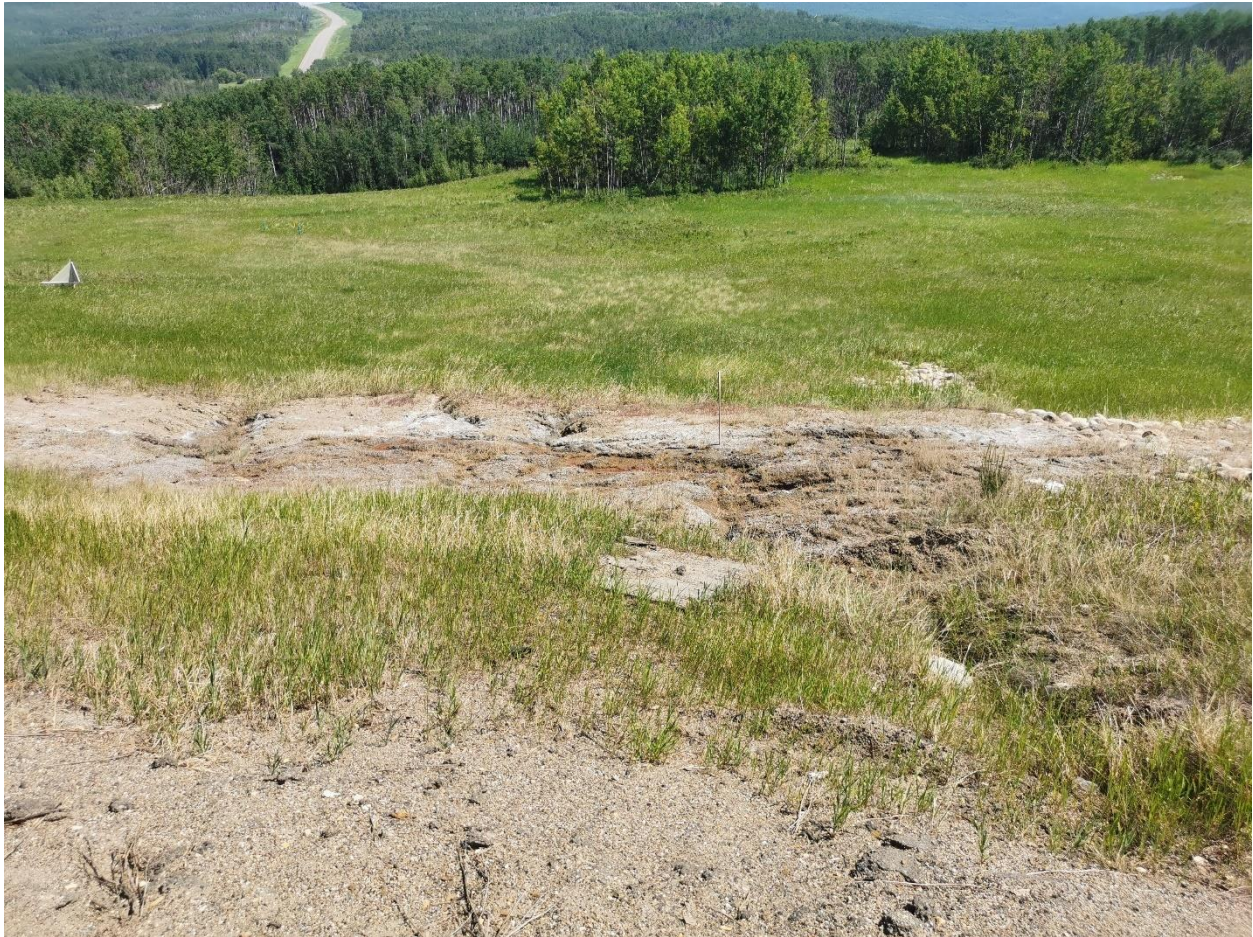
Photo 3 – Looking northeast at rilling on either side of riprap apron.
