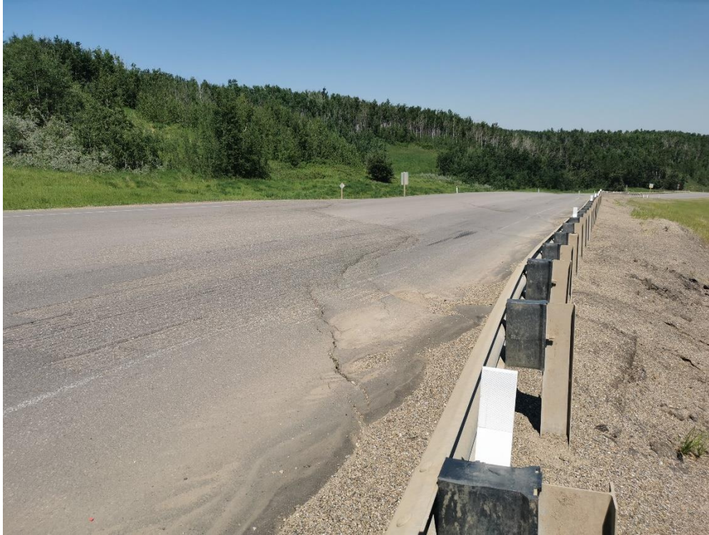
Photo 8 – Overlay and guardrail added in Fall 2020; cracking and differential becoming re-established through the ACP overlay.
