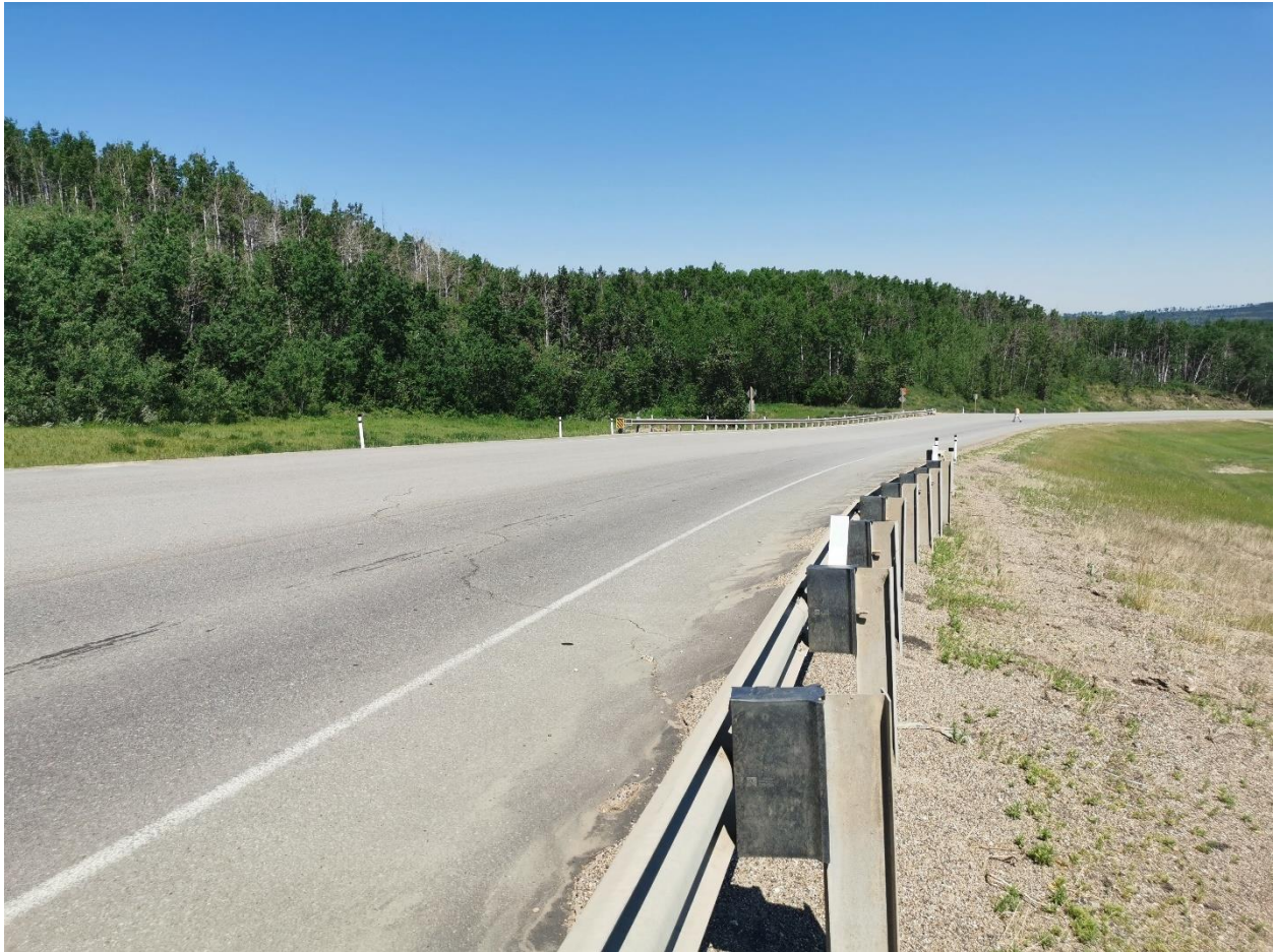
Photo 7 – Looking north at crack adjacent to the north end of the downslope guardrail.
