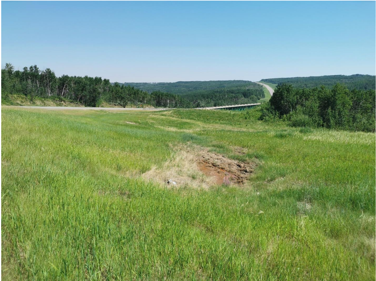
Photo 1 – Looking north at seepage on downslope side of highway at the north end of the site.
