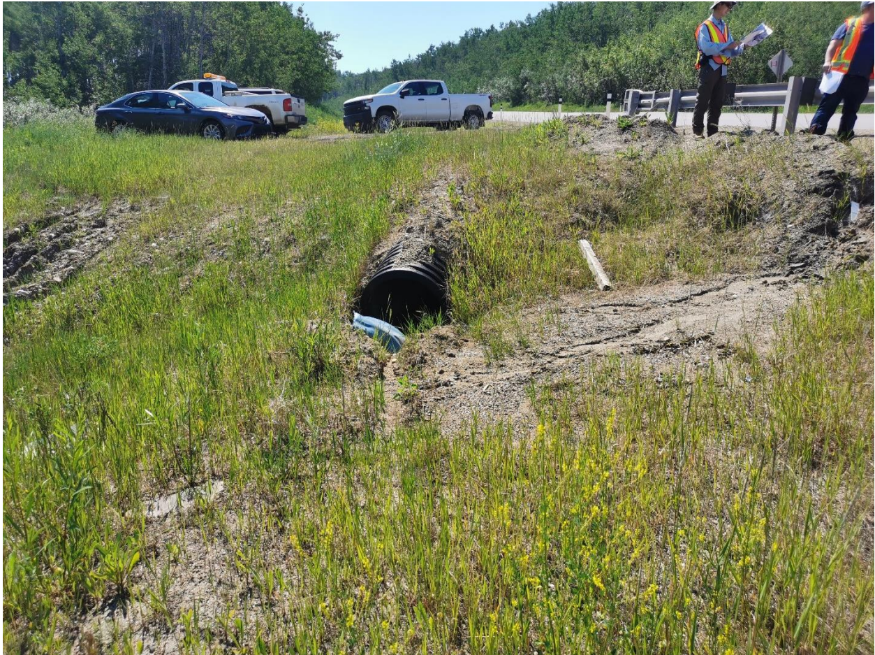
Photo 6 – Looking south at 760 mm culvert joint separation.
