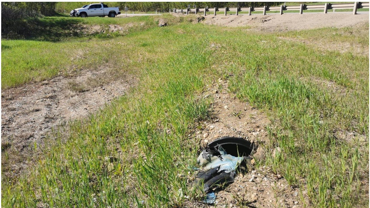
Photo 6 – Looking at 760 mm culvert joint separation.
