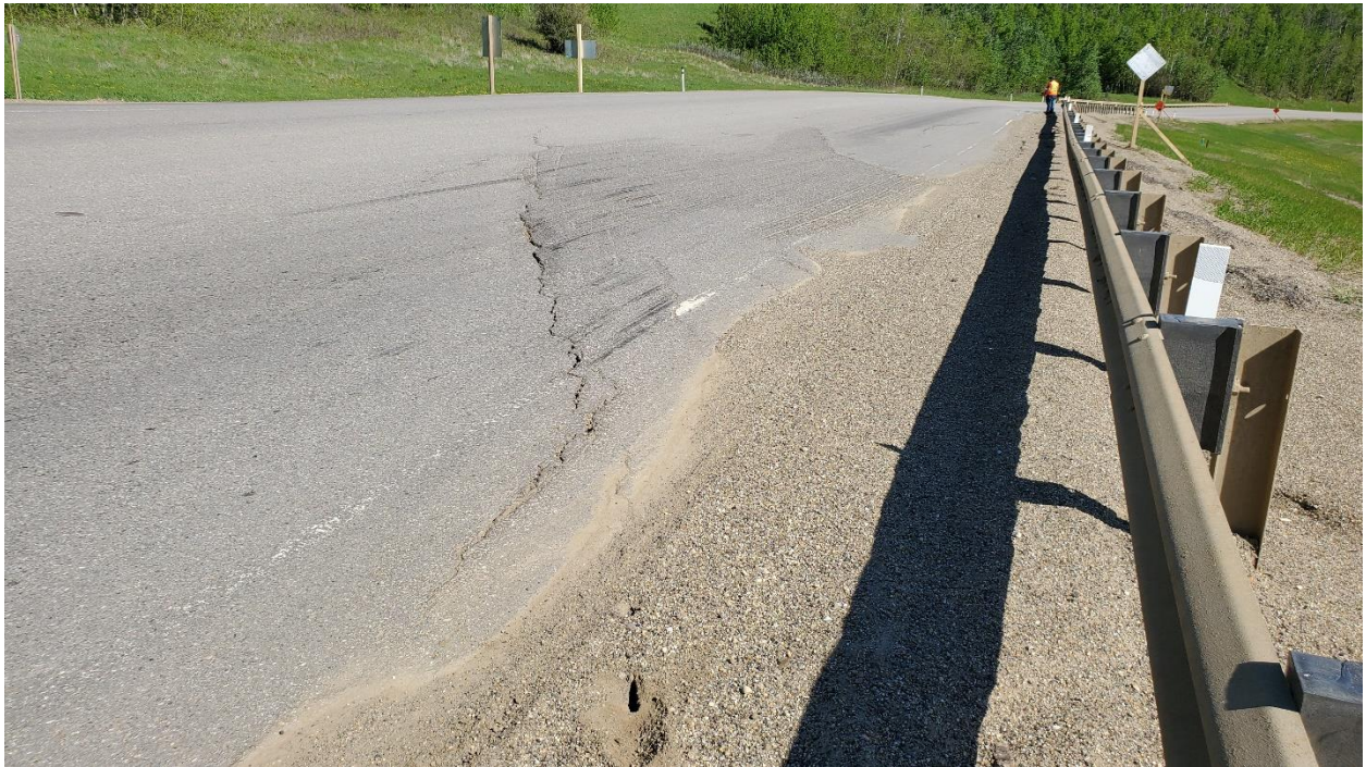
Photo 8 – Cracks across highway at south end of site.
