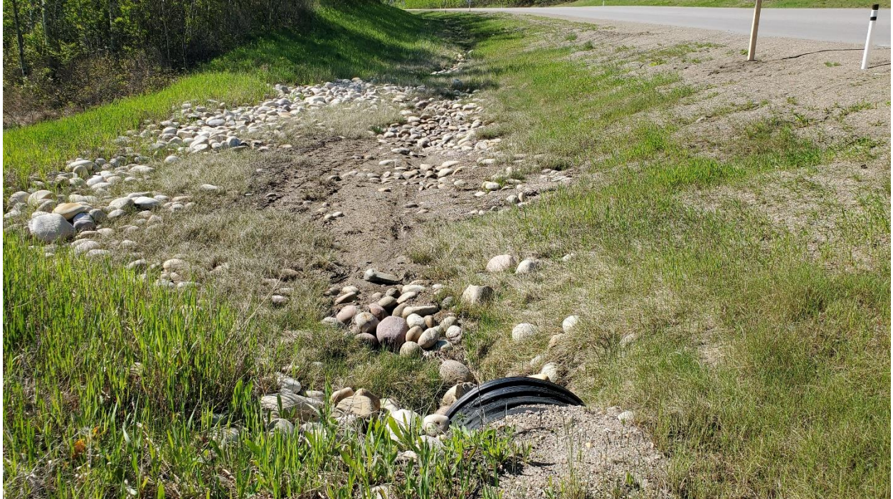
Photo 5 – Looking south along downslope ditch at sedimentation at inlet of 760 mm plastic culvert.
