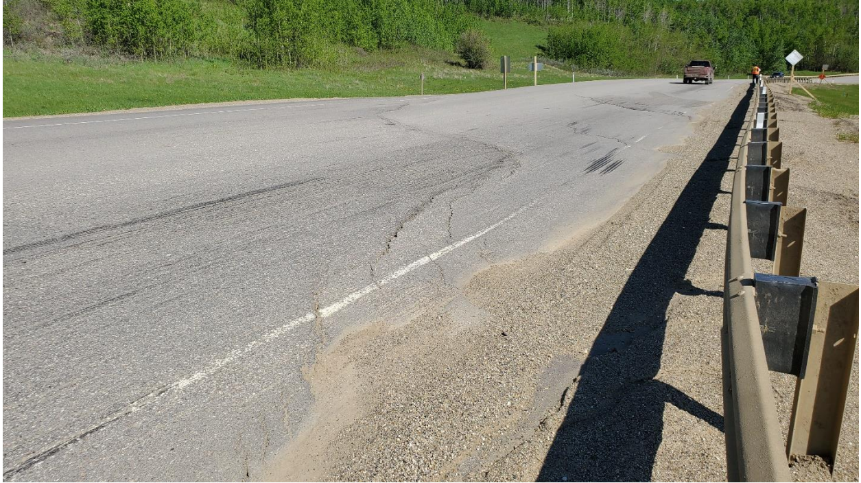
Photo 7 – Looking north at crack just north of the downslope guardrail.
