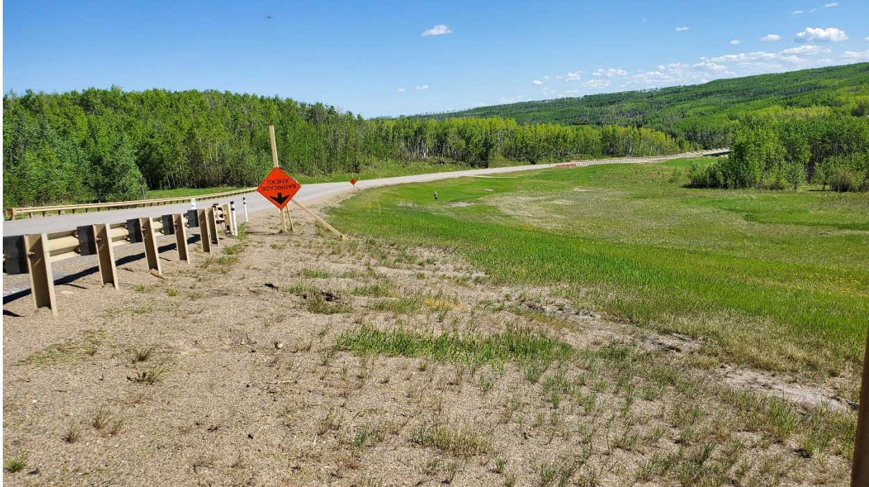
Photo 3 – Looking northeast at rilling below the guardrail.
