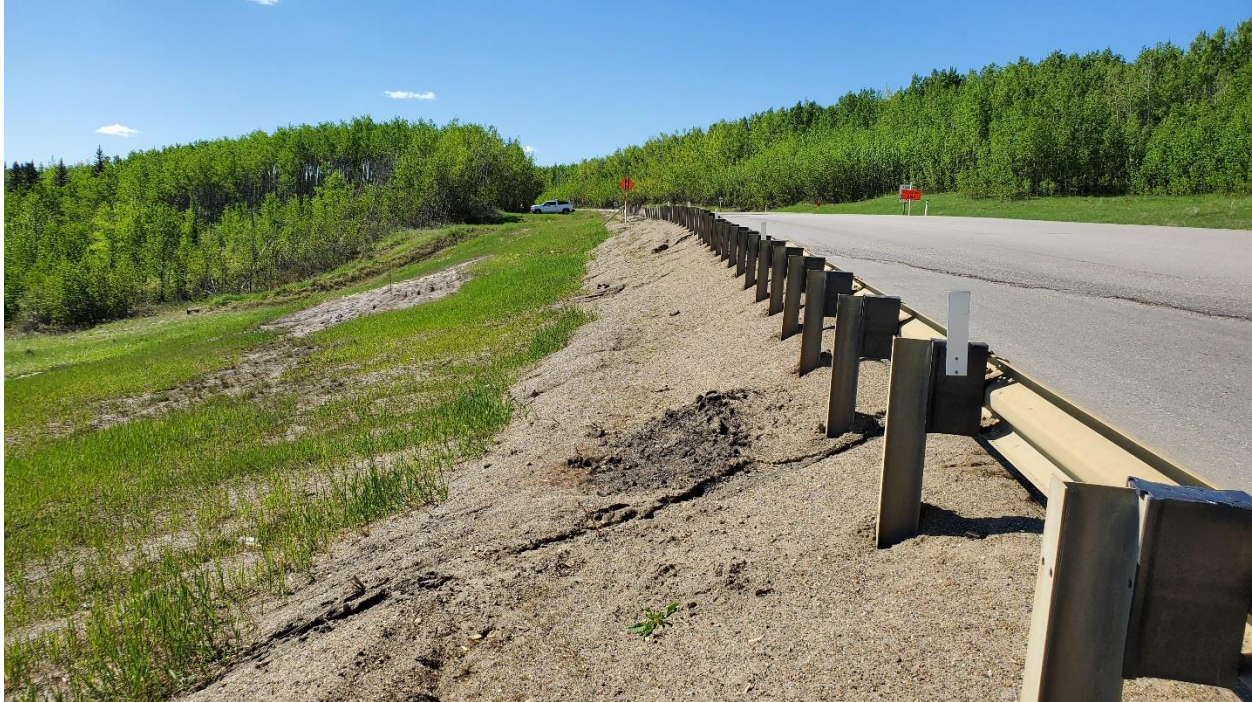
Photo 4 – Looking southwest at guardrail at south end of site. There was a significant sag at this location before the work in 2020.
