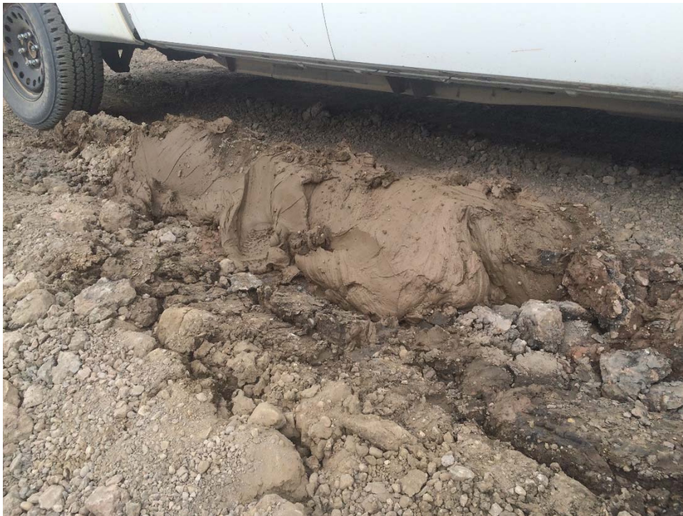
AT Photo 2: Closer view of May 2016 rut.
