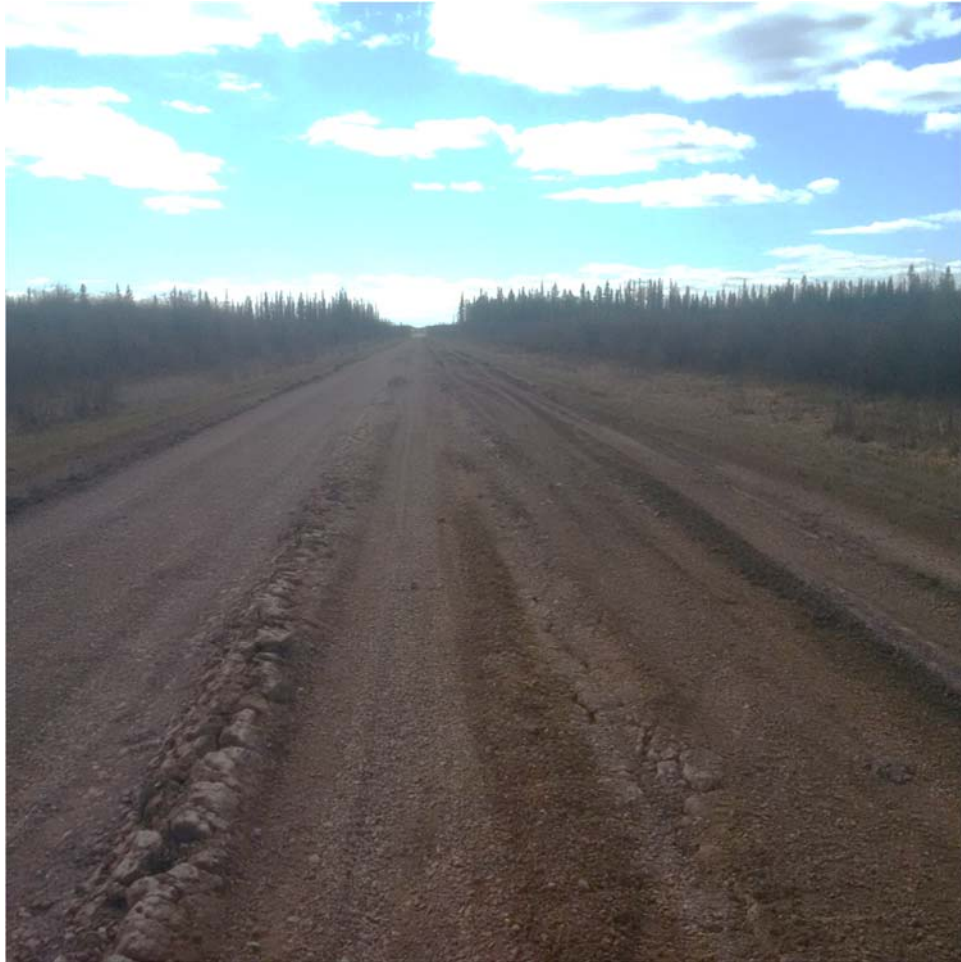
AT Photo 3: Distress in May 2016.
