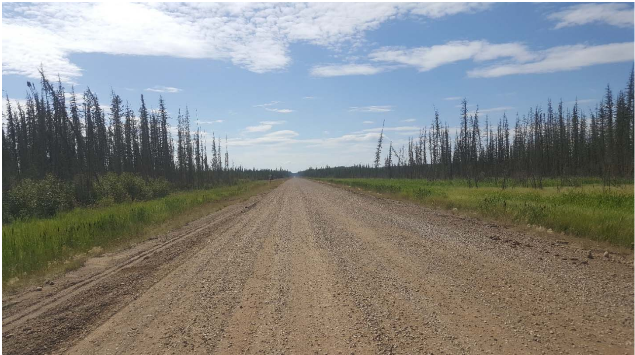
TEL Photo 6: Looking west from km 18.1 near west end of distressed area.
