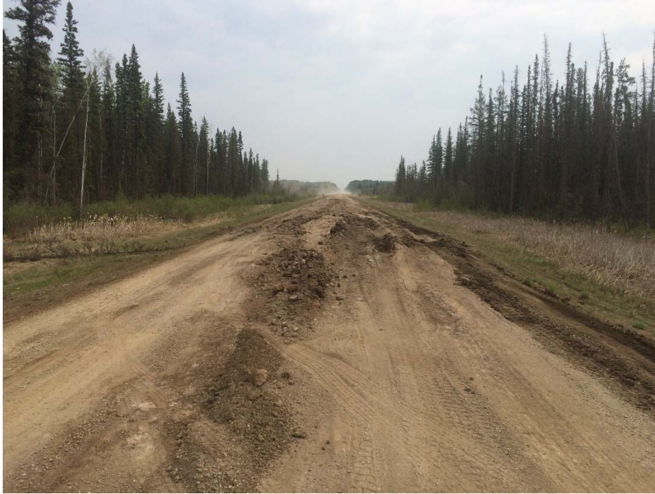
AT Photo 1: Distress in May 2016.
