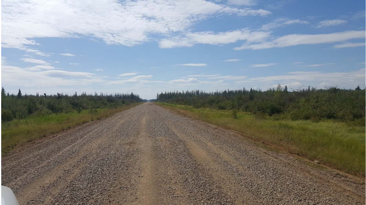
TEL Photo 5: Looking west from km 19.0. near east end of distressed area.
