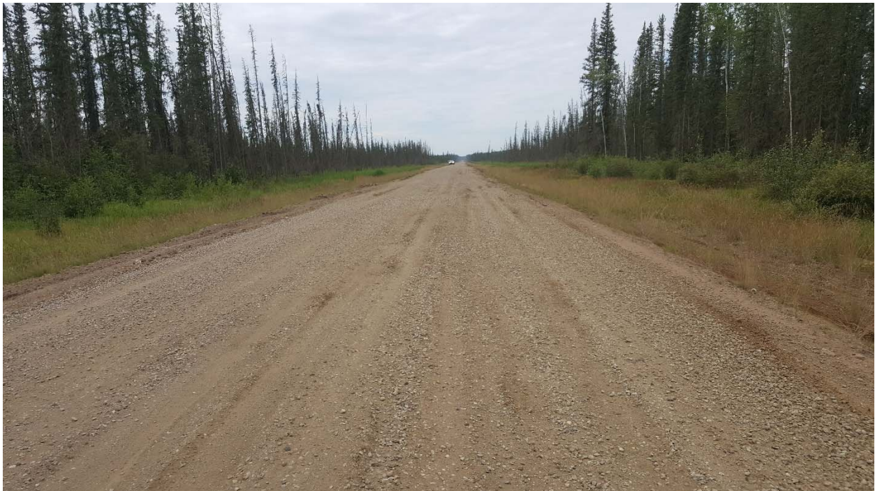
TEL Photo 4: Looking west at local soft spots between km 18.34 and km 18.43.
