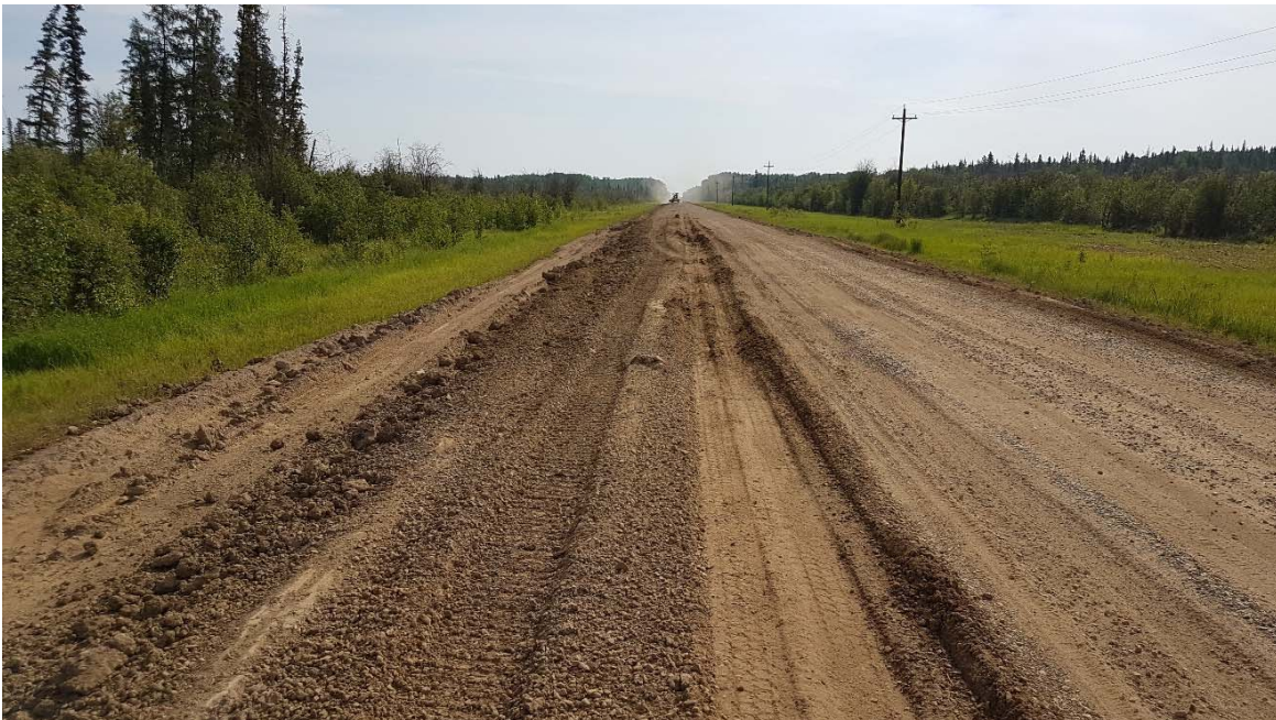
Photo 4 – Looking west at grading underway. Ruts were produced by grader working the highway surface.
