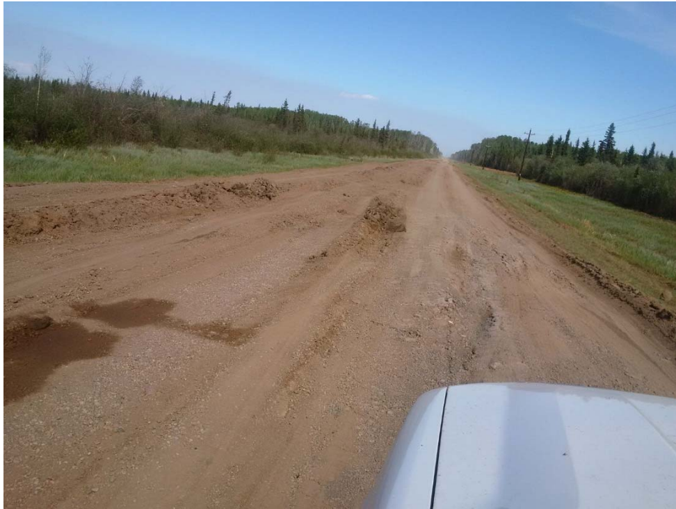
Photo 1 – Looking east at rutting on May 27, 2018 (AT photo)
