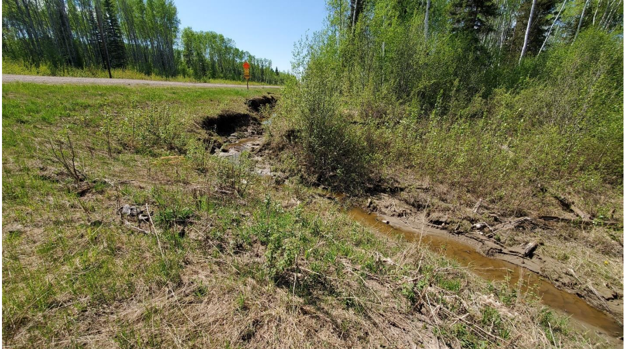
Photo 1 – Looking east at rutting on May 27, 2018 (AT photo)
