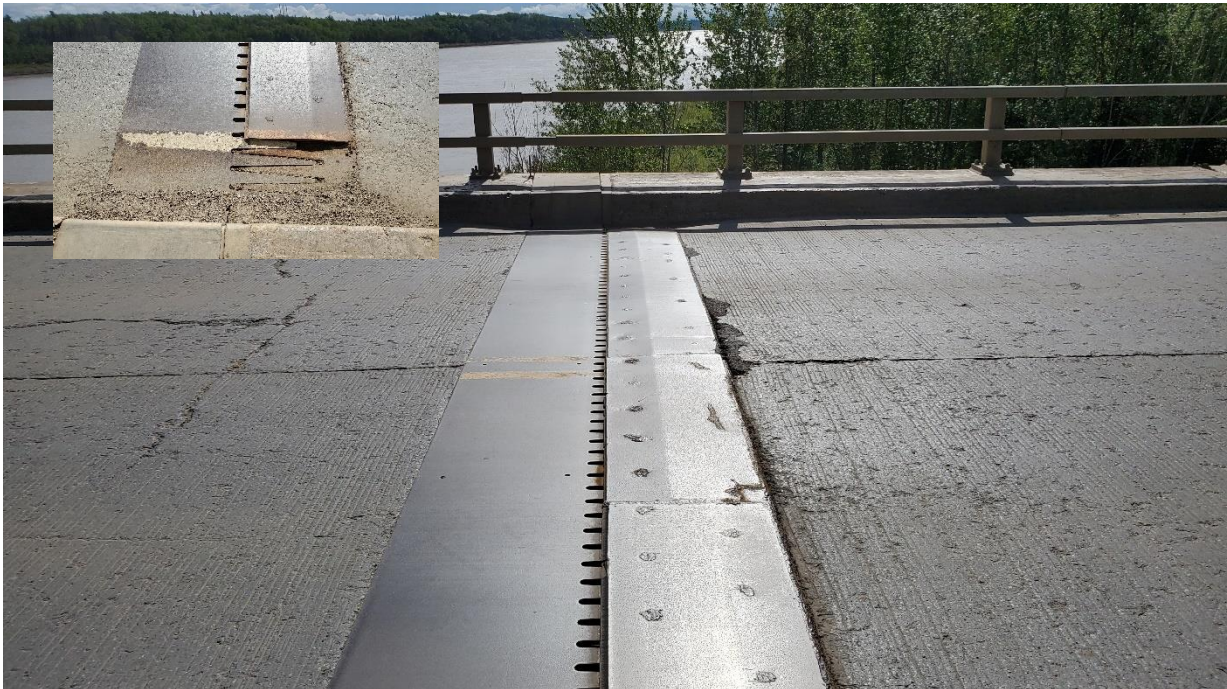
Photo 22, South – Looking east at south abutment finger joints which was covered with a plate between the 2017 and 2018 visits. Plate is loose and rusting at south side (see inset).
