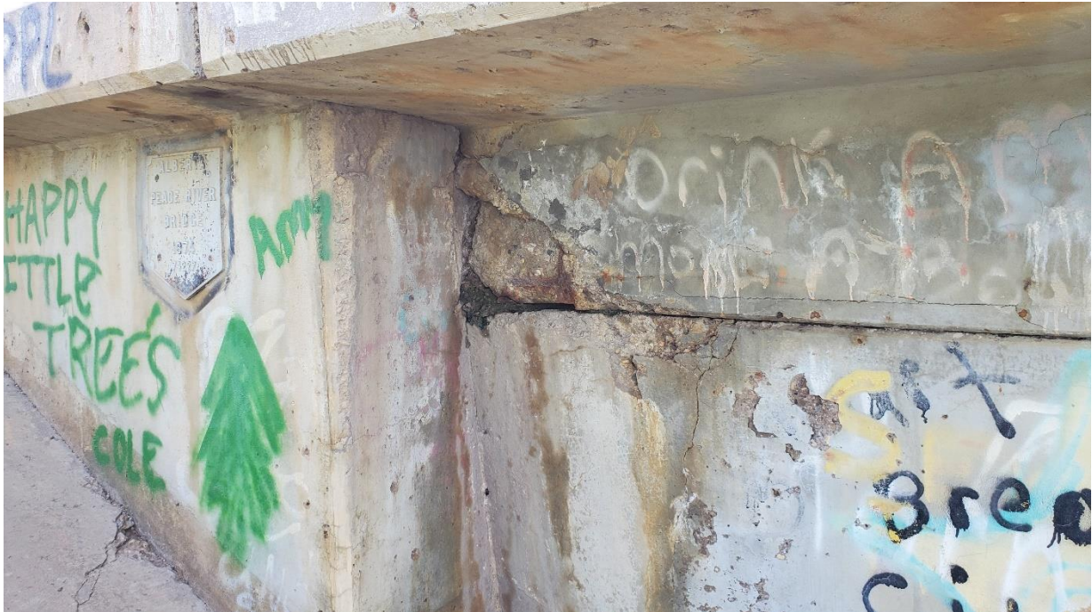
Photo 11B, North – cracking of approach slab beam above west side wingwall.
