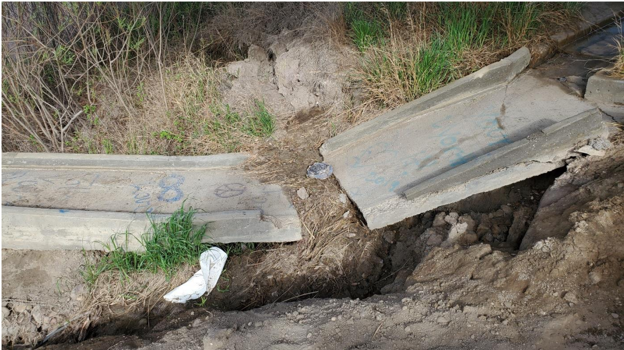
Photo 3B, North – Looking west at cracked and shifting north abutment concrete gutter. Void below the lower portion of the slab up to 350 mm (measured from top of concrete).
