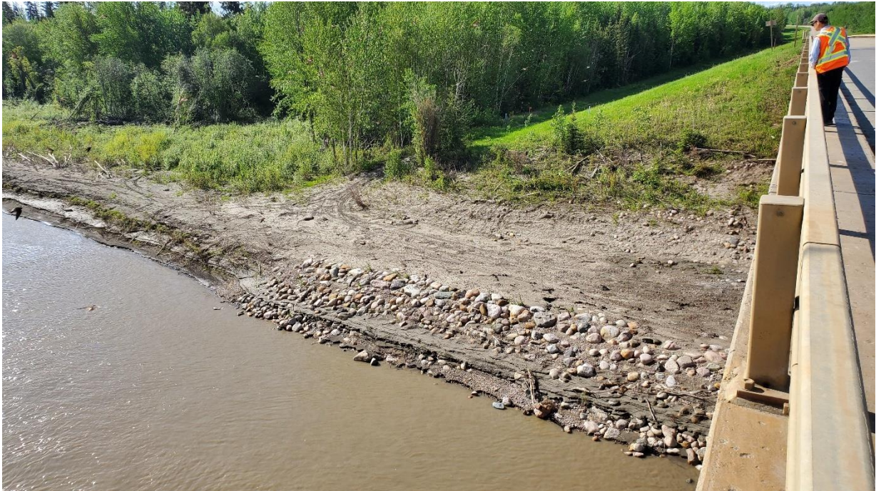
Photo 19, South – Looking south at east side of south abutment with completed construction of toe berm.
