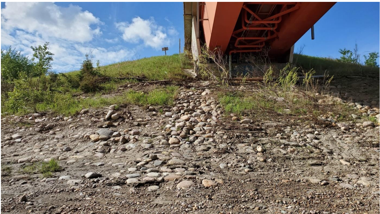
Photo 23B, South – Riprap placed in 2015 on south headslope below east deck drain.
