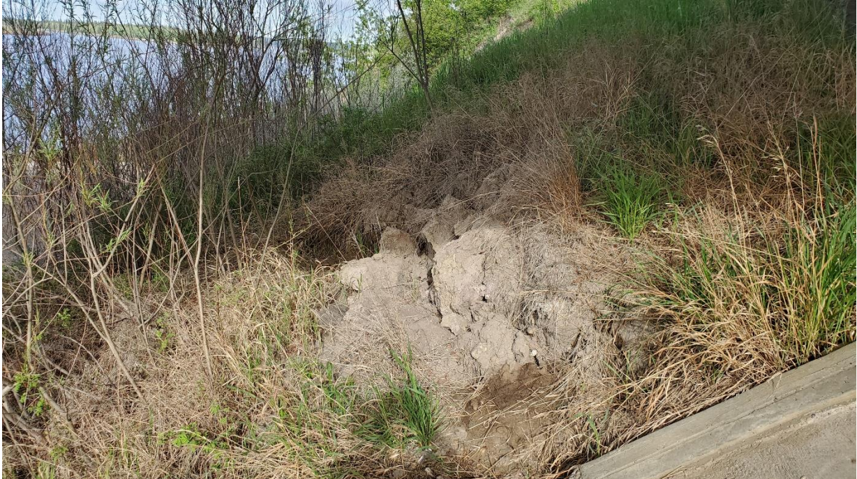
Photo 10, North – Looking northwest at tension cracks on the east side of the north abutment.
