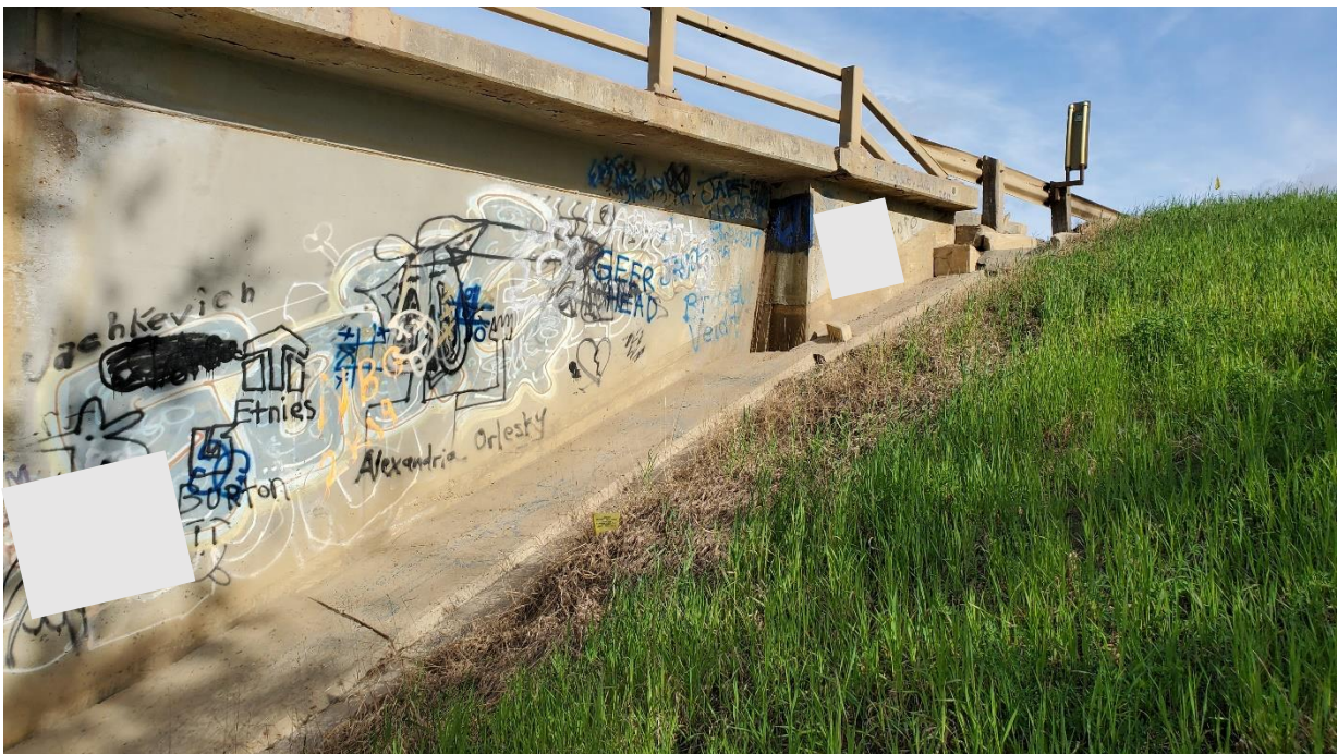
Photo 7, North – Looking northwest at gap between the concrete gutter and north abutment wing wall resulting from settlement of abutment fill.
