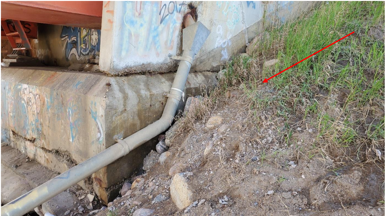
Photo 13, South – Looking southeast at south abutment west side wing wall. Erosion occurring at the base of the wall.
