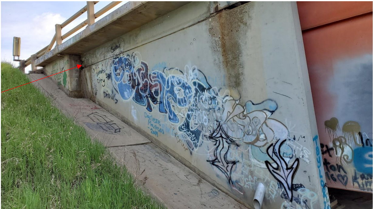
Photo 11A, North – Looking northeast at north abutment west side wing wall. Cracking of beam denoted by red arrow shown in Photo 11B.
