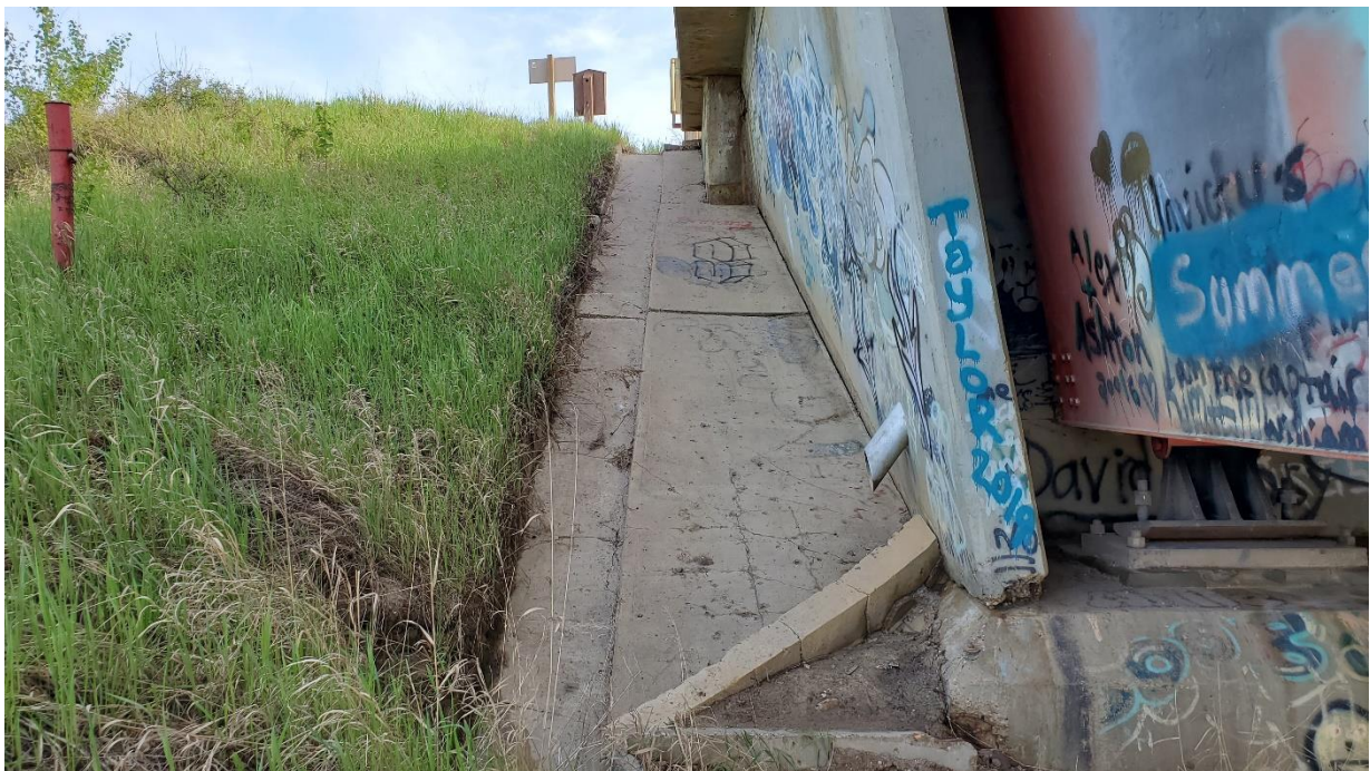
Photo 11C, North – Hump of material creeping into concrete drainage trough adjacent to west wingwall.
