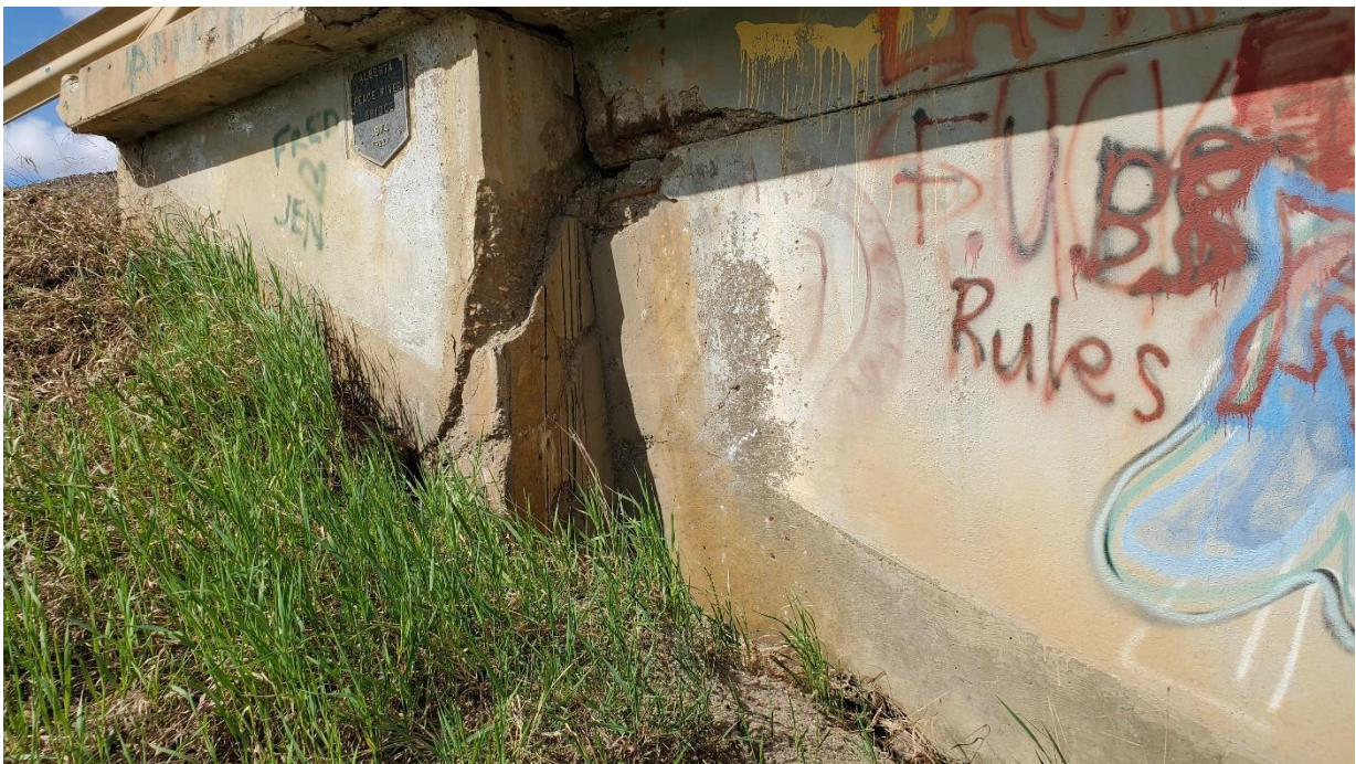
Photo 16B, South – Looking southwest at spalling on south abutment wall.
