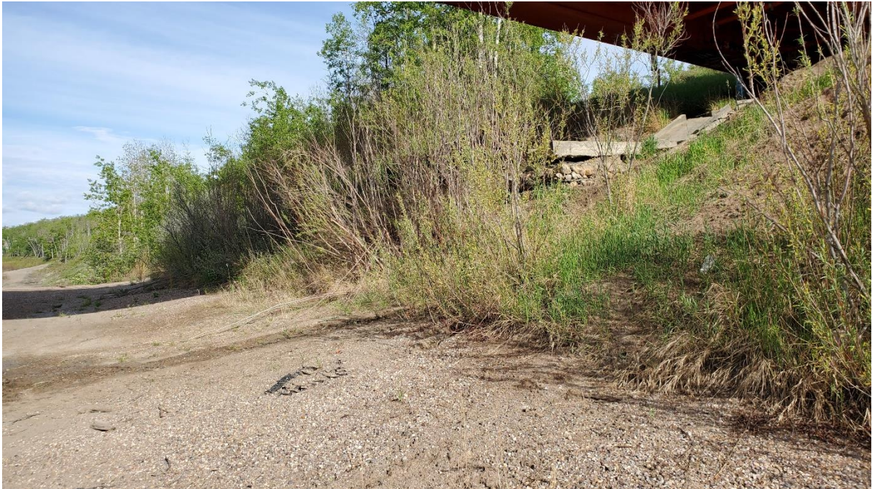
Photo 6, North – Seepage along toe of headslope face just above the top of the toe berm.
