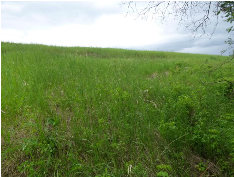
Photo 8 – Looking north up at the slide from the toe of the hwy embankment.
