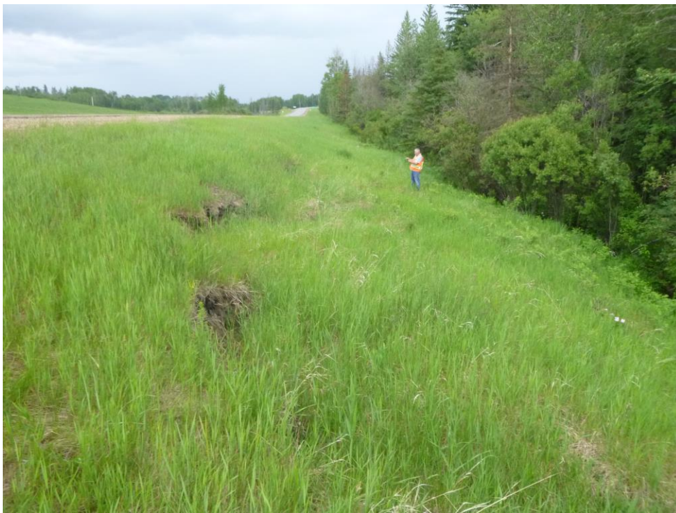
Photo 6 – Looking east across the slide site.
