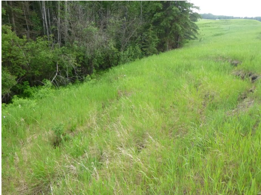
Photo 5 – A close-up view of the slide scarp (looking west) in the south hwy embankment.
