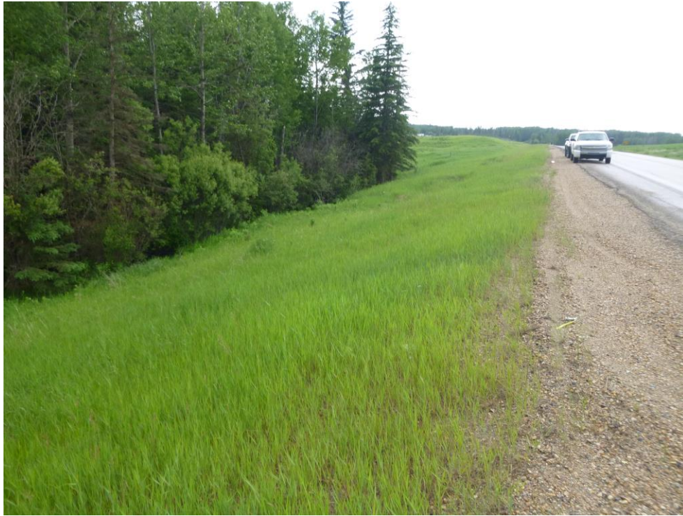
Photo 3 – Looking west across the south hwy embankment (the slide is below the trucks).
