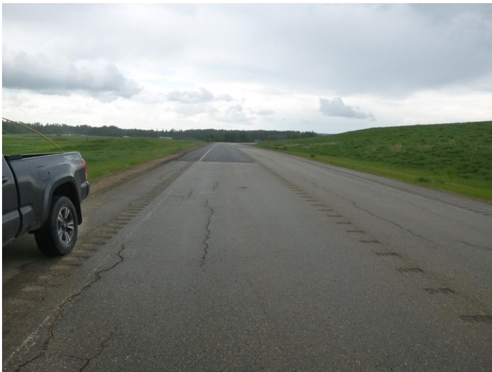
Photo 2 – Looking west along Hwy 679 above the slide site.
