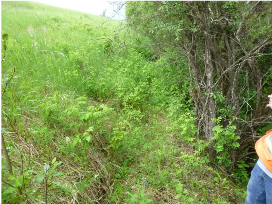
Photo 9 – Looking east along the toe of the hwy embankment and edge of the stream at subsidence at the west edge of the slide.
