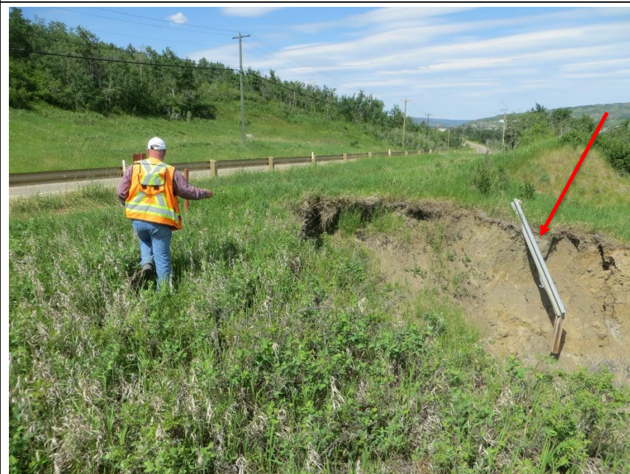
Photo 2. Looking northeast from the south side of Slide 1. Note hanging guardrail.
