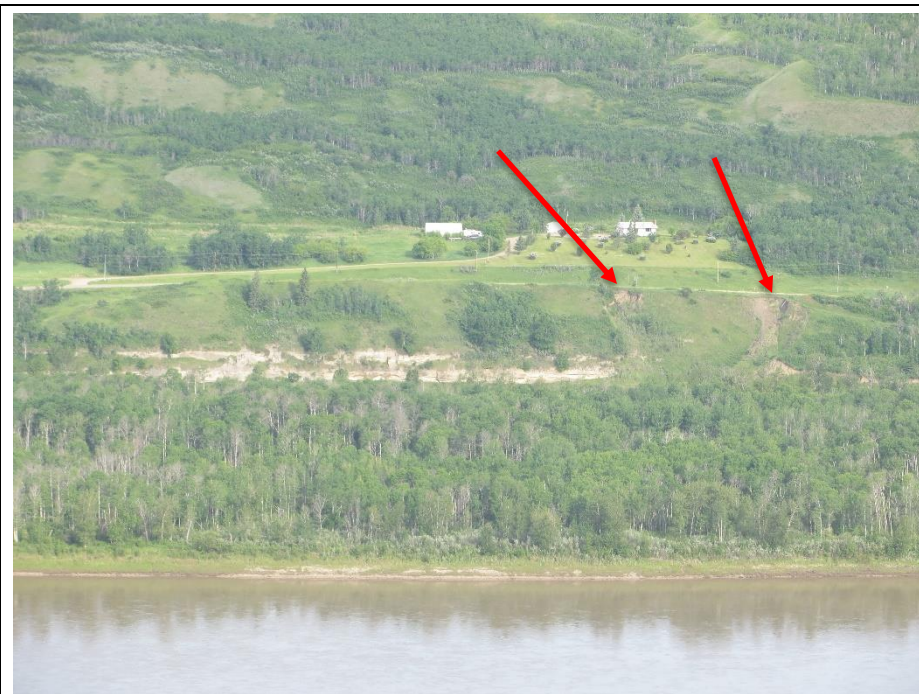
Photo 1. Looking West from the east valley slope of the Peace River towards the two slides on Hwy 684:02.
