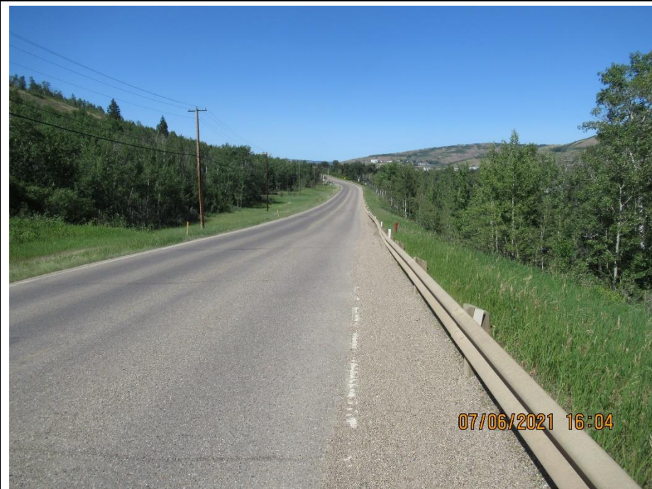
Photo 8. Looking north towards the slide at km 28.6. Note the bow in the guardrail.
