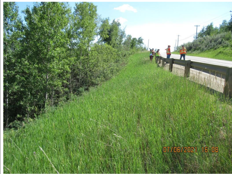
Photo 11. Looking south at the highway side slope below the slide at km 28.6. Note the dip in the guardrail.
