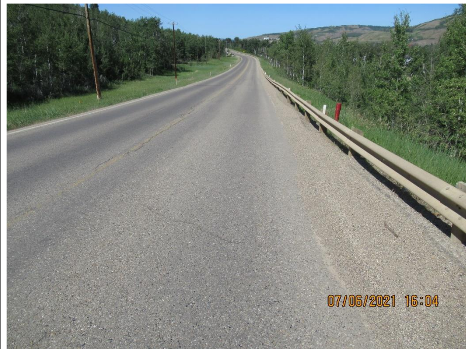
Photo 9. Looking north at the slide at km 28.6. Tension cracks and a dip in the pavement are visible. Cracks along the median are more apparent relative to the 2019 condition.
