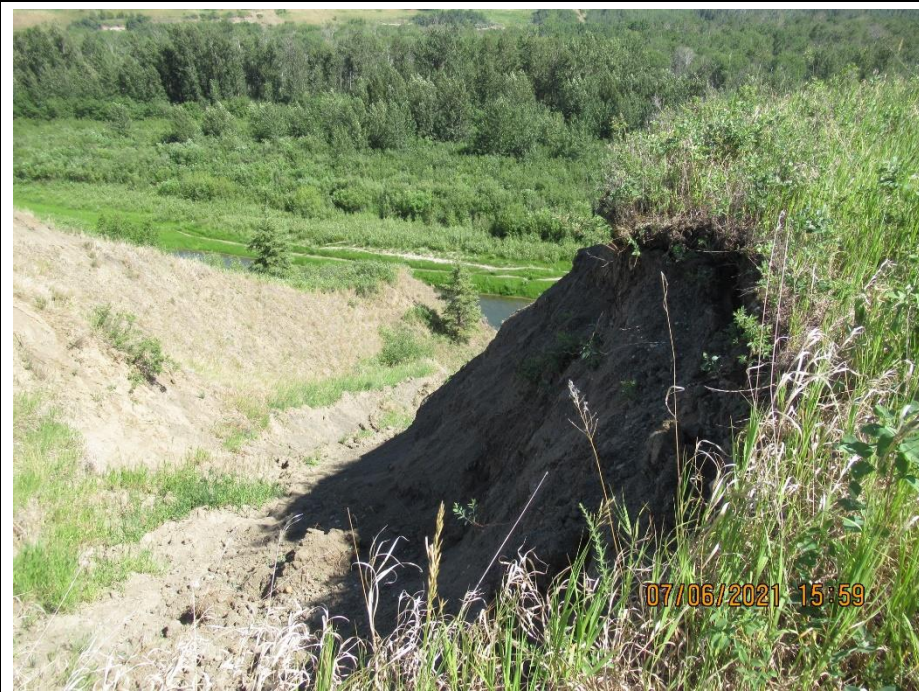
Photo 3. Looking northeast from the south side of the backscarp of Slide 1. There has been some retrogression along the south flank.
