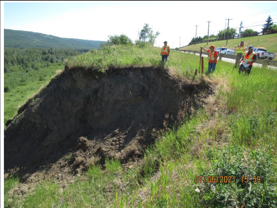
Photo 2. Looking southwest from the north flank of Slide 1. Some retrogression of the south flank of the side has occurred since 2019. Offset to the guardrail was 3.8 m.
