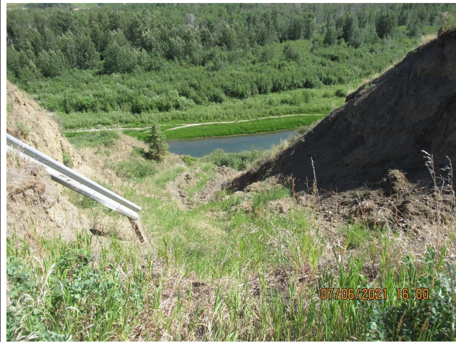
Photo 4. Closeup view of slide debris below the backscarp of Slide 1. Increased vegetation growth on the disturbed soils relative to the 2019 condition.
