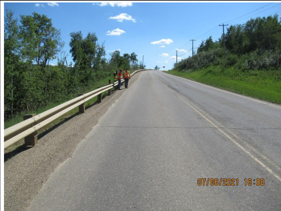
Photo 10. Looking south at the new slide. Note the tension cracks around the road centreline.
