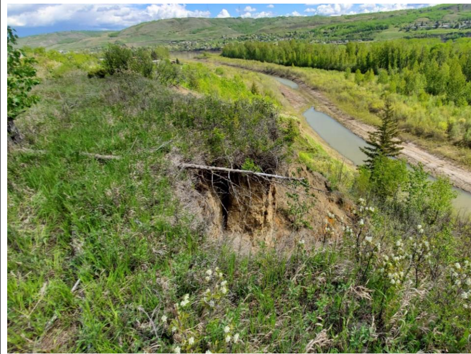
Photo 3. Looking northeast from the south flank of Slide 2.
