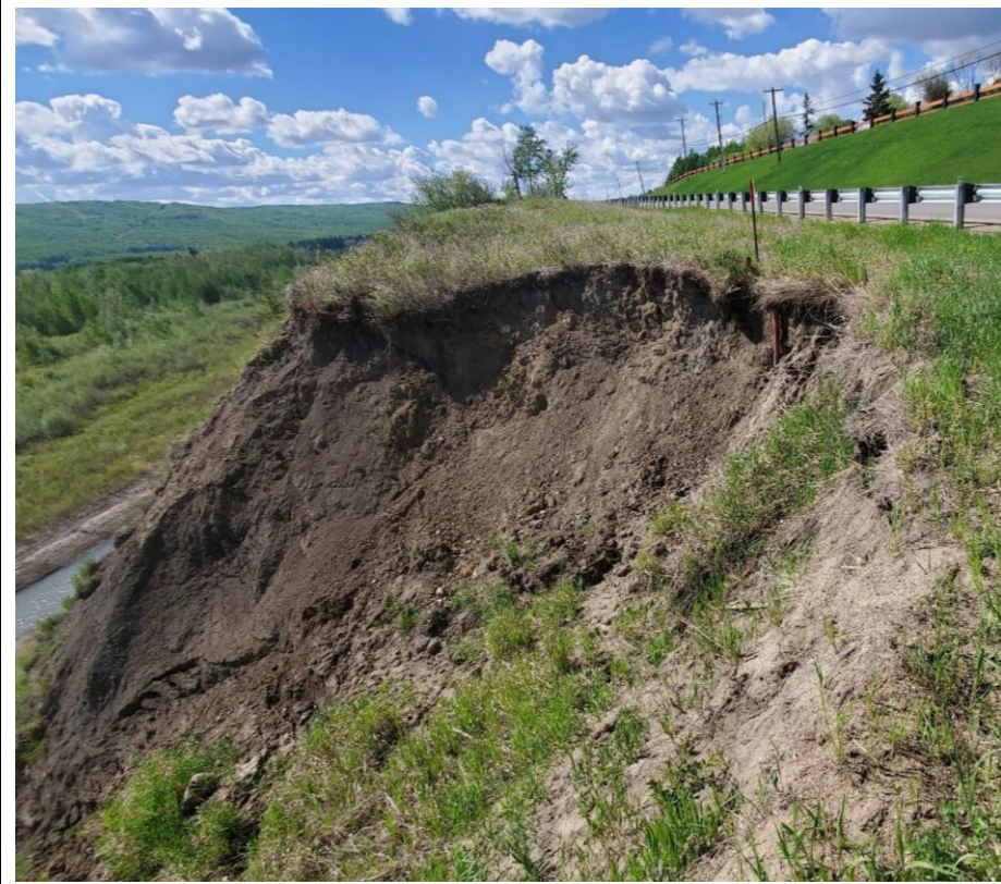
Photo 1. Looking southwest from the north flank of Slide 1. Fresh soil was visible and there was minor retrogression of the south flank since 2021. Minimum offset from the main scarp to the guardrail was 3.4 m.
