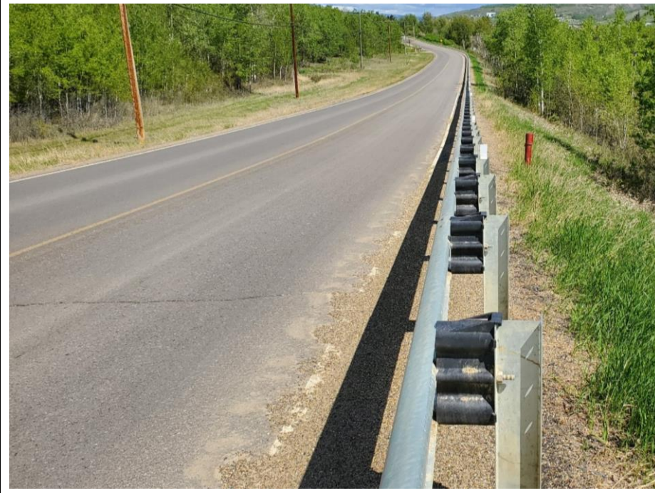
Photo 4. Looking north at the slide at km 28.6. Transverse crack across the pavement is visible. No significant change relative to the 2021 condition.
