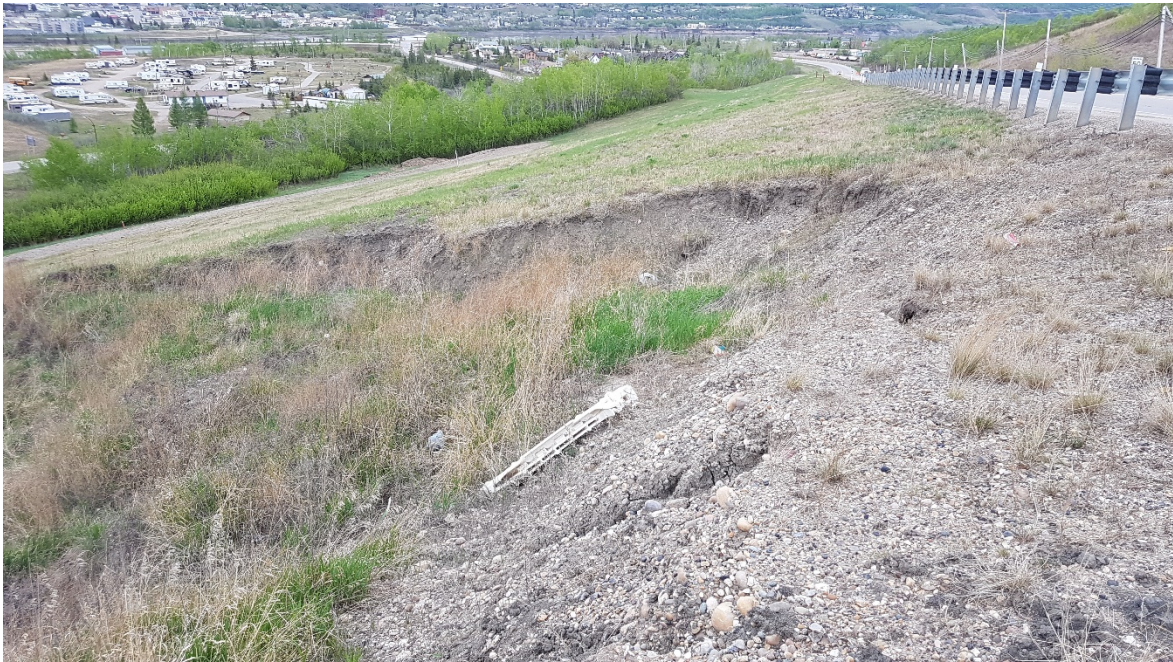
Photo 3: Looking southeast along the NBL shoulder of the Hwy 2 off-ramp at retrogressing backscarp.
