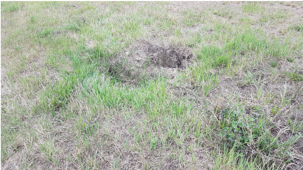
Photo 22: Looking north at a sink hole above the 500 mm SWSP centreline culvert on the sideslope of the NBL of Hwy 2 off-ramp.
