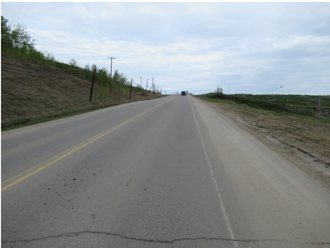
Photo 18: Looking northwest at previous scarp crack faintly visible in NBL through 2016 patch.
