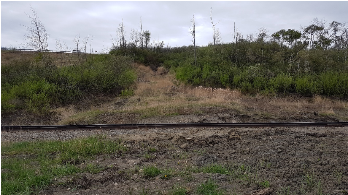
Photo 26: Looking southwest at the debris flow material immediately upslope of the CNR line. Material appears to have been recently excavated.
