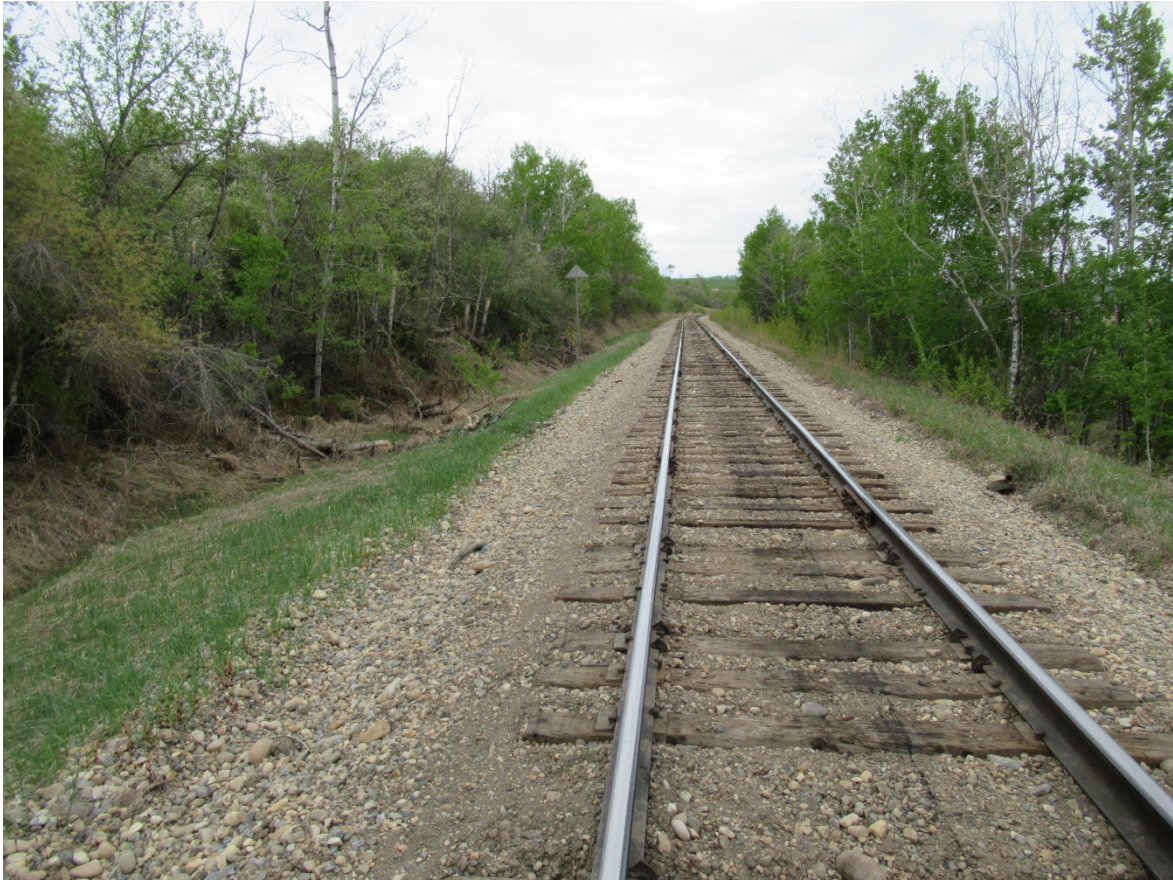
Photo 25: Looking northwest along toe bulge of the landslide below SP09-11 (Photo 23) at the west side of the CNR track.
