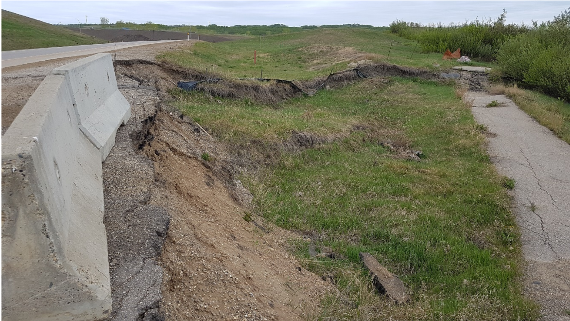
Photo 1: Looking northwest along shoulder of the Hwy 2 off-ramp on the east side of 99 Avenue intersection.
