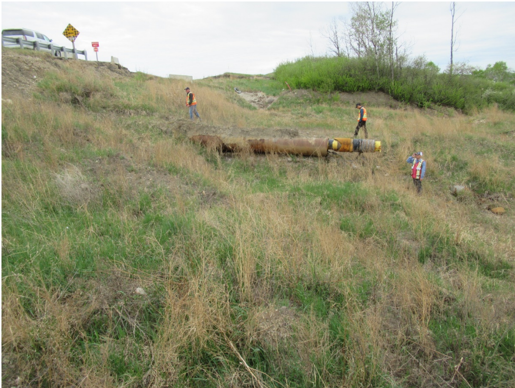
Photo 11: Looking northwest at severed and abandoned storm utility pipe. The new line was installed farther north by the Town in 2016.
