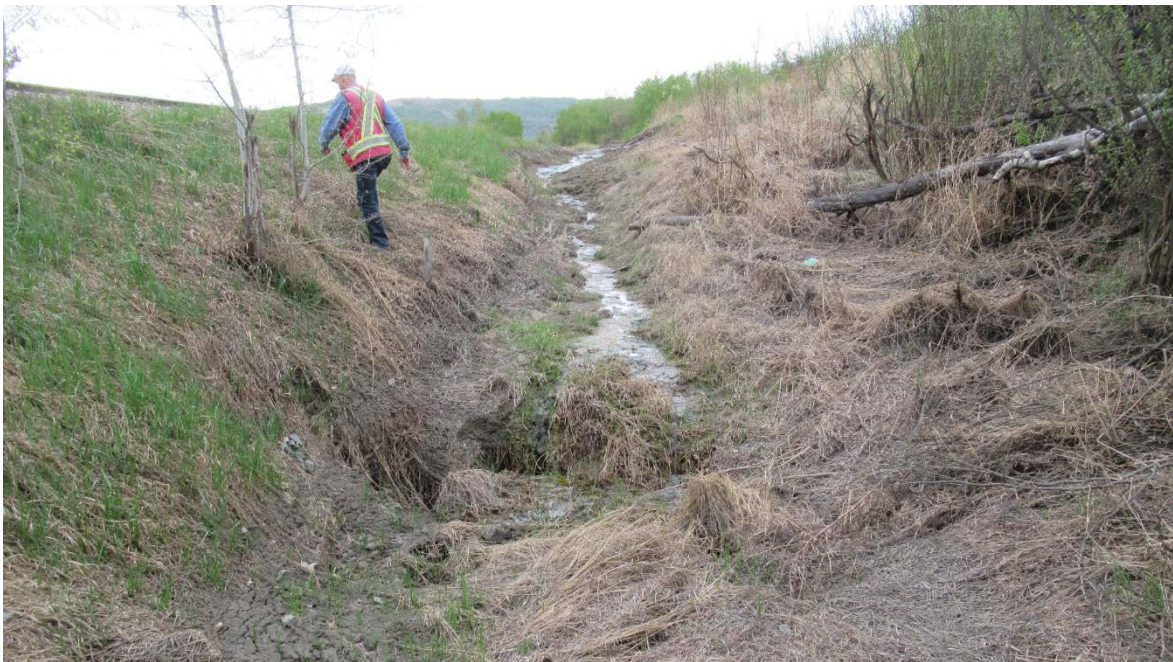
Photo 27: Looking southwest at seepage/ditch flow around debris fan flowing into nearly buried culvert below CNR tracks.
