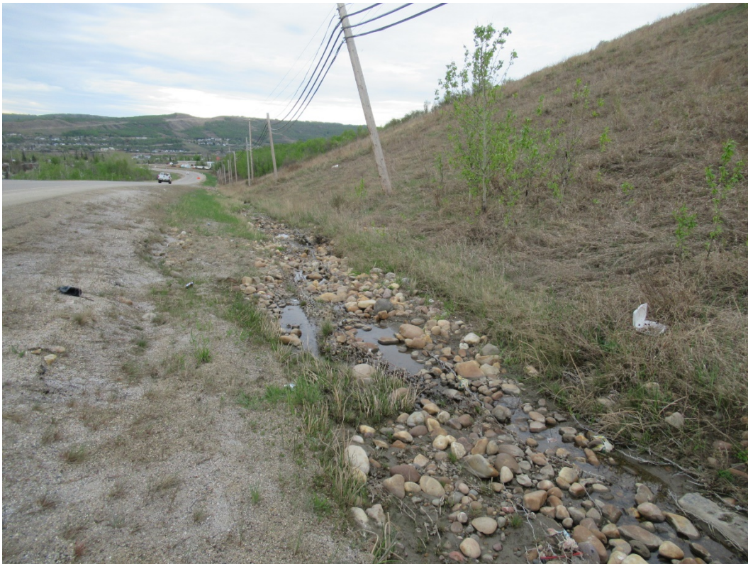
Photo 17: Looking southeast at damaged gabion basket in ditch bottom and leaning power pole
