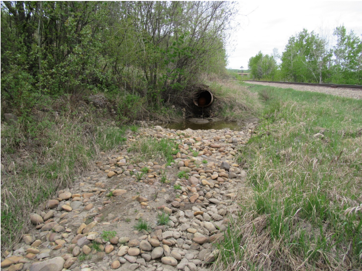
Photo 24: Looking northwest where water has previously ponded below the hanging outlet of the 600 mm CSP that connects to the 500 mm SWSP centreline culvert.
