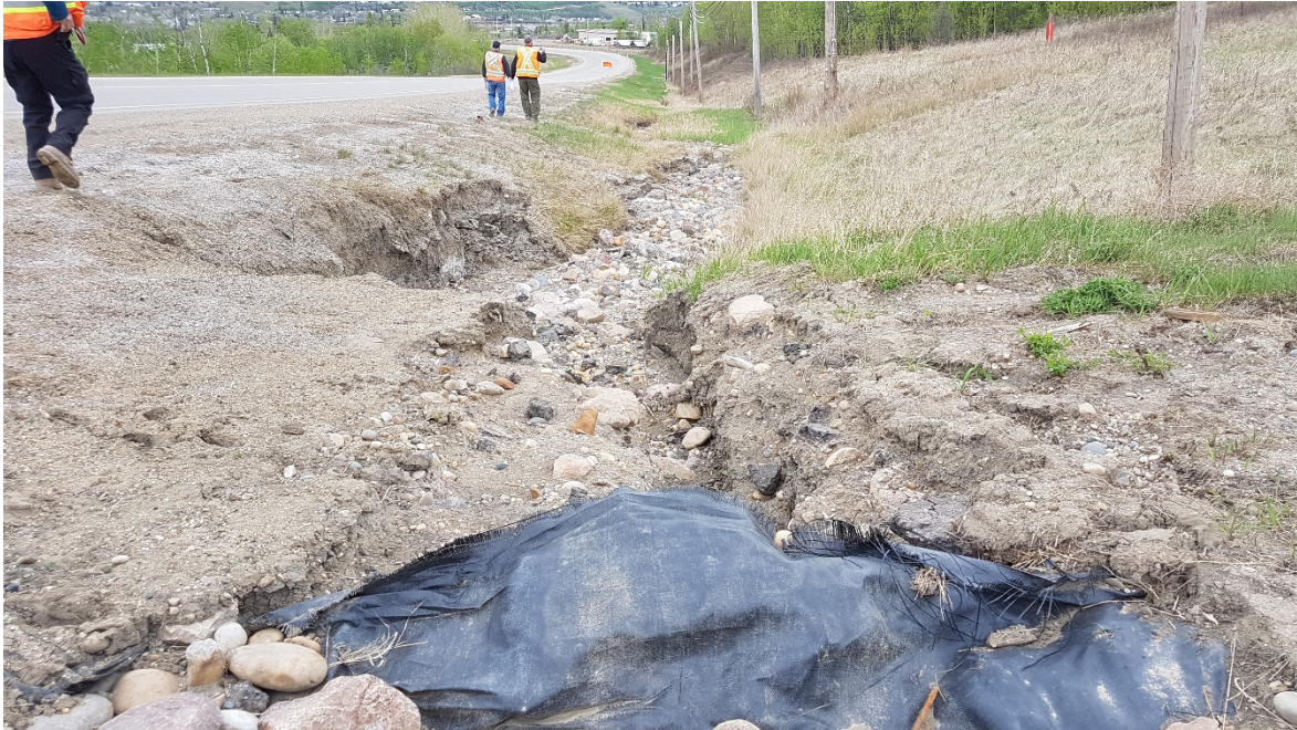
Photo 21: Looking southeast at erosion in ditch below inlet of 500 mm SWSP centerline culvert.
