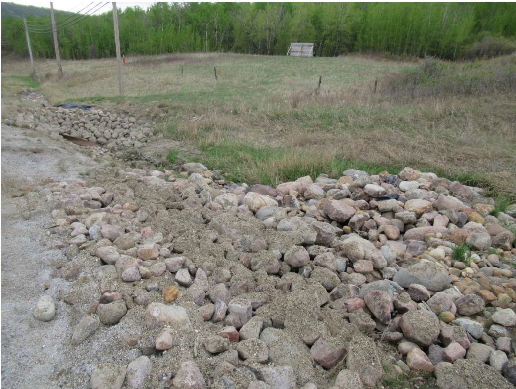
Photo 20: Looking south at riprap pile in ditch north of 500 mm SWSP centerline culvert inlet.
