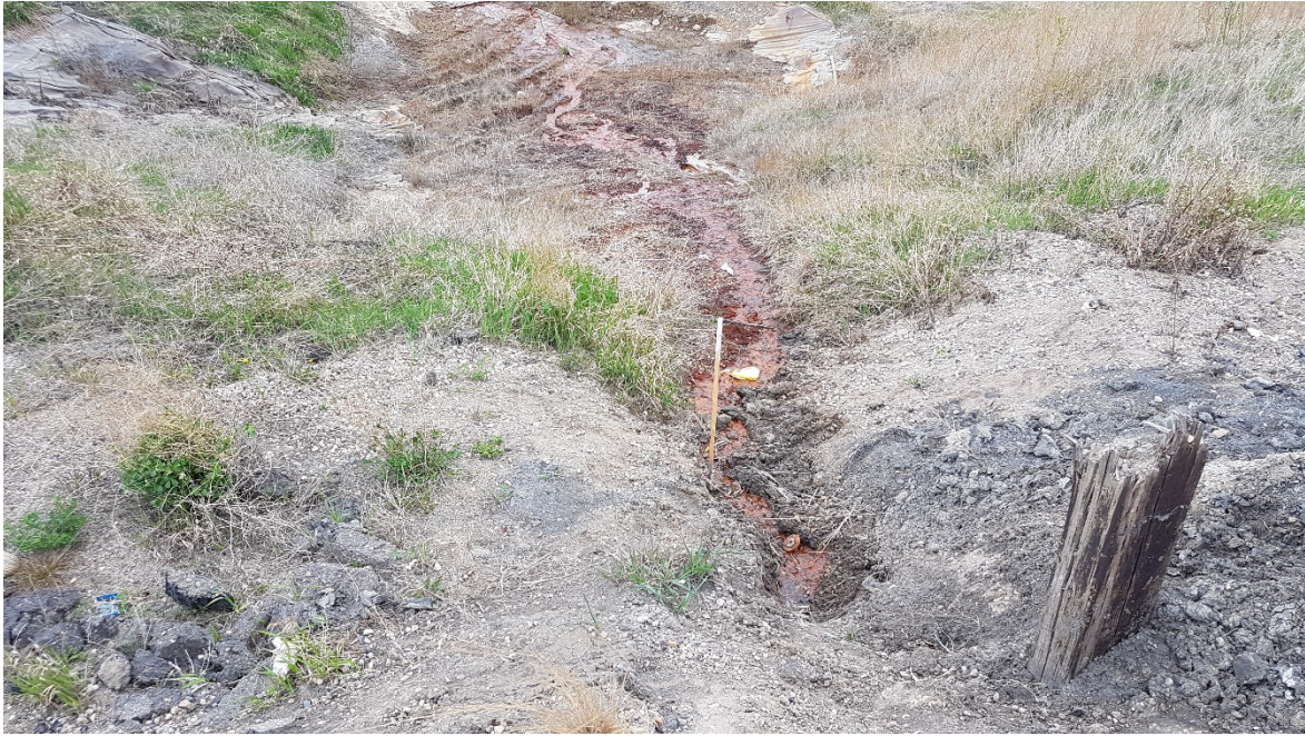
Photo 5: Looking east at seepage from gravel layer in the Hwy 2 off-ramp sideslope draining onto the geomembrane lining.
