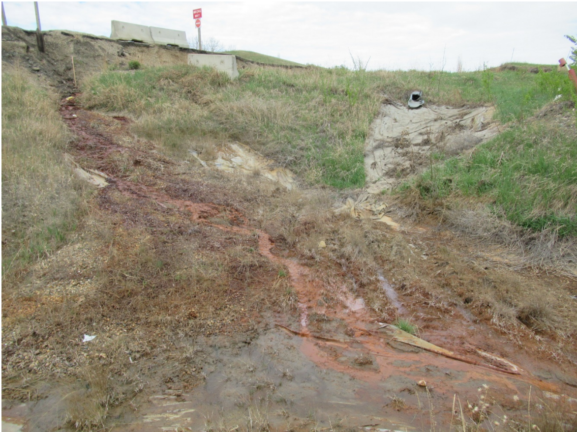
Photo 4: Looking west at springs flowing from the embankment below the Hwy 2 off-ramp at 99 Avenue.
