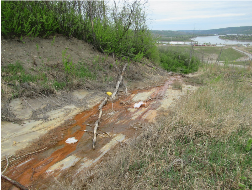
Photo 7: Looking northeast at lower portion of the geomembrance installed by the Town below the 99 Avenue intersection.
