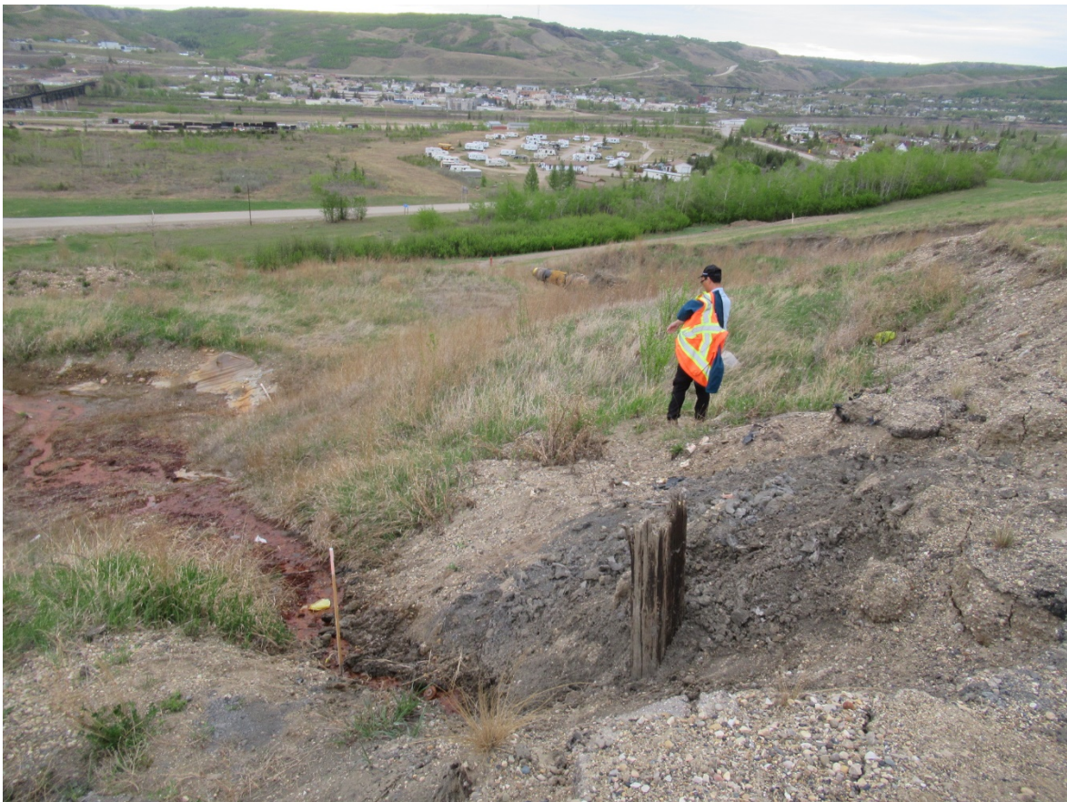
Photo 10: Looking east at the upper portion of the slide.
