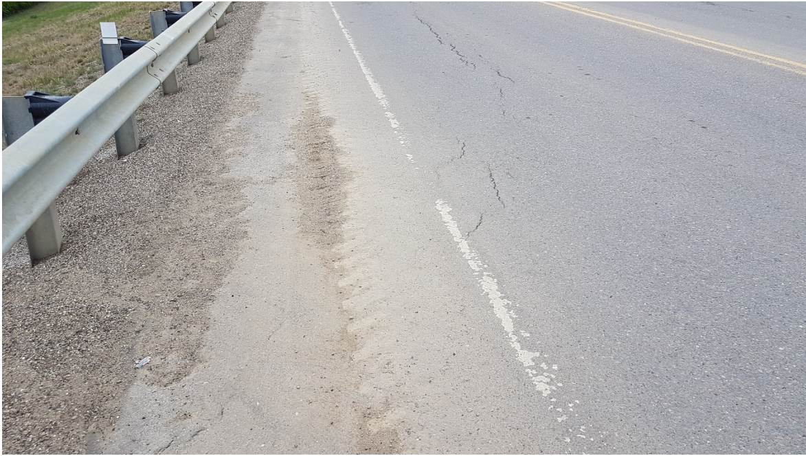
Photo 15: Cracking forming in ACP at the guardrail on the southeast side of 99 Avenue intersection. Crack is coincident with previous semi-active slide scarp.
