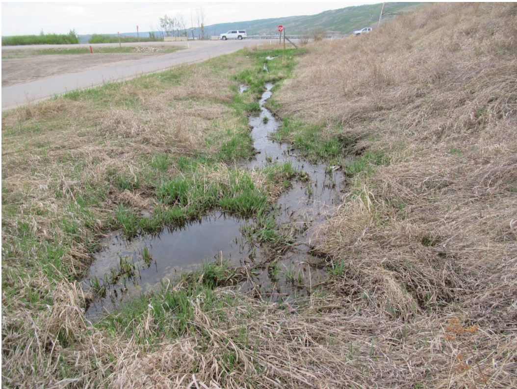
Photo 12: Looking northeast at seepage from 99 Avenue southeast ditch.
