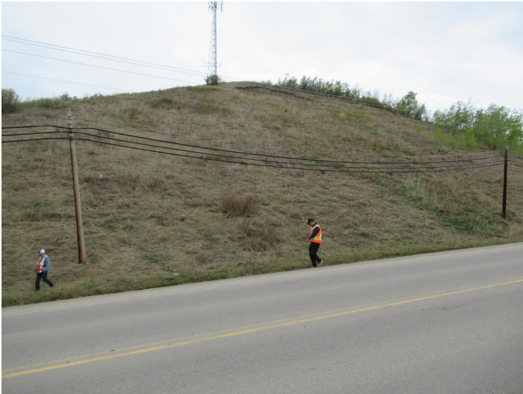
Photo 19: Looking west at skin slide in Hwy 2 backslope below communications tower.
