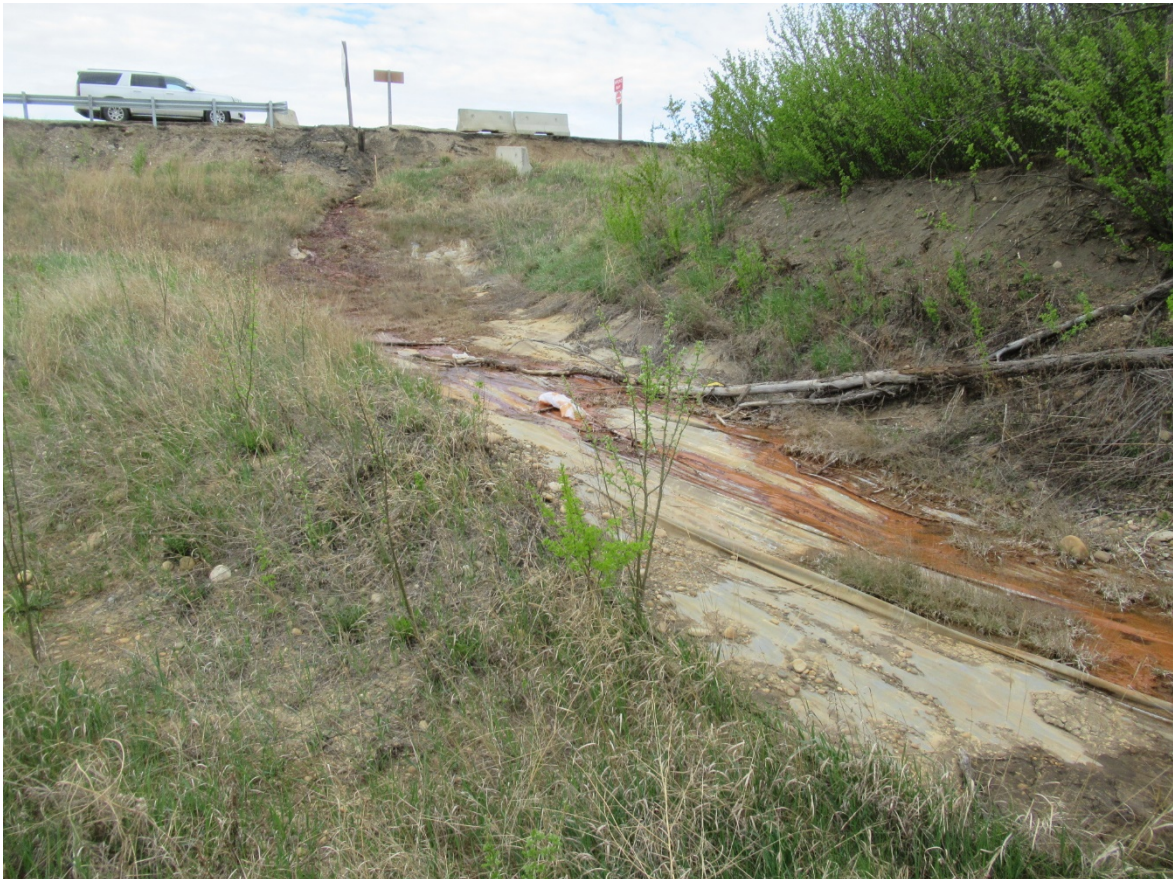
Photo 6: Looking west along the membrane installed by the Town below the 99 Avenue intersection.
