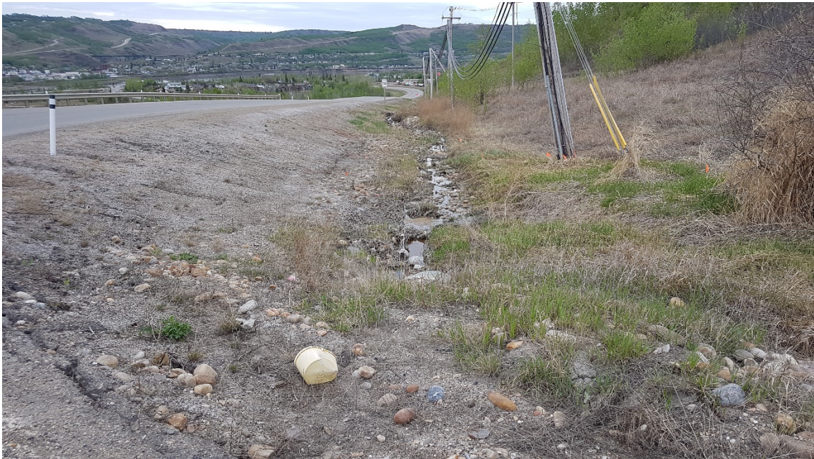
Photo 13: Looking southeast from culvert outlet at 99 Avenue. Note leaning posts and damaged gabion basket ditch lining.
