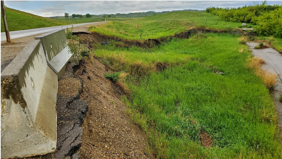
Photo 1: Looking northwest along shoulder of the Hwy 2 off-ramp on the east side of 99 Avenue intersection.
