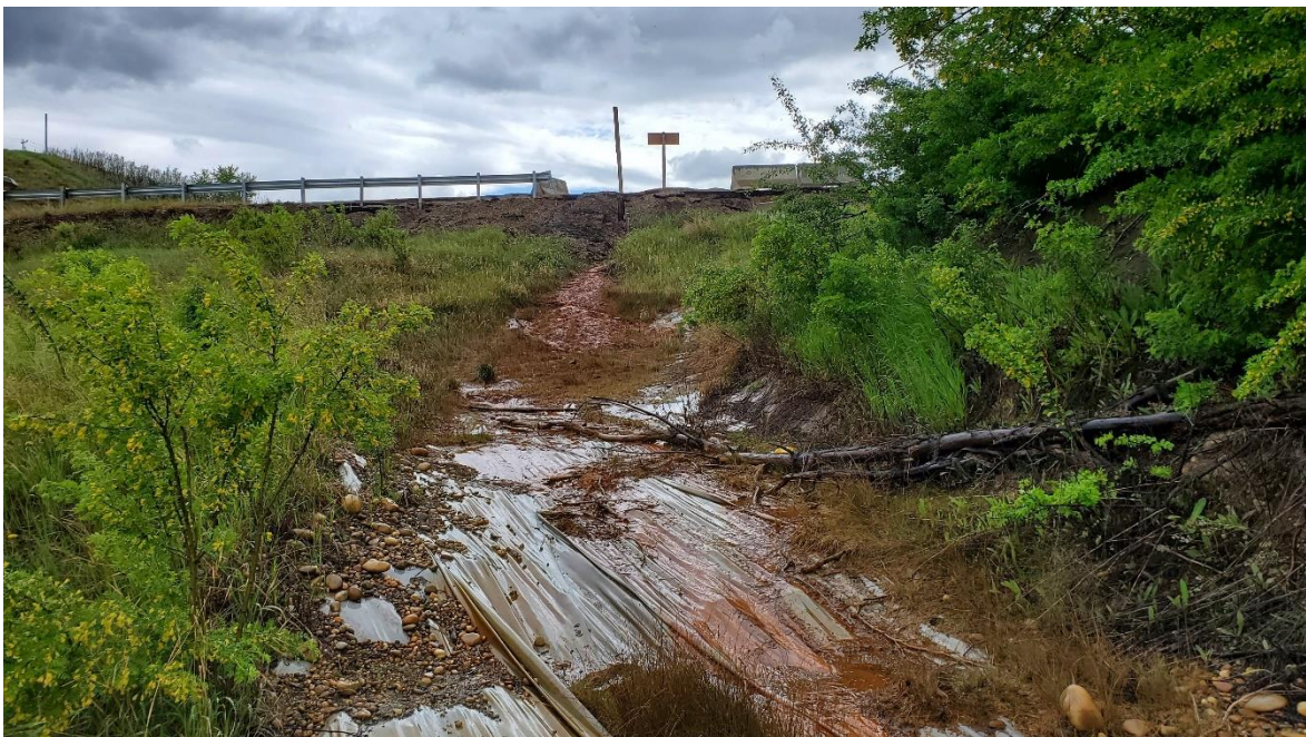
Photo 6: Looking west along the membrane installed by the Town below the 99 Avenue intersection.
