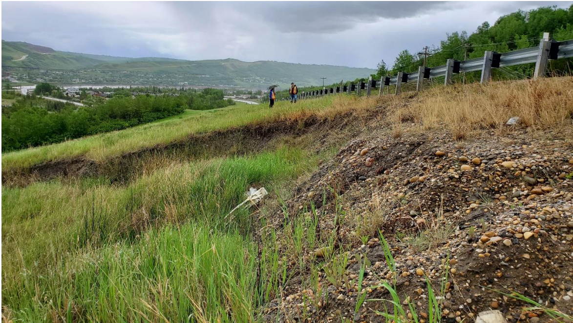
Photo 3: Looking southeast along the NBL shoulder of the Hwy 2 off-ramp at retrogressing backscarp.
