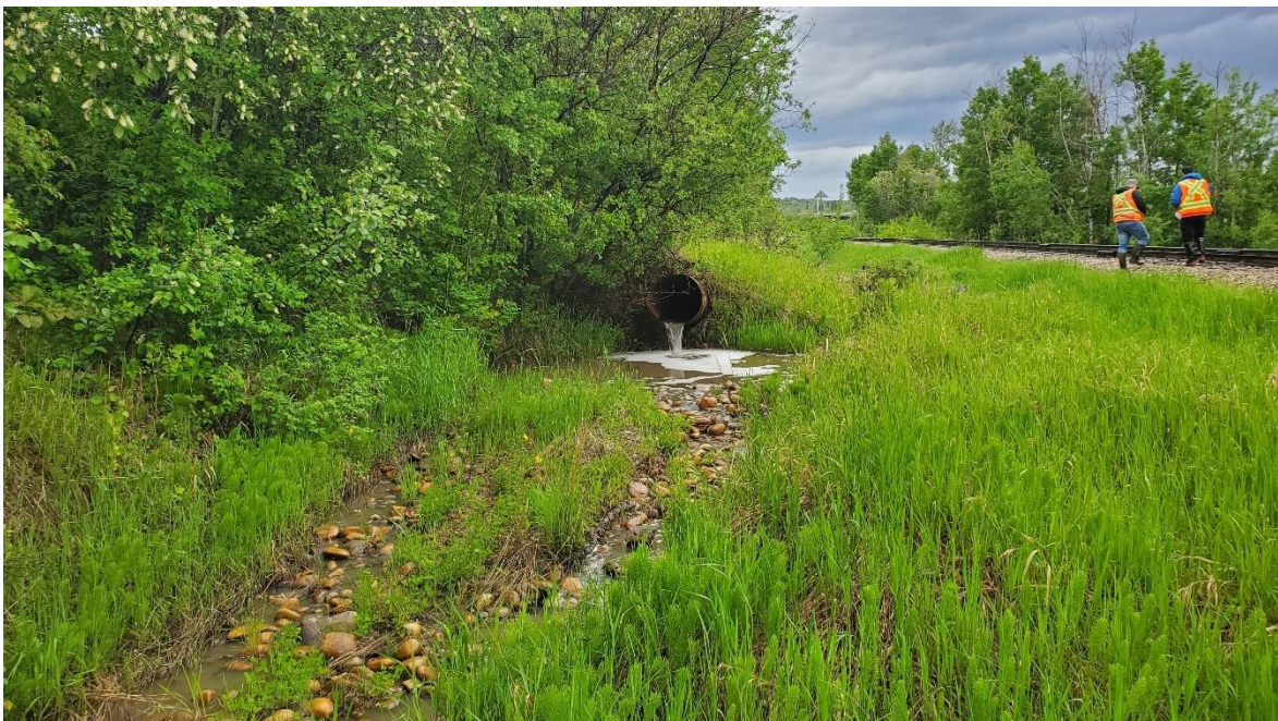
Photo 24: Looking northwest where water has previously ponded below the hanging outlet of the 600 mm CSP that connects to the 500 mm SWSP centreline culvert.
