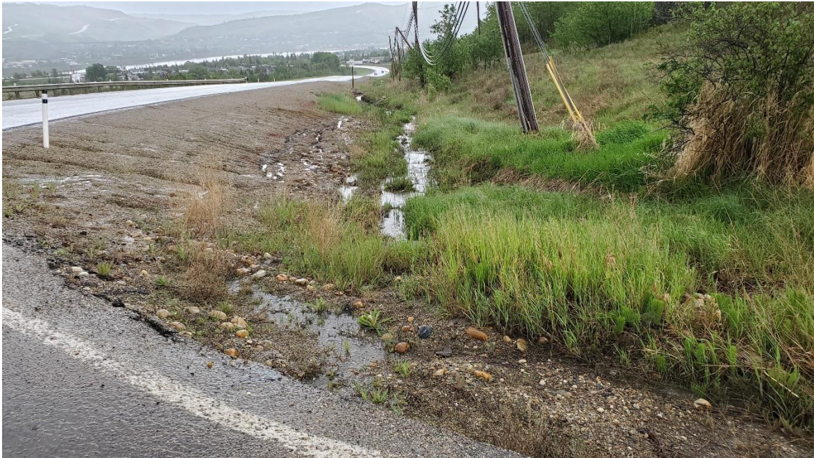
Photo 13: Looking southeast from culvert outlet at 99 Avenue. Note leaning posts and damaged gabion basket ditch lining.
