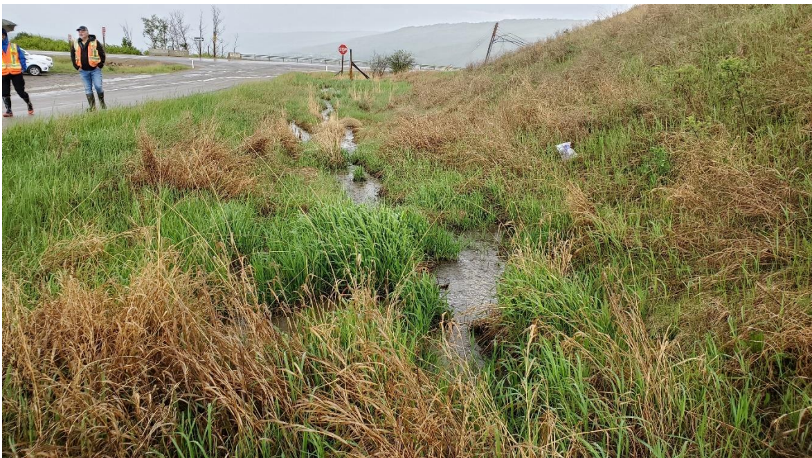
Photo 12: Looking northeast at seepage from 99 Avenue southeast ditch.
