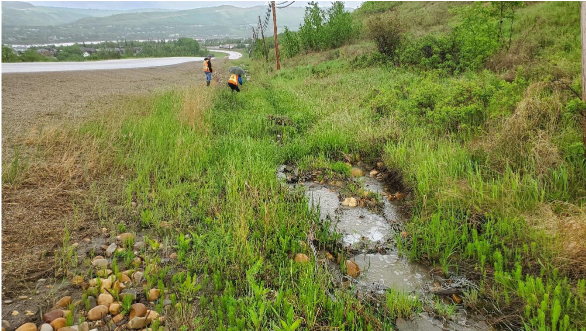
Photo 17: Looking southeast at damaged gabion basket in ditch bottom with leaning power poles in the background.
