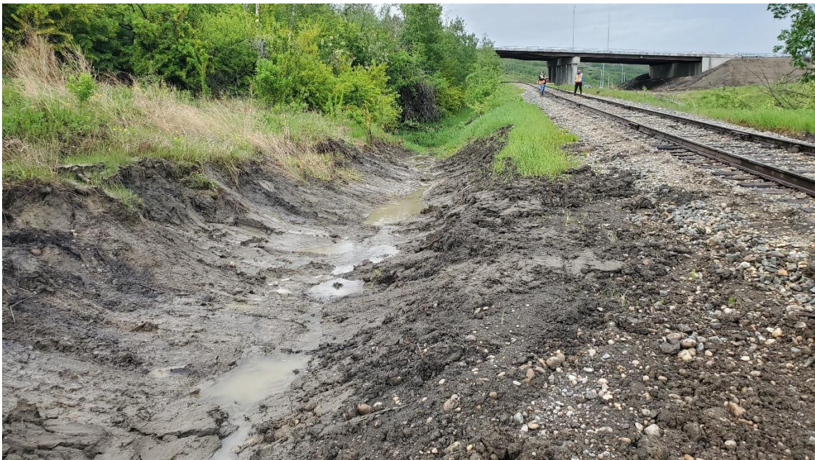
Photo 27: Looking northeast at seepage/ditch flow around debris fan flowing into nearly buried culvert below CNR tracks.
