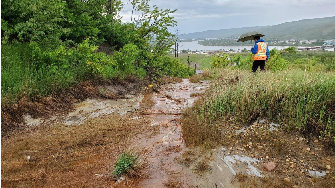
Photo 7: Looking northeast at lower portion of the geomembrane installed by the Town below the 99 Avenue intersection.
