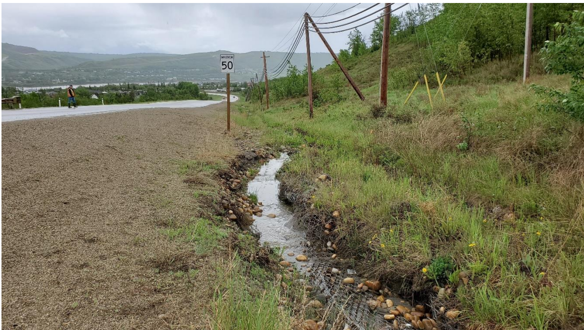
Photo 14: Looking southeast at the scour below gabion mattress in southeast ditch of Hwy 2 off-ramp.
