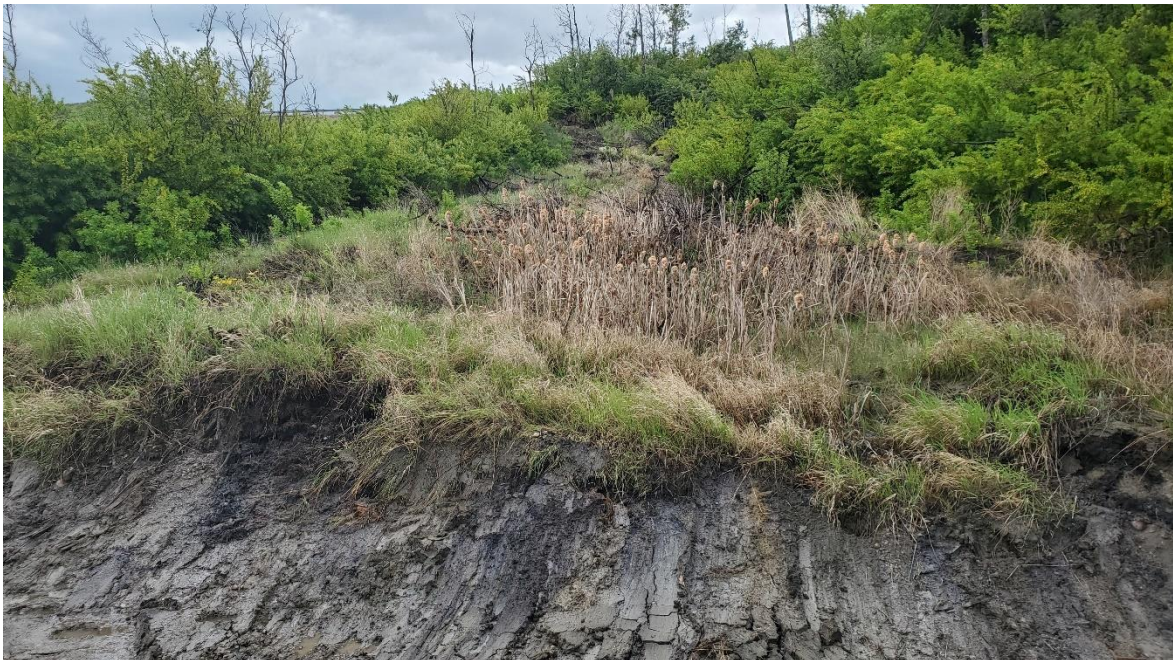
Photo 26: Looking southwest at the debris flow material immediately upslope of the CNR line. Material appears to have been recently excavated.
