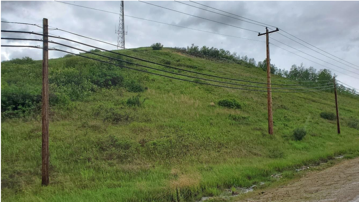
Photo 19: Looking west at shallow slide in Hwy 2 backslope below communications tower.
