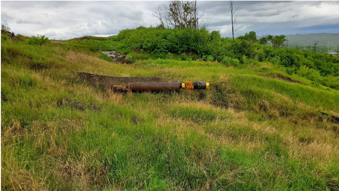
Photo 11: Looking northwest at severed and abandoned storm utility pipe. The new line was installed farther north by the Town in 2016.
