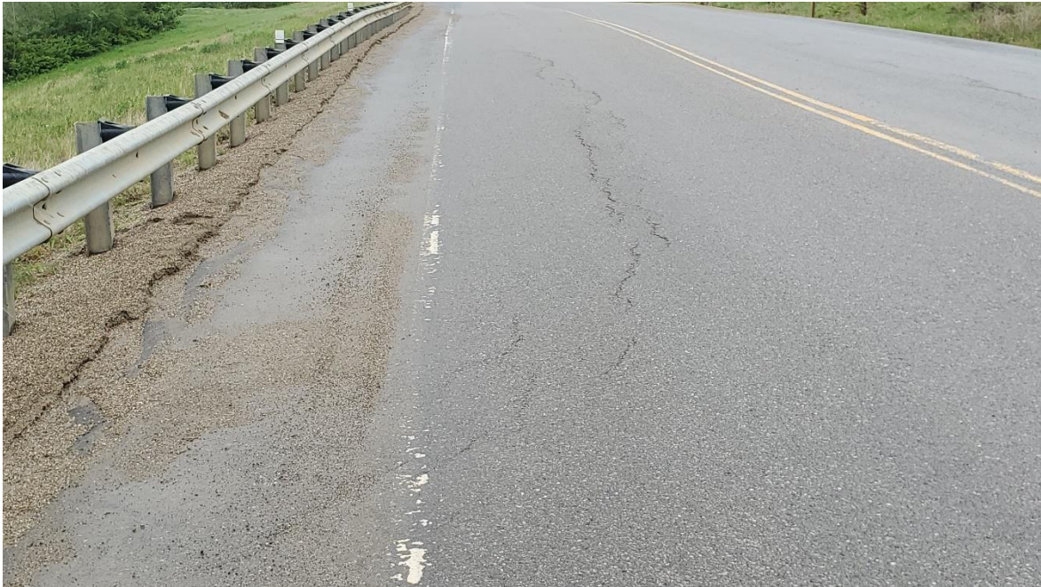
Photo 15: Cracking forming in ACP at the guardrail on the southeast side of 99 Avenue intersection. Crack is coincident with previous semi-active slide scarp. It appeared to be slightly depressed on the guardrail side of the crack.
