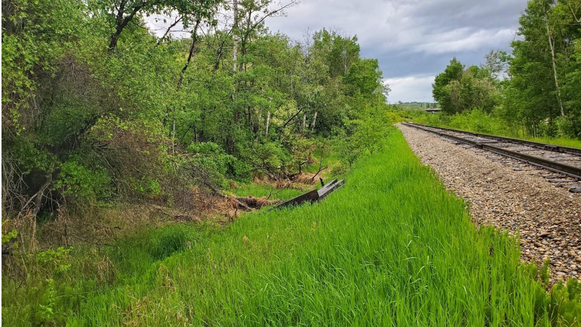
Photo 25: Looking northwest along toe bulge of the landslide below SP09-11 (Photo 23) at the west side of the CNR track.
