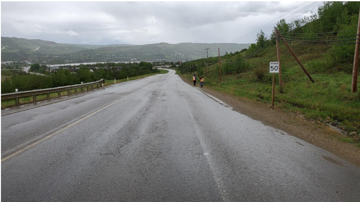
Photo 16: Looking southeast at continuation of crack from Photo 15.
