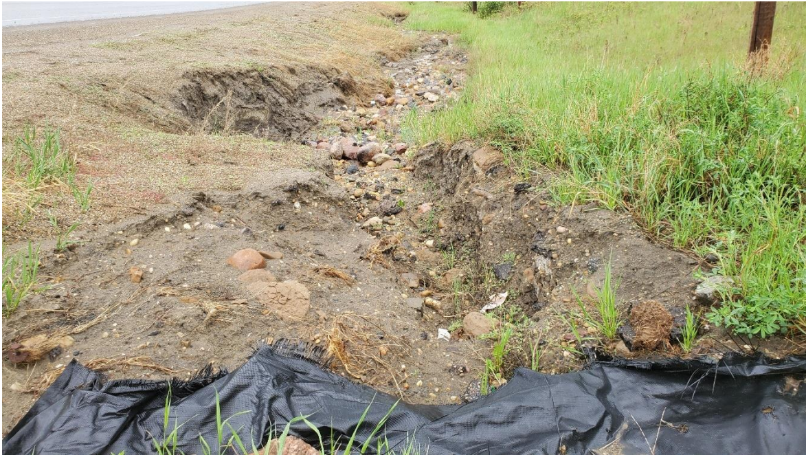
Photo 21: Looking southeast at erosion in ditch downslope inlet of 500 mm SWSP centerline culvert.
