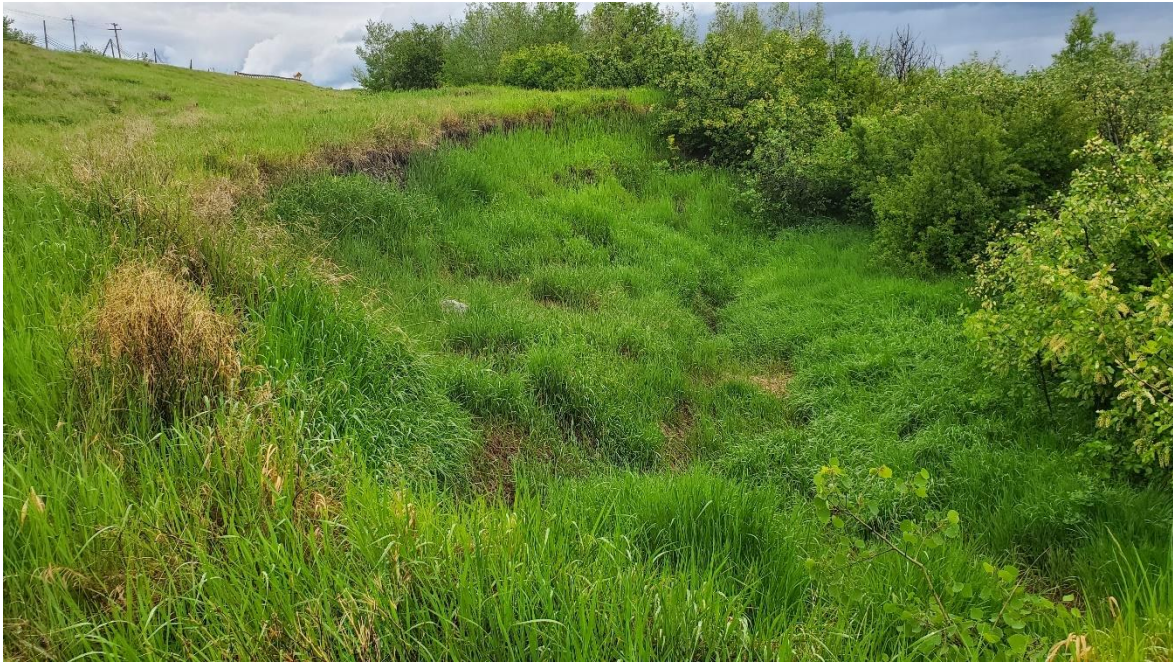
Photo 23: Looking northwest along the backscarp of the landslide downslope of the Hwy 2 off-ramp (below SP09-11).
