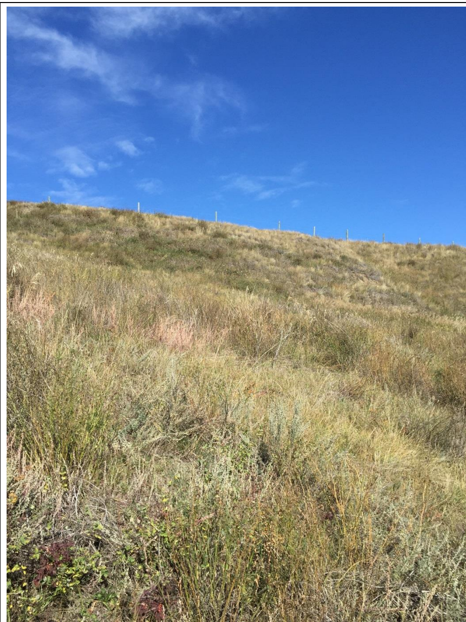
Photo 6. Looking NW upslope from the approximate center of the bulge in highway embankment sideslope below bows in guardrail and fence and the cracks in the roadway.
