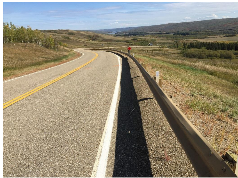
Photo 1. Looking NE from SBL shoulder towards new landslide cracks.
