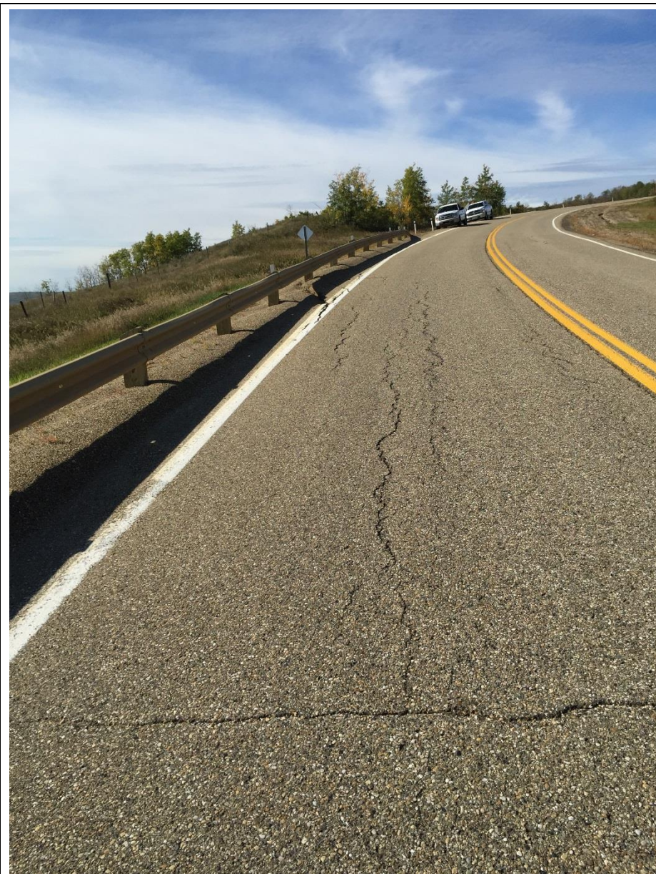
Photo 3. Looking SW at new cracks in SBL.
