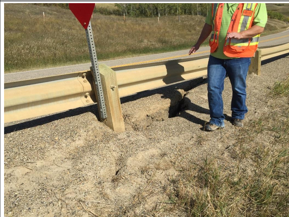
Photo 5. Looking north at cracks in SBL embankment sideslope. Cracks are open to 100 mm and drop is as much as 200 mm.
