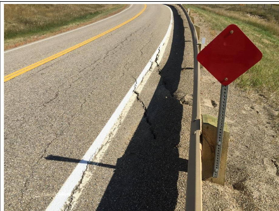
Photo 4. Looking NE at new cracks in SBL, shoulder and embankment sideslope.
