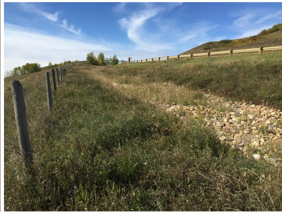
Photo 7. Looking SW along the SBL rip rap lined ditch. Bow in barbed wire fence extends 1.5 m past fence alignment. A bow in the guardrail along the SBL shoulder is also noticeable.
