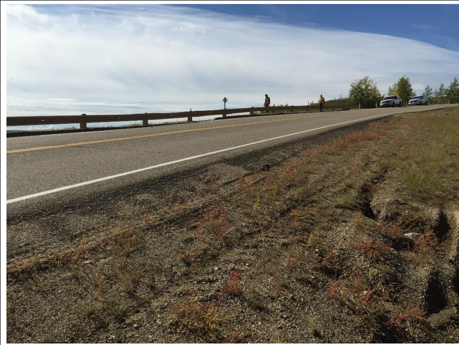
Photo 2. Looking south from NBL ditch towards new cracks. Dip in guardrail is also noticeable.
