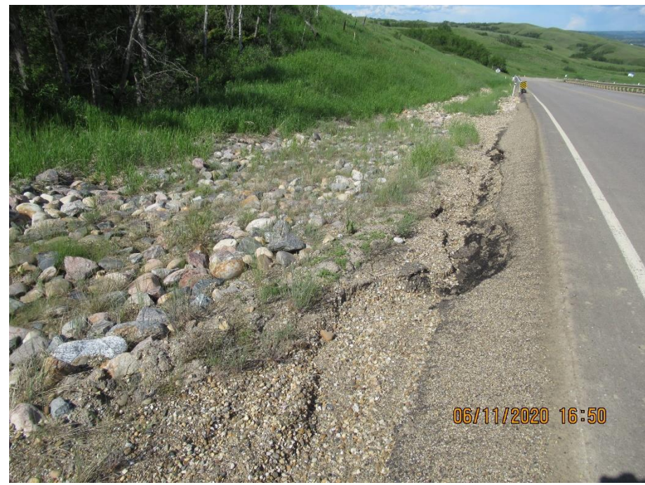
Photo 9. Erosion along the north shoulder of the highway.
