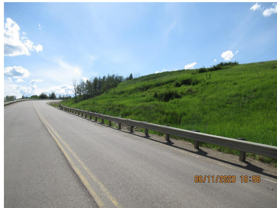
Photo 7. Looking southwest at an old grass covered slump in the backslope.
