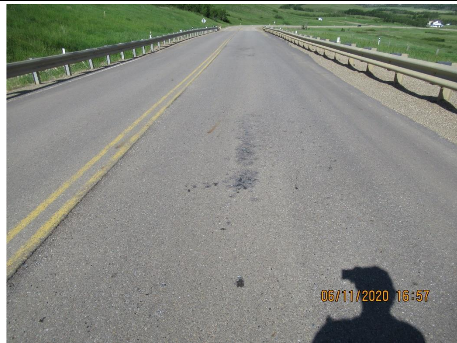
Photo 8. Seepage from the pavement.
