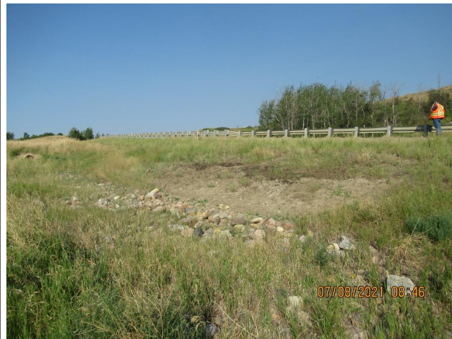
Photo 9. Wet area in fill sideslope where mower has rutted the ground surface
