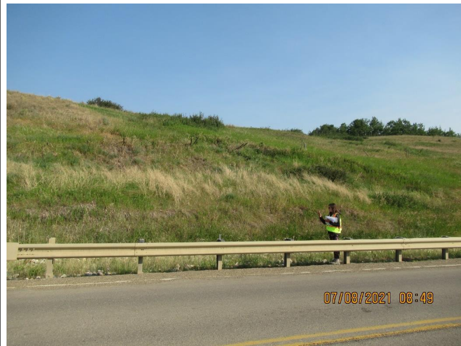
Photo 11. Grass covered backslope slumps
