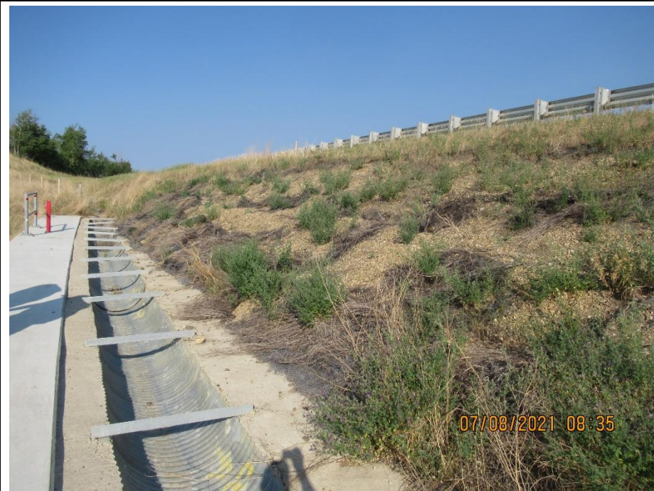
Photo 6. Looking west along the drainage trough and pile wall. Note the disturbance caused by mowers to the fill slope surface above the drain trough
