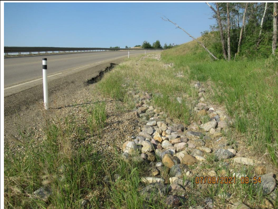
Photo 12. Looking west at eroded shoulder of road
