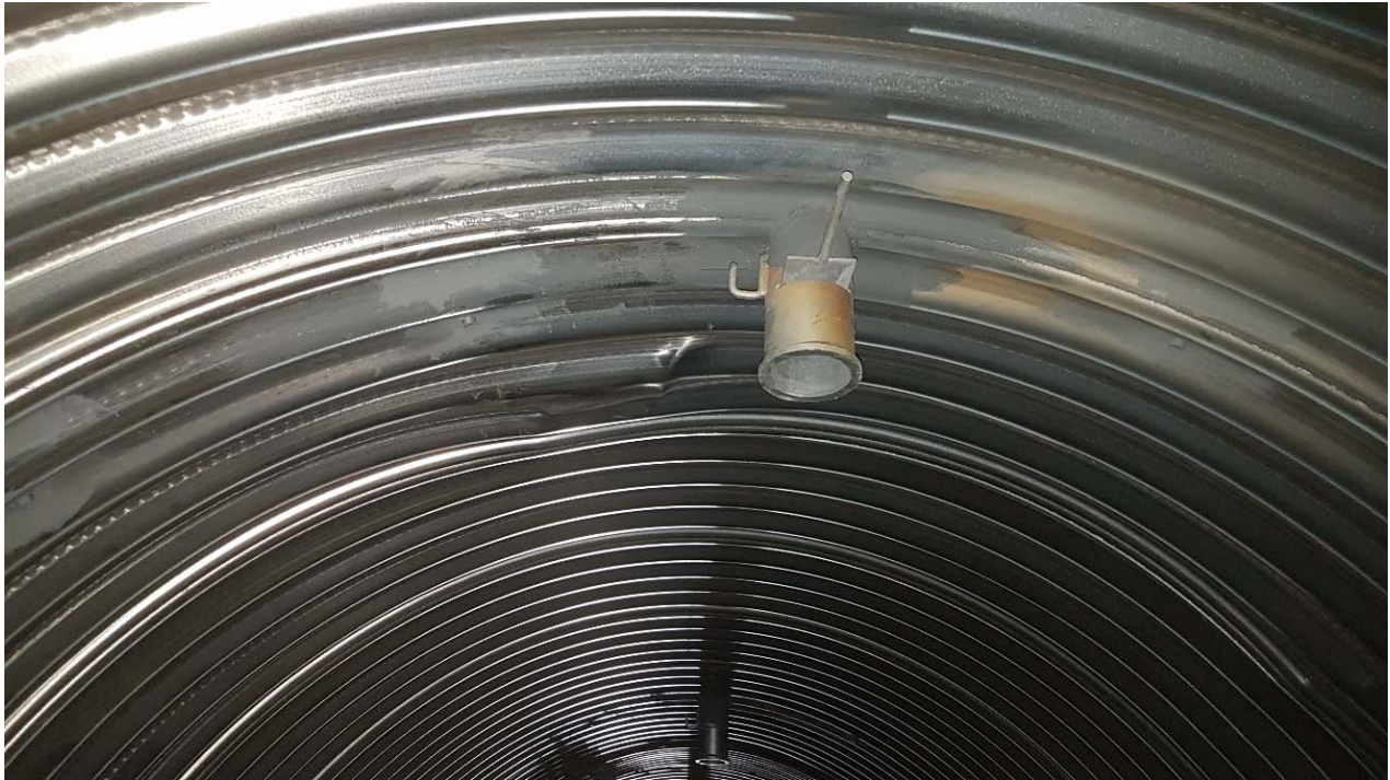
Photo 11: Deflection in roof of culvert liner approximately 30 m from the current outlet.
