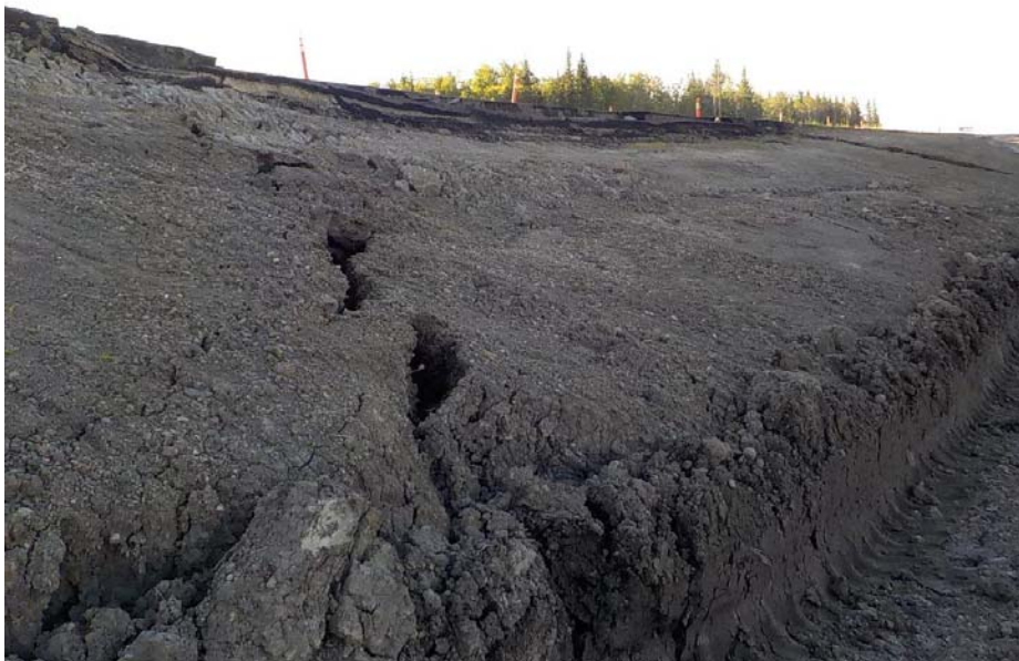
Photo 2: Looking south at north edge of cracking shortly after slide initiated (by others, Sept. 1, 2017)
