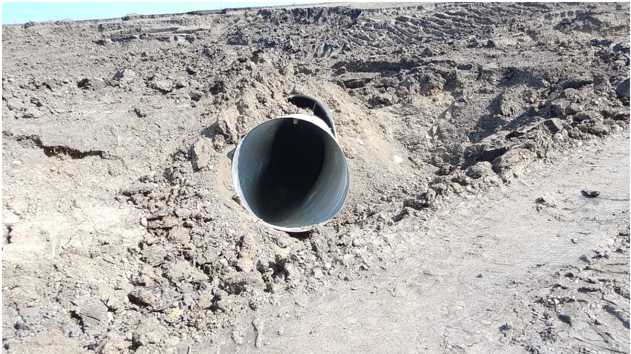
Photo 10: Looking east at deformed liner of the culvert extension.
