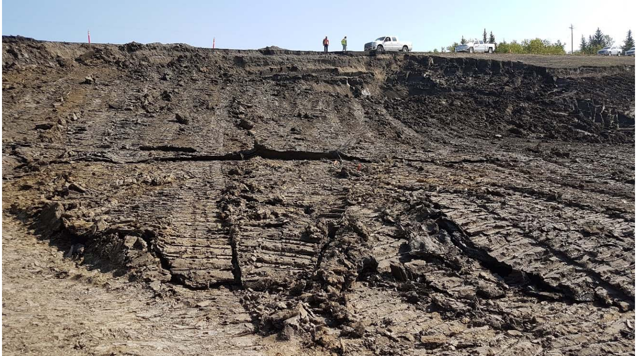
Photo 9: Looking east at toe roll material from upper portion of the slide.
