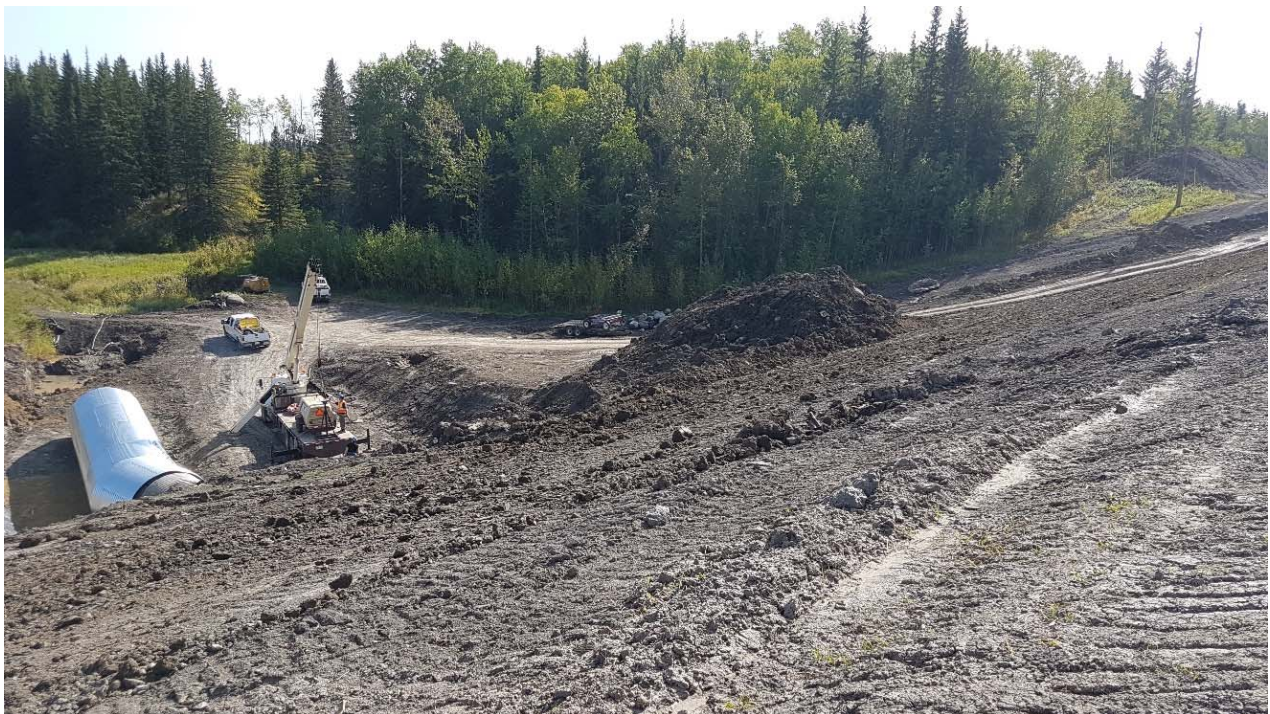
Photo 12: Looking southeast at east culvert extension. It was recommended to remove the stockpile of material located south of the excavation.
