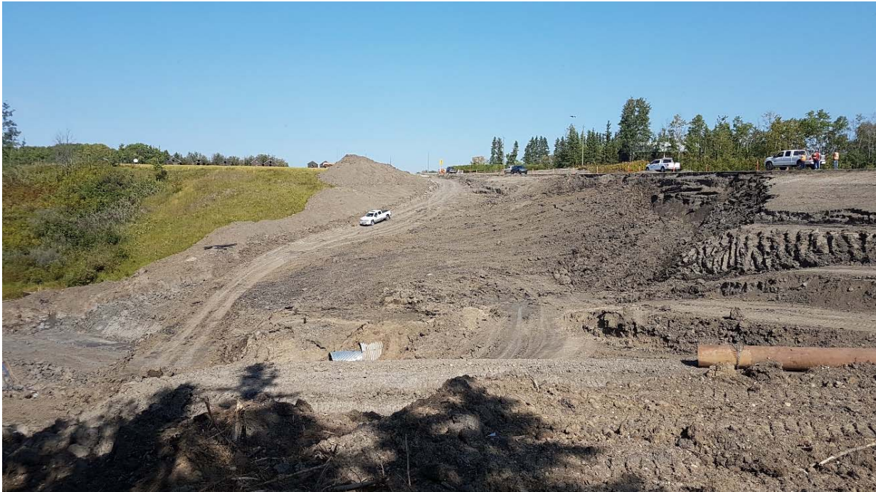
Photo 5: Looking northeast at west slide. It is recommended that topsoil stockpiles on the north slope be removed.
