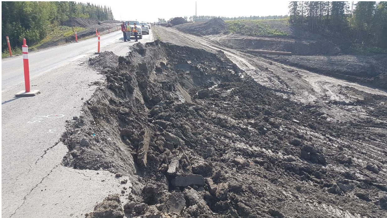
Photo 4: Looking south at west slide. Note that there has been excavation and fill placement in the slide bowl in efforts to reduce movement rates.
