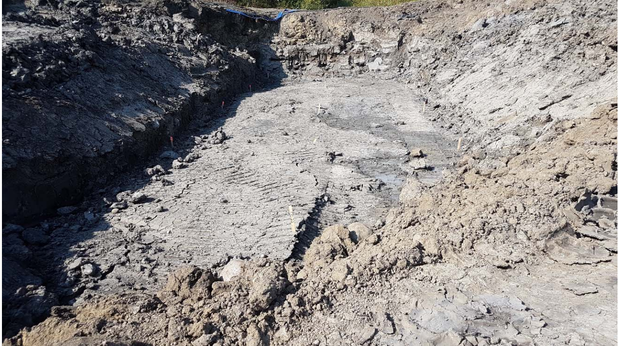
Photo 7: Looking at basal heave in west culvert extension excavation.
