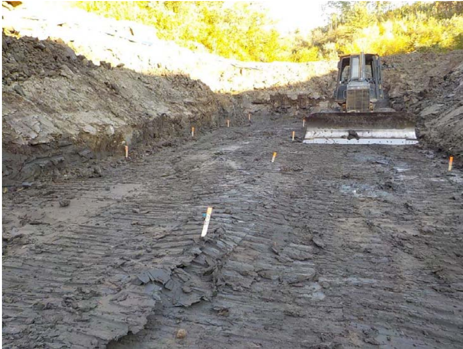
Photo 3: Start of heave in base of culvert extension excavation. Note cracks and leaning grade stake in the foreground (by others, Sept 1, 2017)
