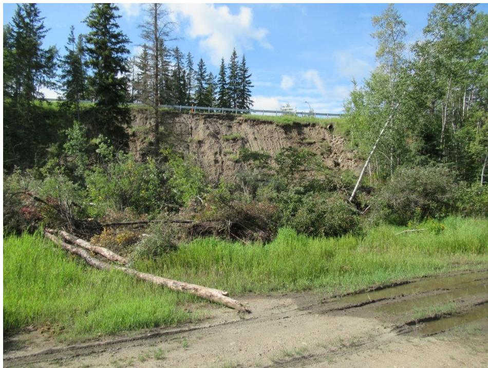
Photo 8, Looking south at the failed slope from the alley behind the mobile homes
