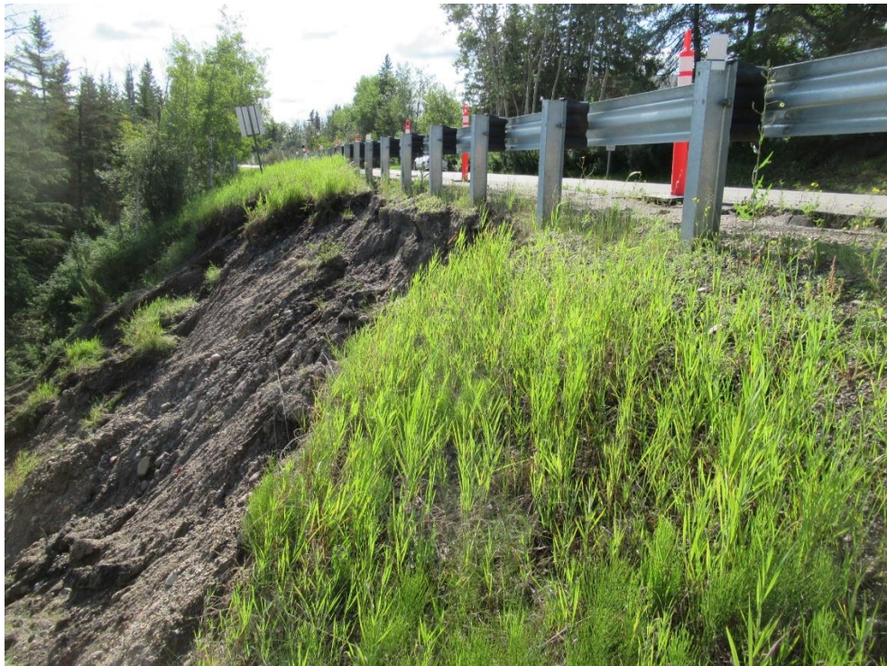
Photo 2, Backscarp of landslide is at the guardrail along Hwy. 691.
