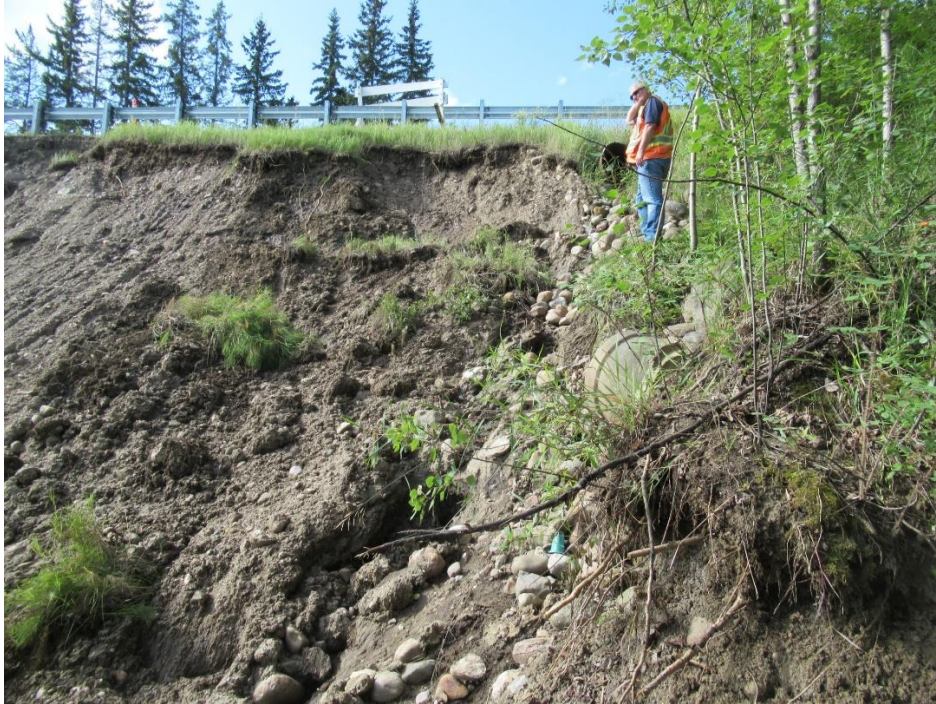
Photo 3, A 600 mm dia. C.S.P. outlets at the west flank of the slide. A 600 mm dia. Concrete pipe is located at the flank further down the slope.
