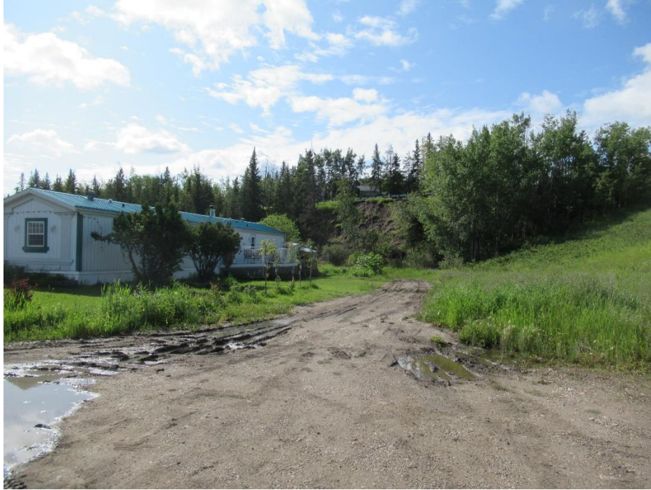
Photo 9, Looking south at the failed slope from the north end of the alley.
