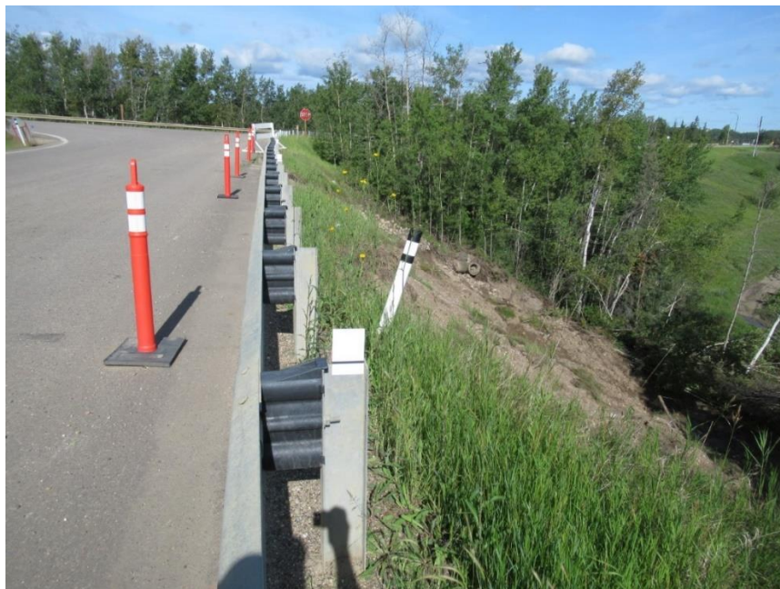
Photo 6, Looking west along Hwy. 691 at the landslide.
