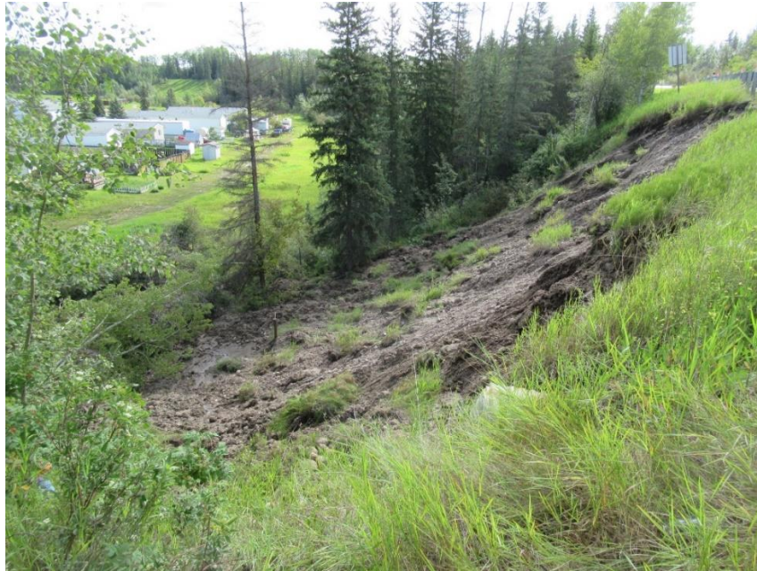
Photo 5, Looking east at the failed slope. The culvert outlet is in the forefront.
