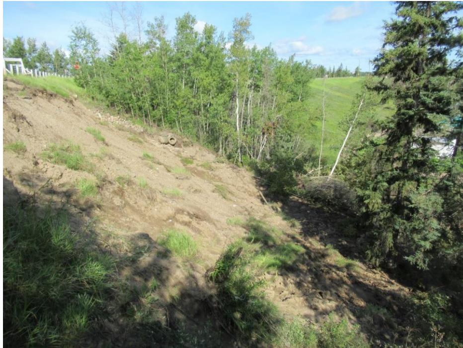
Photo 7, Looking west at the failed slope with slide mass and fallen/tilted trees at toe.
