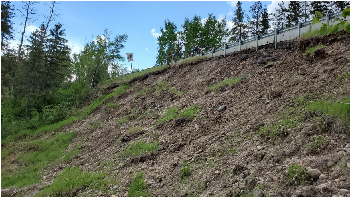
Photo 4, Exposed till in the backscarp at the slide mass. Seepage was observed in this face at the time of the callout but appeared dry in June 2020.
