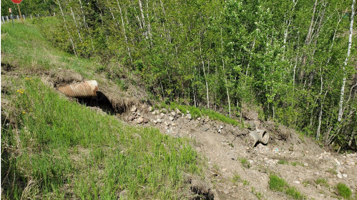
Photo 3, A 600 mm dia. C.S.P. outlets in the west flank of the slide. A 600 mm dia. concrete pipe piece is located at the flank further down the slope.
