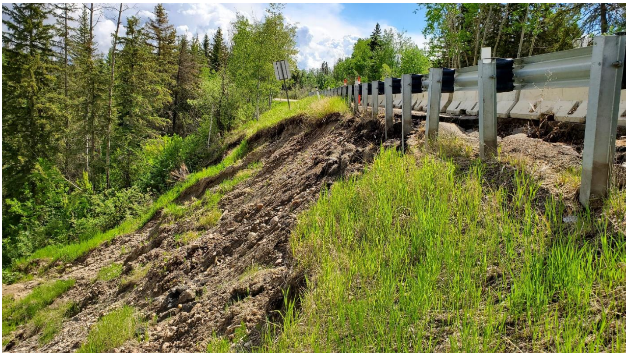
Photo 2, Backscarp of landslide is at the guardrail along Hwy. 691.
