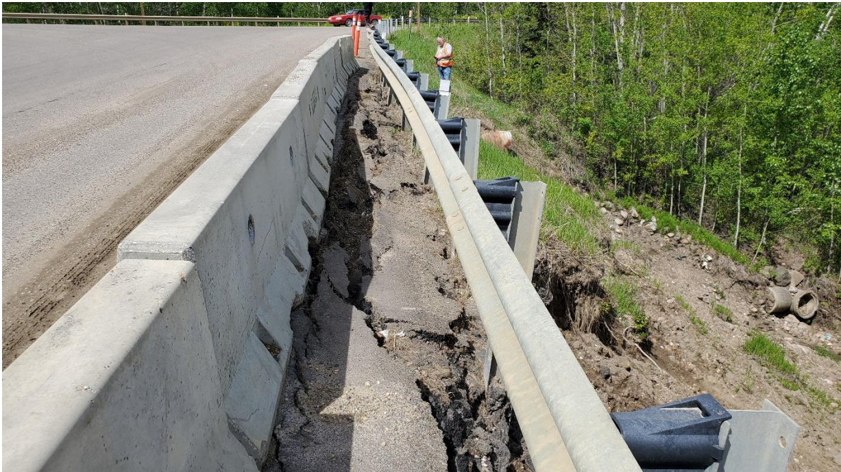
Photo 6, Looking west along Hwy. 691 at the landslide cracks in the highway surface.
