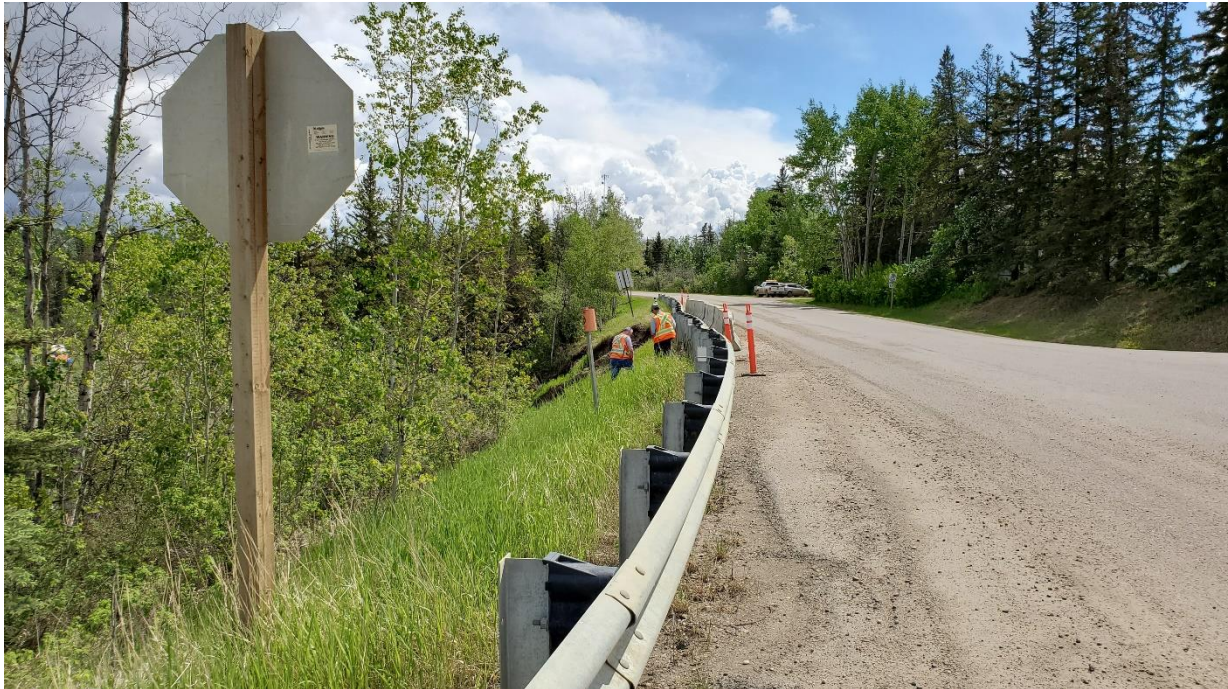
Photo 1 – Looking East along Hwy. 691 toward the landslide.
