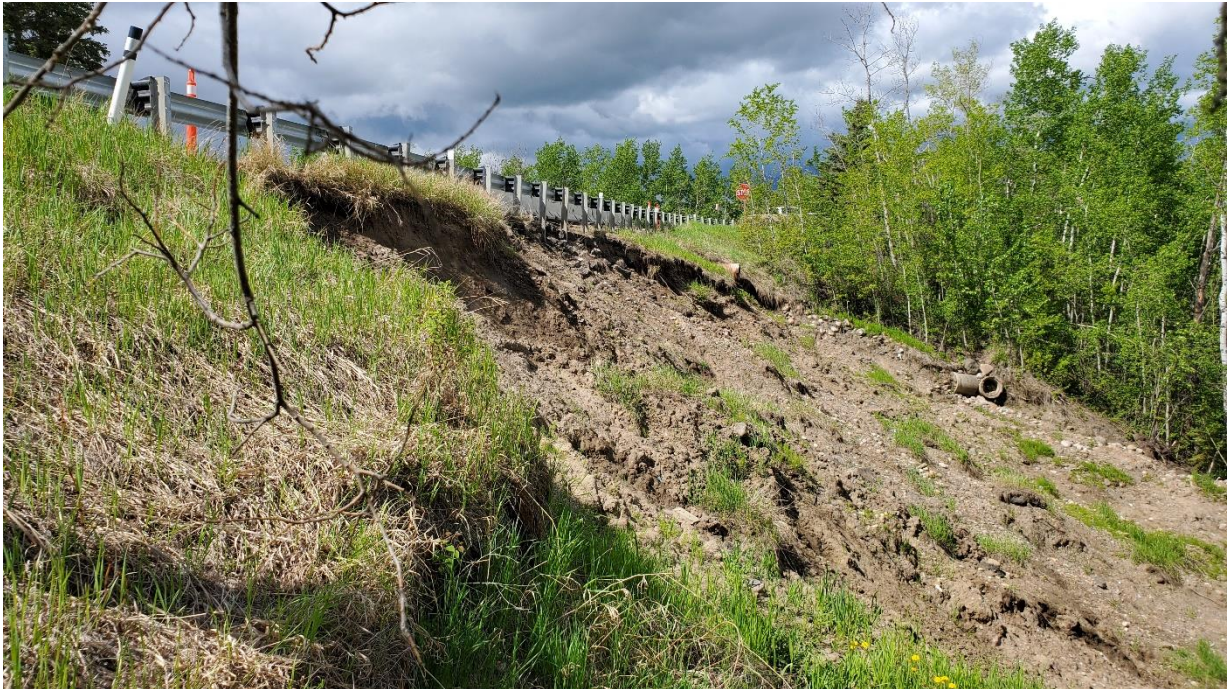
Photo 7, Looking west at the failed slope with slide mass and fallen/tilted trees at toe.
