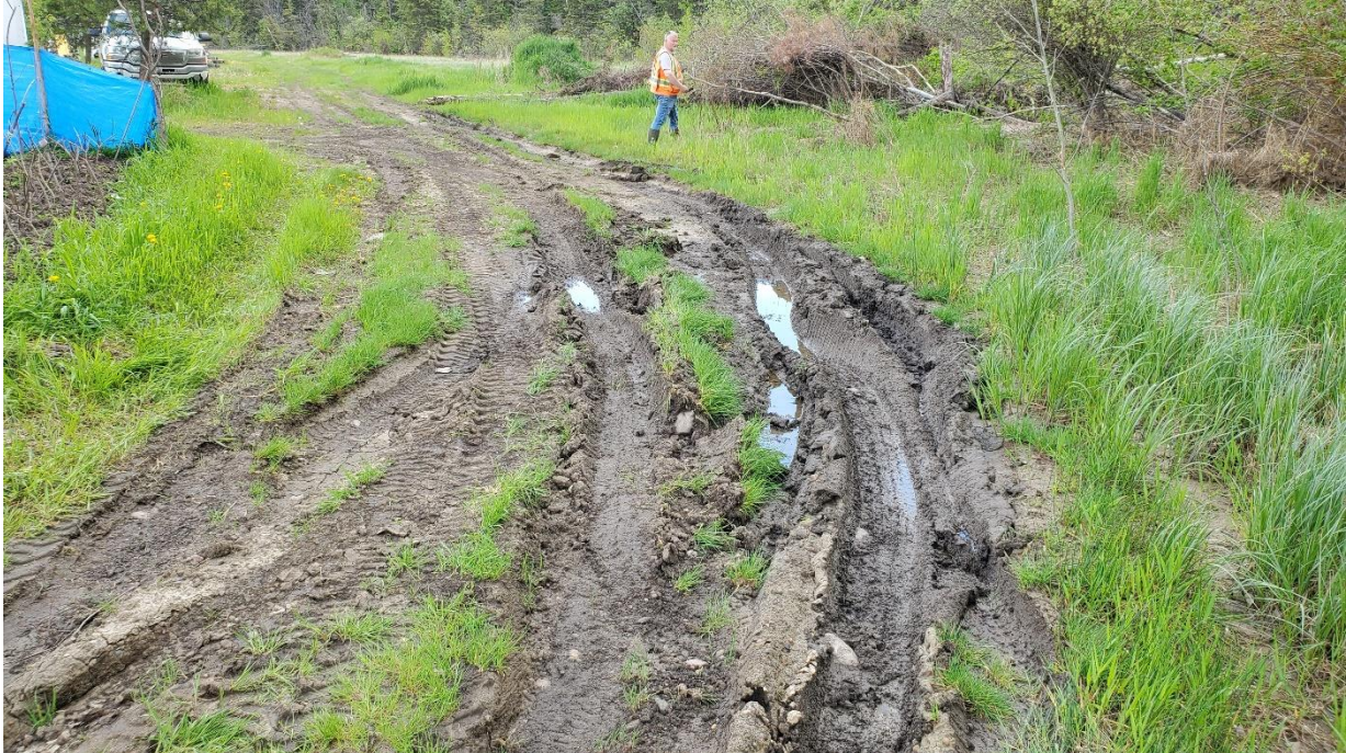
Photo 9, Looking east at wet and soft ground of alley at toe of slide.
