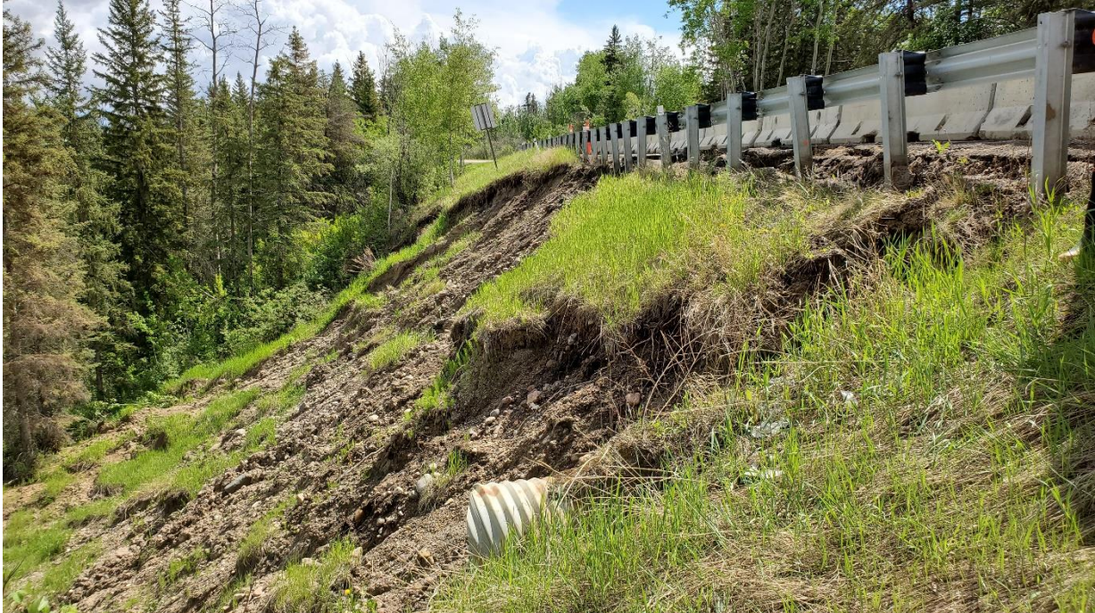
Photo 5, Looking east at the failed slope. The culvert outlet is in the forefront.
