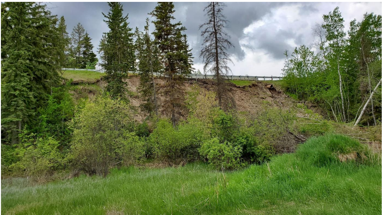
Photo 8, Looking south at the failed slope from the alley behind the mobile homes
