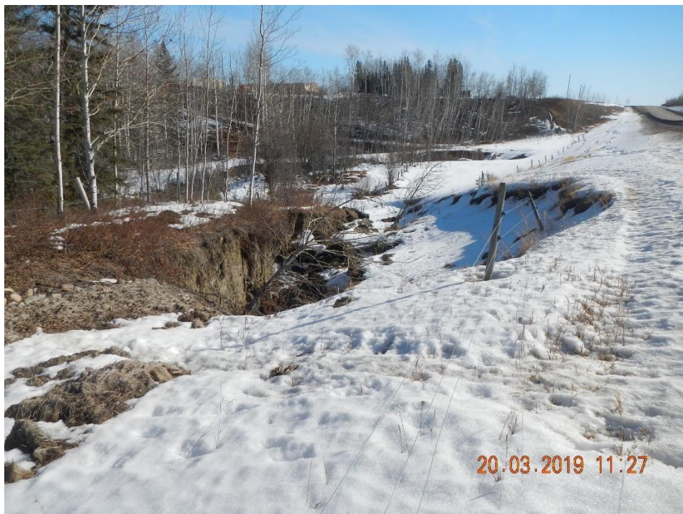
Photo 6 (MCI, March 20, 2019) – Looking east at widening erosion gully.
