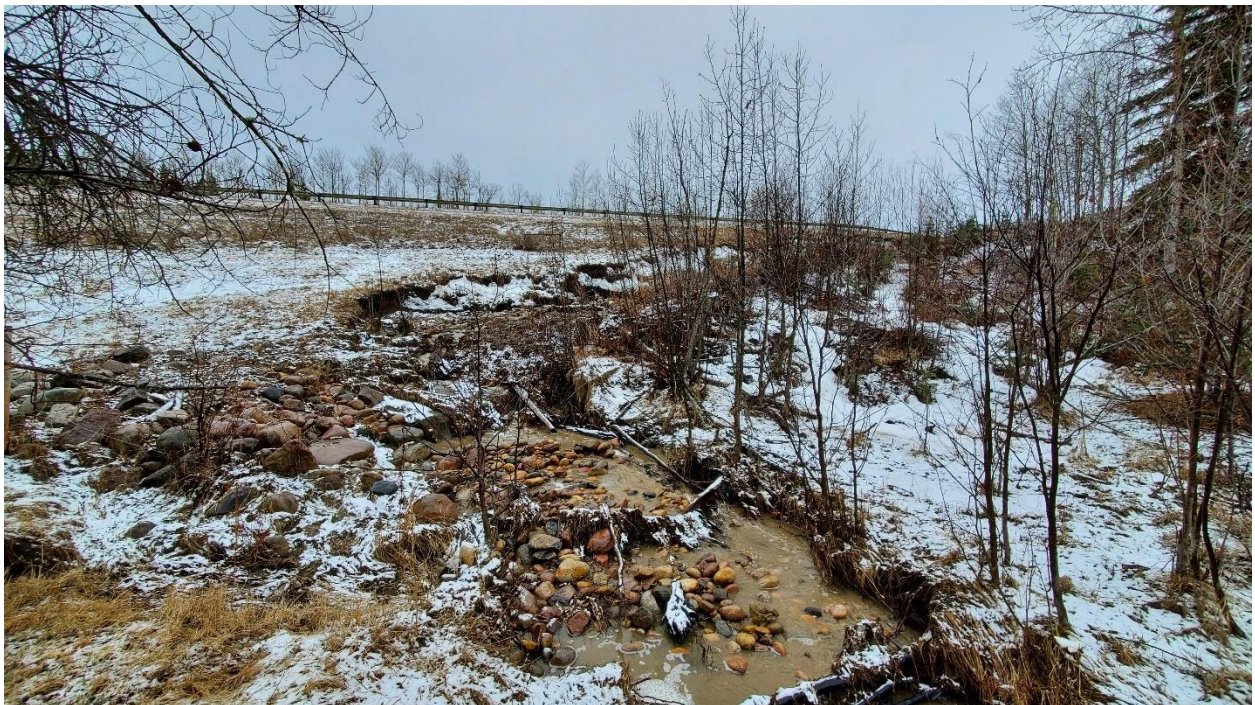
Photo 16 (April 28, 2022) – Looking south downstream of the bend in the erosion gully.
