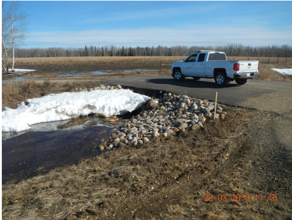
Photo 5 (MCI, March 28, 2019) – Approach culvert inlet under high flow. Approach was paved.
