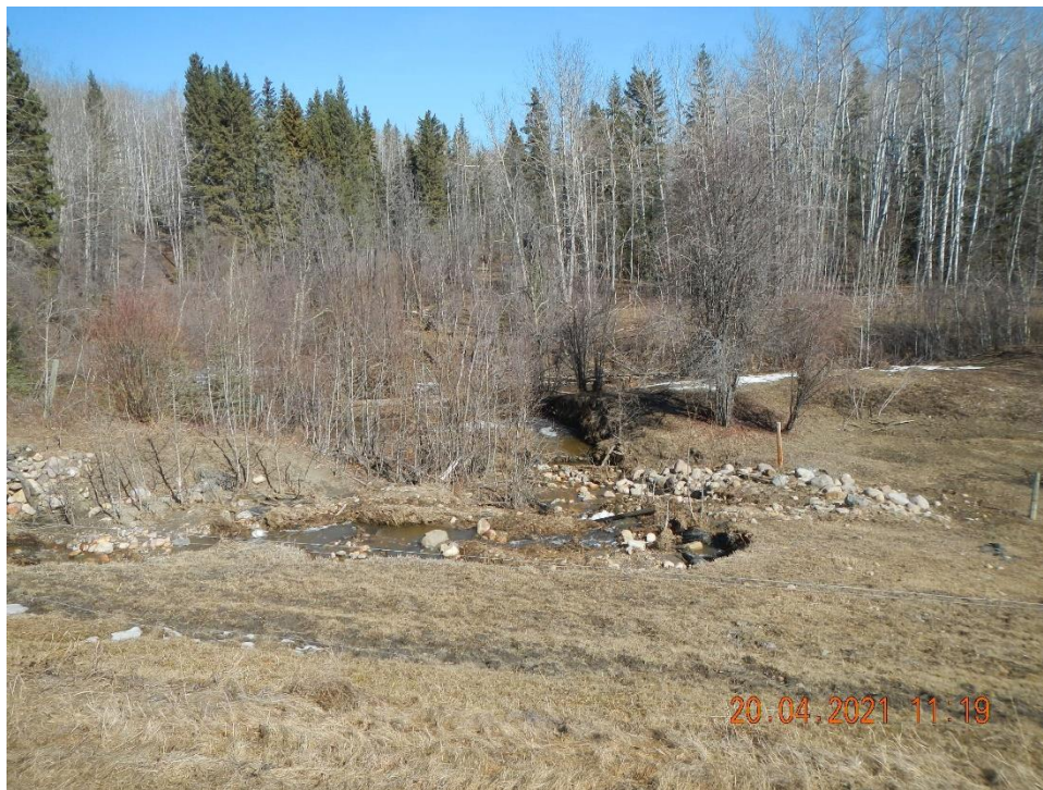
Photo 10 (MCI, April 20, 2021) – Looking north where the ditch discharges to Gravina Creek. A slump has formed at the bend.
