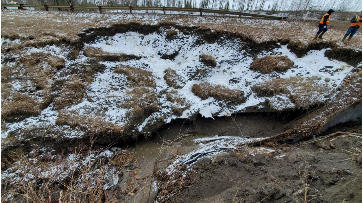
Photo 15 (April 28, 2022) – Looking south at the main slump in the highway embankment.
