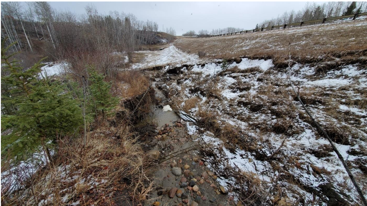
Photo 18 (April 28, 2022) – Looking east along the erosion gully at the east flank of the embankment slump and the undercut north side.
