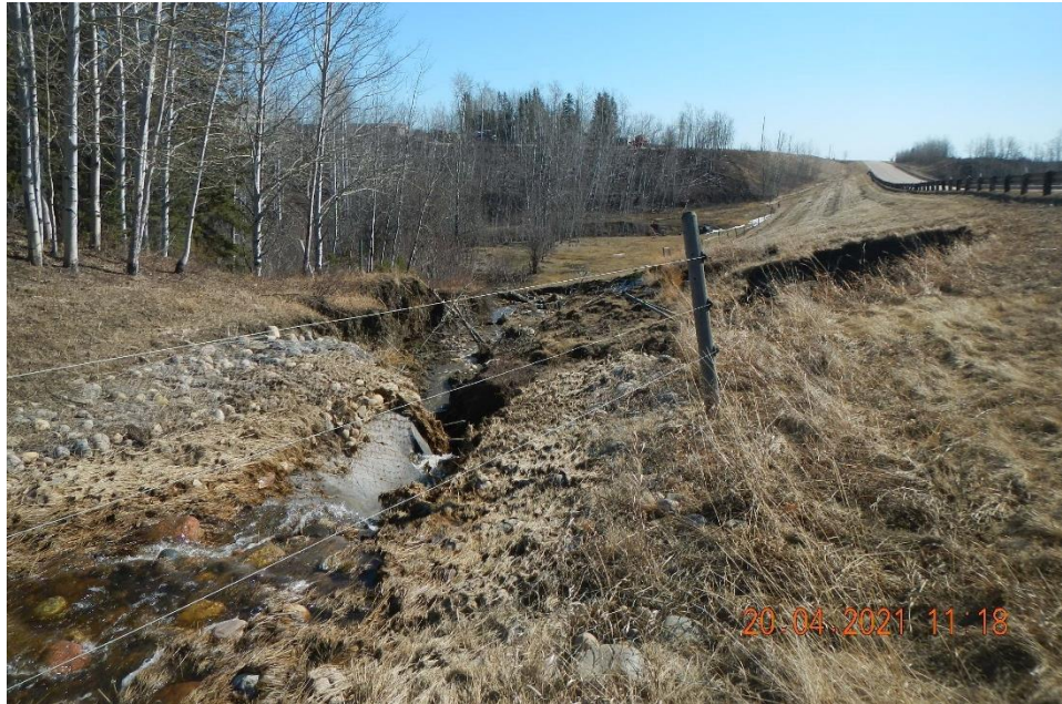
Photo 9 (MCI, April 20, 2021) – Looking east at the erosion gully which has slumped toward the road.
