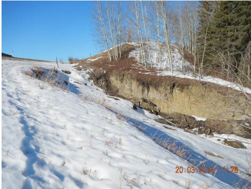
Photo 7 (MCI, March 20, 2019) – Looking west at growing erosion gully.
