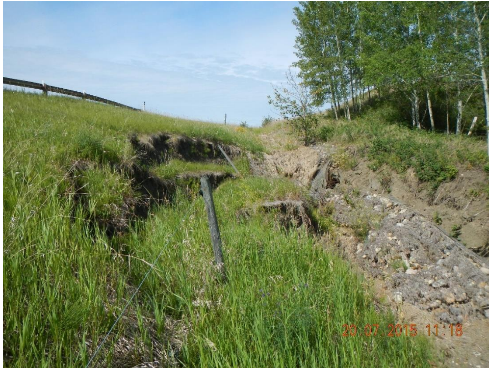
Photo 1 (MCI, July 20, 2015) – Looking west at erosion gully forming.
