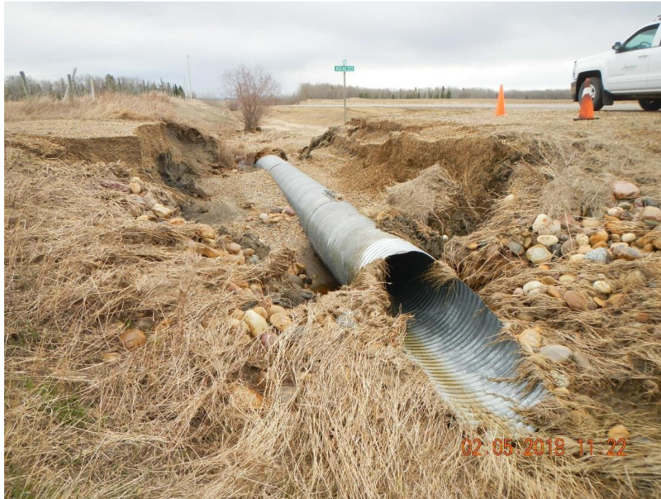
Photo 3 (MCI, May 2, 2018) – Looking east at the approach culvert wash-out.
