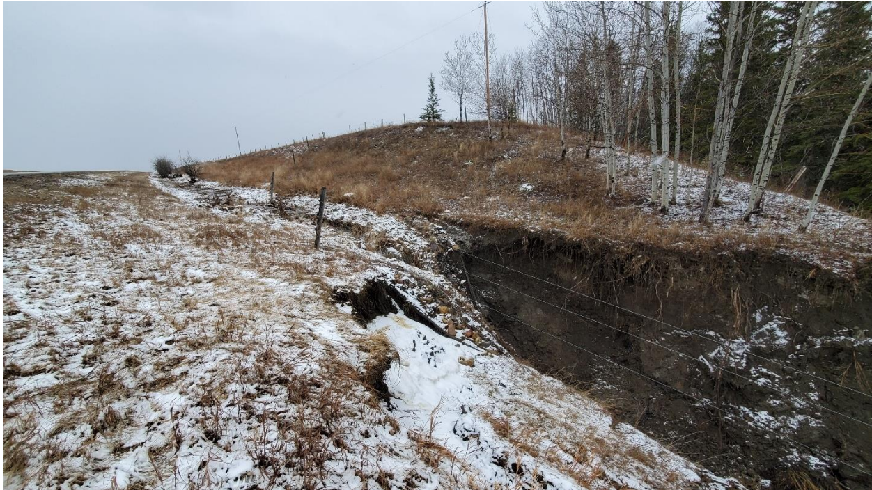
Photo 13 (April 28, 2022) – Looking west at the nick point of the gully.
