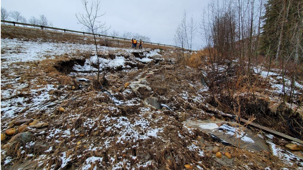
Photo 17 (April 28, 2022) – Looking west at the end of the erosion gully. Pieces of gabion basket are visible.
