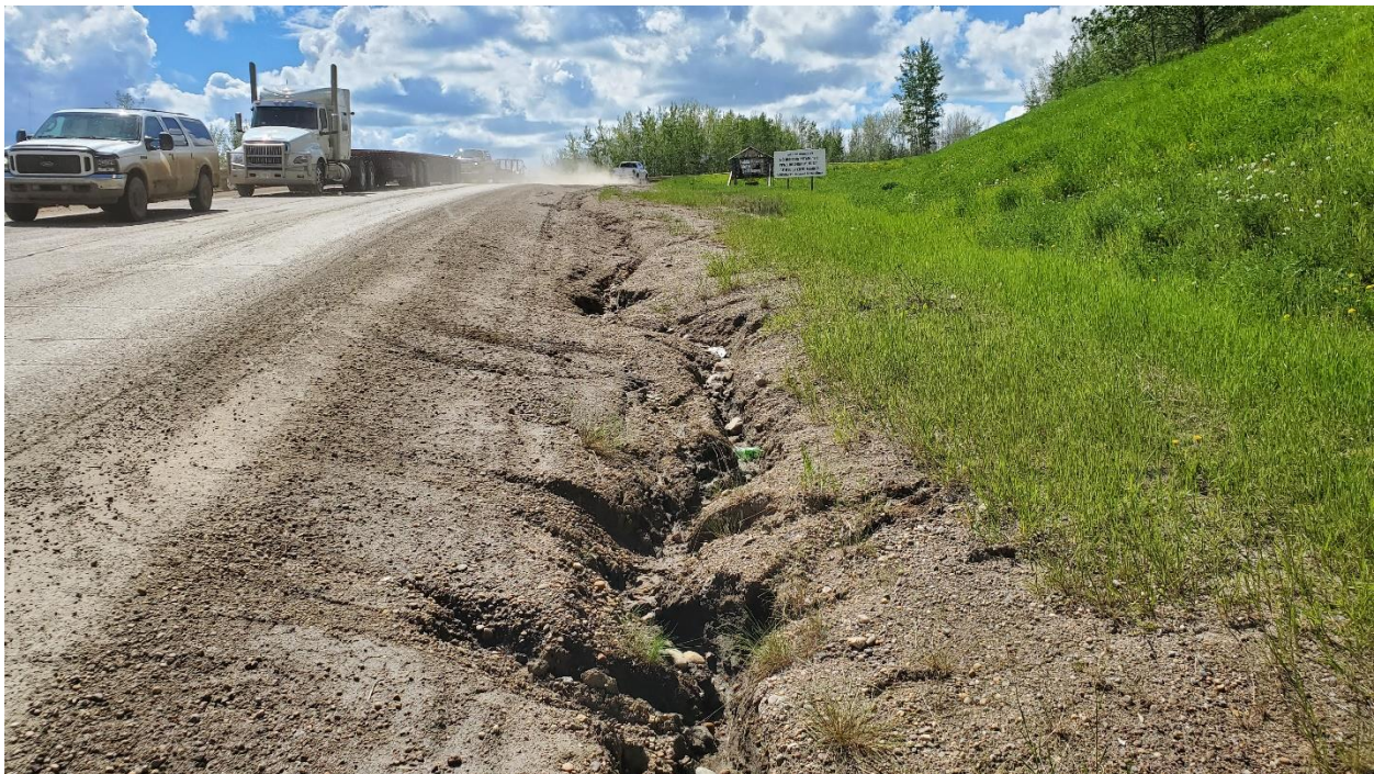
Photo 8 – Looking west at ditch erosion near bottom of valley.
