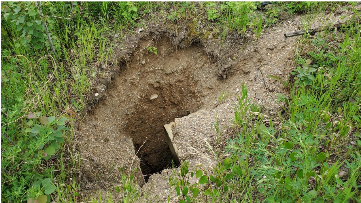
Photo 6 – Sinkhole at separated 800 mm CSP downpipe south of the highway.
