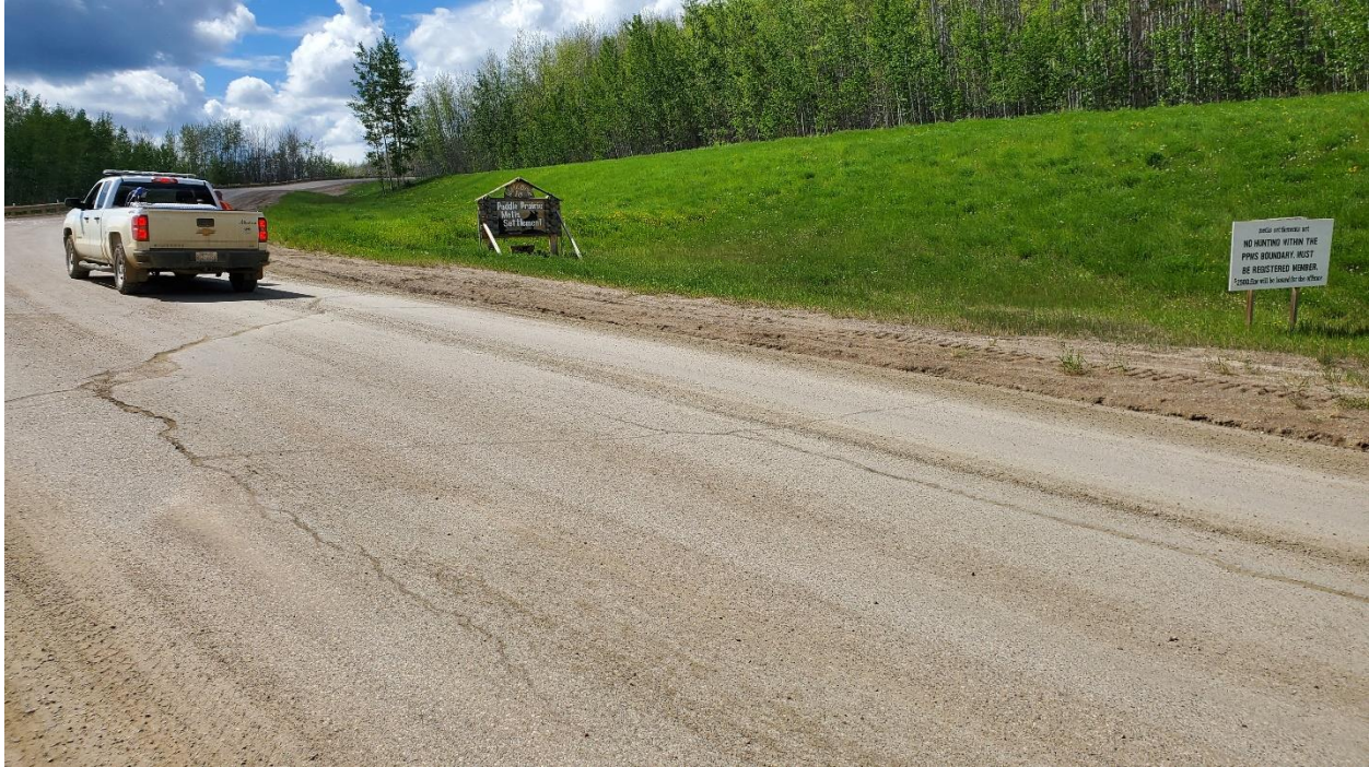
Photo 9 – Cracks on highway near bottom of valley.
