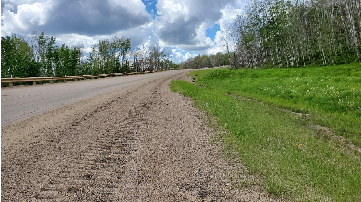
Photo 3 – Looking southwest at erosion in north ditch.
