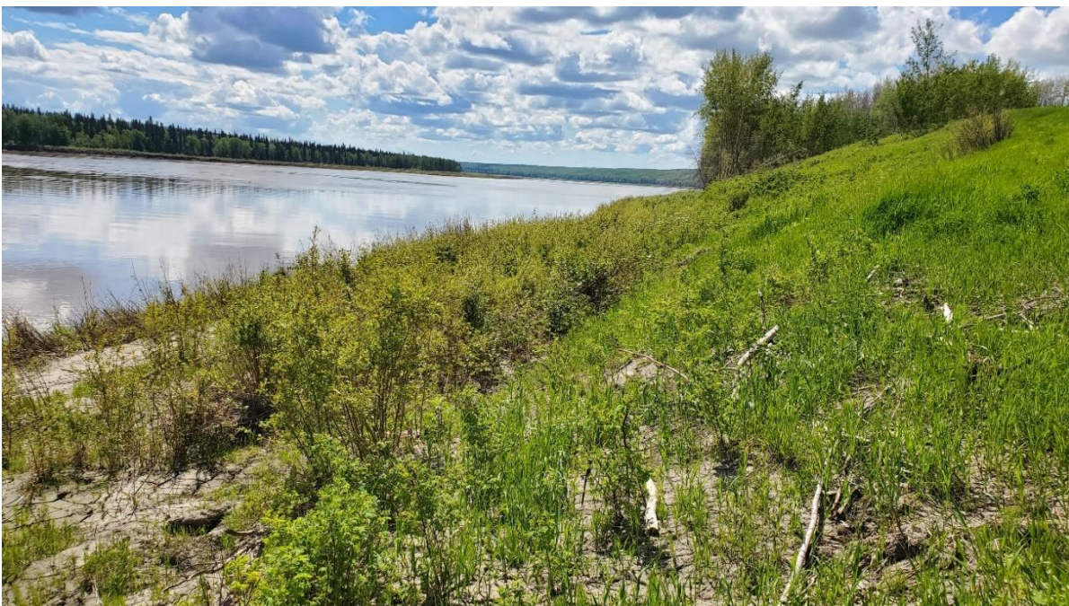
Photo 2 – Looking south at slope with ongoing movement in the northeast portion of the site. Note that much of the vegetation along the river bank was destroyed by flooding in Spring 2018 and covered again with silt and debris in Spring 2020 (higher water level than 2018).
