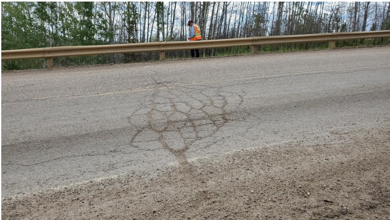
Photo 4 – Alligator cracking near the southwest end of the site.
