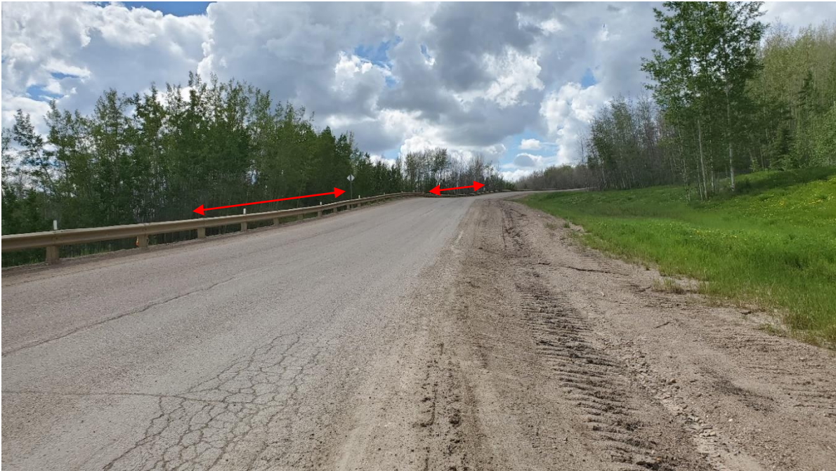
Photo 1 – Looking southwest at one of the dips in the road and deteriorating asphalt surface. A second dip is visible further up the road.
