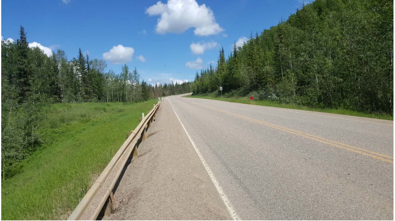
Photo 1 – Looking northeast at hump in the highway.
