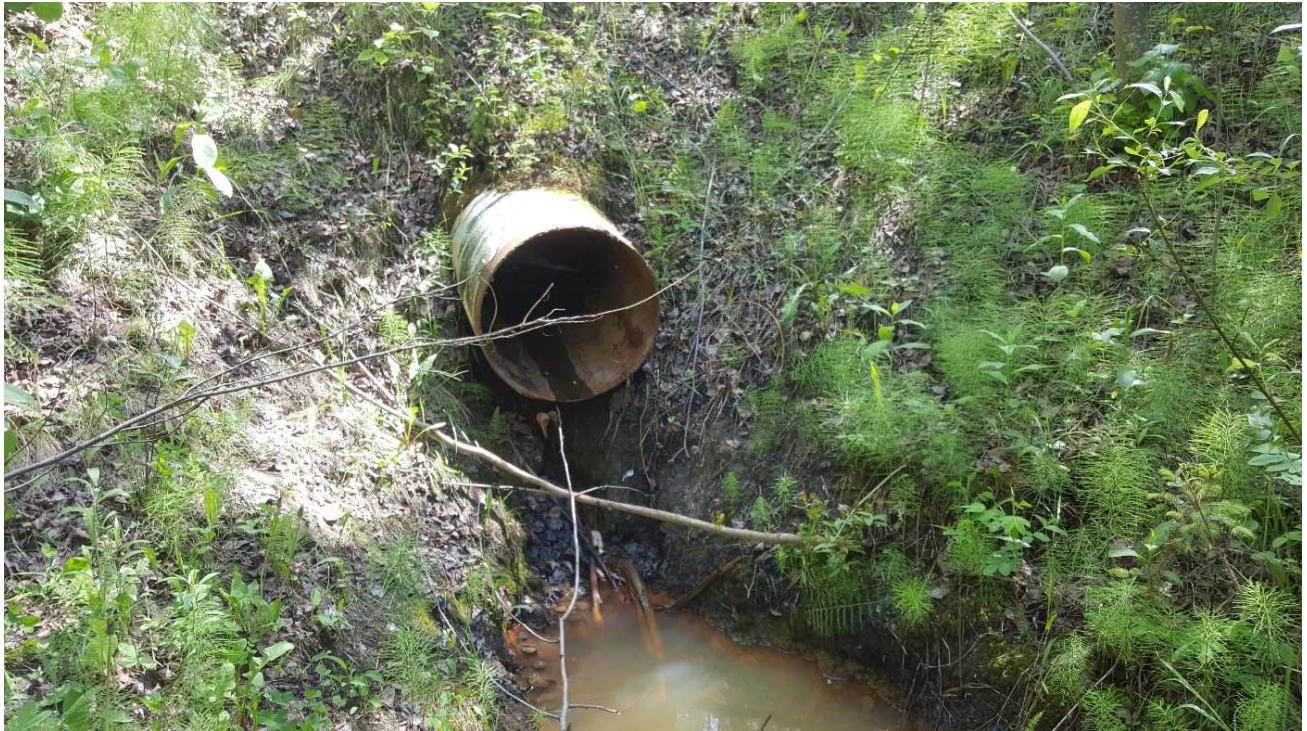
Photo 6 – Hanging culvert outlet.
